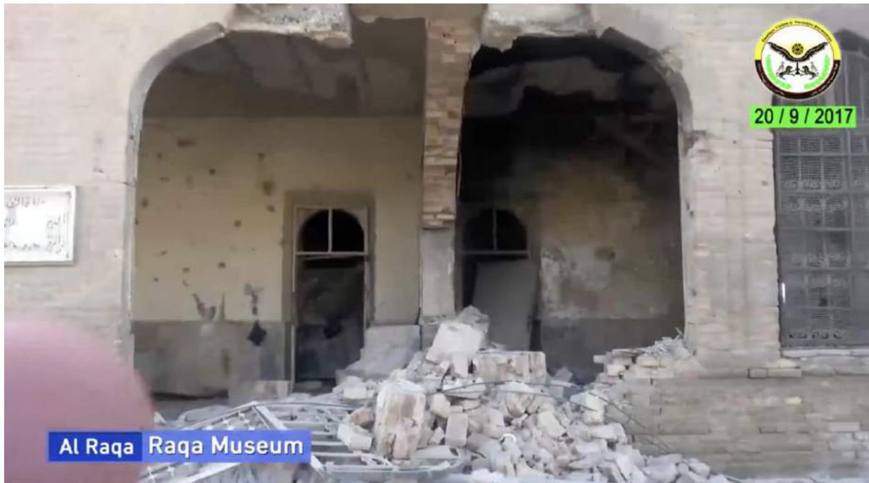
Video still of the hole in the eastern facade (ATPA; September 28, 2017)
