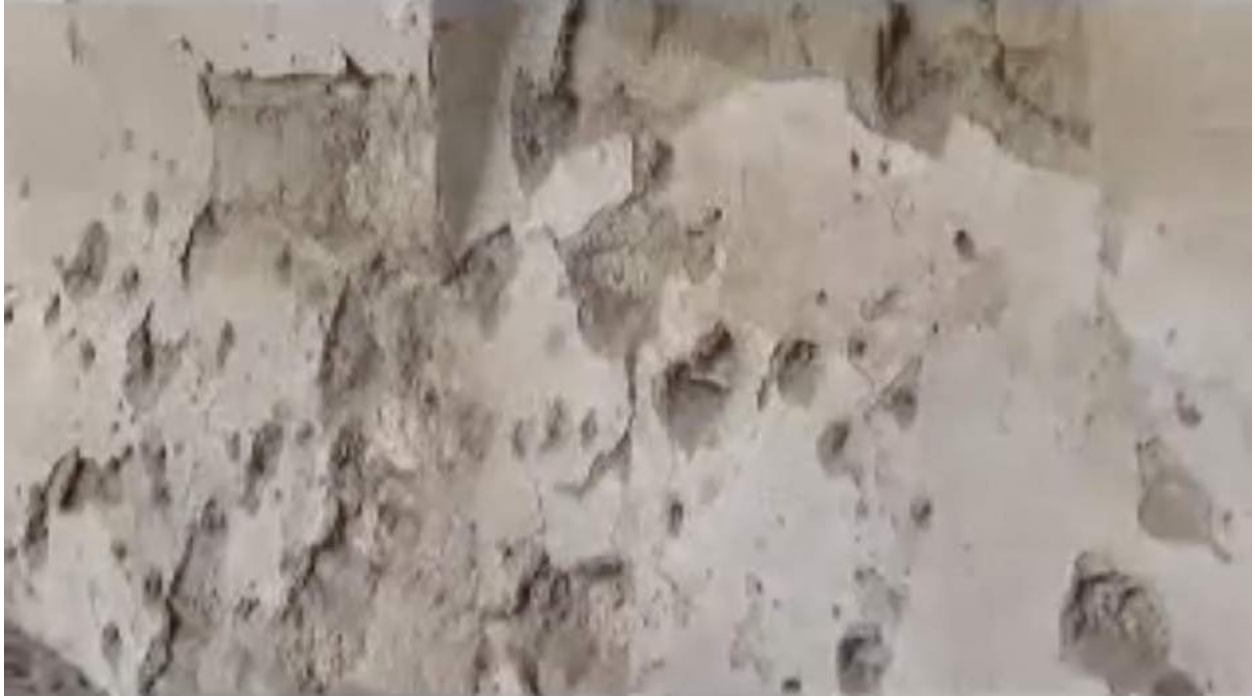
Video still of damage to a wall alongside the mosque's courtyard (Sarmin Coordination; September 1, 2012)
