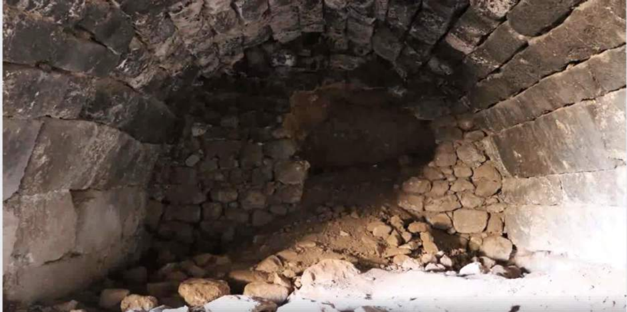
Damage to Byzantine structure near Tell Danit (Society for the Rescue of Archaeological Sites in Northern Syria/Facebook; September 15, 2017)
