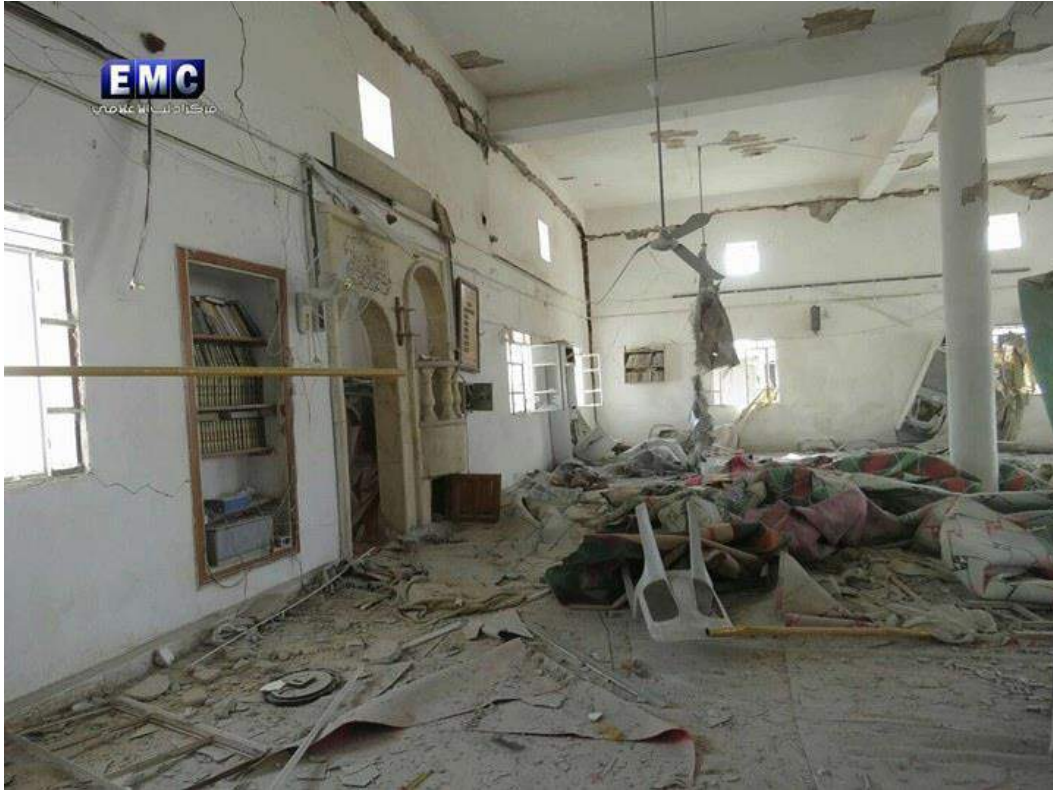
Damage to the interior of Abu Bakr al-Siddiq Mosque. Note the large cracks along the corners and tops of the walls that were caused by the force of the explosion (SNHR; September 20, 2017)
