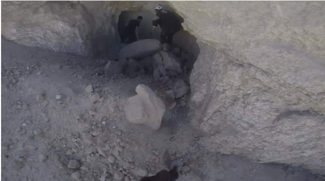
Video still of damage to a contemporary subterranean structure at Ebla (SCD-IG; September 23, 2017)
