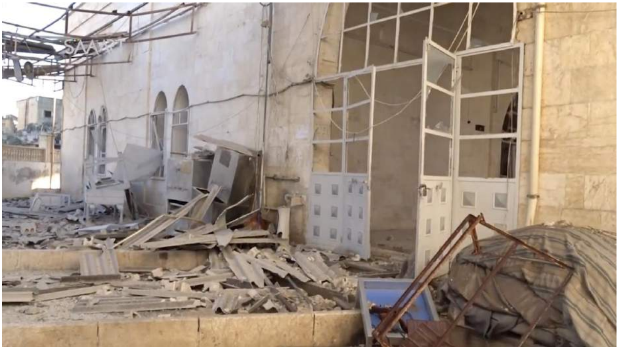
Video still of damage to the mosque's exterior (SMART News Agency; September 28, 2017)
