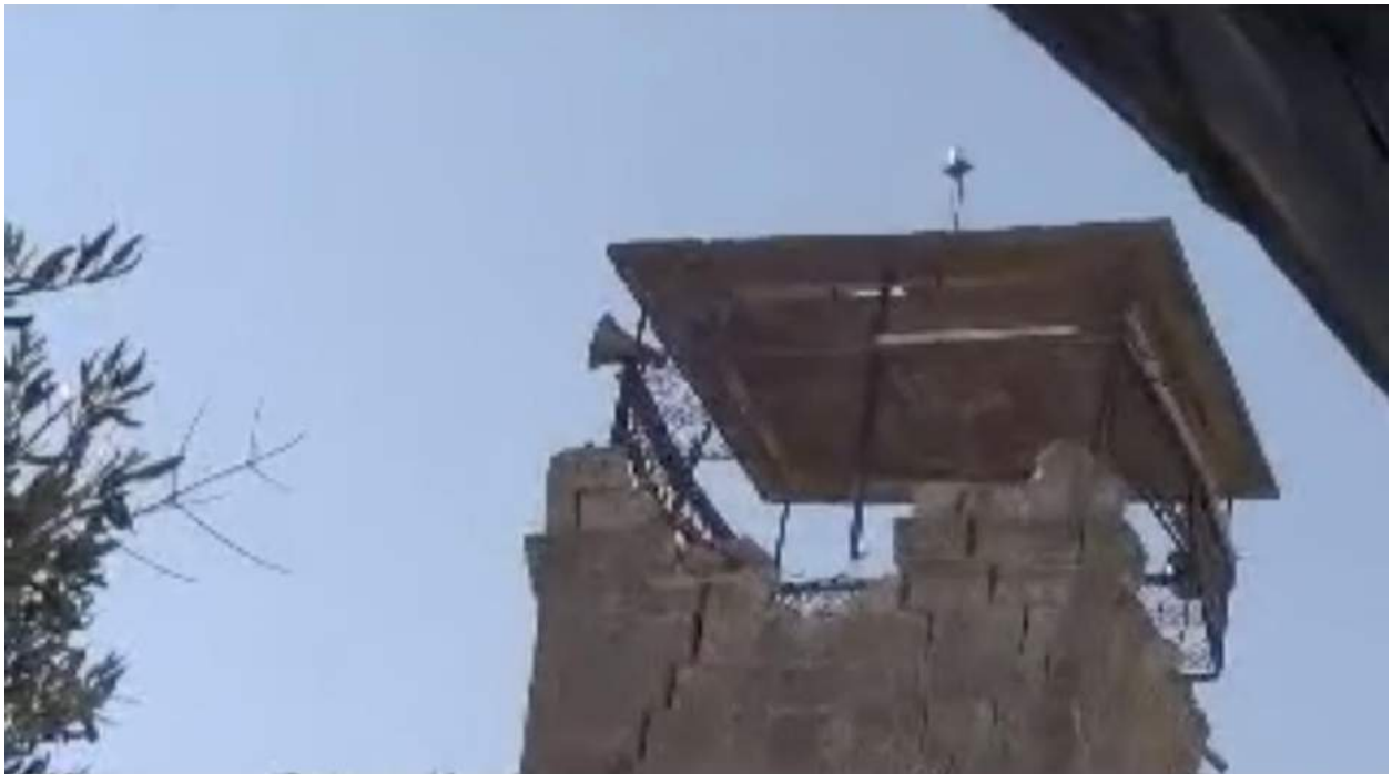
Video still of damage to the mosque's minaret (Sarmin Coordination; September 1, 2012)
