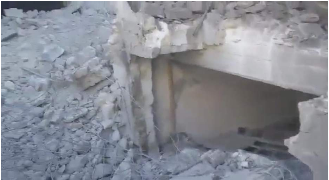
Video still of damage to the mosque, seen from the outside (SNHR; September 29, 2017)
