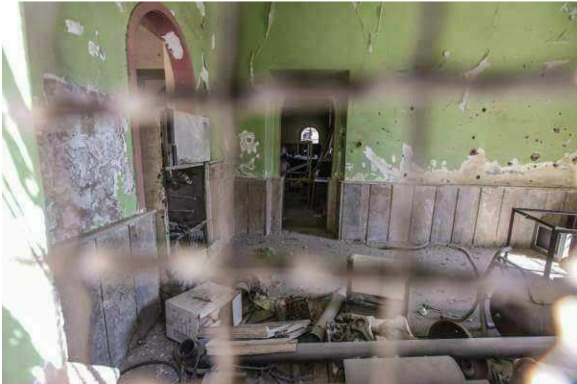
Damage to the interior of the museum (RBSS; September 15, 2017)
