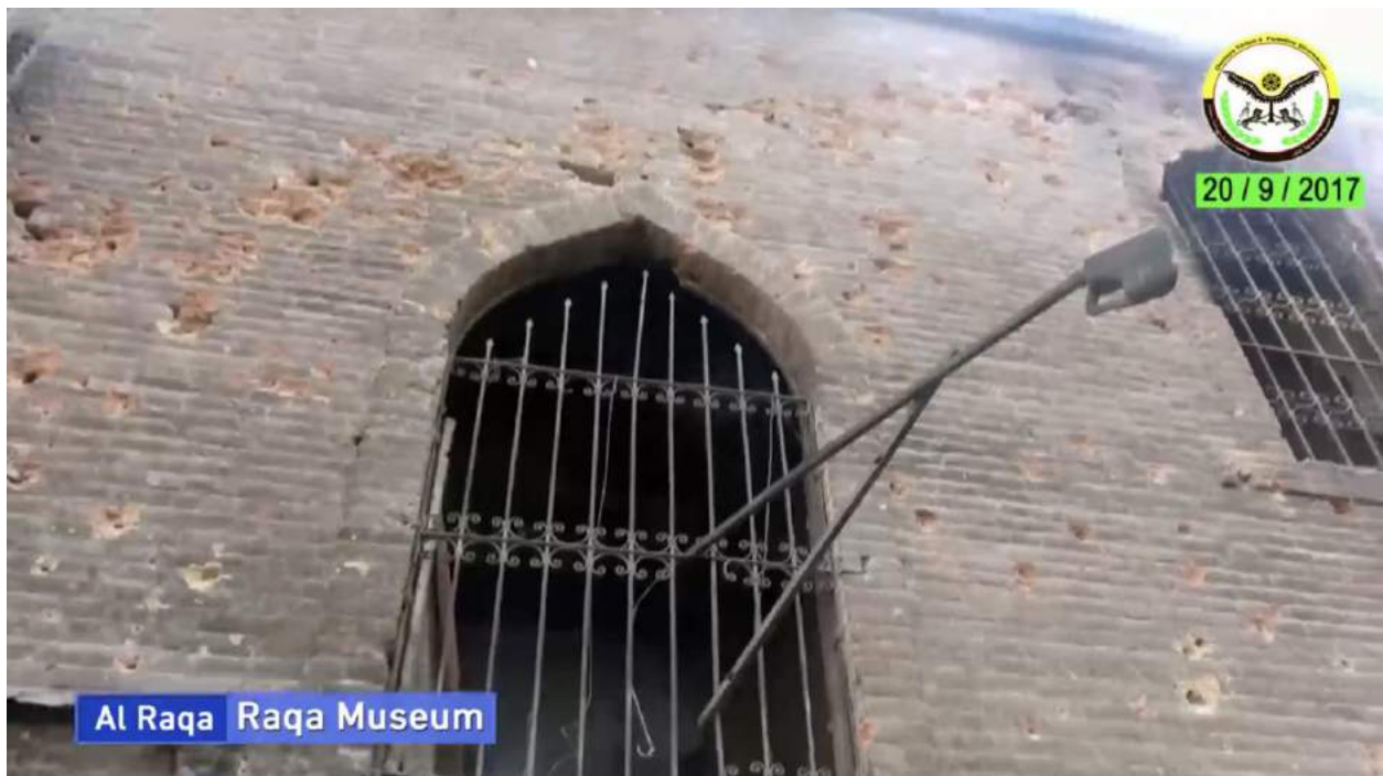
Video still of damage to the northern facade (ATPA; September 28, 2017)
