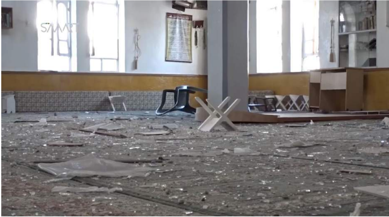
Video still of damage to the mosque's interior (SMART News Agency; September 28, 2017)
