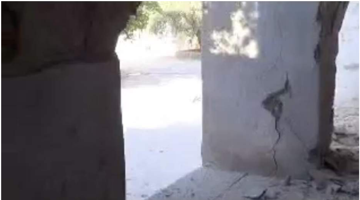
Video still of damage to a column alongside the mosque's courtyard (Sarmin Coordination; September 1, 2012)
