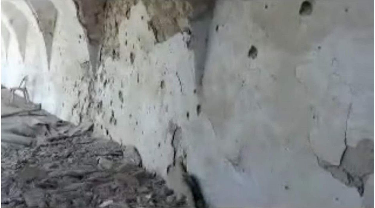
Video still of damage to a wall alongside the mosque's courtyard (Sarmin Coordination; September 1, 2012)
