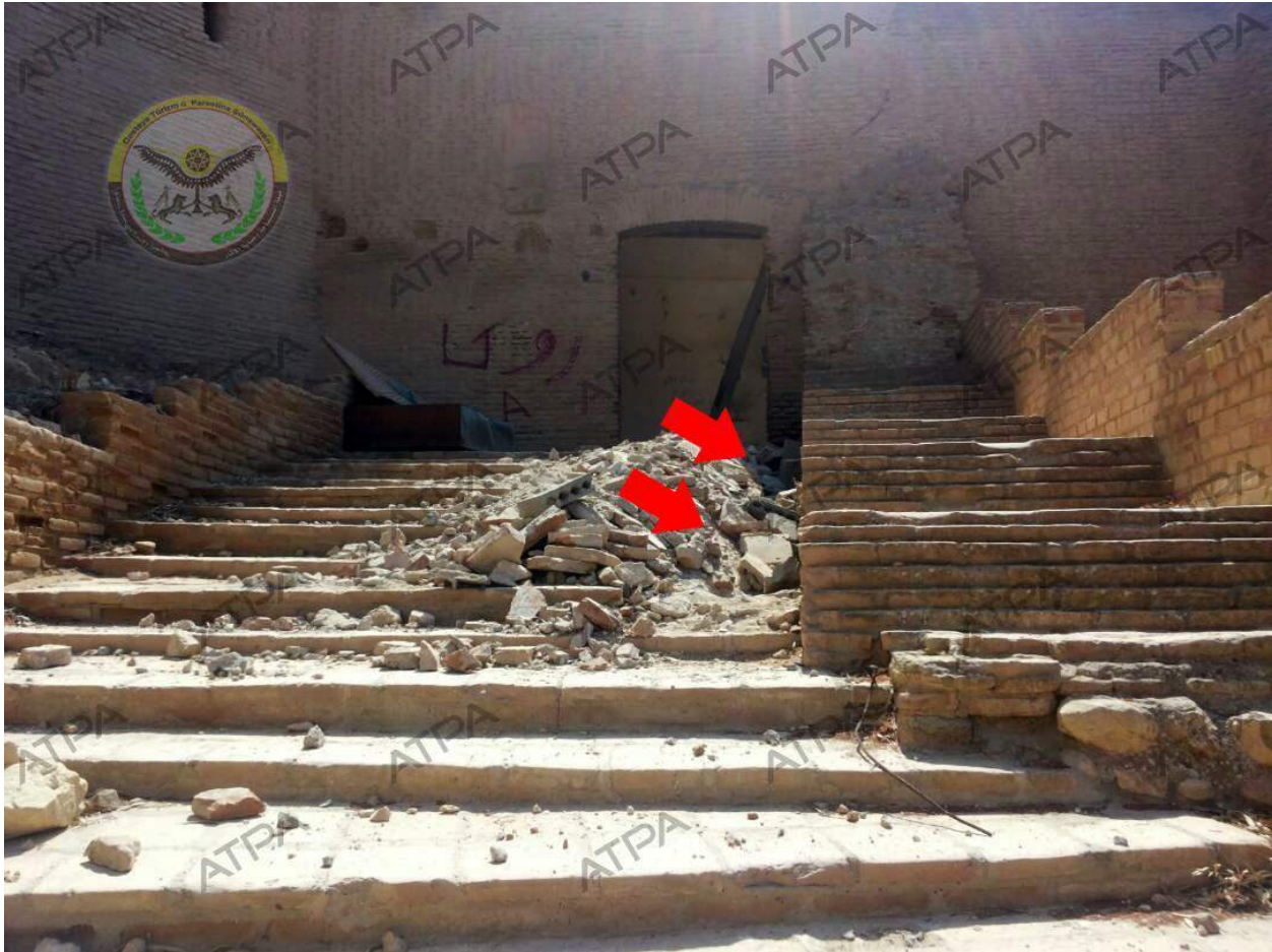
Damage to the entrance of the building as a result of the theft (ATPA; September 23, 2017)
