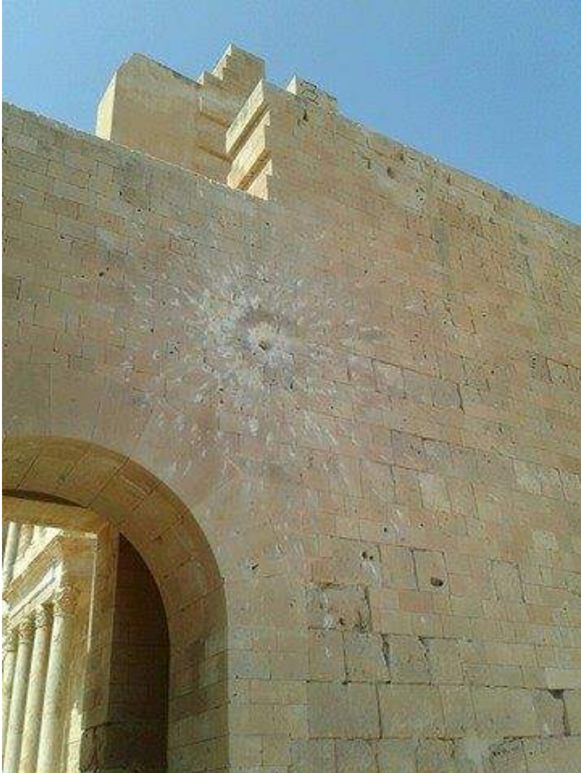
Damage inflicted by what appears to be the detonation of a rocket propelled grenade against the side of the Sabratha Theatre (Source: Sabrata; September 17, 2017)
