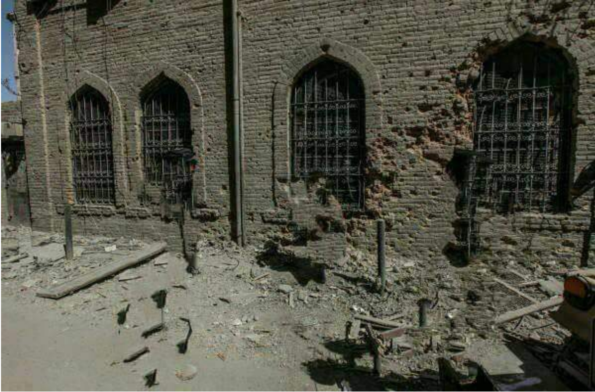
Damage to the western facade of the building (RBSS; September 15, 2017)
