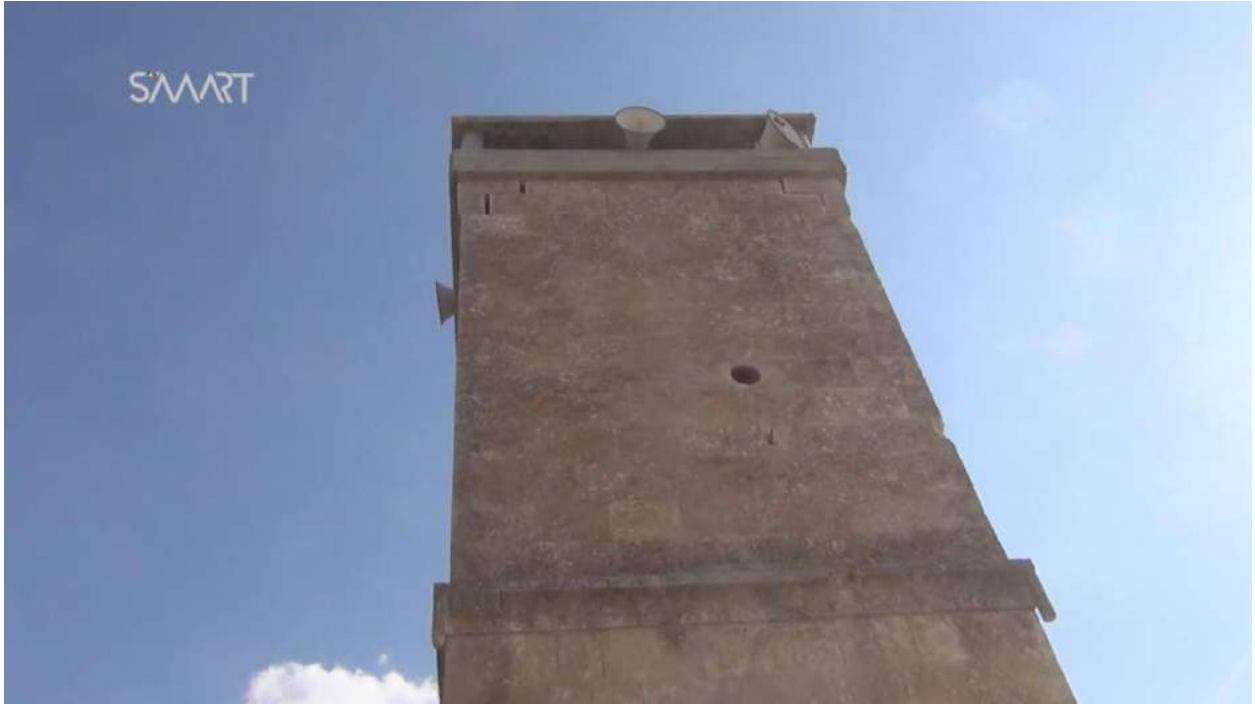
Video still of repairs to the top of the minaret (SMART News Agency; September 28, 2017)
