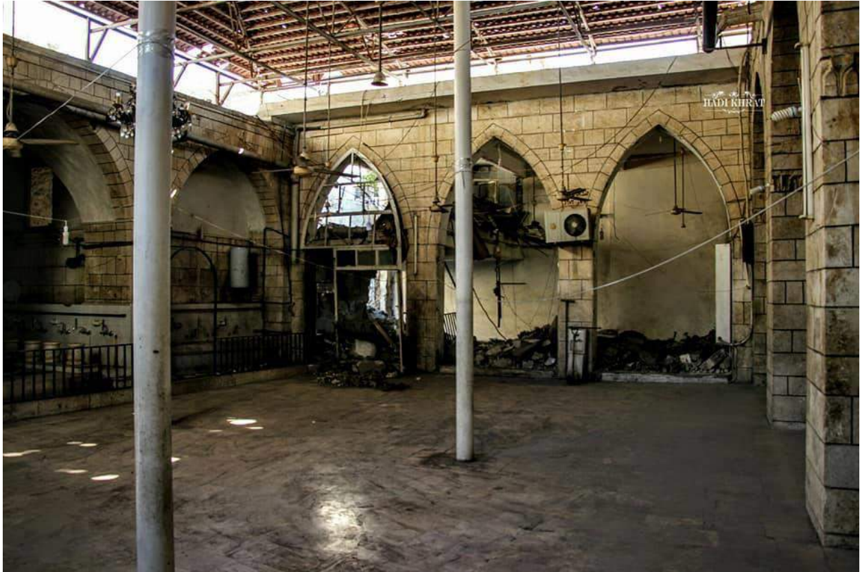
The damaged area of al-Kabir Mosque, visible beyond the arches (SNHR; September 28, 2017)
