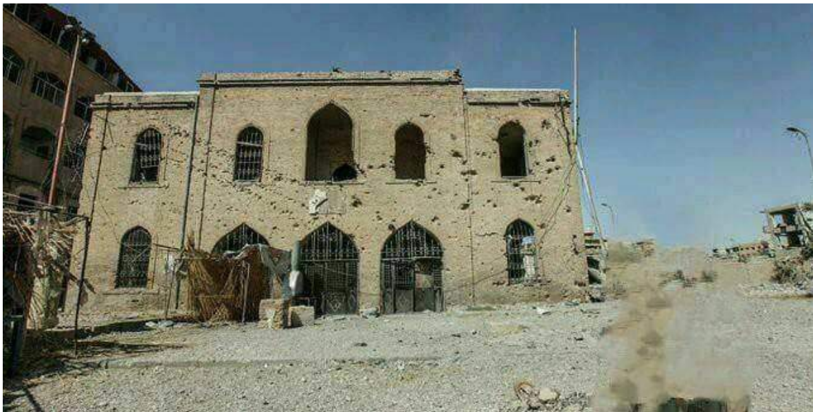
Damage to the southern facade of the museum. The damage on the right half of the facade occurred in November 2014. The three parallel bands on the left half were created more recently (RBSS; September 15, 2017)
