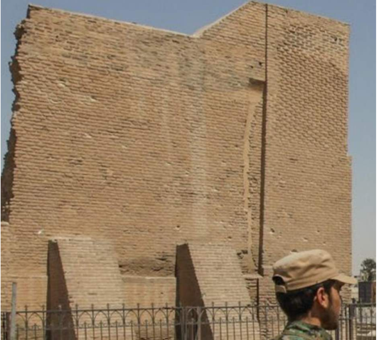
Damage to the southern facade (Personal Twitter Account; September 6, 2017)
