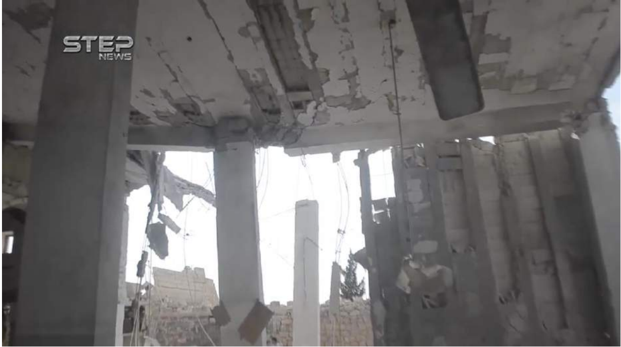
Video still of damage to the mosque's ceiling (SNHR; September 22, 2017)
