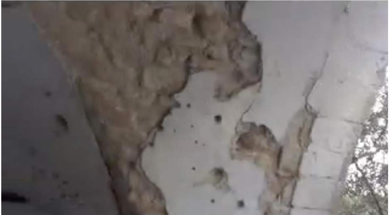
Video still of damage to an arch alongside the mosque's courtyard (Sarmin Coordination; September 1, 2012)
