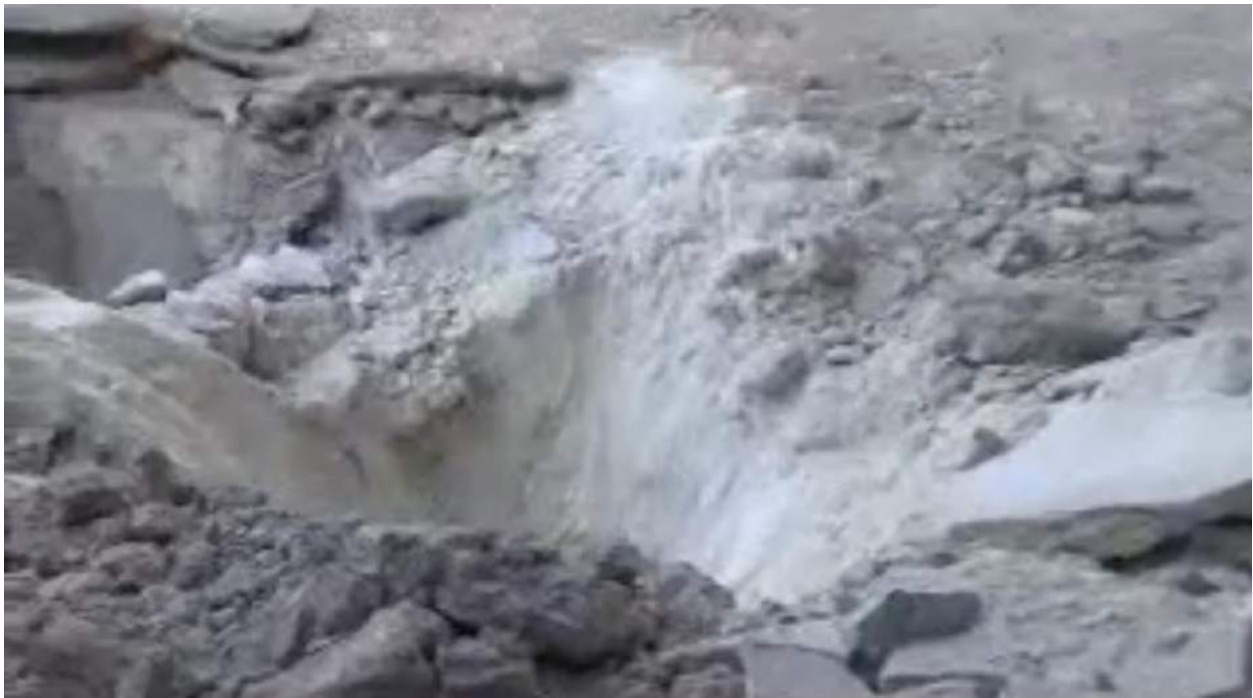
Video still of damage to the floor of an arcade alongside the courtyard (Sarmin Coordination; September 1, 2012)
