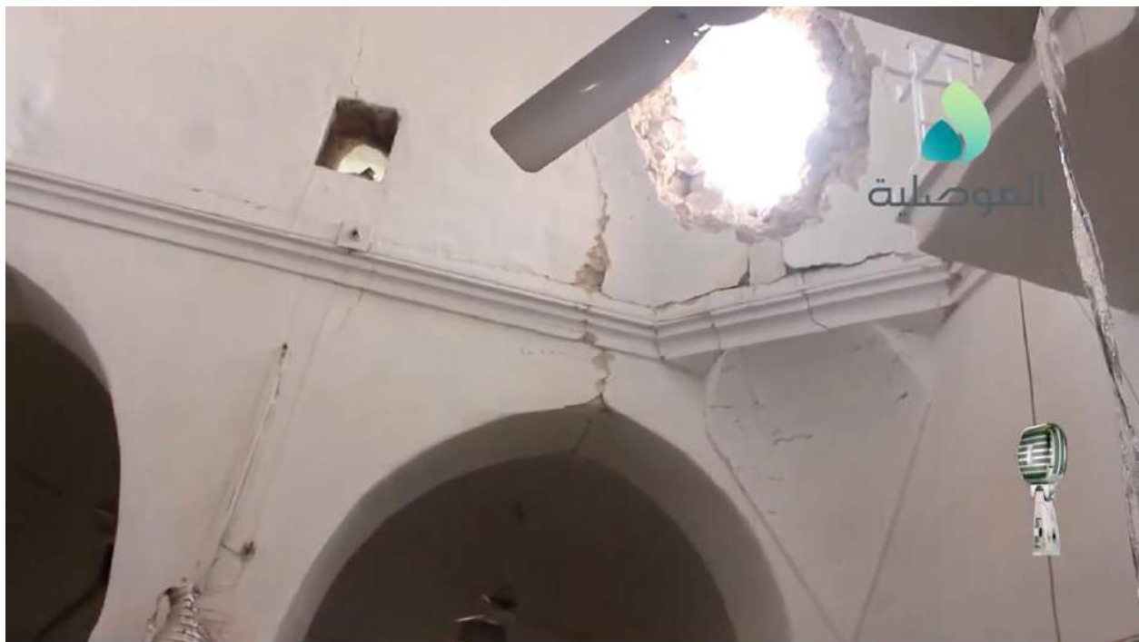
Video still of the interior of al-Nour Mosque showing a hole in the dome above the mihrab (al-Mosuliya; September 6, 2017)
