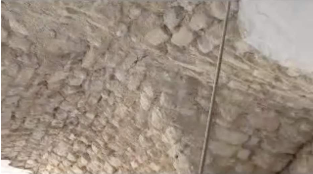
Video still of damage to the roof of an arcade alongside the courtyard (Sarmin Coordination; September 1, 2012)
