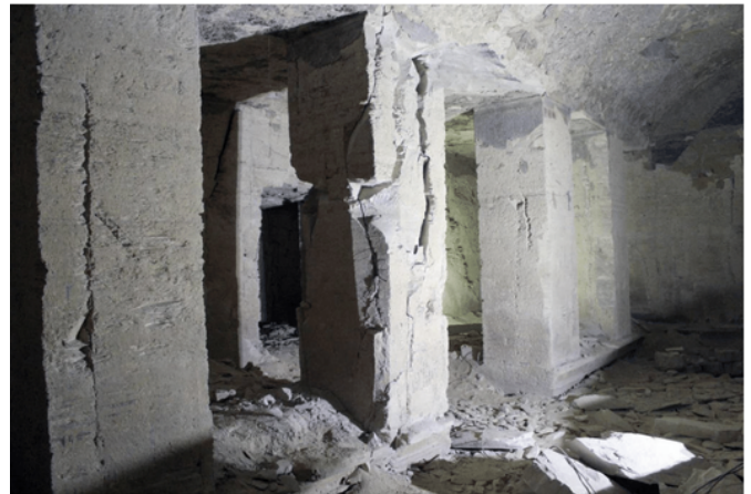
Fig. 3. Pillars in the burial chamber of KV 11 before initial treatment. P1, P5, and P7 (above). P2, P4, P6, and P8 (below). ©The Ministry of Tourism and Antiquities, The Ramesses III (KV 11) Publication and Conservation Project, photos: A. Weber, 2019
