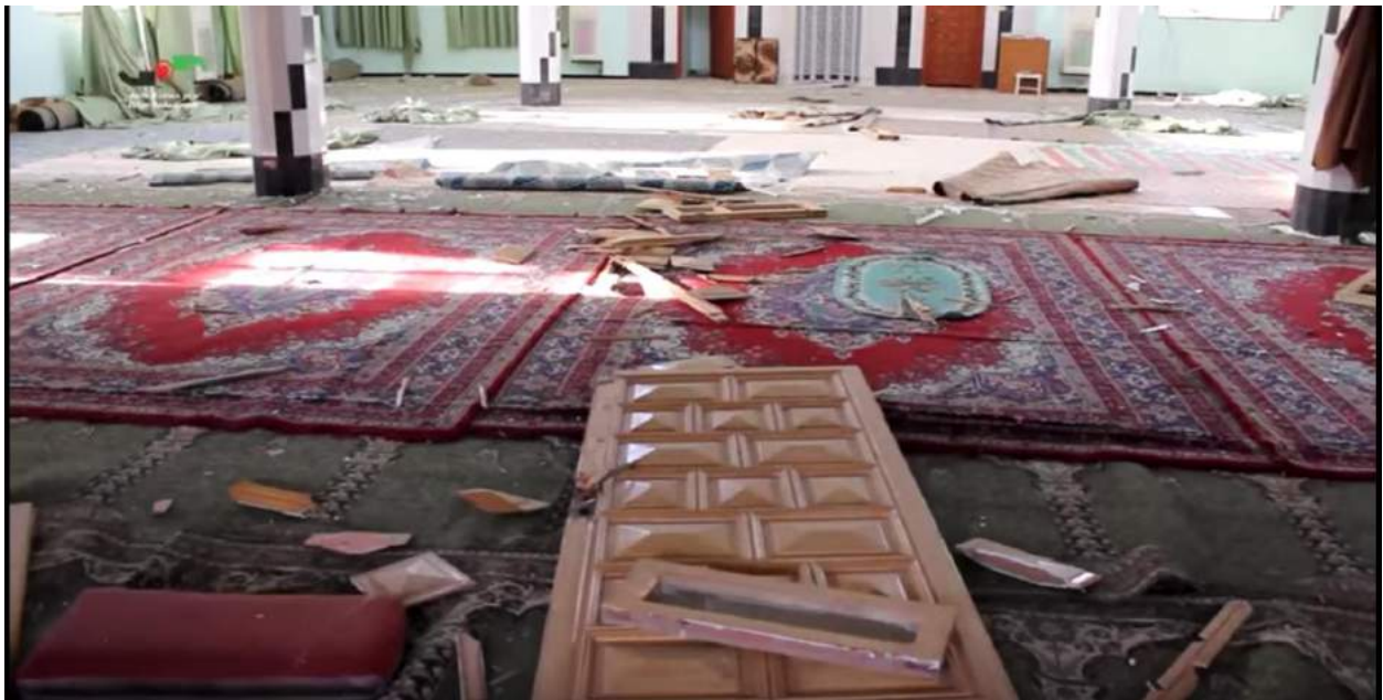
Debris and damage in Abi bin Ali Talib Mosque interior (Homs Media Center; May 20, 2016)
