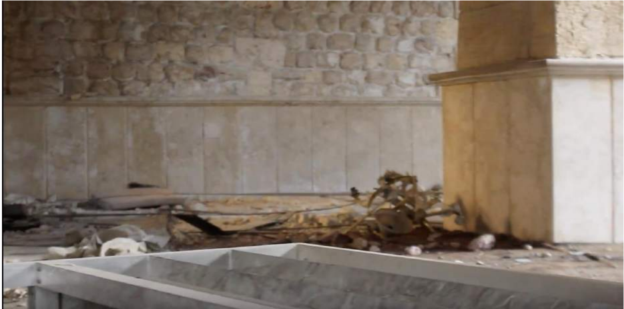
Interior damage in the Haddadin Mosque (Ahmed Melham; May 19, 2016)
