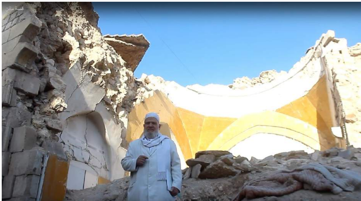
Video still of the damage to Haron Dada Mosque (Ahmed Melham; May 19, 2016)
