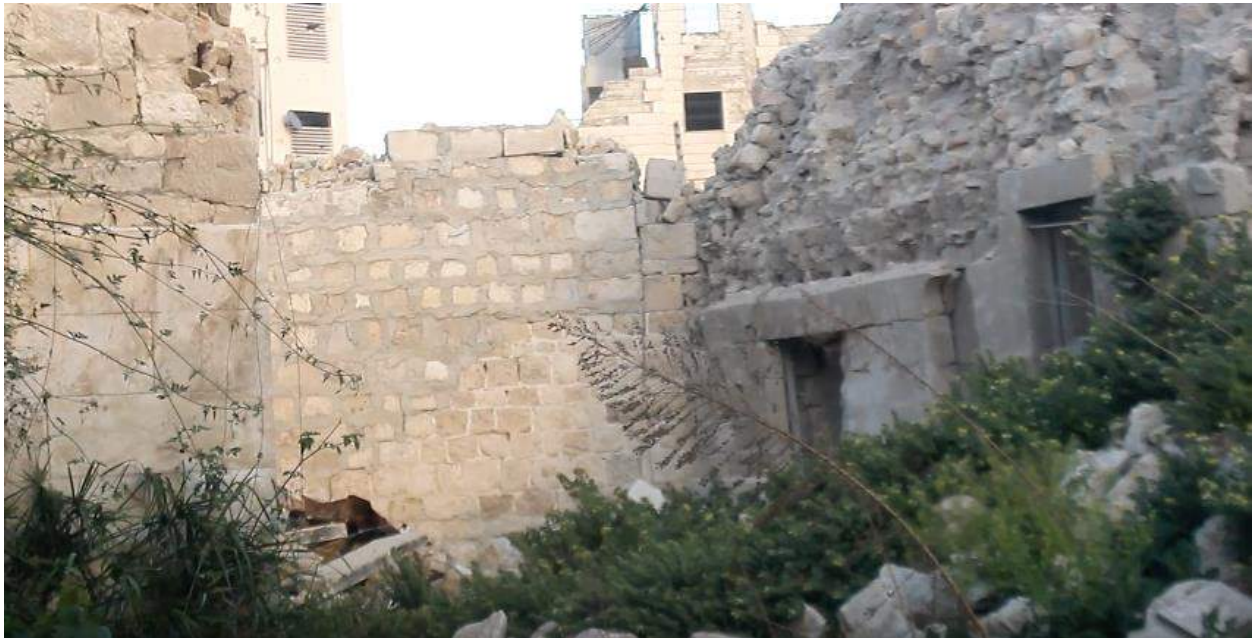
Video still of damage to Al Midani Mosque (Ahmed Melham; May 19, 2016)
