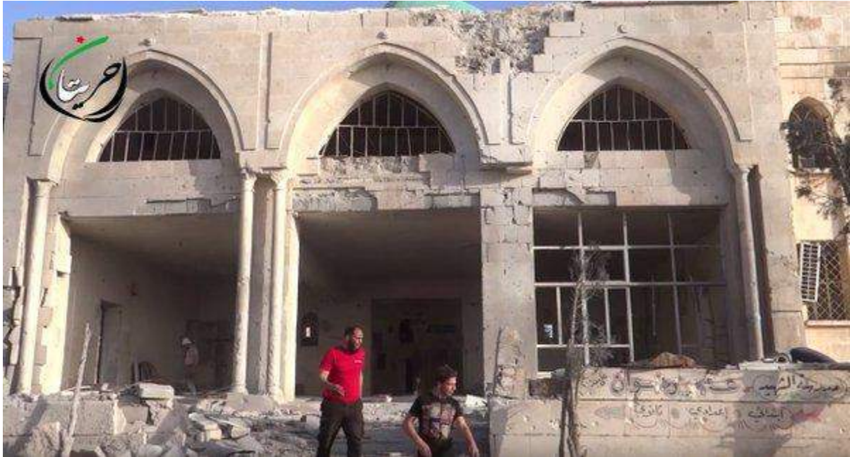
Damage to exterior of Al Bara bin Malek Mosque (Information Center of Hraytan; May 22, 2016)
