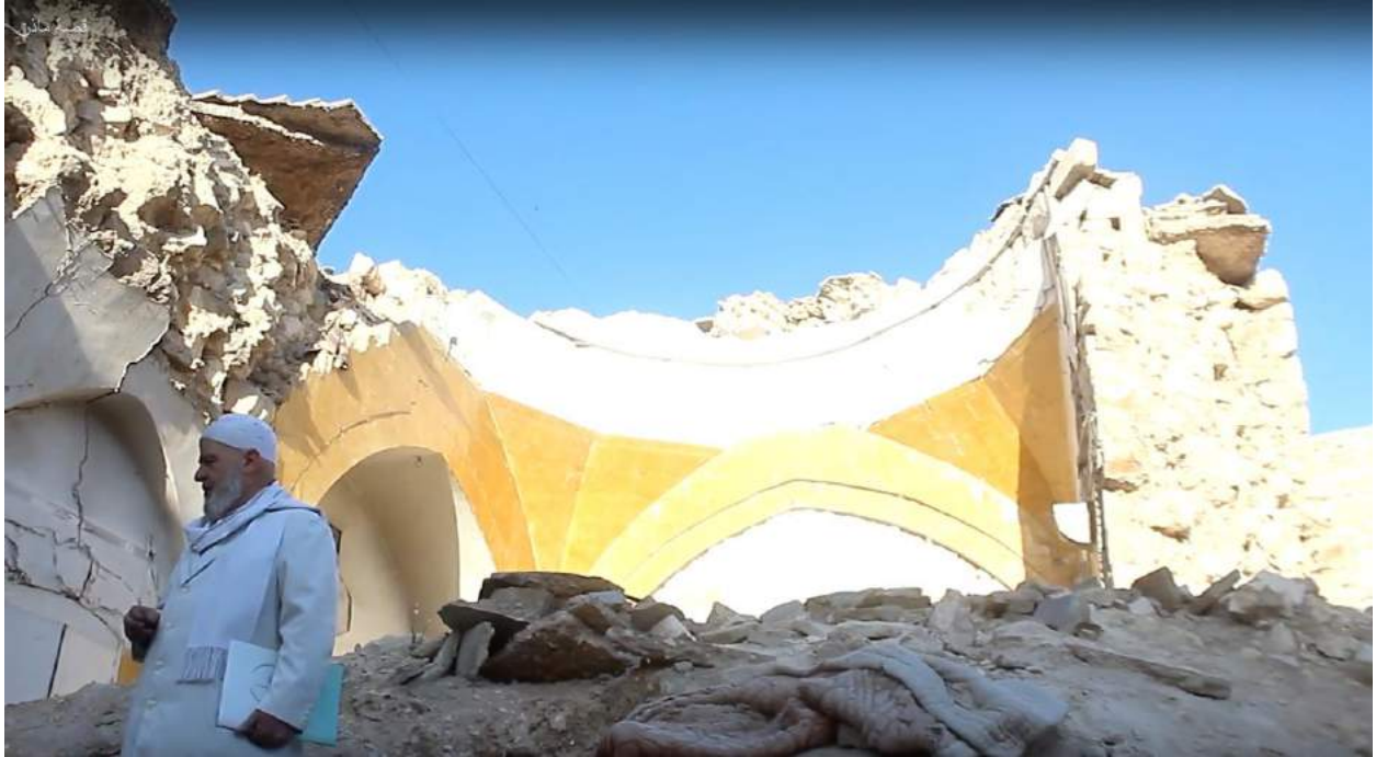
Video still of the damage to Haron Dada Mosque (Ahmed Melham; May 19, 2016)
