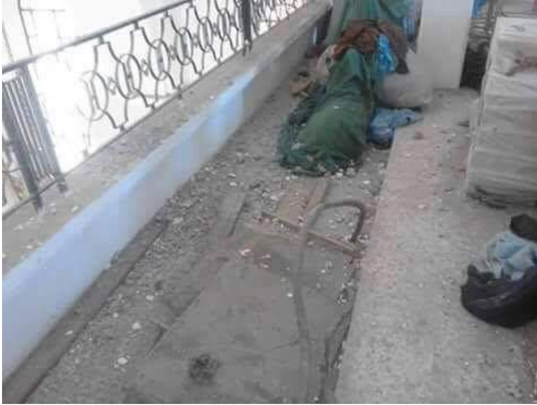
Damage to St George Church (Khaled al Homs; May 19, 2016)
