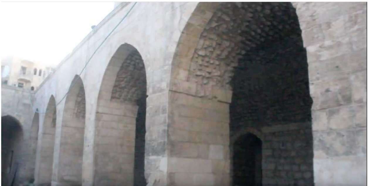
Video still of the exterior of the Haddadin Mosque (Ahmed Melham; May 19, 2016)
