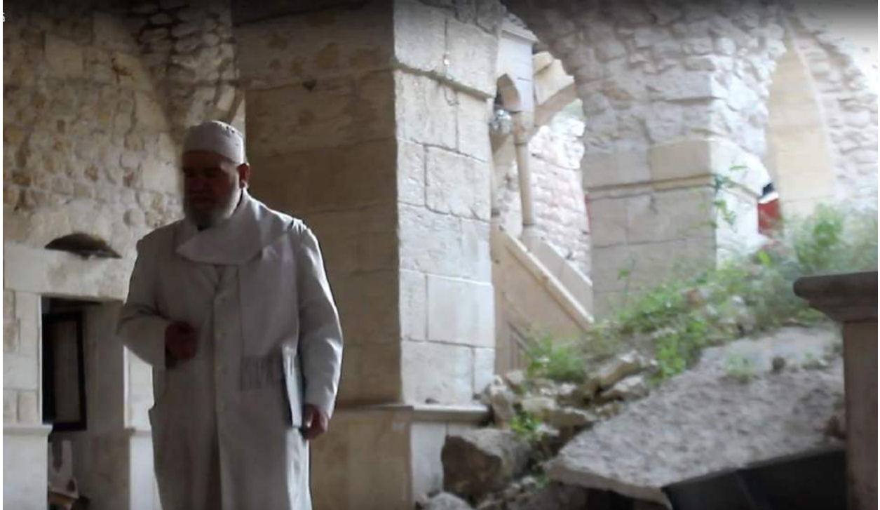
Video still of interior damage to the Haddadin Mosque (Ahmed Melham; May 19, 2016)
