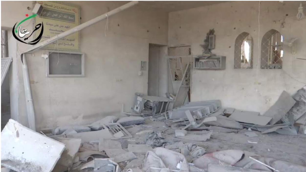
Video still of interior damage to Al Bara bin Malek Mosque (Information Center of Hraytan; May 20, 2016)
