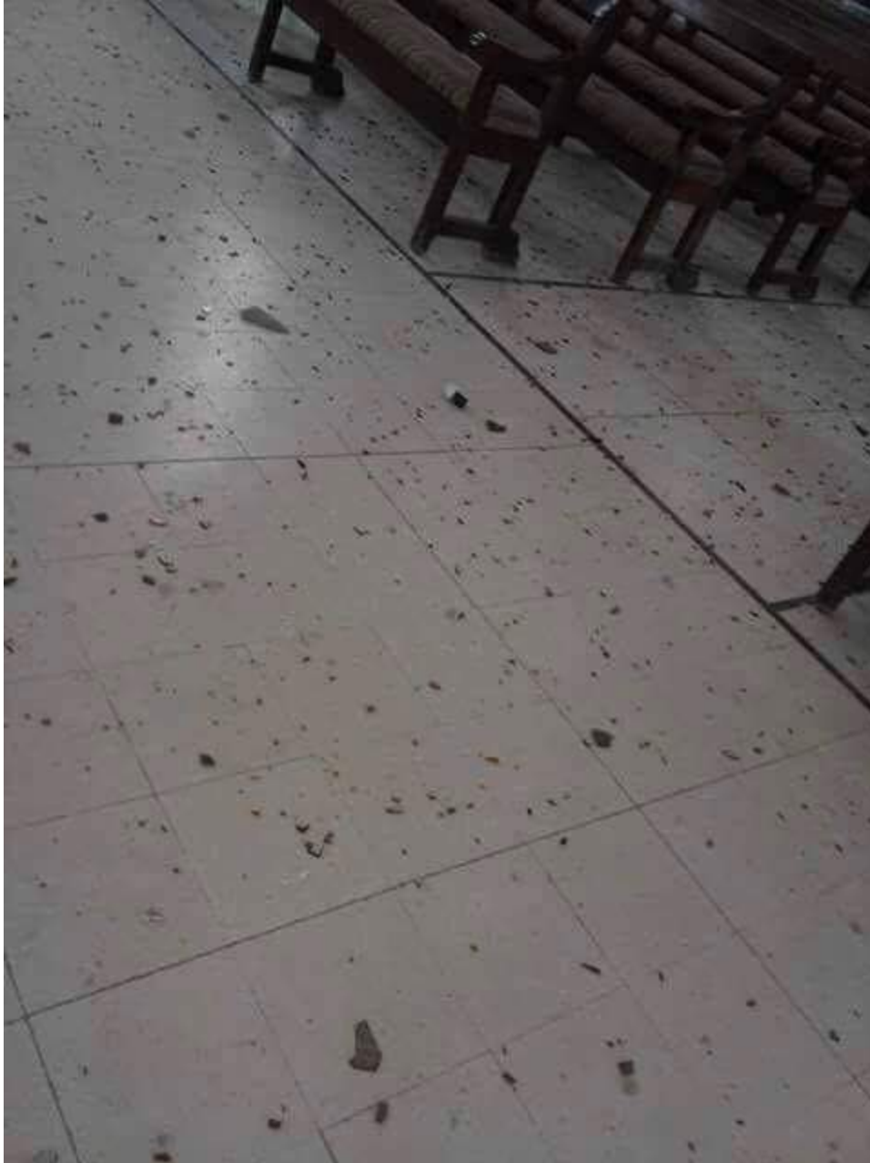
Damage to the interior of St George Church (Khaled al Homs; May 19, 2016)
