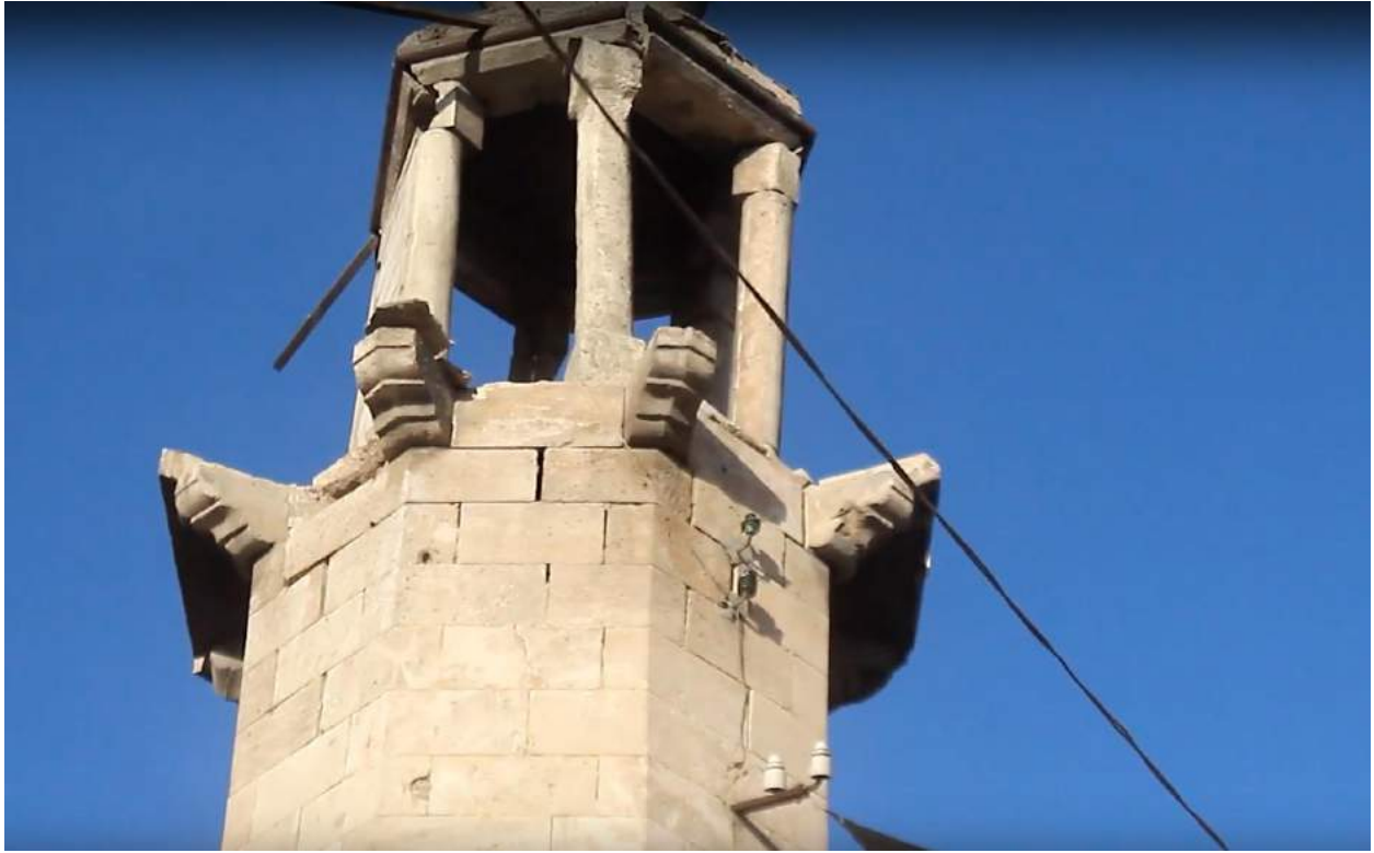
Video still of the damaged minaret at Qadi Askar Mosque (Ahmed Melham; May 19, 2016)
