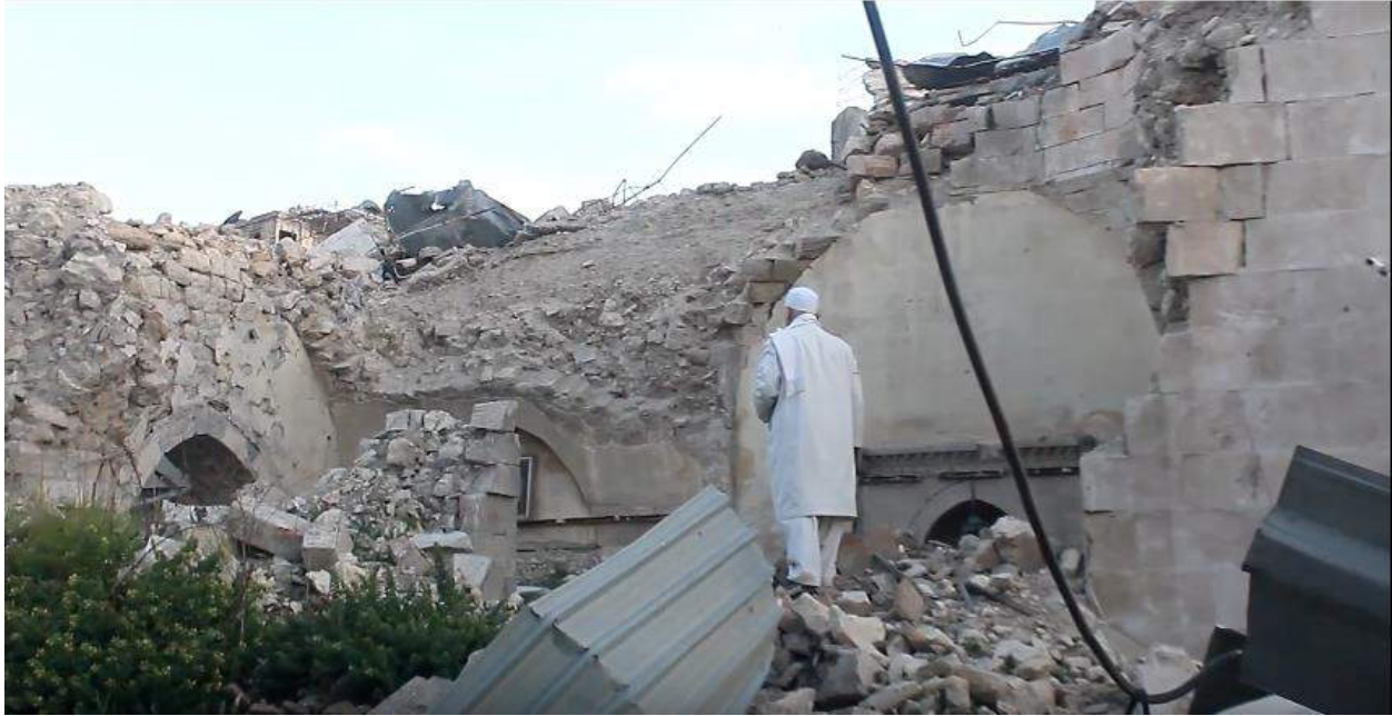
Video still of severe damage to Al Midani Mosque (Ahmed Melham; May 19, 2016)
