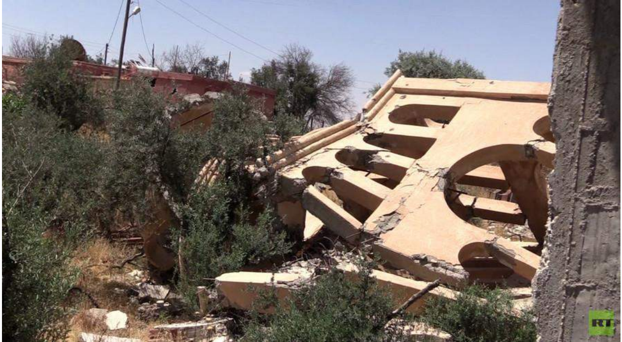
A fallen wall at the Church of the Virgin Mary (RT Arabic/RT; May 22, 2016)
