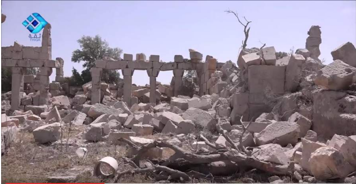
Destruction of south and west walls of monastery (from interior, facing south) (Wikalat Thiqa; May 13, 2016)
