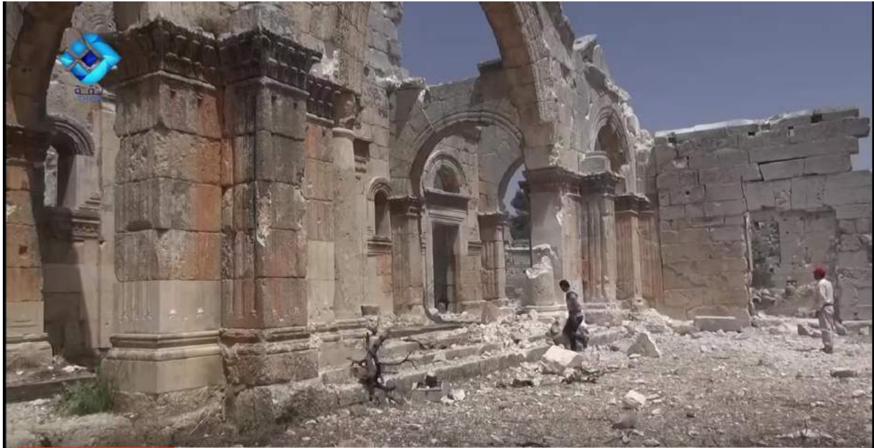
View of damage to central and eastern arches of main entrance (looking east) (Wikalat Thiqa; May 13, 2016)
