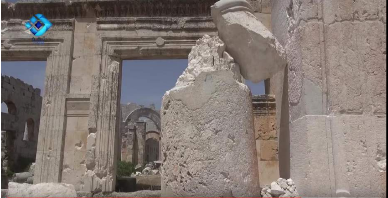
Damage to pillar on central arch of main entrance (Wikalat Thiqa; May 13, 2016)
