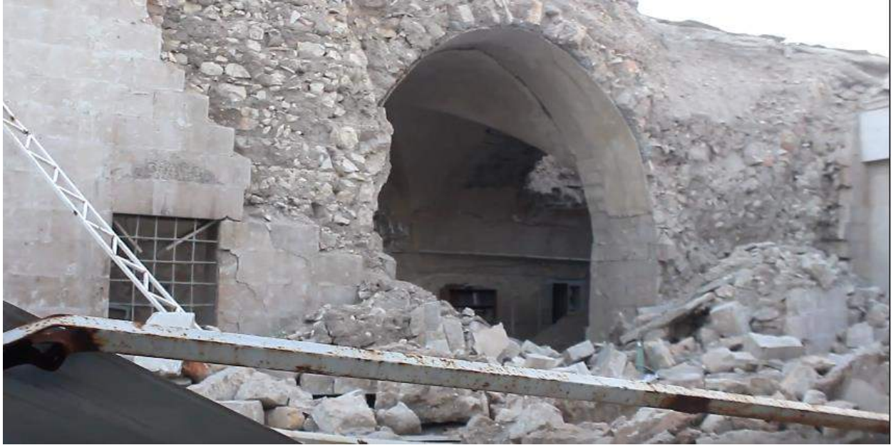
Video still of damage to Al Midani Mosque (Ahmed Melham; May 19, 2016)
