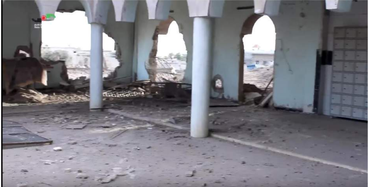
Severe structural damage to Abi bin Ali Talib Mosque (Homs Media Center; May 20, 2016)
