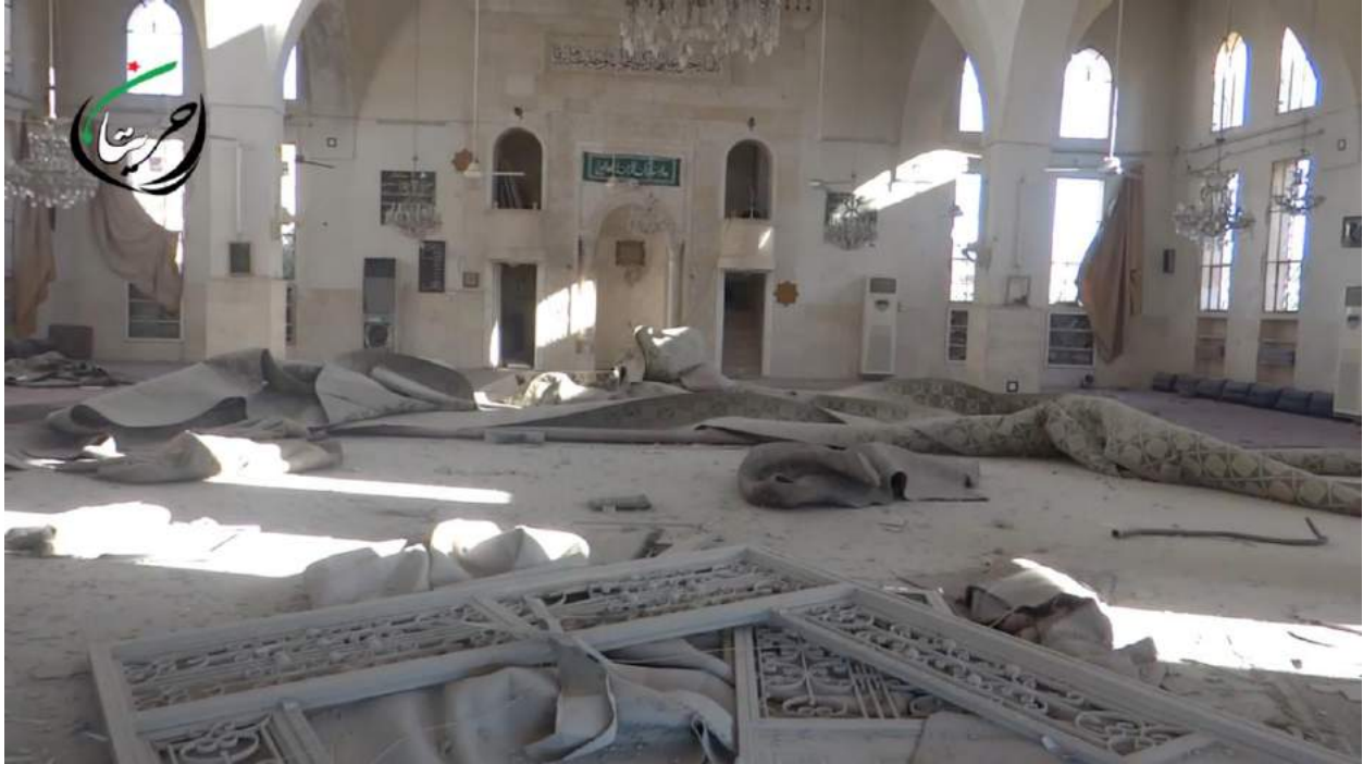
Video still of interior damage to Al Bara bin Malek Mosque(Information Center of Hraytan; May 20, 2016)
