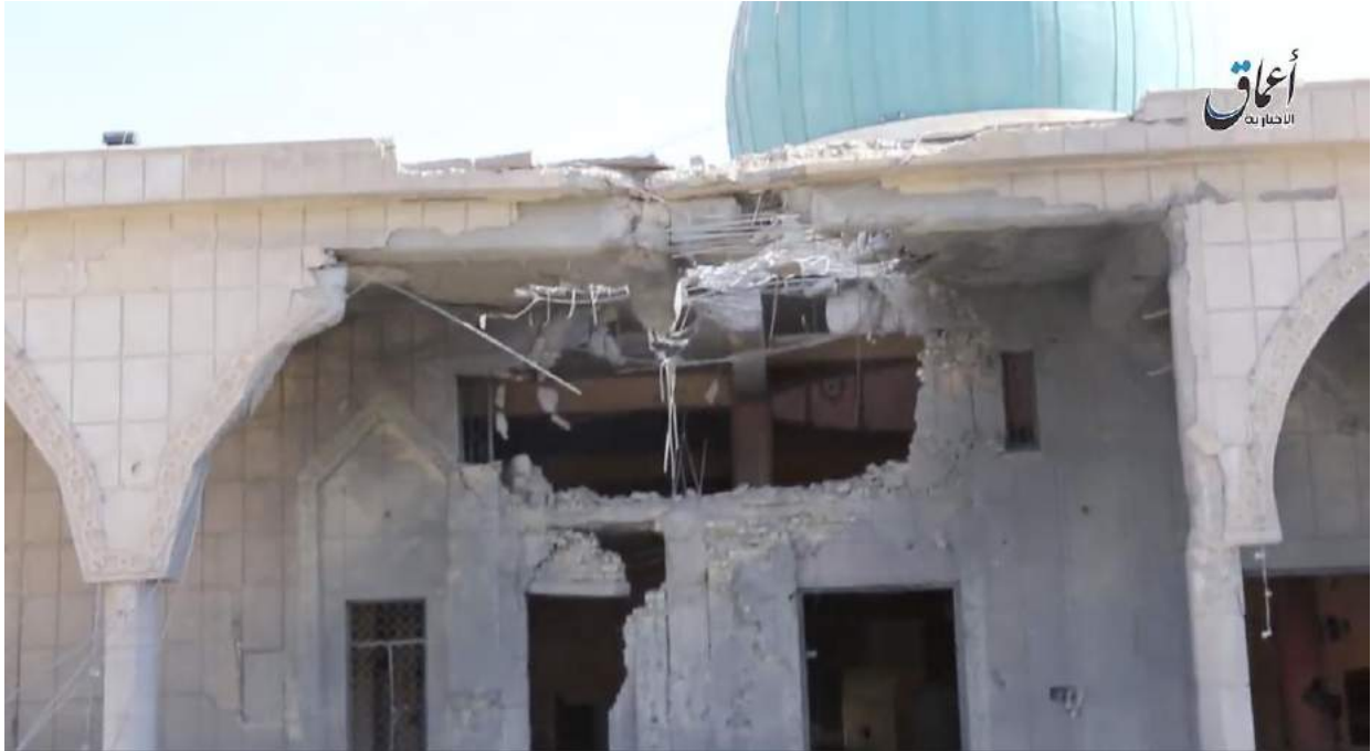
Detail of damage to Al Raqib Mosque (Amaq News Agency; May 23, 2016)
