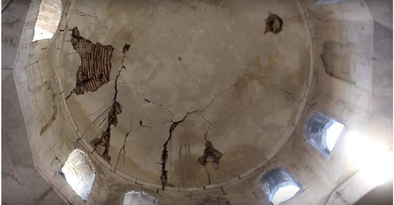
Video still of damage to unidentified mosque (Ahmed Malhim; May 19, 2016)
