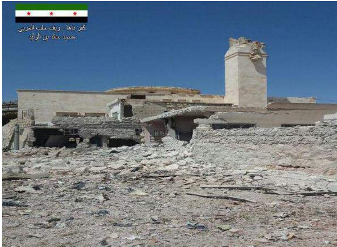
Damage to Khalid Ibn Al-Walid Mosque (Twitter; May 23, 2016) 158
