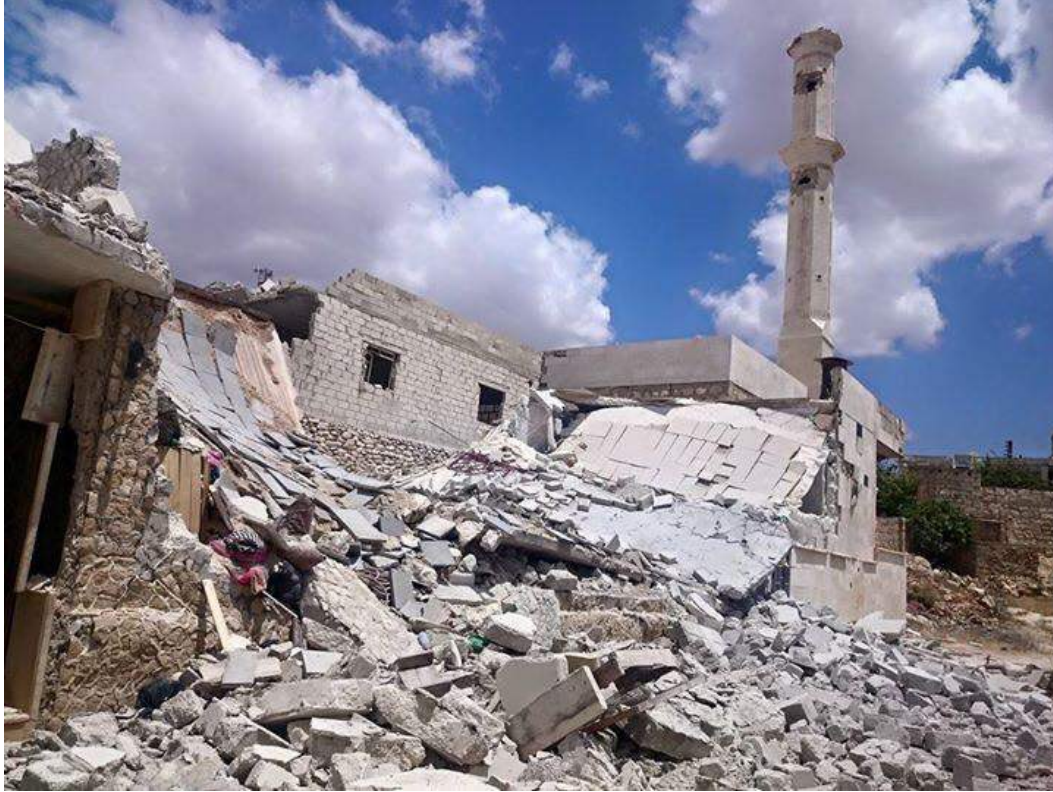
Extensive damage to Ammar Bin Yasser Mosque (Shahba Press/Kafar Hamra Media Center; May 23, 2016)
