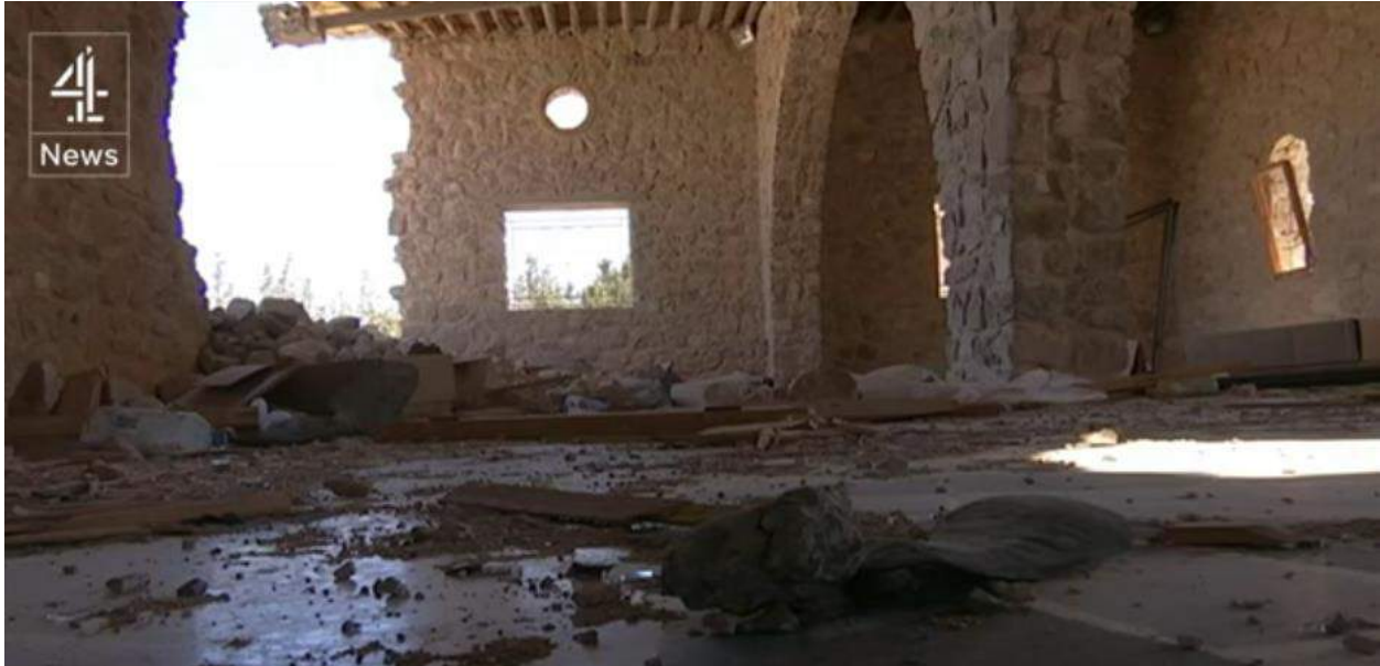
Video still of damage to Mar Elian Monastery (Channel 4 News; April 4, 2016)
