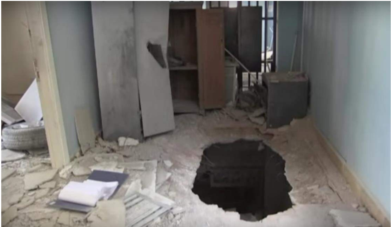
Video still of possible airstrike damage to the floor of the museum (AFP; April 1, 2016)
