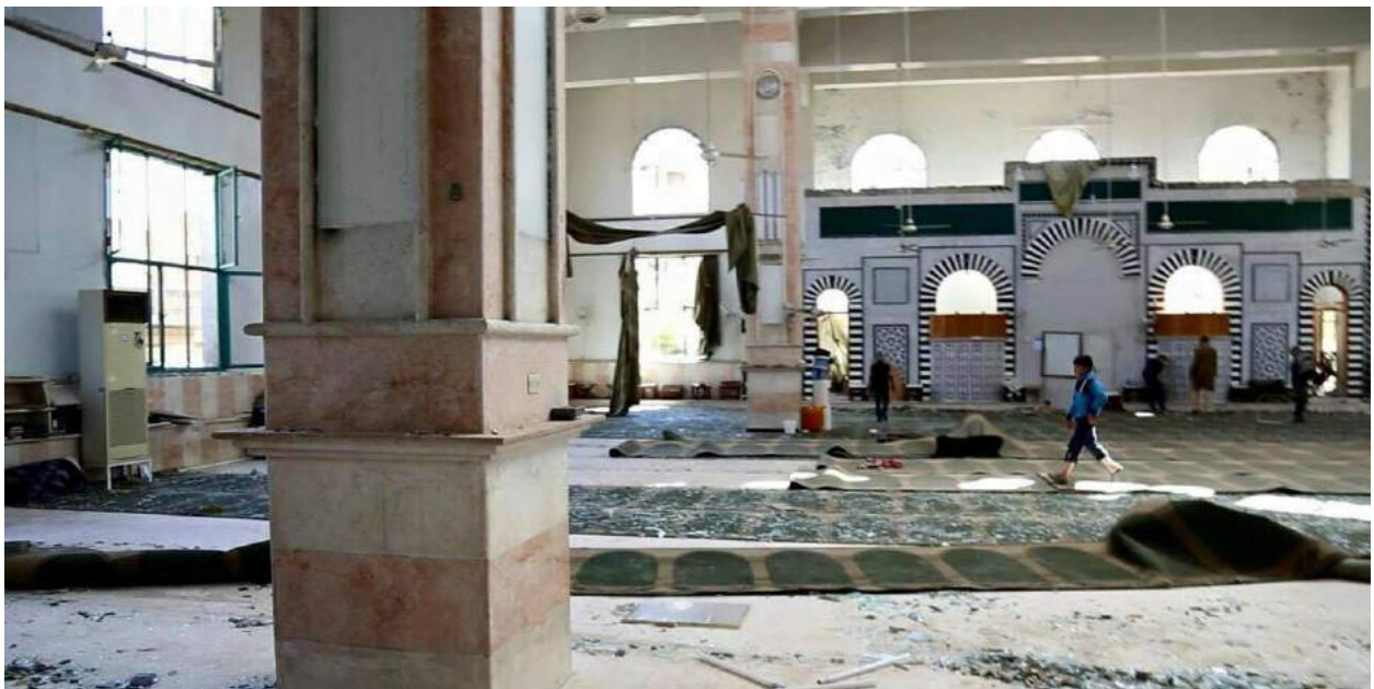
Broken glass and debris inside al-Nur Mosque (RBSS; April 1, 2016)
