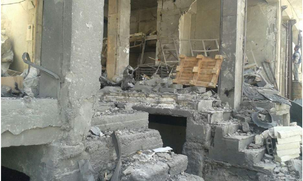
Damage to the exterior of al-Kabir Mosque (TDA; Provided to ASOR CHI on April 7, 2016)
