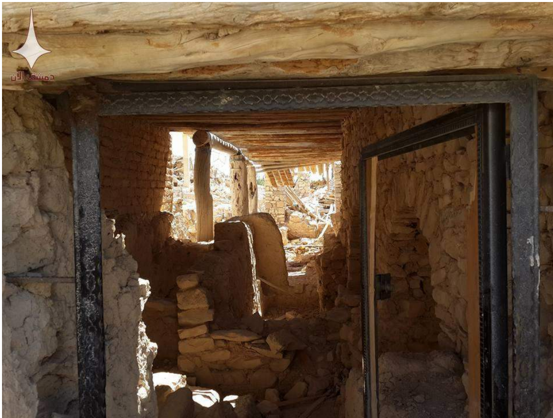
Damage to Mar Elia Monastery (Dimashq Al An; April 4, 2016)
