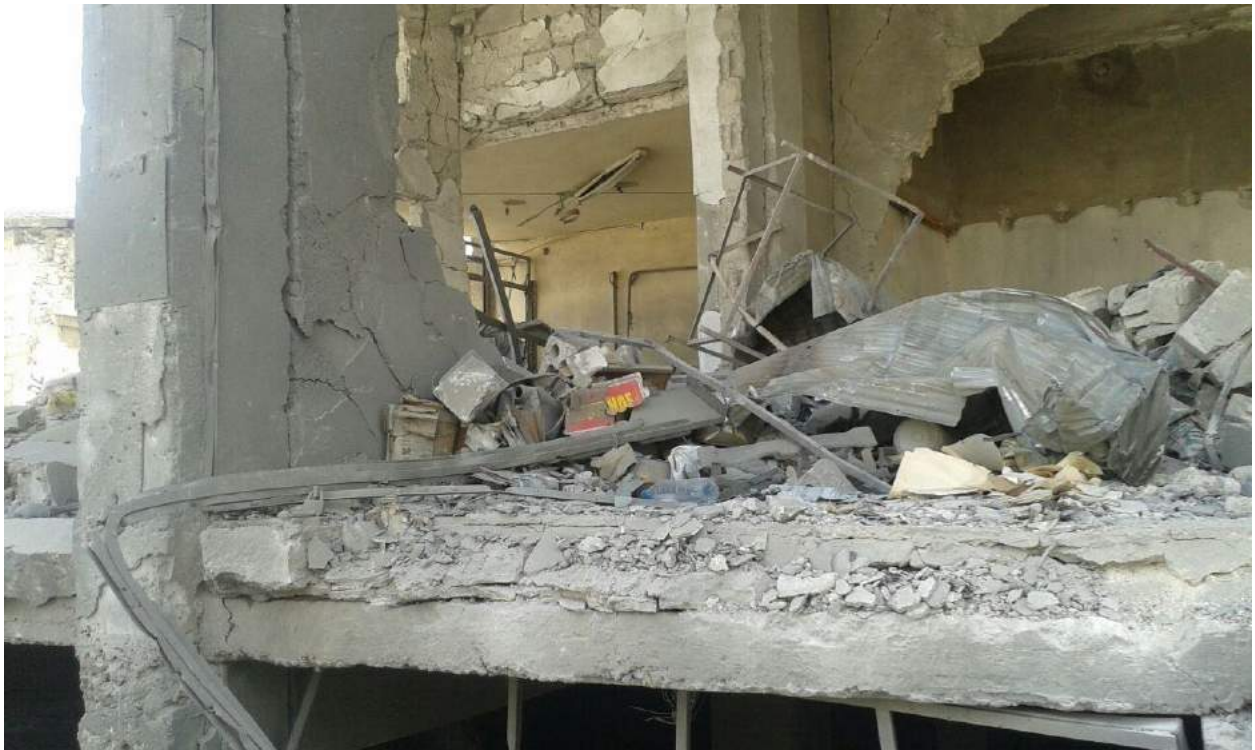
Damage to the exterior of al-Kabir Mosque (TDA; Provided to ASOR CHI on April 7, 2016)
