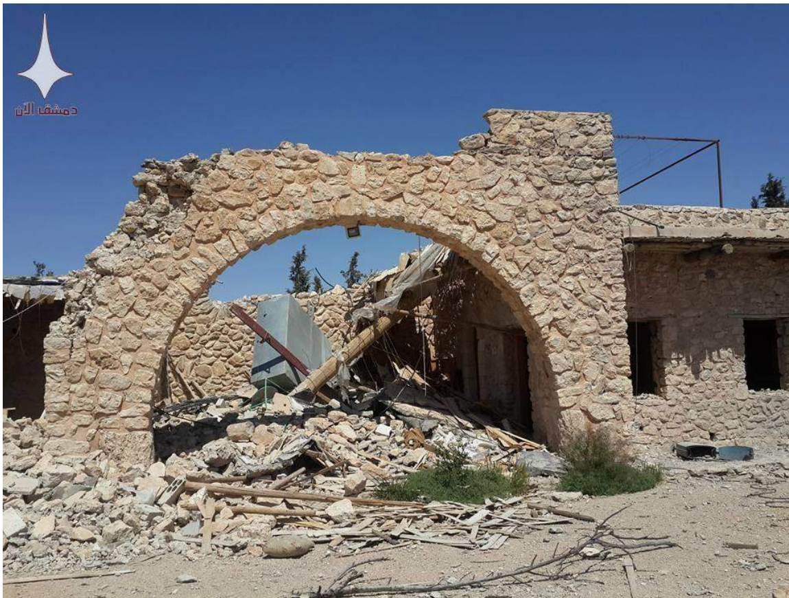
Detail of damage to Mar Elia Monastery (Dimashq Al An; April 4, 2016)
