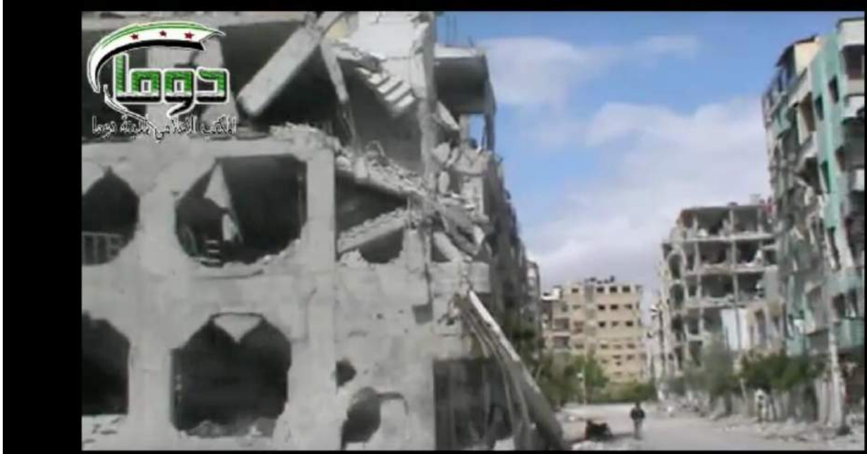
Severe damage to the ar-Rawda Mosque from an airstrike (Free Syr/Youtube; April 23, 2013)
