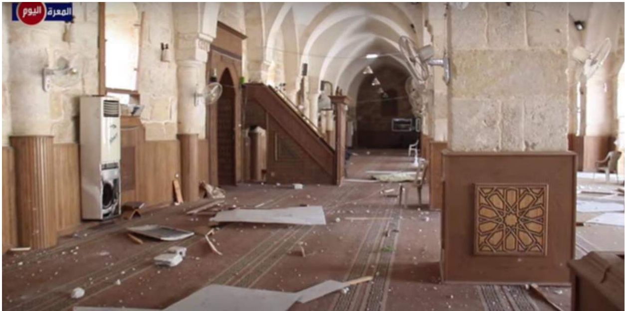
Video still of damage and debris in interior of al-Kabir Mosque (Al-Marra Today; April 5, 2016)
