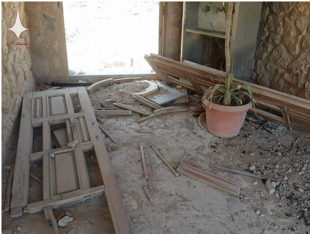
Damage to Mary Elian Monastery (Dimashq Al An; April 4, 2016)
