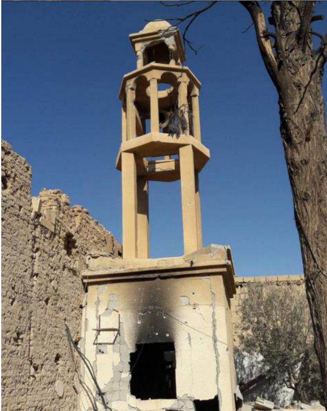
Damage to Mar Elian Monastery (Lizzie Phelan; April 4, 2016)
