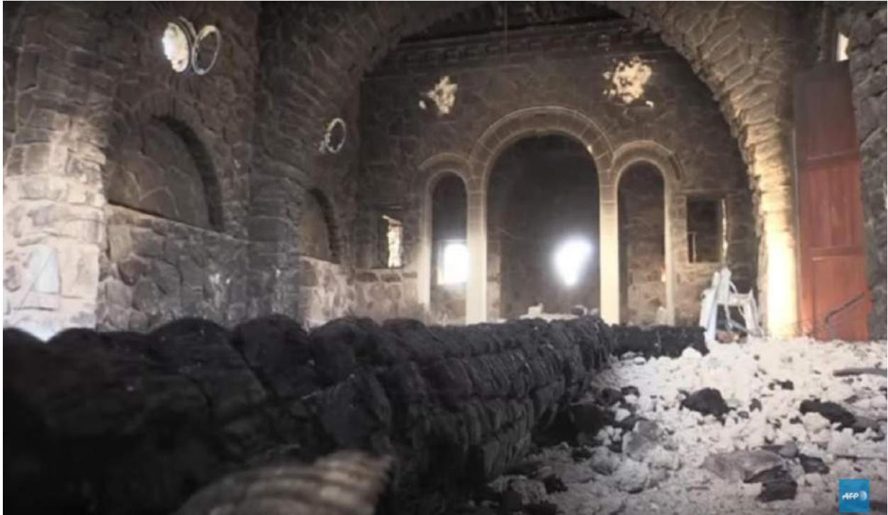
Video still of possible burned ceiling beam inside Mar Elian Monastery (AFP; April 4, 2016)
