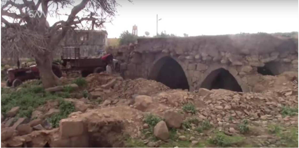
Video still of damage caused by what appears to be ongoing theft at Rafid (APSA; April 11, 2016)
