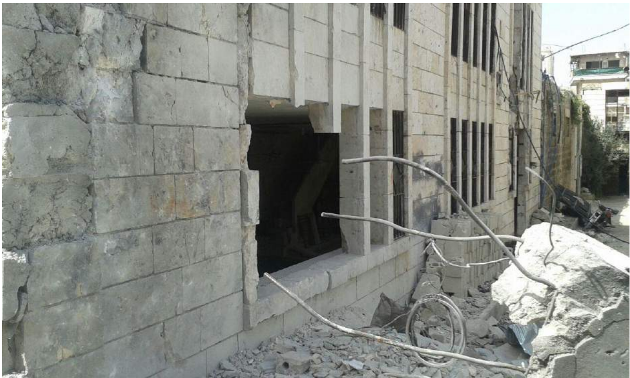
Damage to the exterior of al-Kabir Mosque (The Day After Heritage Protection Initiative (TDA); Provided to ASOR CHI on April 7, 2016)
