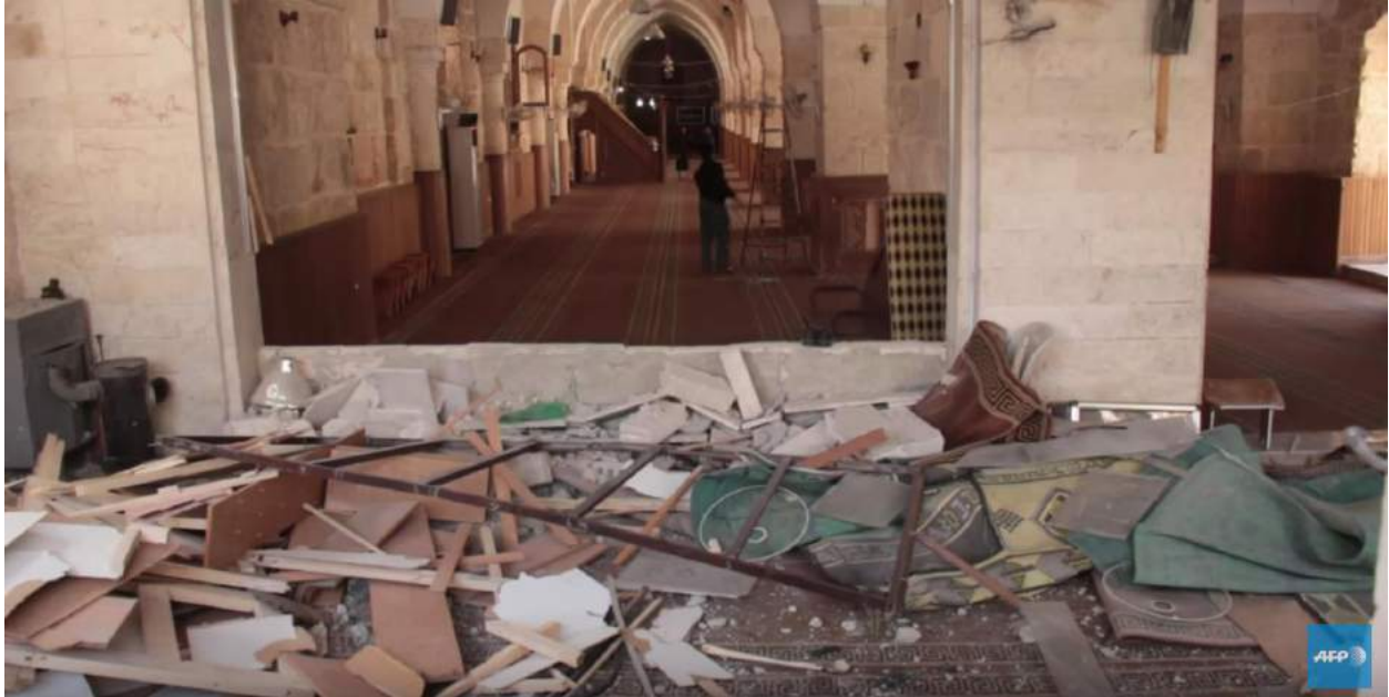
Damage and debris in interior of al-Kabir Mosque (AFP via SOHR; April 5, 2016)
