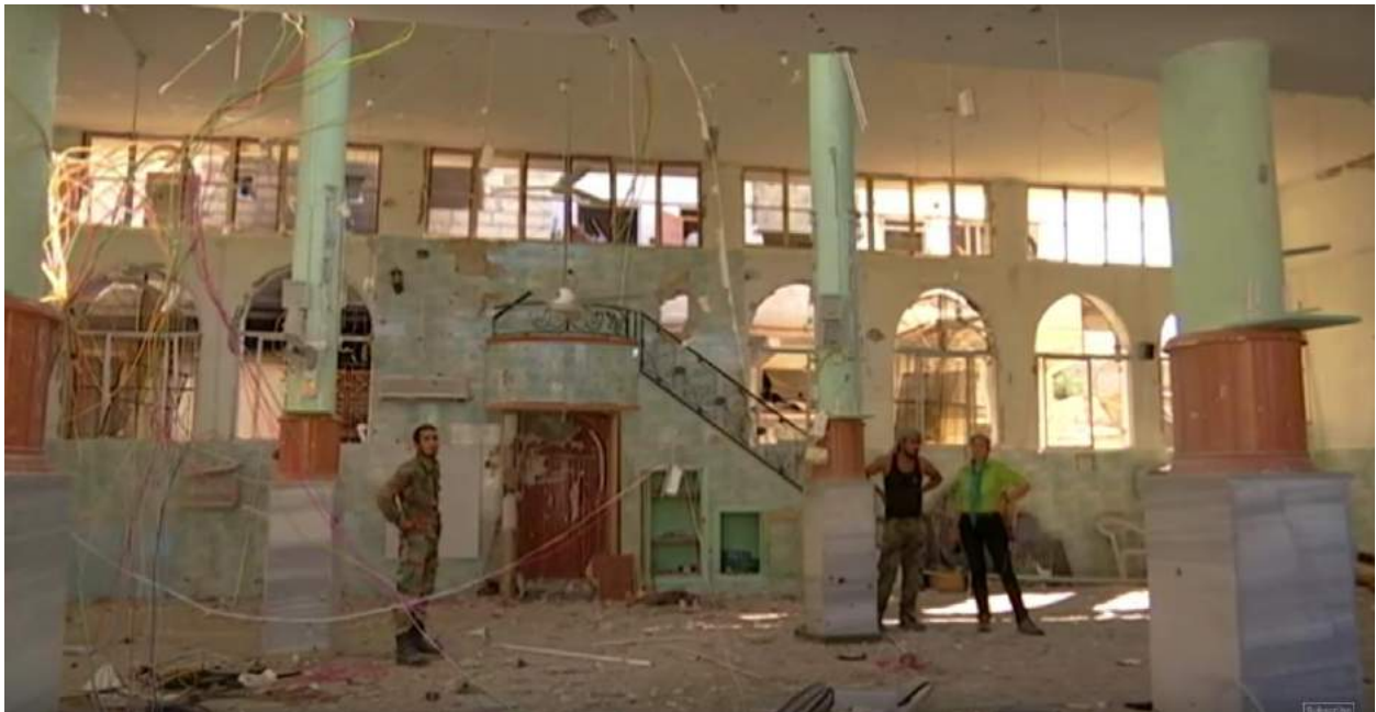
Video still of the damaged interior of Bilal Mosque (Channel 4 News; April 5, 2016)
