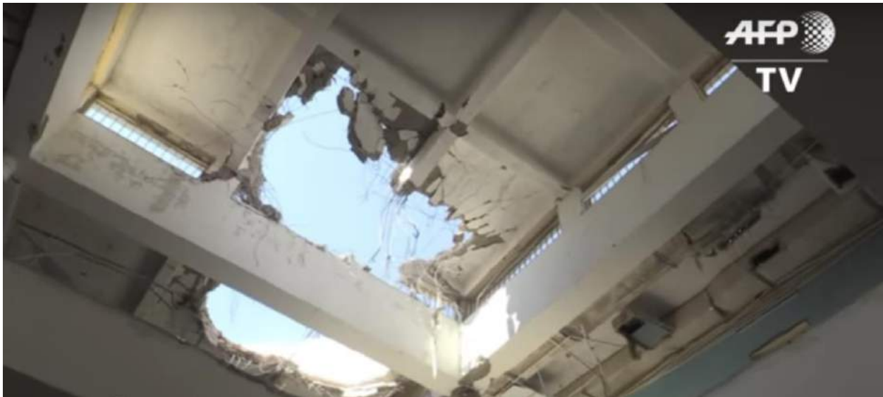
Video still of possible airstrike damage to the ceiling of the museum (AFP; April 1, 2016)
