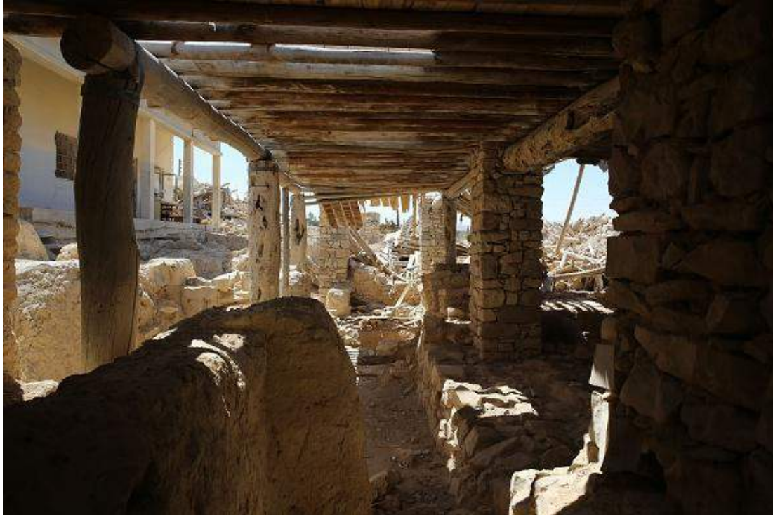
Damage to Mar Elia Monastery (Joseph Eid/Getty Images; April 4, 2016)
