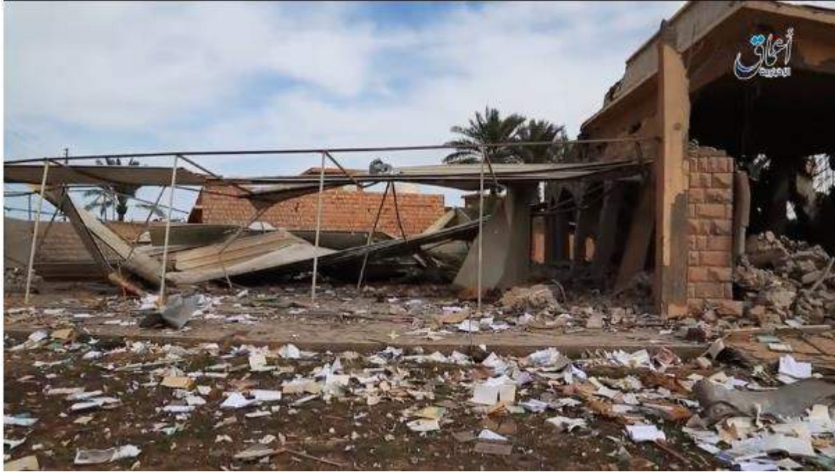
Still image of the damage to the surrounding area of Al-Farooq Mosque (Internet Archive; March 15, 2016)
