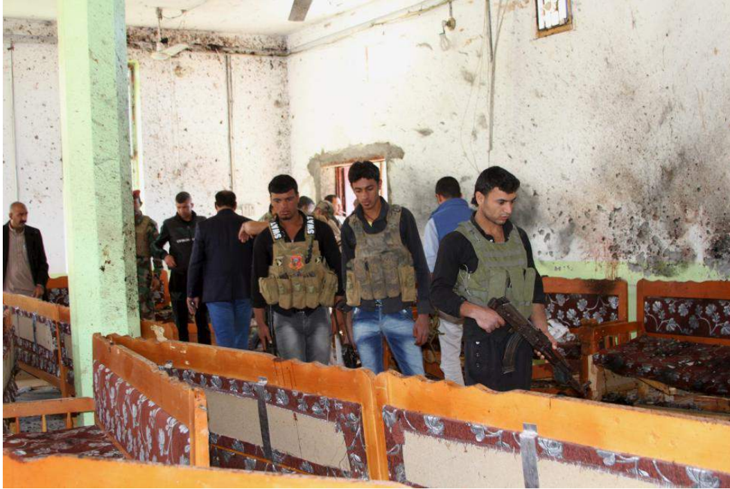
Interior of the Shia Mosque in Muqdadia showing material damage (Reuters; March 1, 2016)
