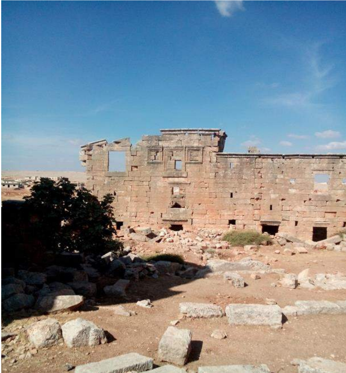
Illicit digging at the site and near to the walls causing damage to buildings and foundations.
