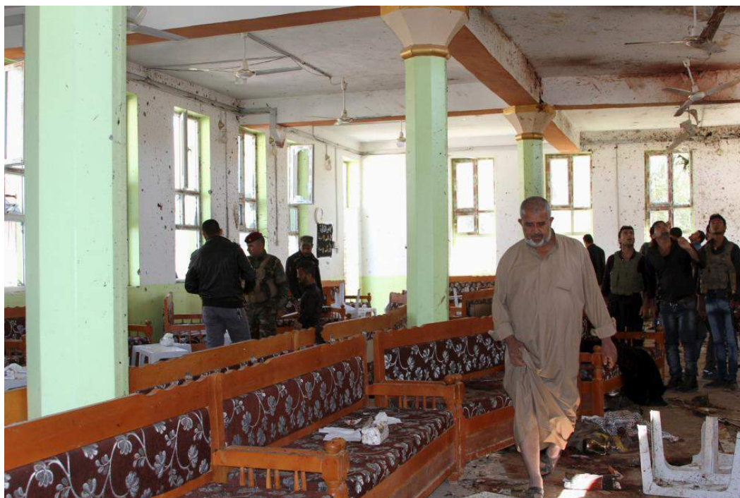
Damage to the interior of the Shia Mosque (Reuters; March 1, 2016)
