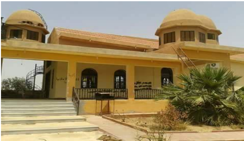
Damage to Mar Zaia Church, Tel Goran (Halmon.net; Poste June 13, 2015)
