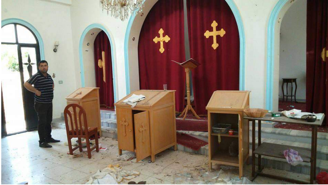
Damage to the interior of Mar Sawa Church, Tel Jadiya (Halmon.net; Posted June 5, 2015)
