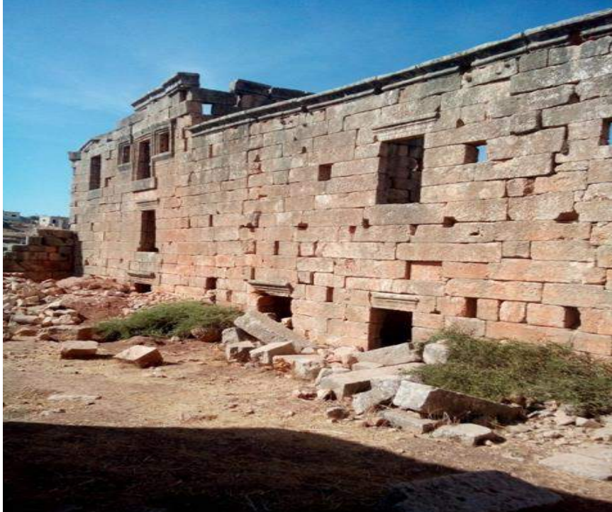
Damage caused by vegetation
