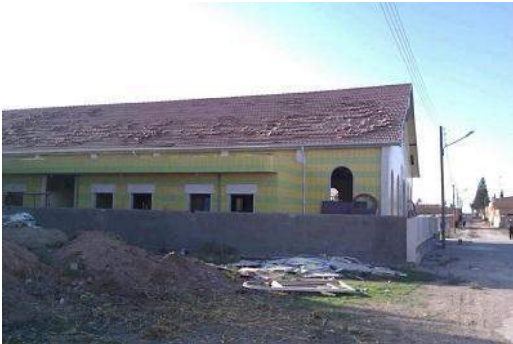
Damage to Church of the Virgin Mary, Tel Nasri (AINA; Posted November 15, 2012)
