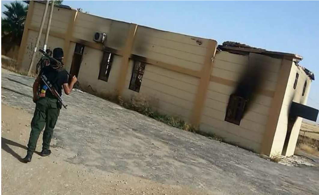
Damage to Mar Haneina Church, Tel Sakra (Halmon.net; Posted May 29, 2015)
