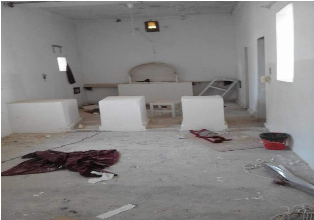
Damage to Mar Shimon Prusbai, Tel Kharita (Halmon.net; Posted June 16, 2015)
