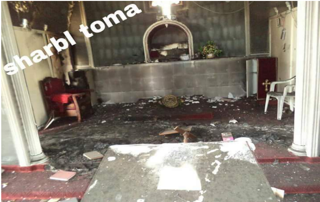
Damage to the interior of Mar Giorgis and Mar Shimon Prusbai Church, Tel Balua (Halmon.net; Posted June 5, 2015)
