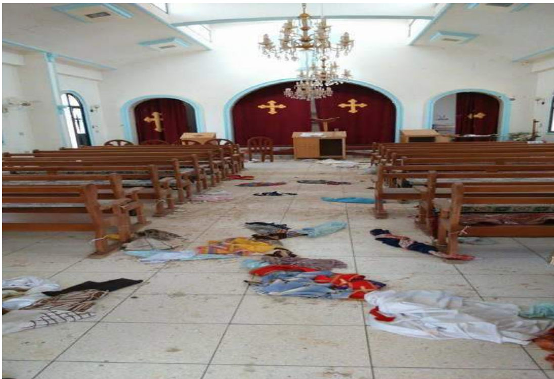
Damage to the interior of Mar Sawa Church, Tel Jadiya (Halmon.net; Posted June 5, 2015)
