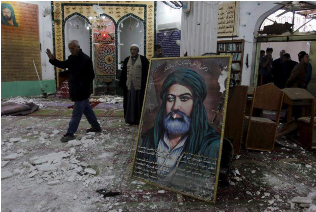
Interior of Rasul al-Azam Mosque showing material and structural damage (Reuters/Khalid al-Mousily; February 26, 2016)
