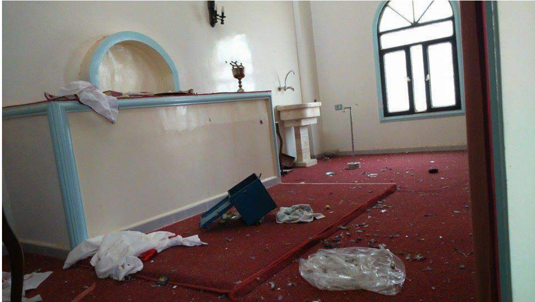
Damage to the interior of Mar Sawa Church, Tel Jadiya (Halmon.net; Posted June 5, 2015)
