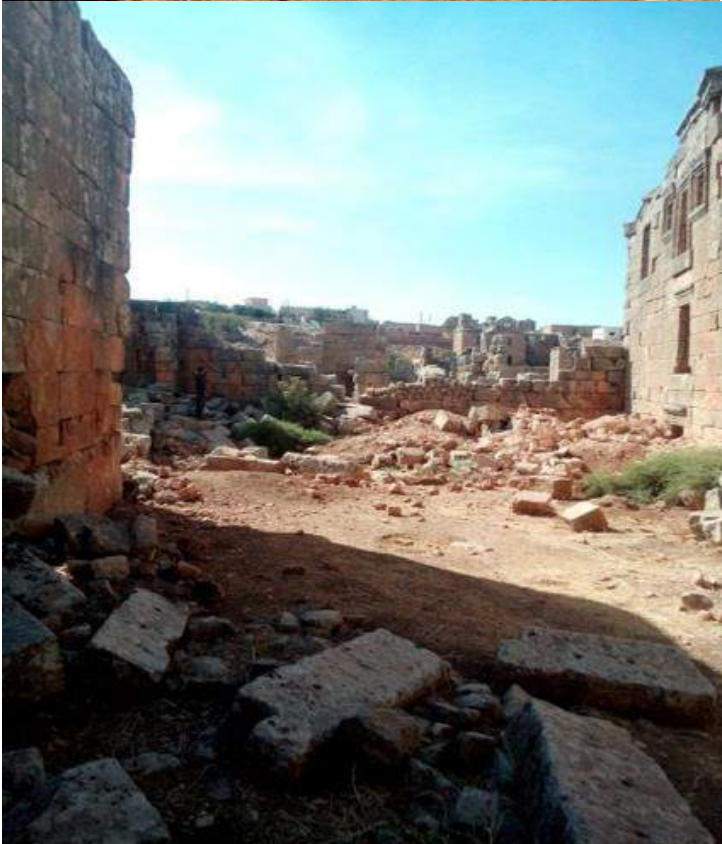
Damage caused by vegetation
