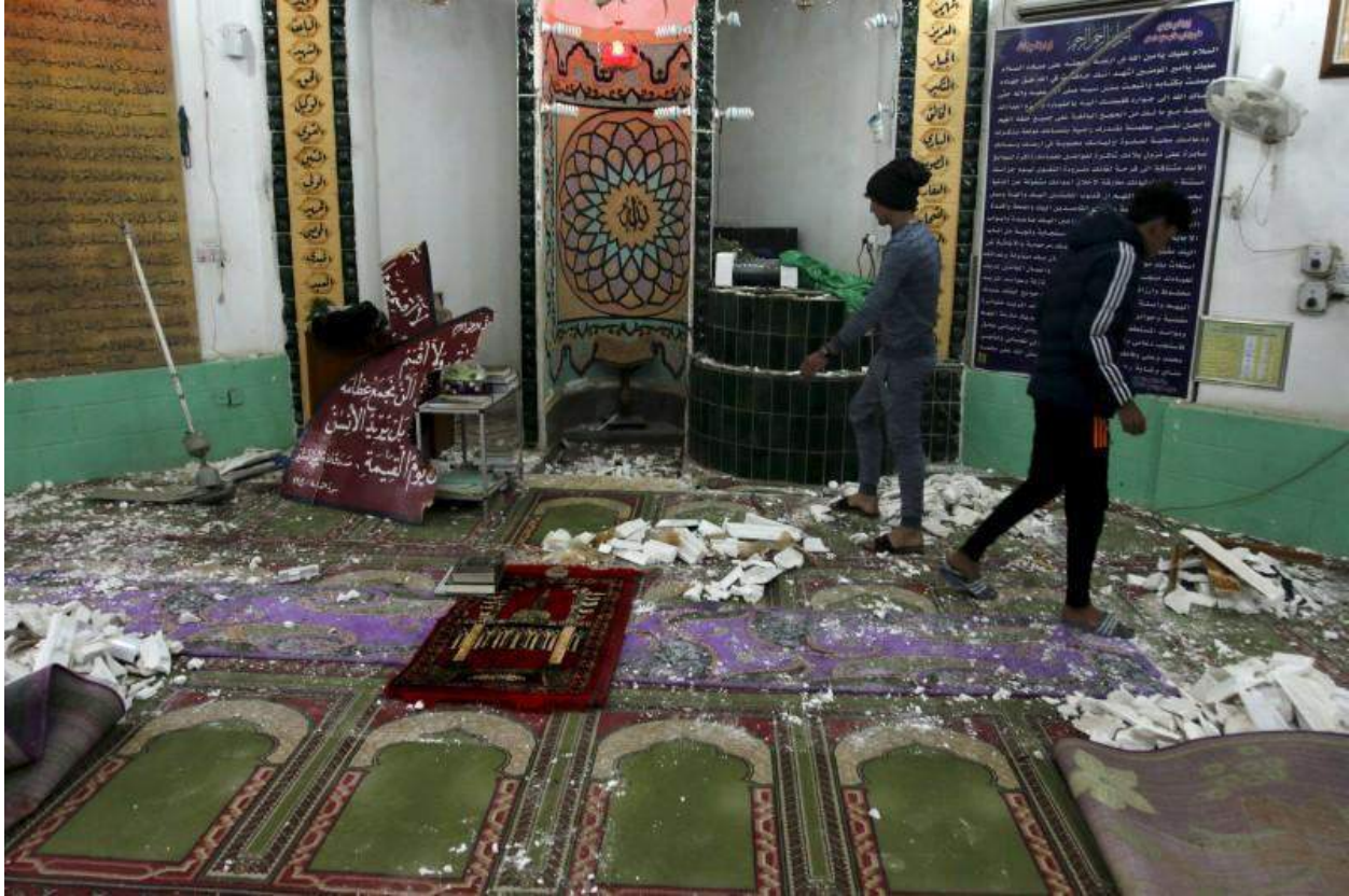
Interior of Rasul al-Azam Mosque showing material and structural damage (Reuters/Khalid al-Mousily; February 26, 2016)
