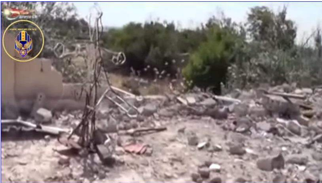
Close up of damage to Mar Bisho Church, Tel Shamiram (AINA; December 13, 2015)
