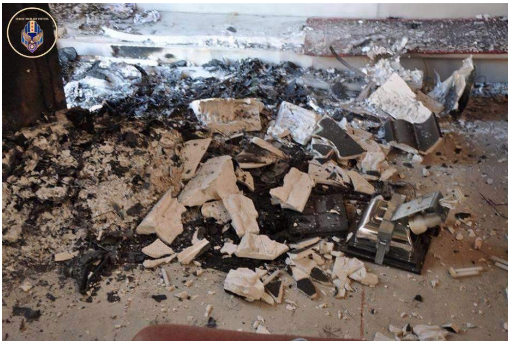
Damage to the interior of Mar Giorgis Church, Tel Maghas (AINA; March 16, 2015)
