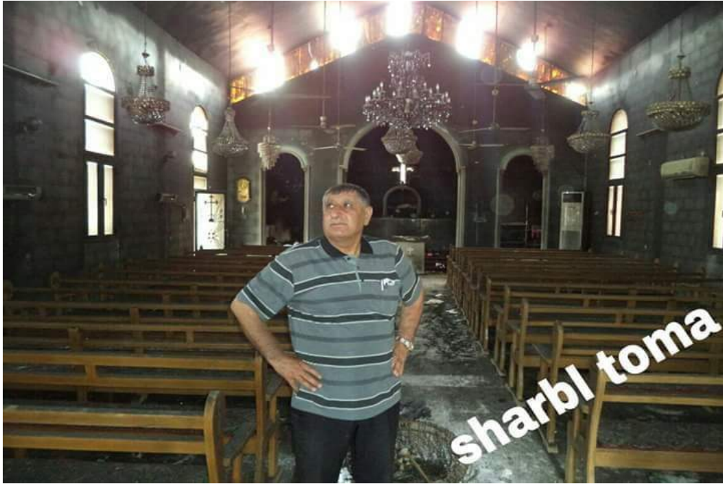
Damage to the interior of Mar Giorgis and Mar Shimon Prusbai Church, Tel Balua (Halmon.net; Posted June 5, 2015)
