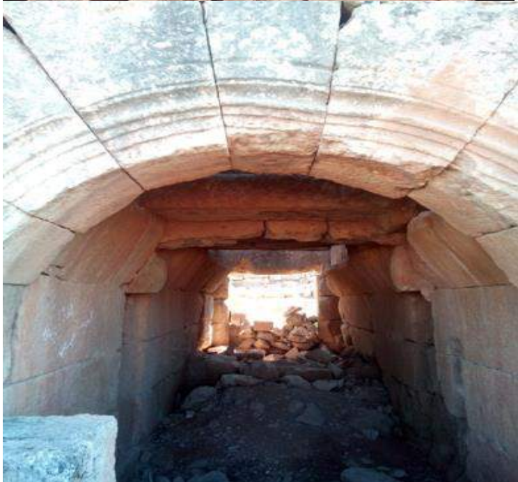
Damage caused by neglect
