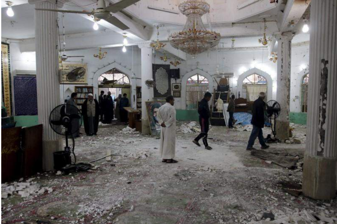
Interior of Rasul al-Azam Mosque showing material and structural damage (Reuters/Khalid al-Mousily; February 26, 2016)
