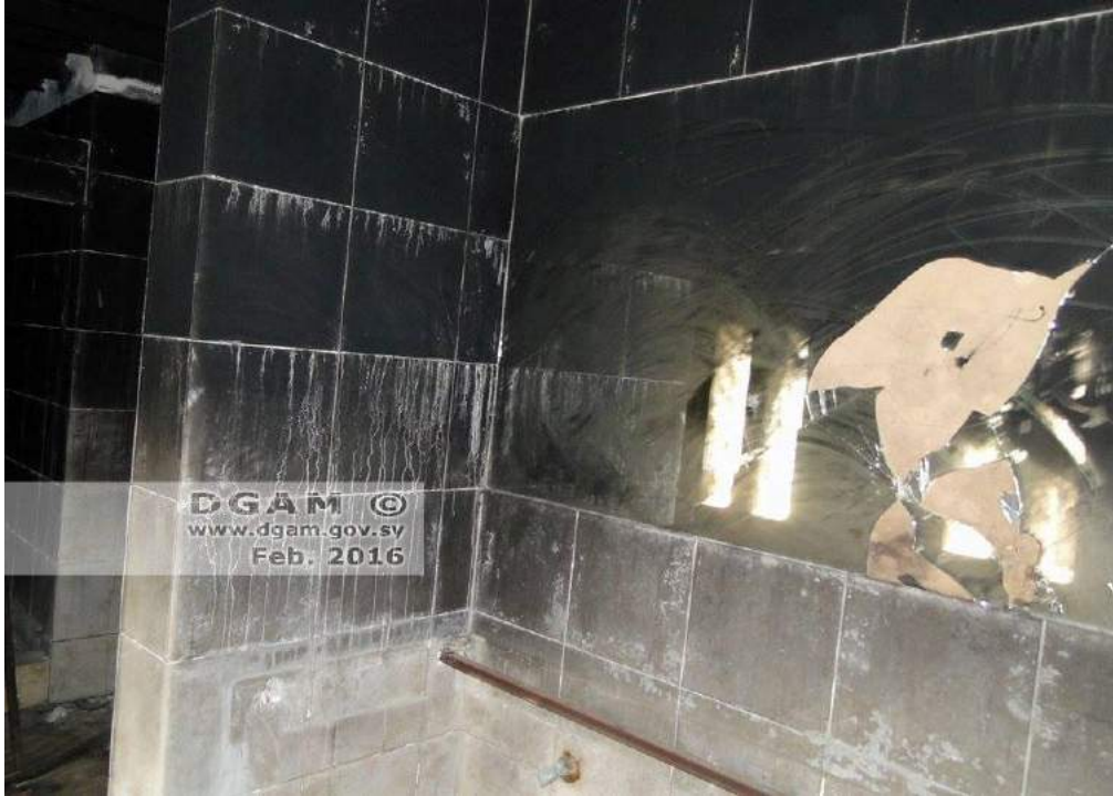
Fire damage in visitor center restroom (DGAM; February 16, 2016)
