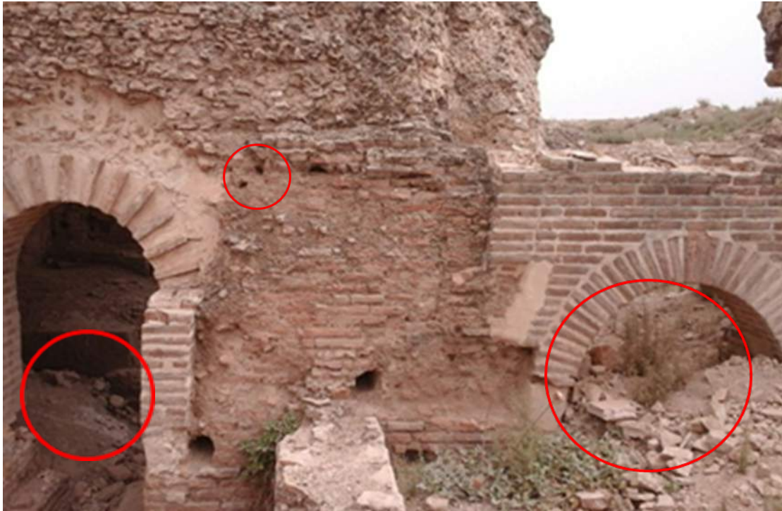
Damage sustained due to regime forces military operations
