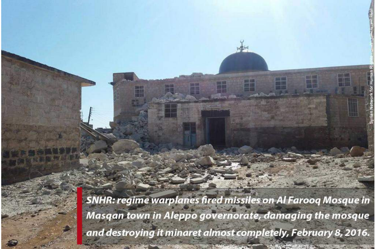
Damage to Al Farooq Mosque (SNHR; February 8, 2016)
