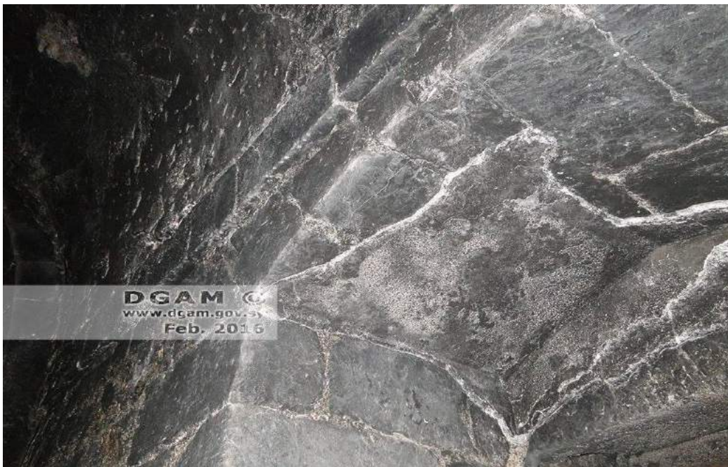
Fire damage to Ayyubid mosque (DGAM; February 16, 2016)
