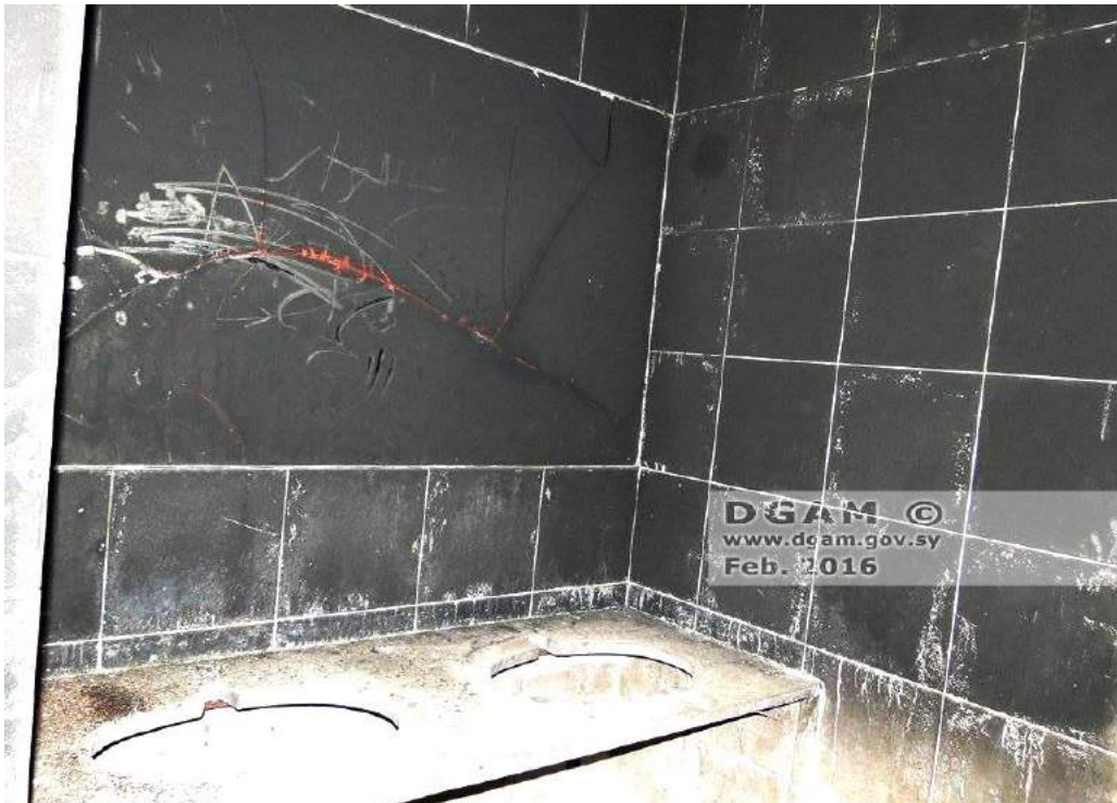
Fire damage and vandalism in the visitor center bathroom (DGAM; February 16, 2016)
