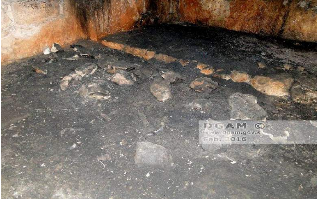
Fire damage to Ayyubid mosque (DGAM; February 16, 2016)
