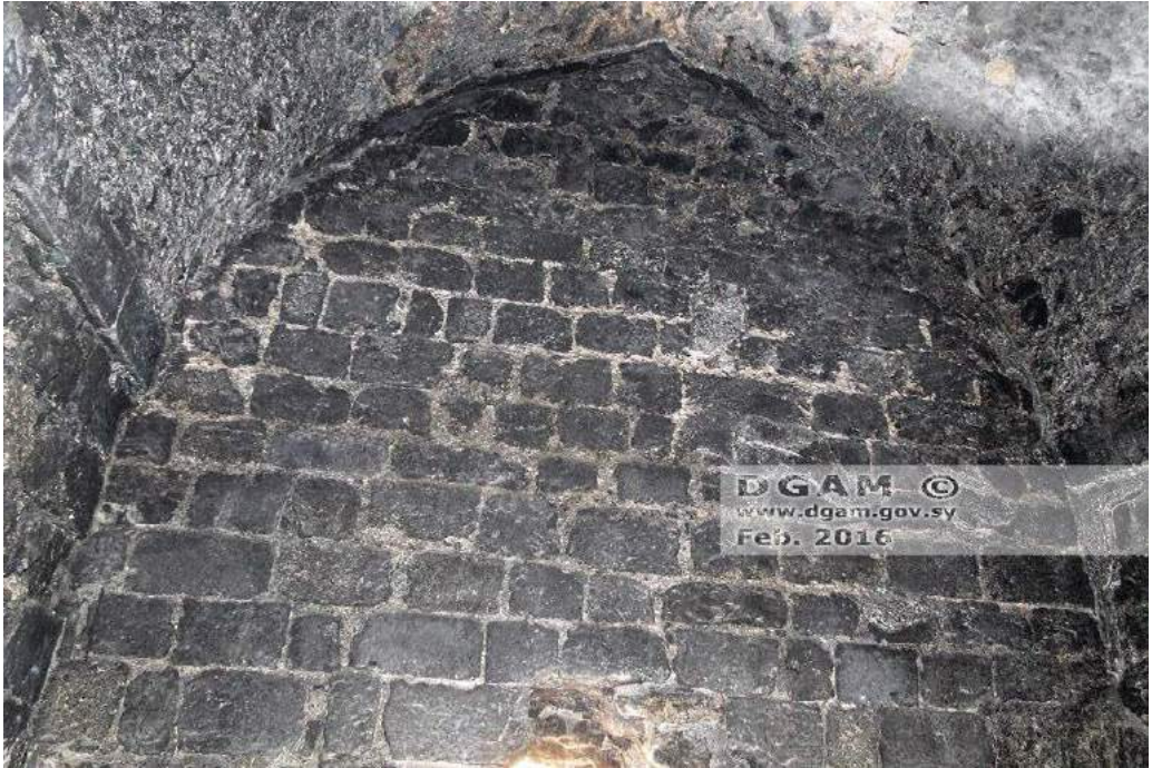
Fire damage to Ayyubid mosque (DGAM; February 16, 2016)
