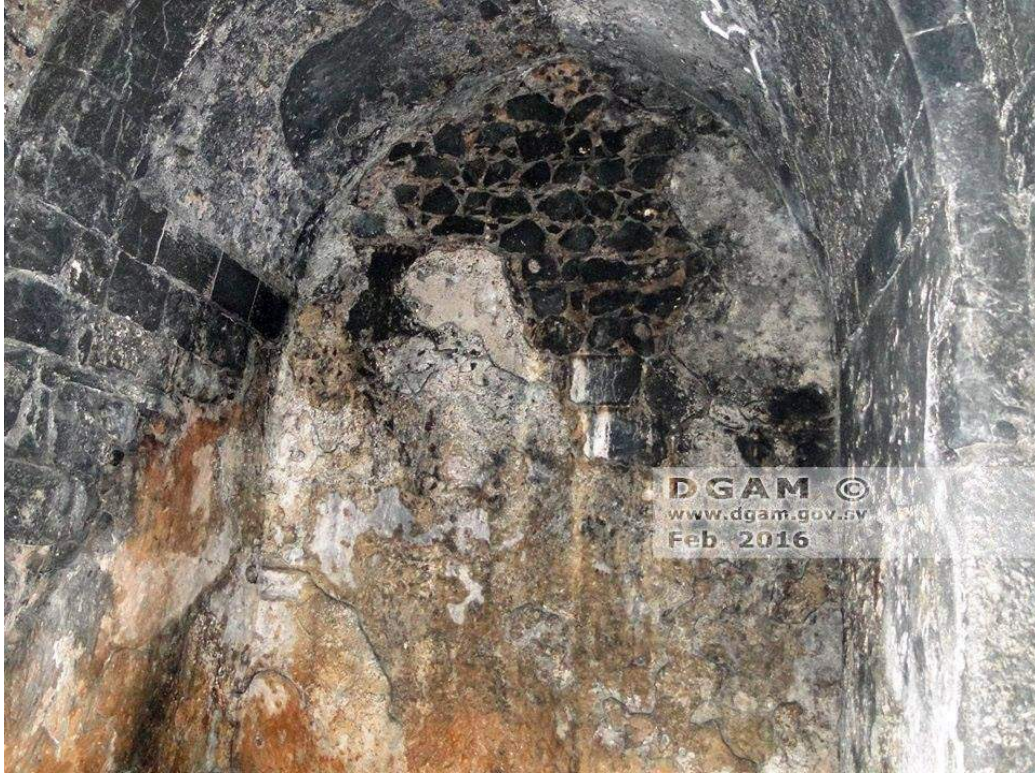
Fire damage to Ayyubid mosque (DGAM; February 16, 2016)
