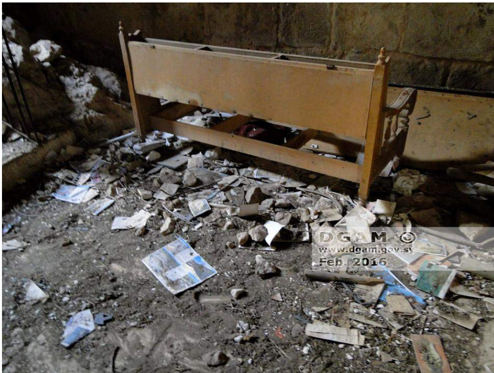
Damage and debris in the visitor center (DGAM; February 16, 2016)
