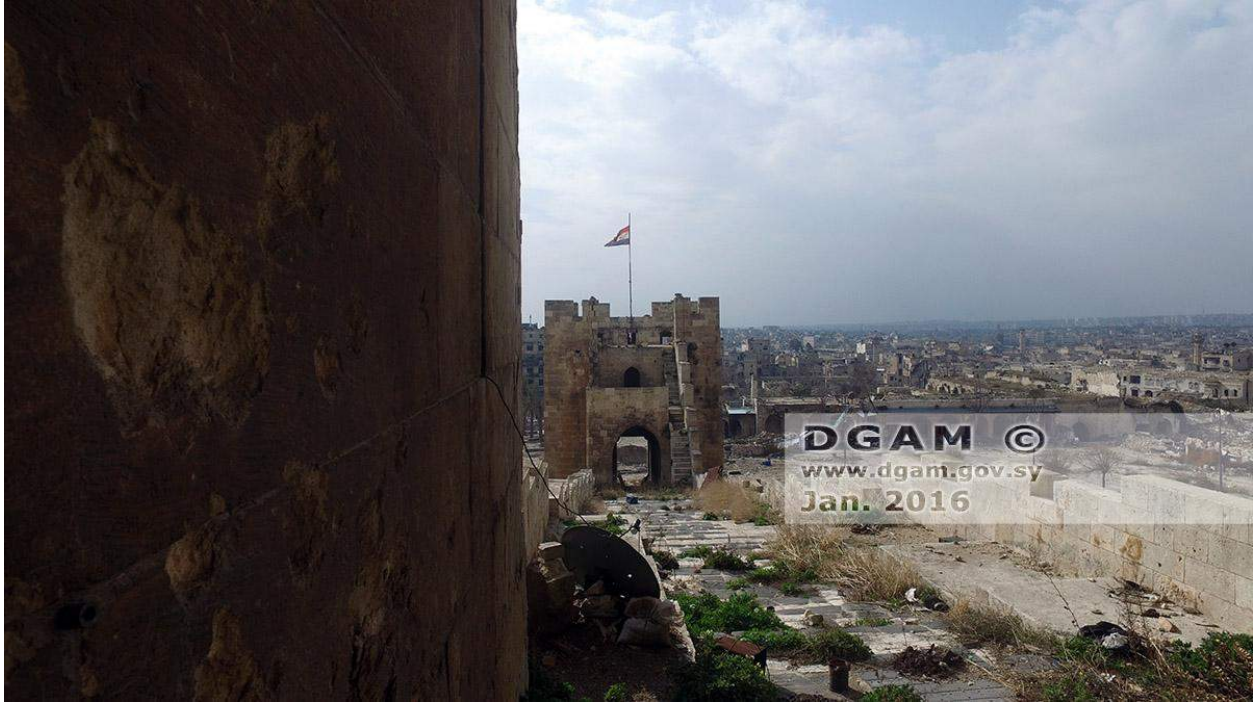
Shelling damage and debris on citadel bridge (DGAM; published February 15, 2016)
