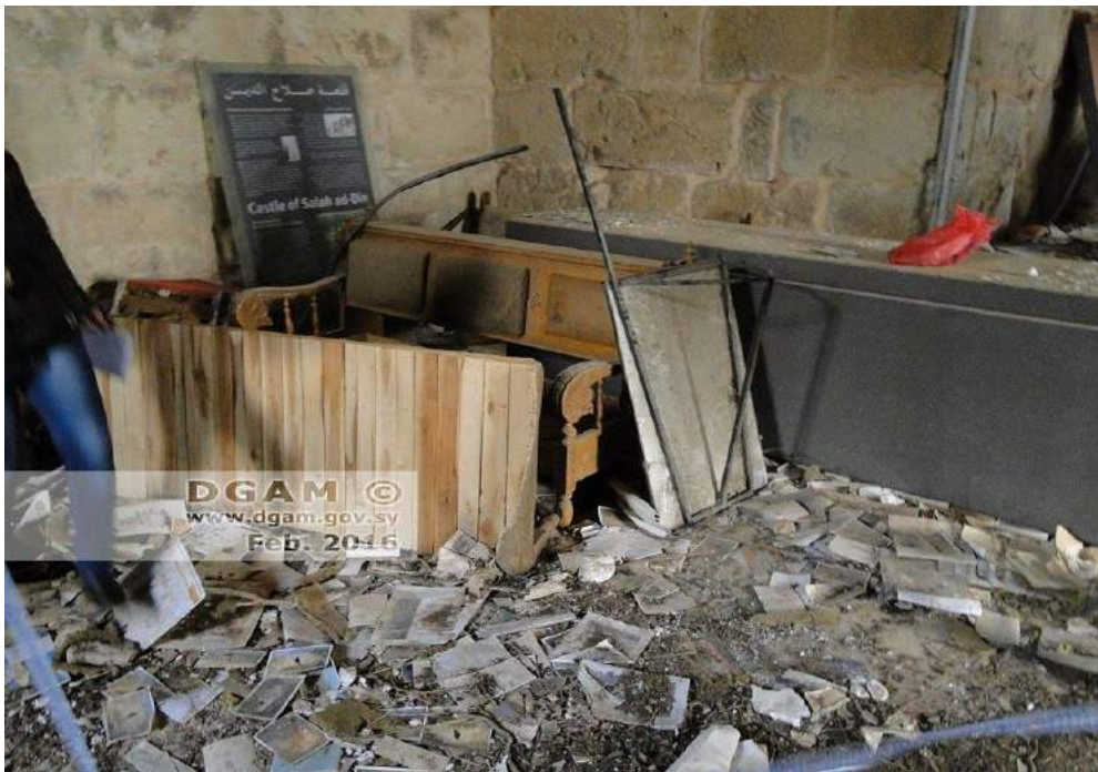
Damage and debris in the visitor center (DGAM; February 16, 2016)
