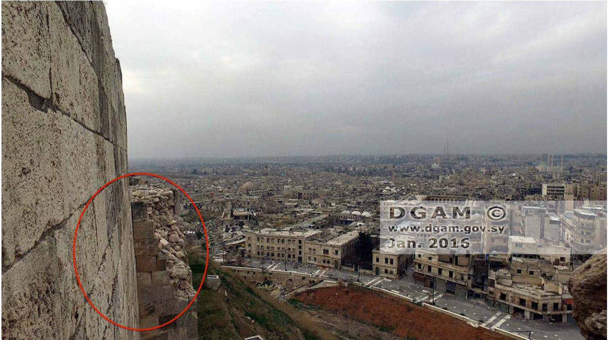
Damage to portion of western wall of Citadel (DGAM; published February 15, 2016)
