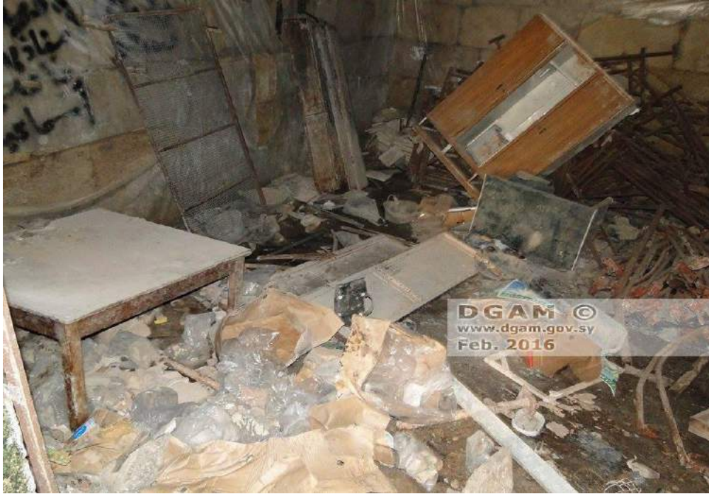
Damage, vandalism, and debris in the visitor center (DGAM; February 16, 2016)
