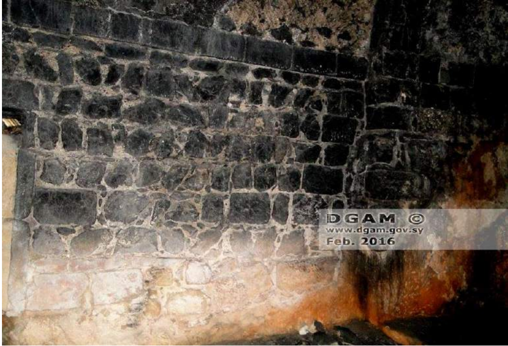
Fire damage to Ayyubid mosque (DGAM; February 16, 2016)
