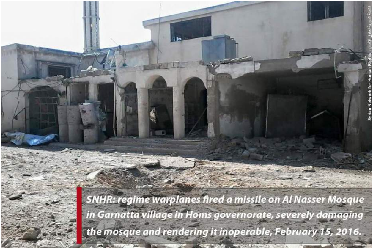
Damage to al-Nasr Mosque (SNHR; February 15, 2016)
