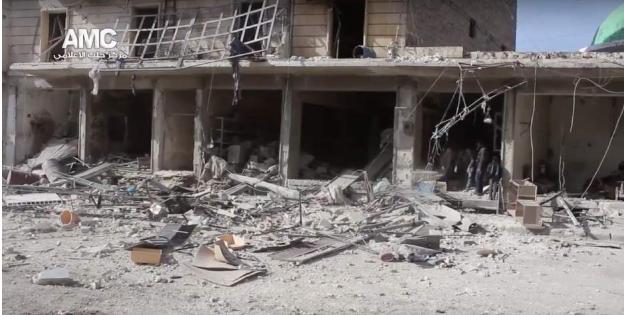
Damage to Khayrat Mosque and adjacent building (Aleppo Media Center; February 5, 2016)
