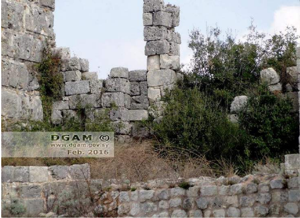
Overgrown vegetation (DGAM; February 16, 2016)
