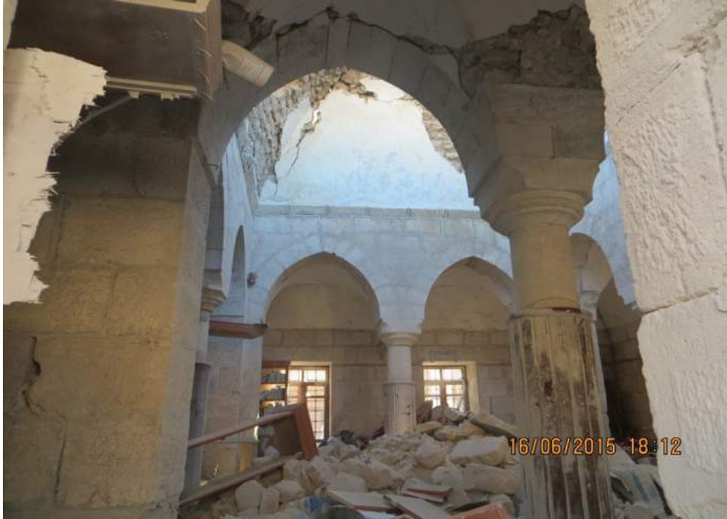
Partial collapse of al-Takkiyah. Represented by the total collapse of the ceiling and great damage of the walls. Keep in mind that al-Takkiyah contains the Al-I'layah Library.
