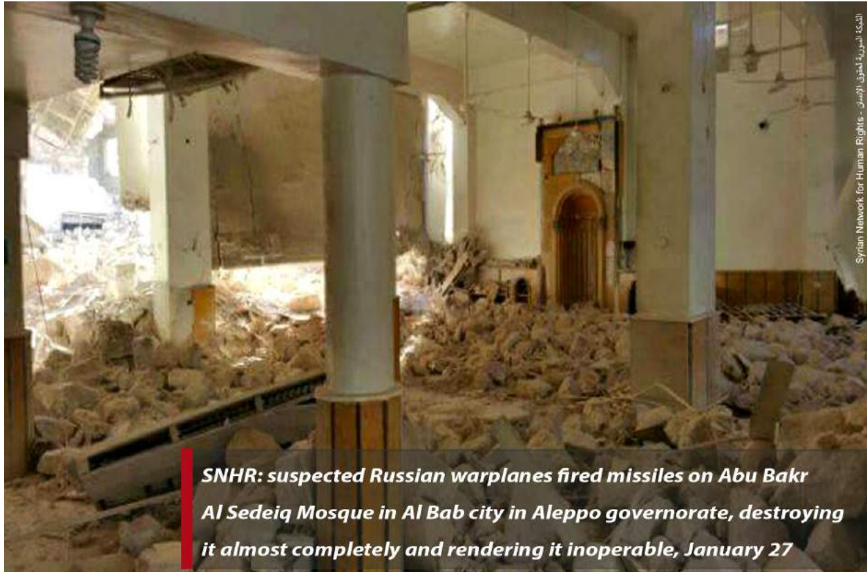
Abu Bakr Al Sedeiq Mosque showing extensive damage (Syrian Network for Human Rights; January 28, 2016)
