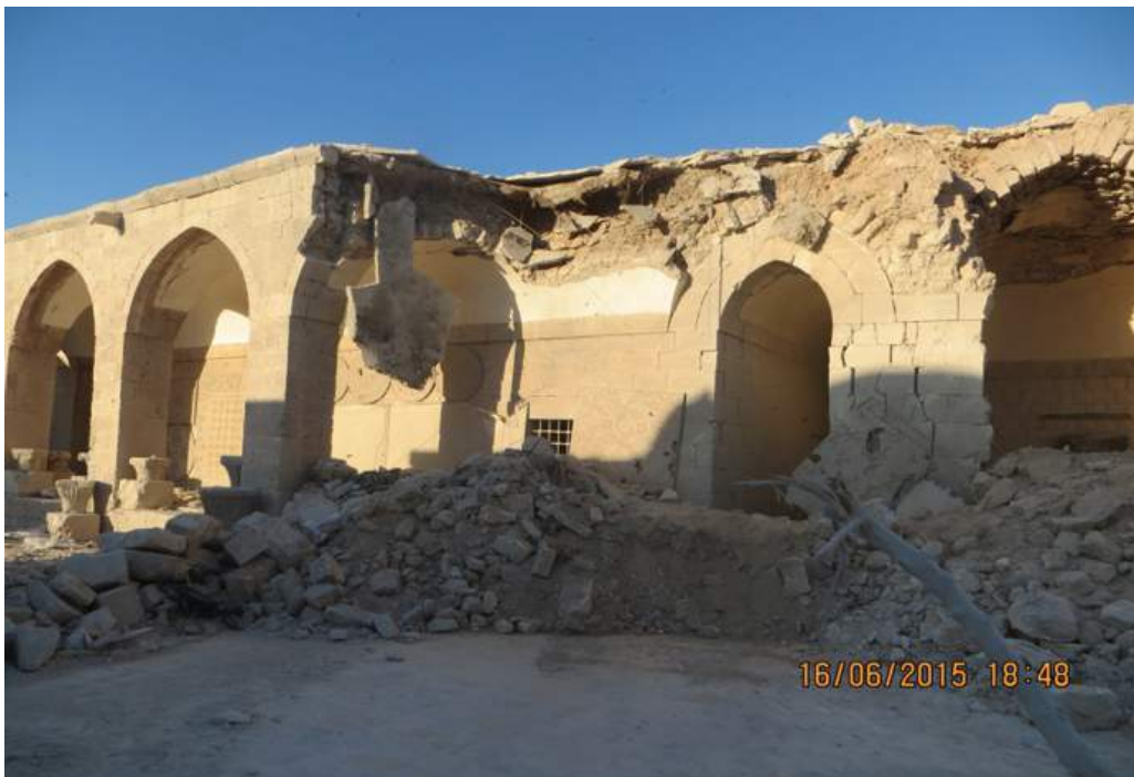
The eastern front is greatly damaged and in need of immediate repair.
