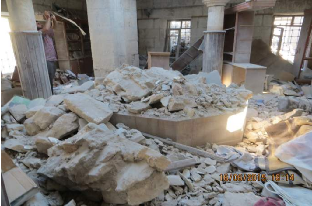
A partial collapse of the halls in the first and second wings, as well as a room used as an office:
