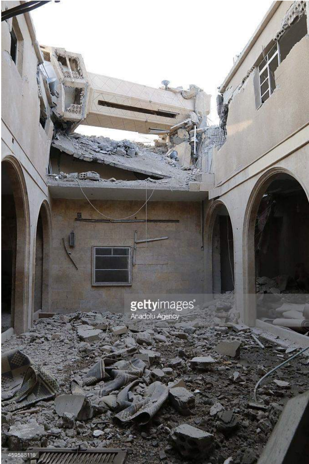
Collapse of Hinni Mosque minaret and roof damage (Anadolu Agency Getty Images; November 26, 2014)
