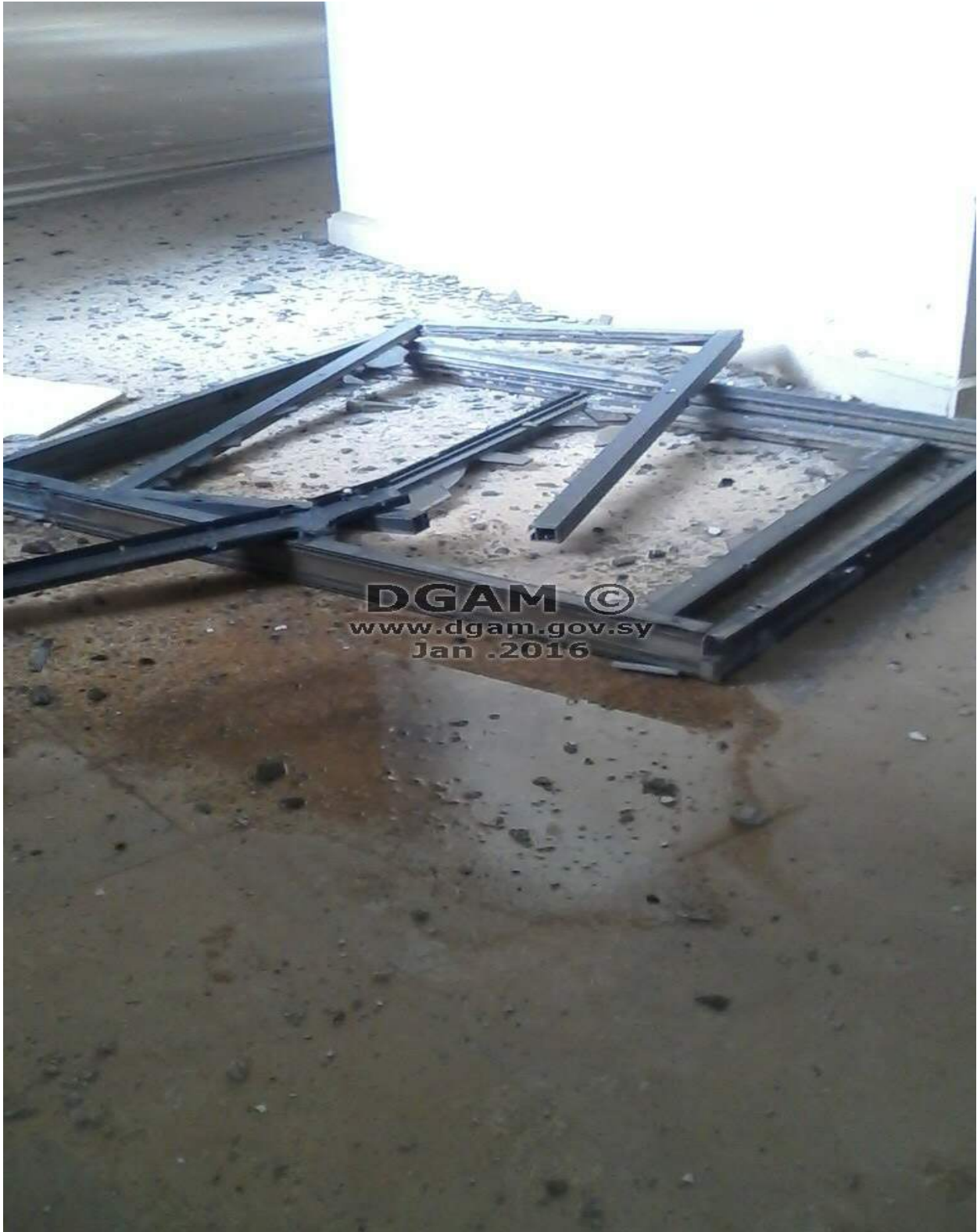
Mortar damage to Daraa Museum windows (DGAM; January 20, 2016)
