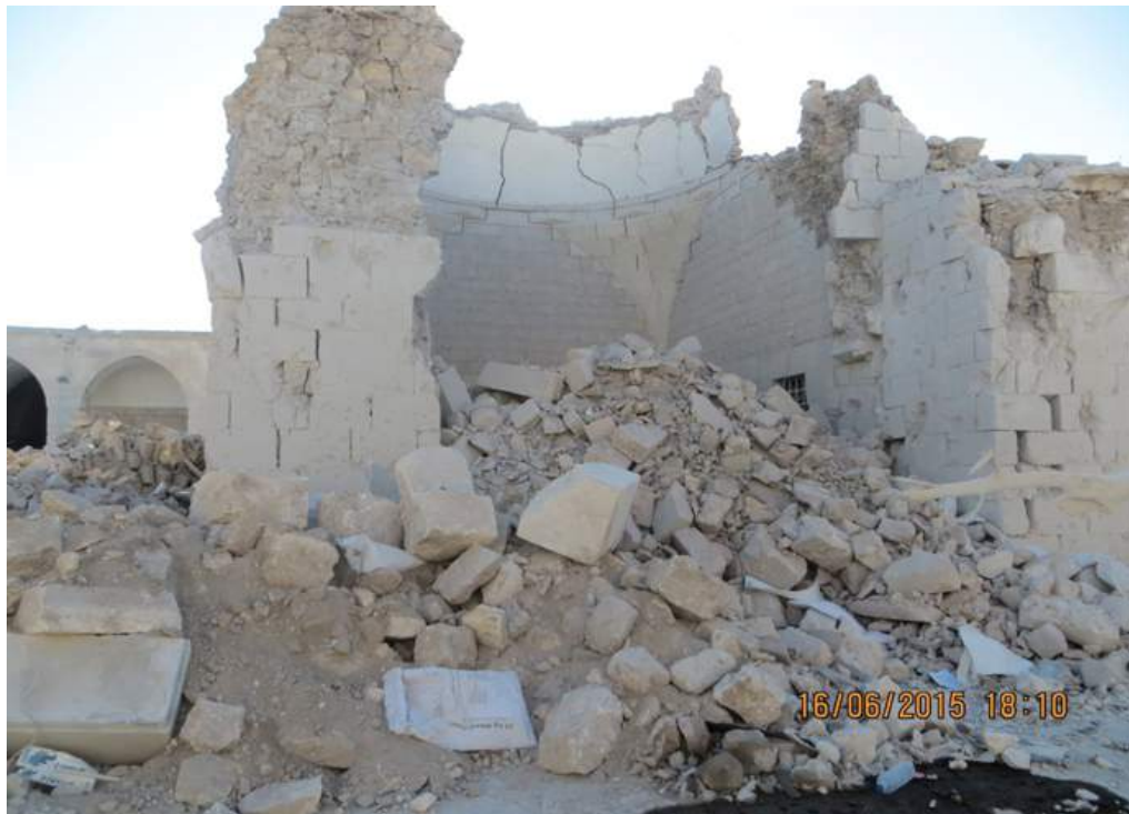
The complete collapse of the mosque. The ceiling and the eastern side were completely destroyed and the southern front was partially damaged.
