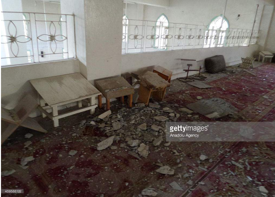
Interior damage to Hinni Mosque (Anadolu Agency Getty Images; November 26, 2014)
