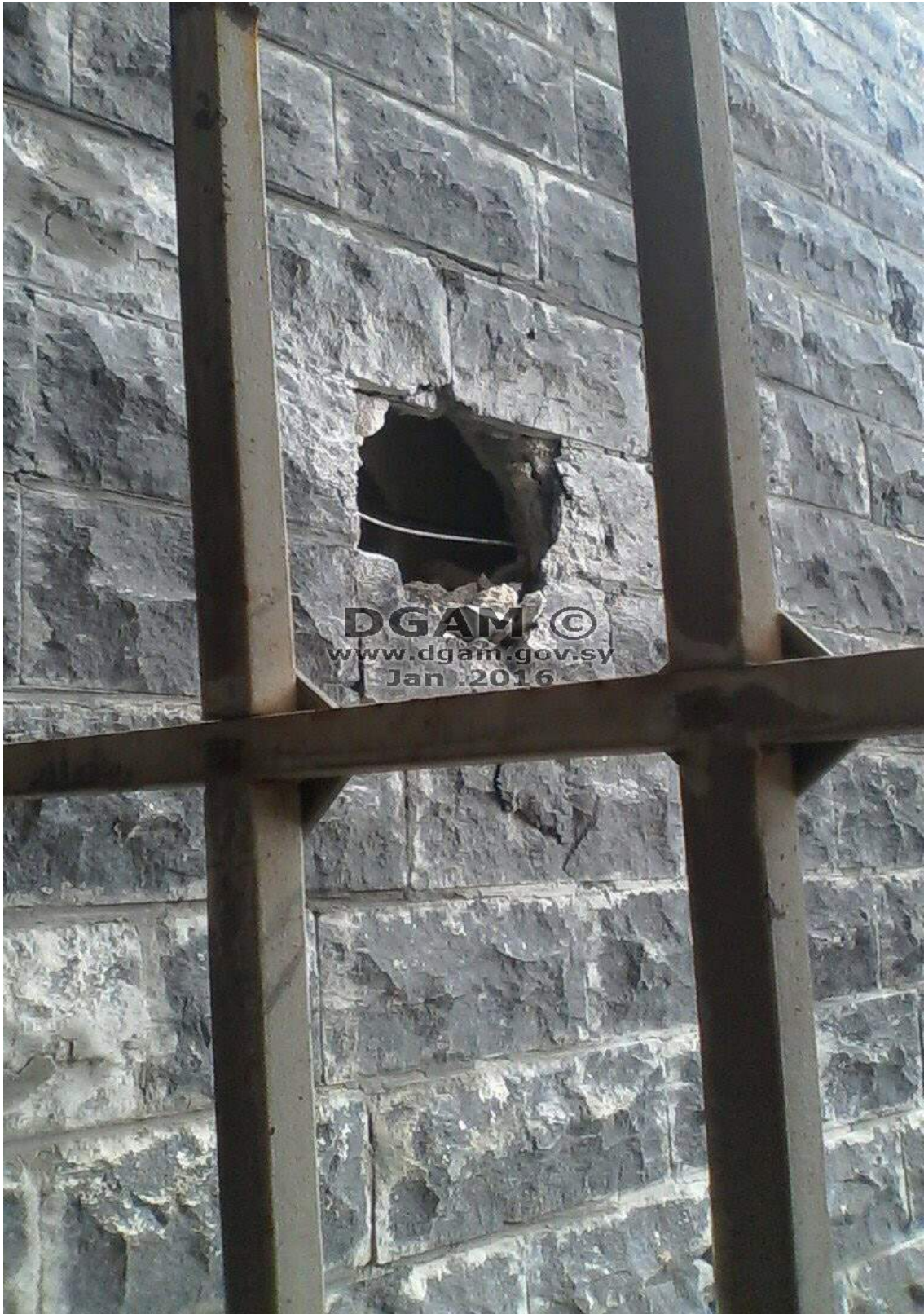
Mortar damage to Daraa Museum exterior (DGAM; January 20, 2016)
