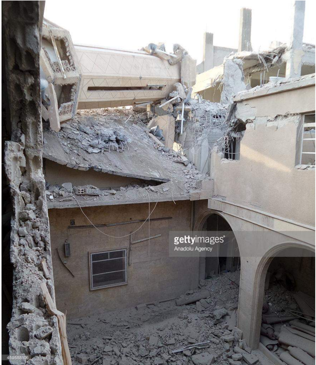
Collapse of Hinni Mosque minaret and roof damage (Anadolu Agency Getty Images; November 26, 2014)
