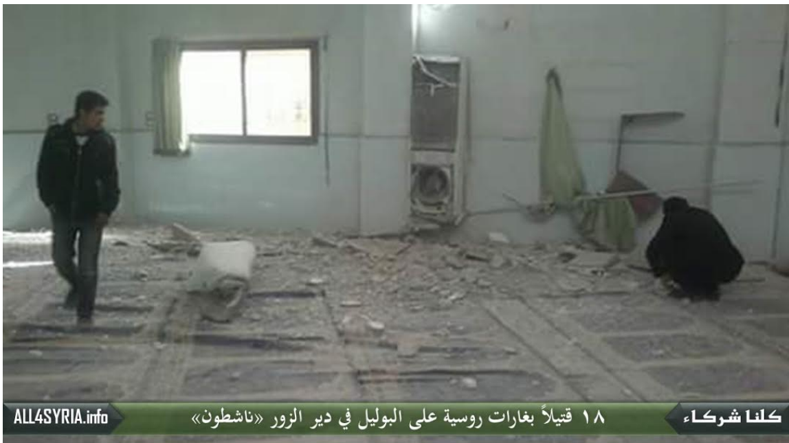
Damage to interior of Al Nour Mosque (All4Syria; January 19, 2016) 56
