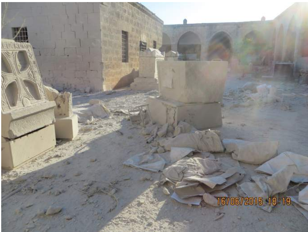
Sand bags scattered due to the explosion.
