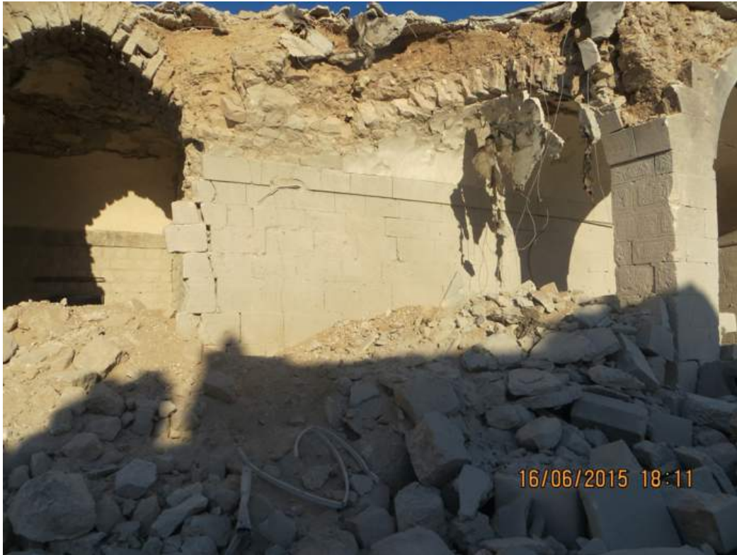
The eastern front is greatly damaged and in need of immediate repair.
