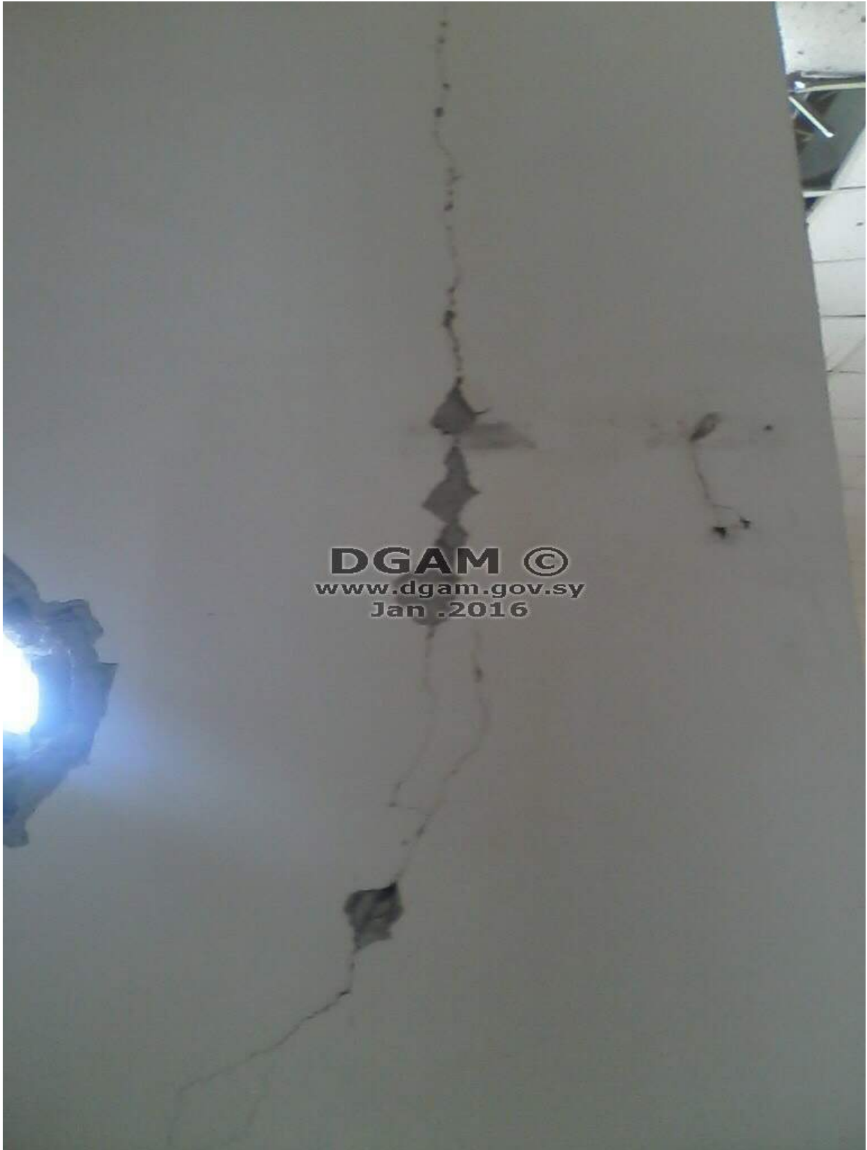
Mortar damage to Daraa Museum walls (DGAM; January 20, 2016)
