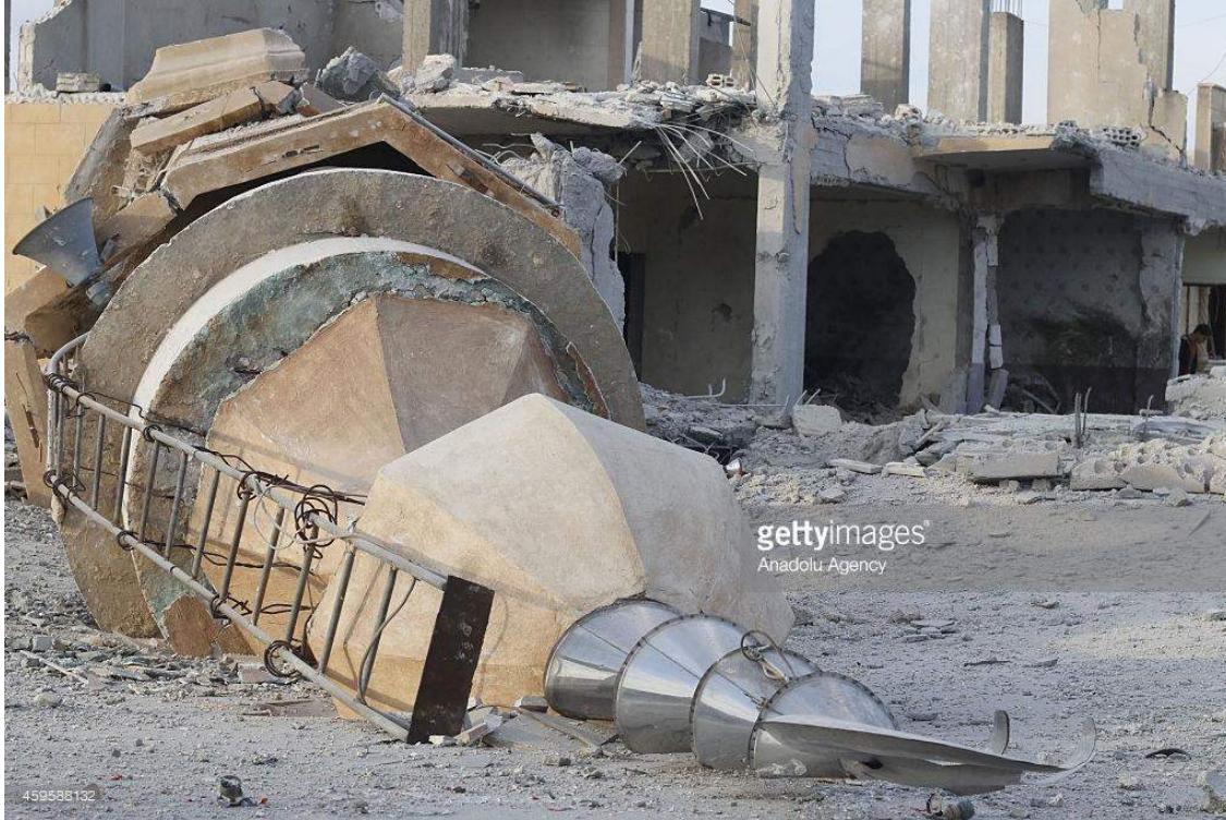
Collapse of Hinni Mosque minaret and roof damage (Anadolu Agency Getty Images; November 26, 2014)
