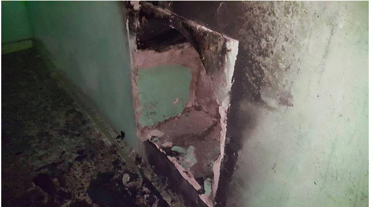
Damage to the interior of Imam Hassan Shrine (Arabic 21; January 24, 2015)
