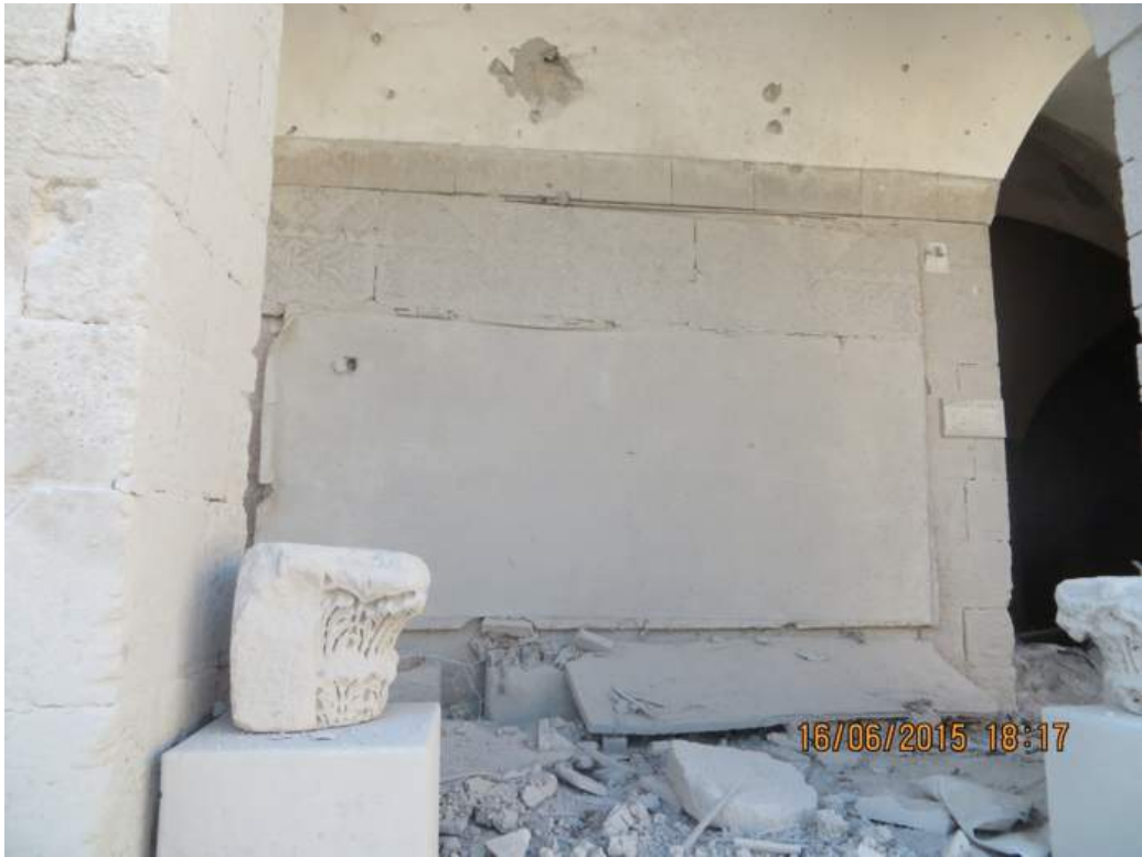
A tableau covered with a layer of glue and cloth after the fall of the sand bags.
