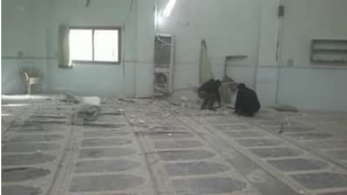
Damage to interior of Al Nour Mosque (Deir Ezzor is Being Slaughtered Silently; January 19, 2016) 55
