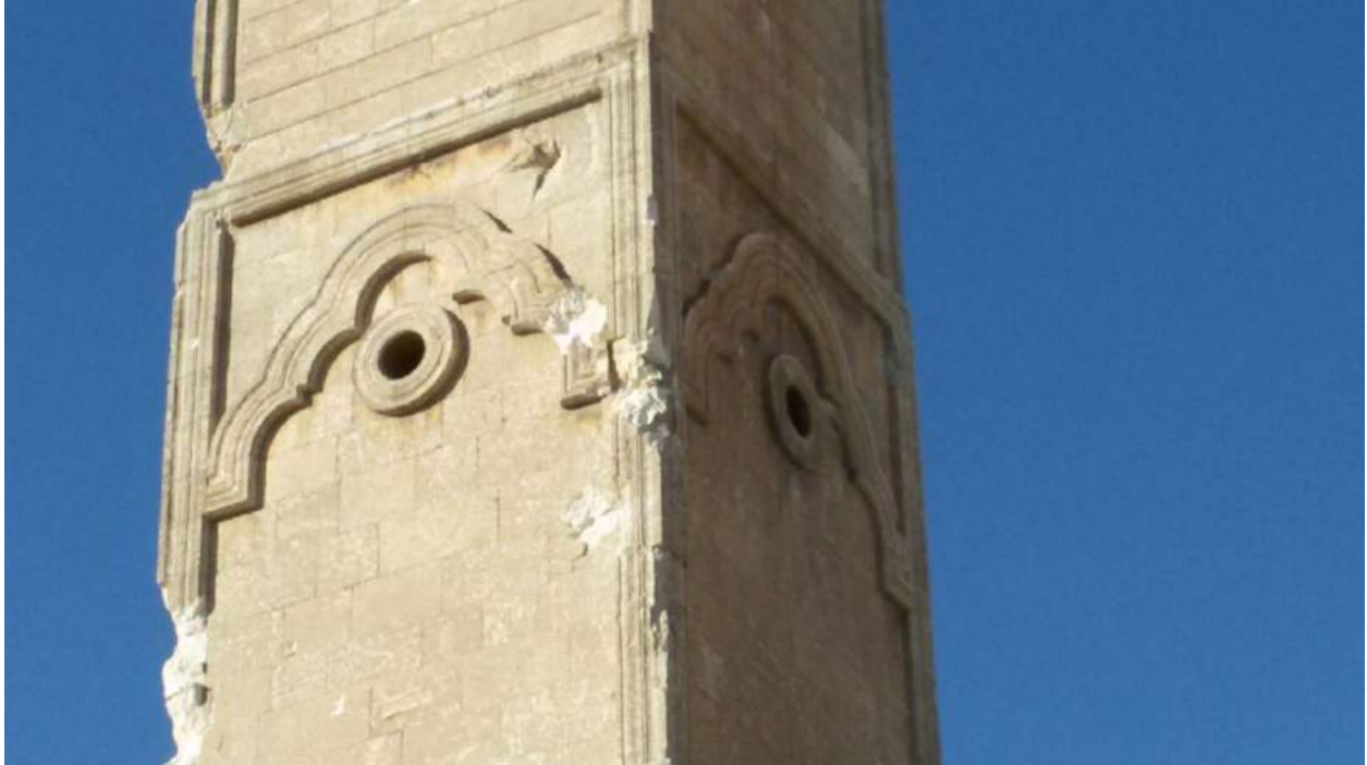
Damage to Maraat al-Numan minaret (ASOR CHI in-country sources; November 2, 2015)
