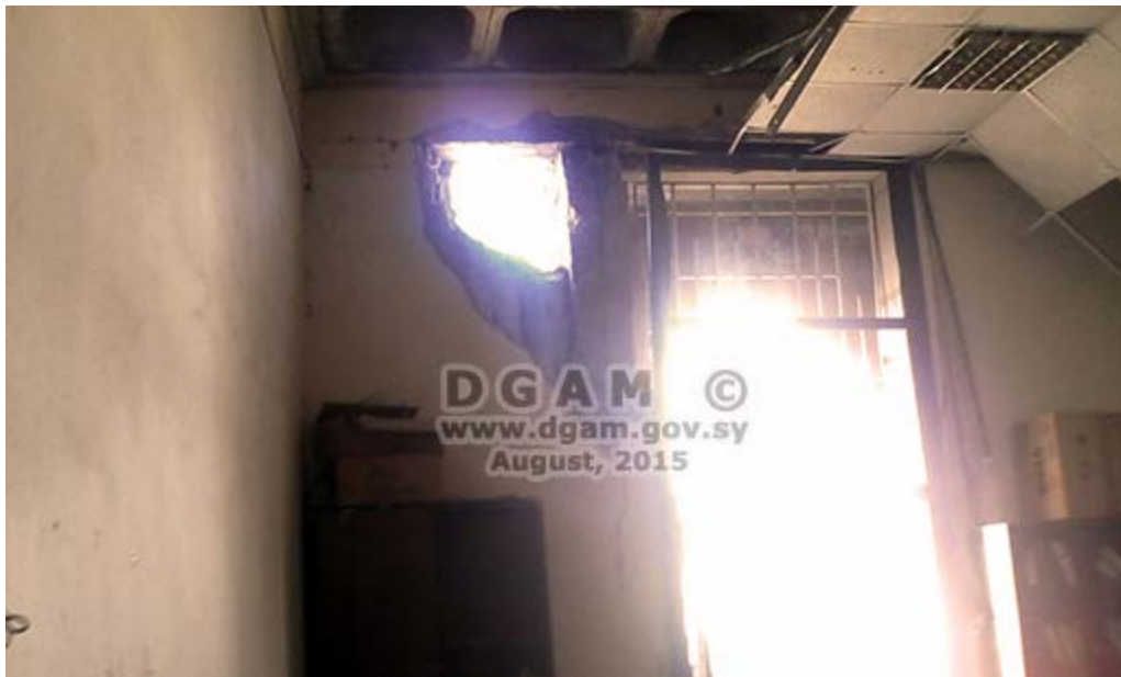
Museum of Daraa, interior damage (DGAM; August 12, 2015)
