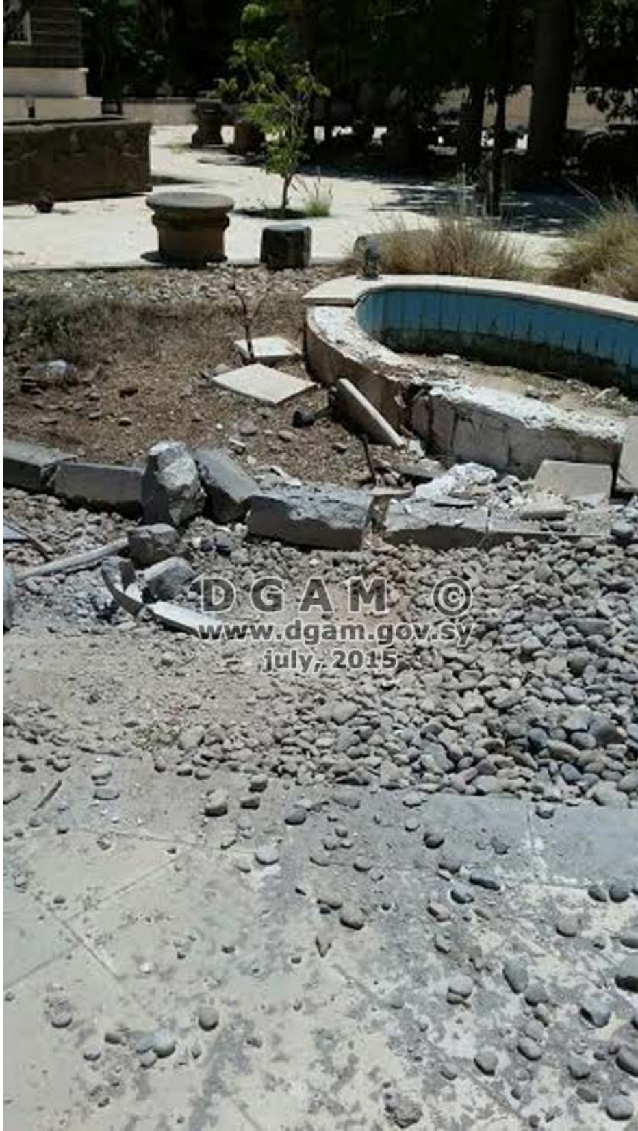
Museum of Daraa, exterior damage (DGAM; July, 3, 2015)
