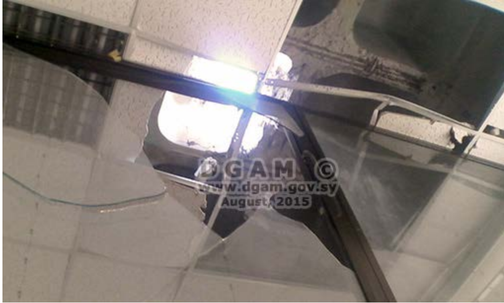
Museum of Daraa, interior damage (DGAM; August 12, 2015)
