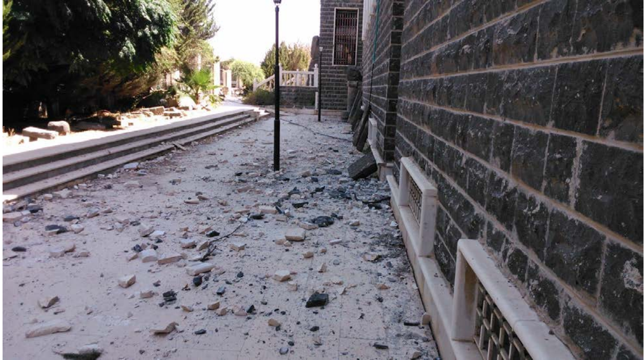
Museum of Daraa, exterior damage (Anonymous source; August 12, 2015)
