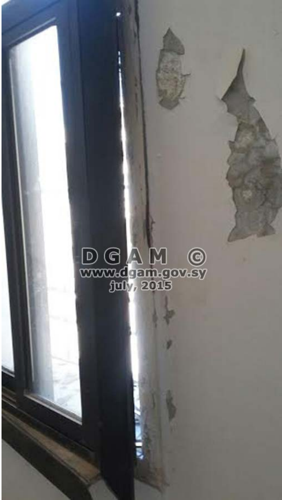
Museum of Daraa, interior damage (DGAM; July, 3, 2015)
