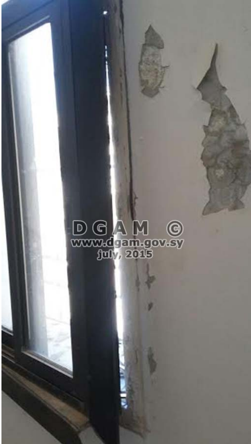
Museum of Deraa, interior damage (July 3, 2015; DGAM)
