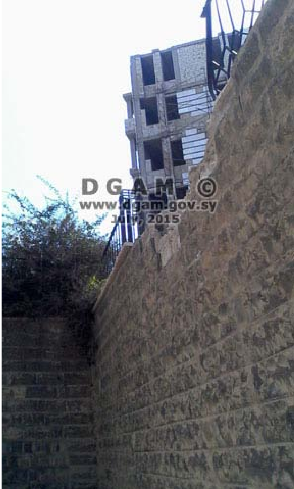
Museum of Deraa, exterior damage (July 30, 2015; DGAM)
