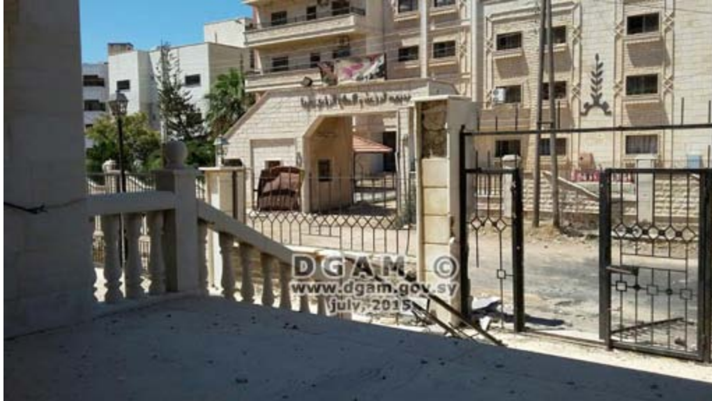
Museum of Deraa, exterior damage, (July 3, 2015; DGAM)
