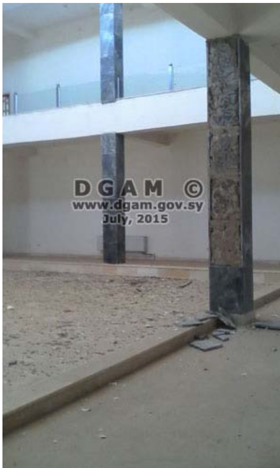
Museum of Deraa, interior damage (July 30, 2015; DGAM)
