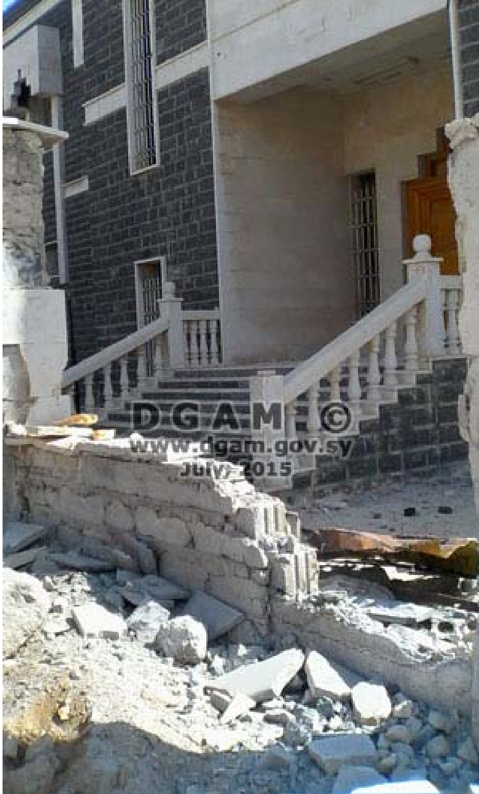
Museum of Deraa, exterior damage to the garden wall (July 30, 2015; DGAM)
