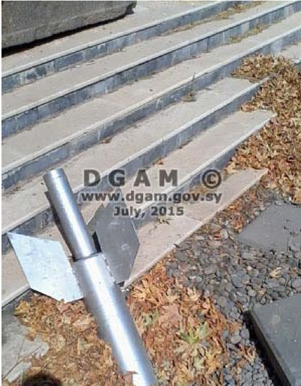
Museum of Deraa, exterior damage (July 30, 2015; DGAM)
