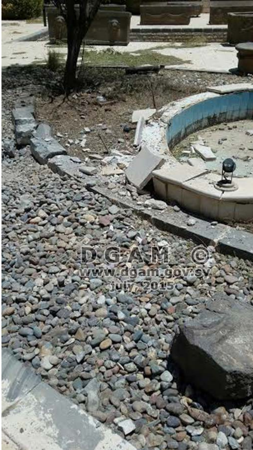
Museum of Daraa, exterior damage (DGAM; July 3, 2015)
