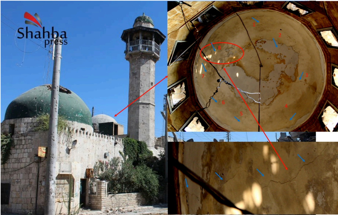
The current state of the Bardabak (Qastal al-Haramia) Mosque, Qastal al-Harami neighborhood, Aleppo (Shahba Press)
