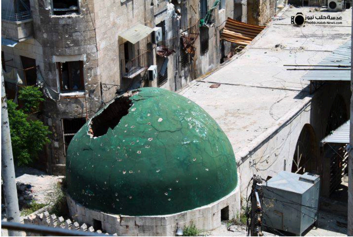
The current state of the Bardabak (Qastal al-Haramia) Mosque, Qastal al-Harami neighborhood, Aleppo (Halab News)
