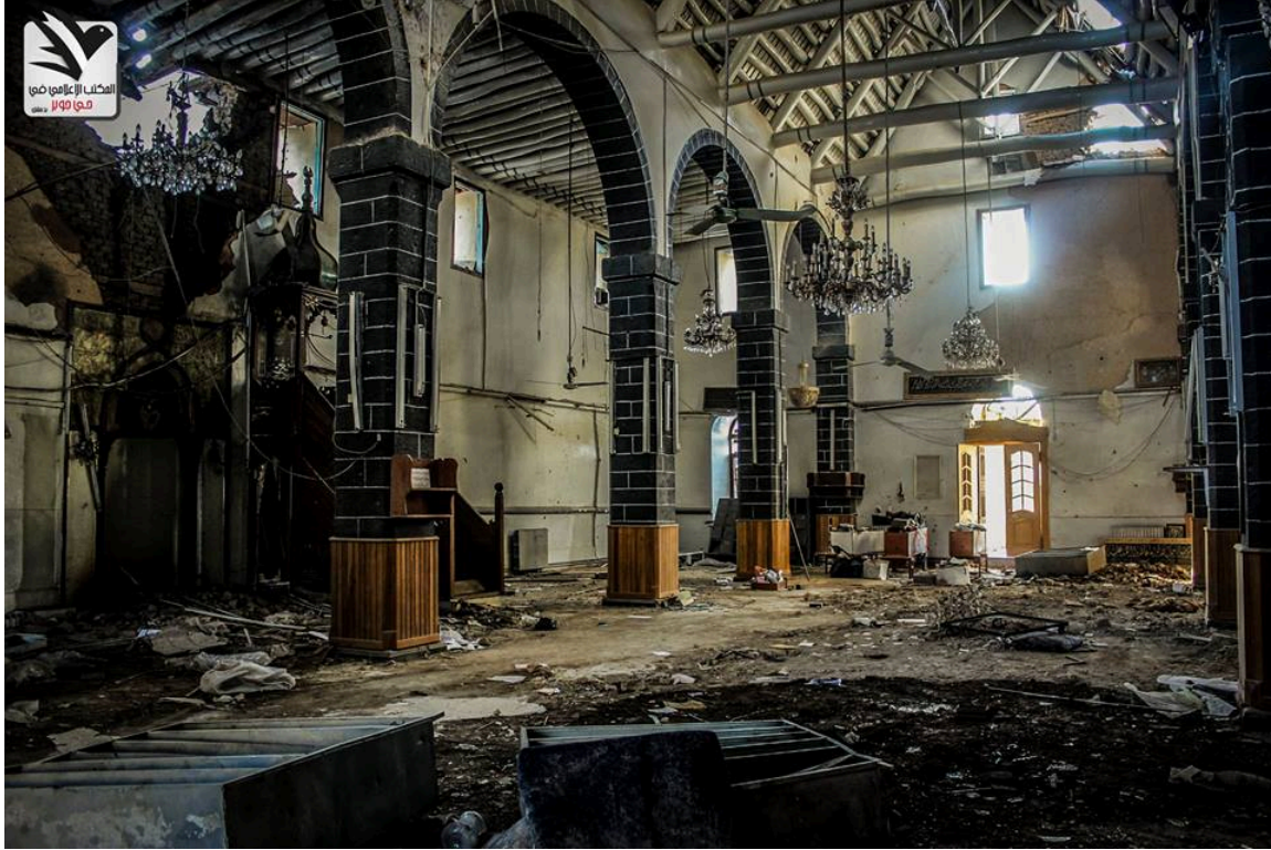
Image showing damage to Great Mosque of Jobar, interior (APSA)
