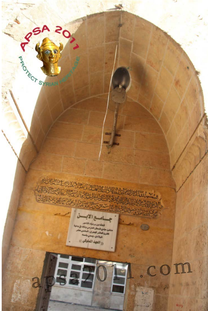
The current state of the al-Ibn Mosque, Qastal al-Harami neighborhood, Aleppo (APSA)
