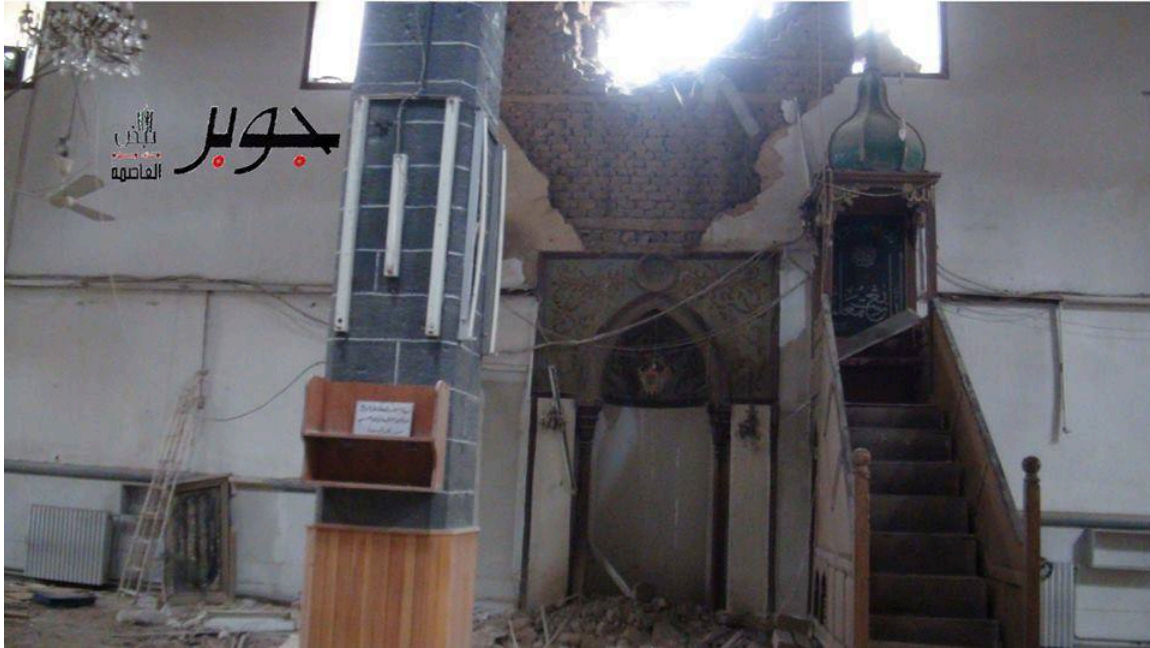
Image showing damage to Great Mosque of Jobar, interior (APSA)
