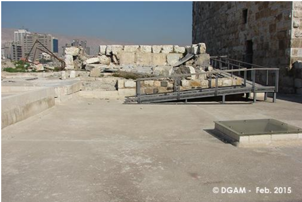
Damage to the Damascus Citadel Northwest Ayyubid Tower (DGAM)
