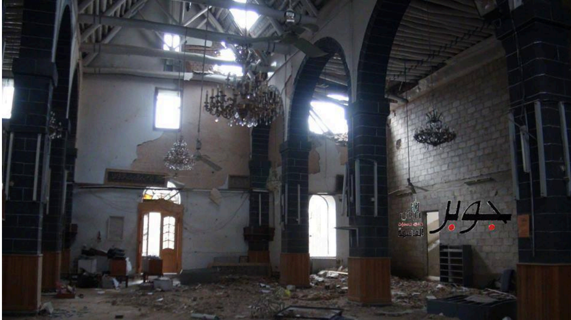
Image showing damage to Great Mosque of Jobar, interior (APSA)
