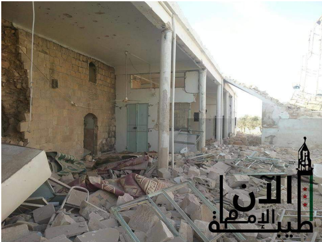
Destruction of the minaret and damage to al-Imam Mosque (APSA/Facebook; November 15, 2016)
