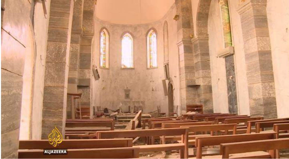
Video still of damage to the interior of Mart Shmone Church in Bashiqa (Al Jazeera, November 21, 2016)
