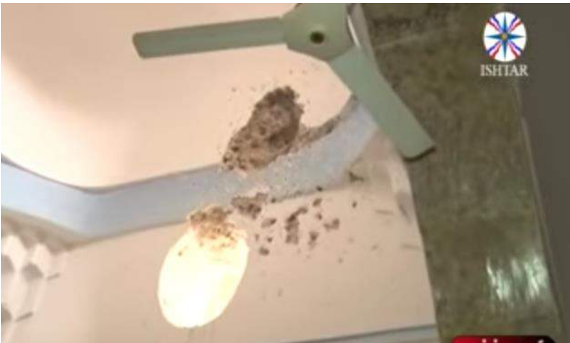
Video still of damage inside Mart Shmone Church in Bashiqa (Ishtar TV; November 11, 2016)
