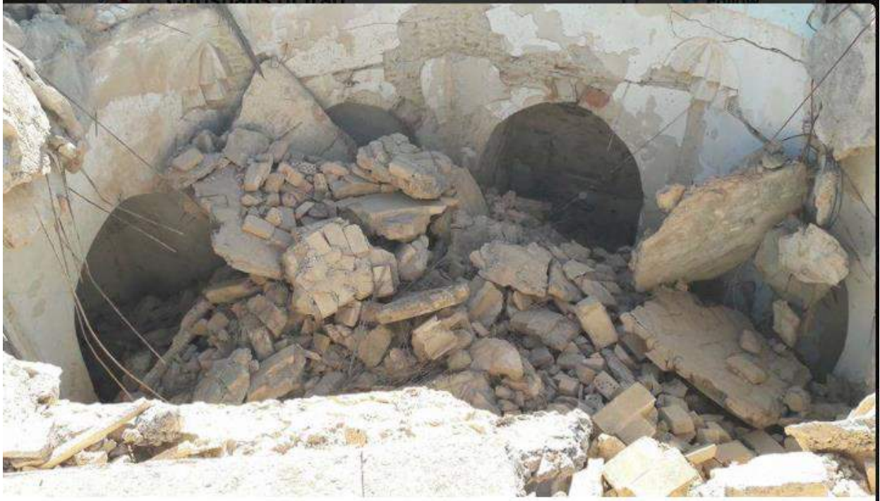
Collapsed roof of the Mar Behnam and Mart Sarah's Tombs (Christians of Iraq/Twitter; November 23, 2016)
