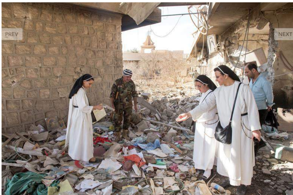
Dominican sisters of Saint Catherine de Sienne look through the damage to their convent (Thomas Goisque; November 20, 2016)
