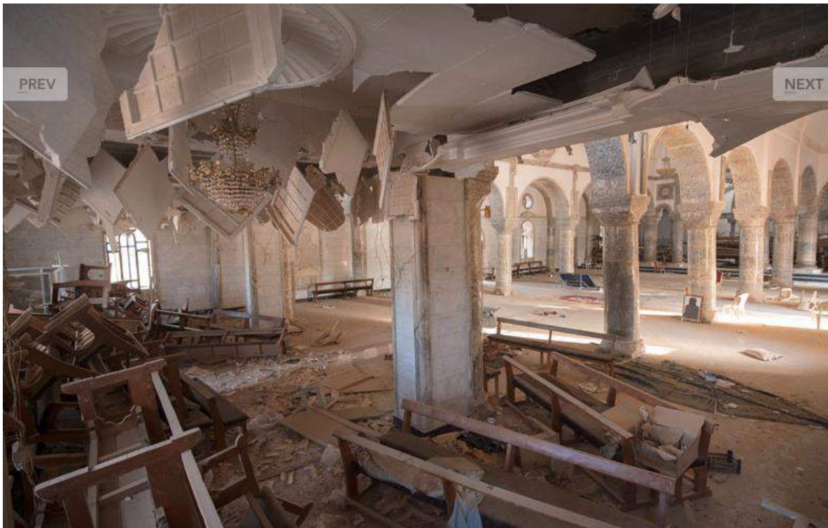
Damage to the inside of Mar Yohanna Church (Thomas Goisque; November 20, 2016)
