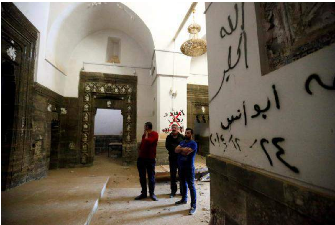
Damage and graffiti on the inside of Mar Behnam Monastery (Reuters; November 21, 2016)
