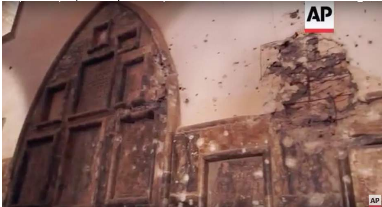
Video still of damage to the inside of al-Tahira Church (AP; November 17, 2016)
