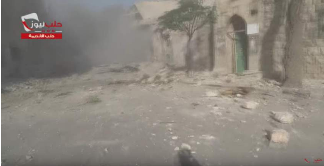
Video still of damage to an exterior wall of Barsin Mosque and surrounding area (SNHR/Youtube; November 17, 2016)
