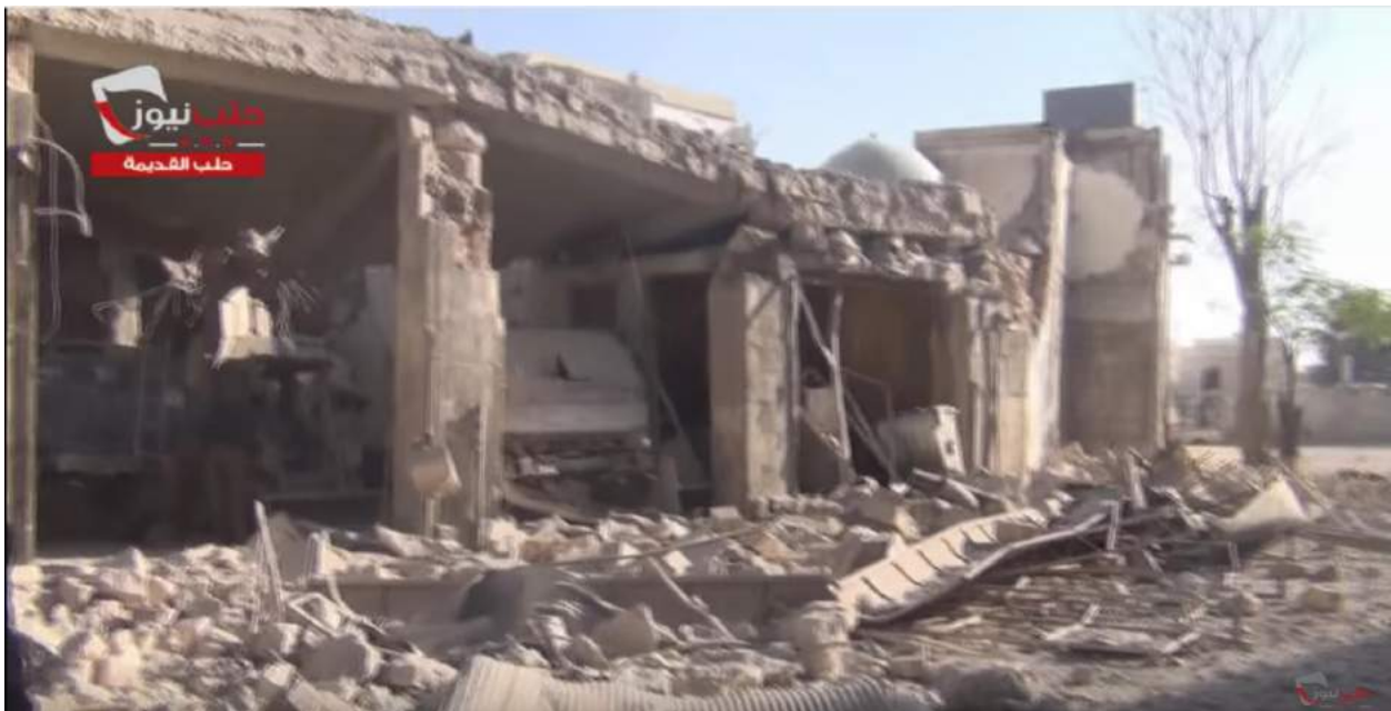
Video still of damage to the exterior of Barsin Mosque and surrounding area (SNHR/Youtube; November 17, 2016)
