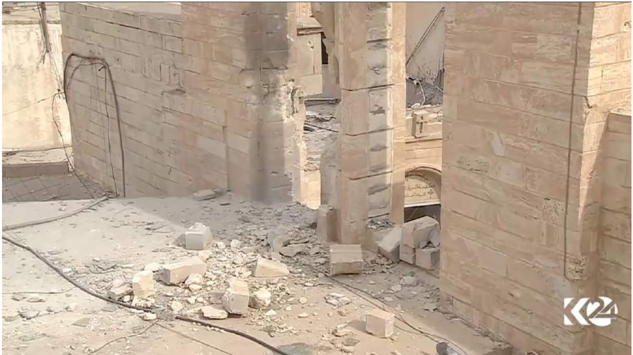
Video still of damage to Mart Shmone Church in Bashiqa (Kurdistan 24; November 10, 2016)
