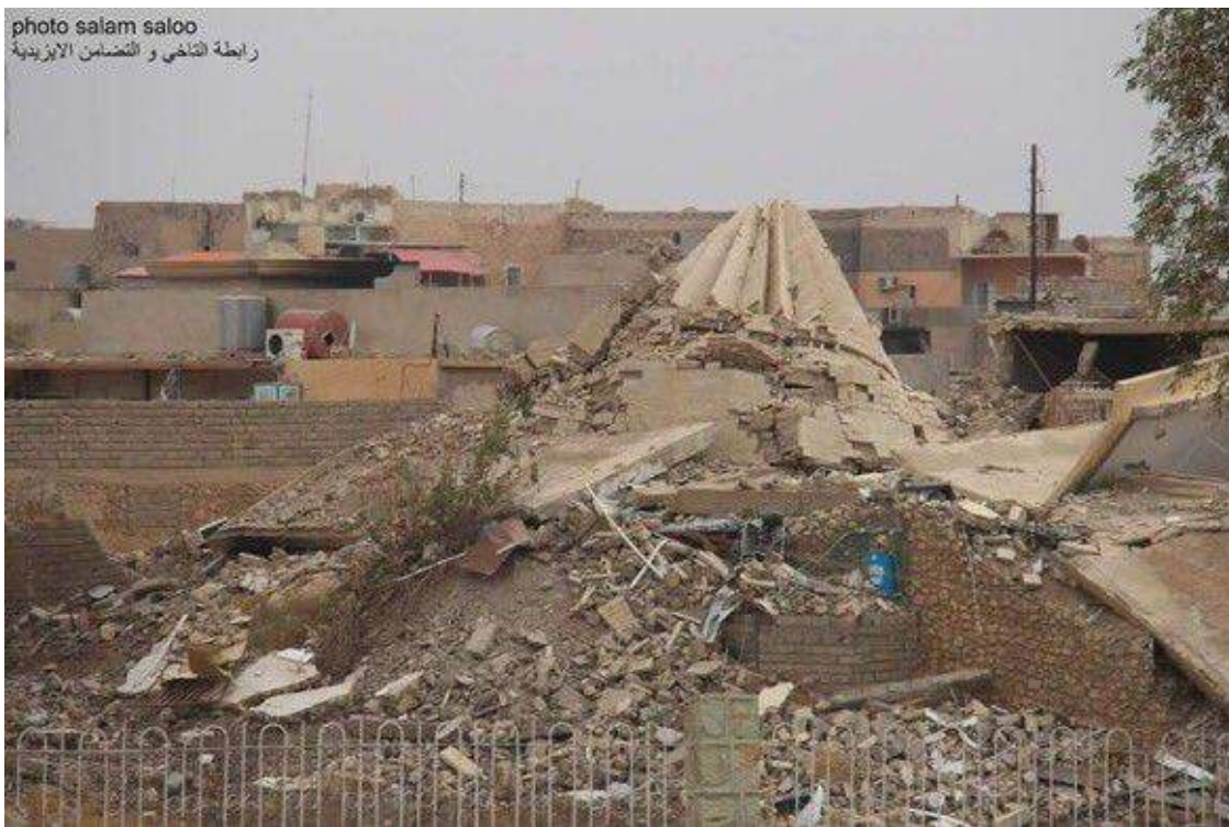
Damage to a Yezidi Shrine (Yezidi/Twitter: November 10, 2016)
