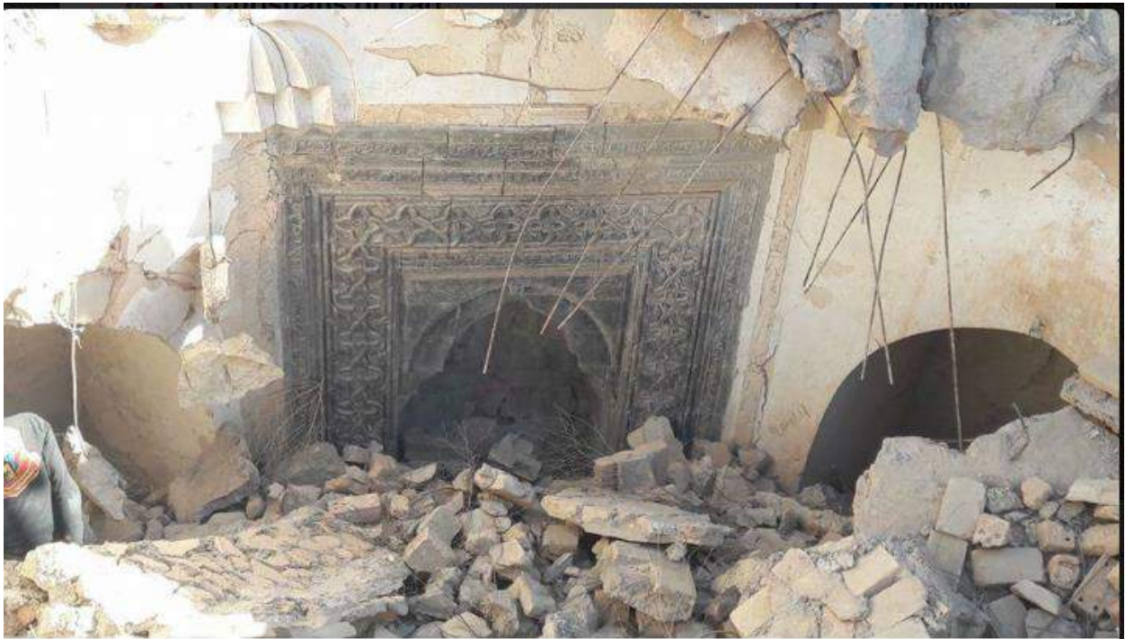
Collapse of the roof of Mar Behnam and Mart Sarah's Tombs (Christians of Iraq/Twitter; November 23, 2016)
