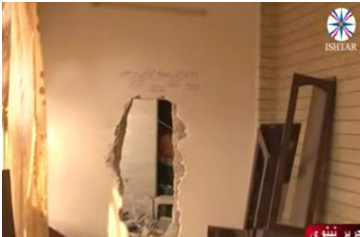
Video still of holes created in between walls by ISIL inside Mar Gerges Church in Bahzani (Ishtar TV; November 11, 2016)
