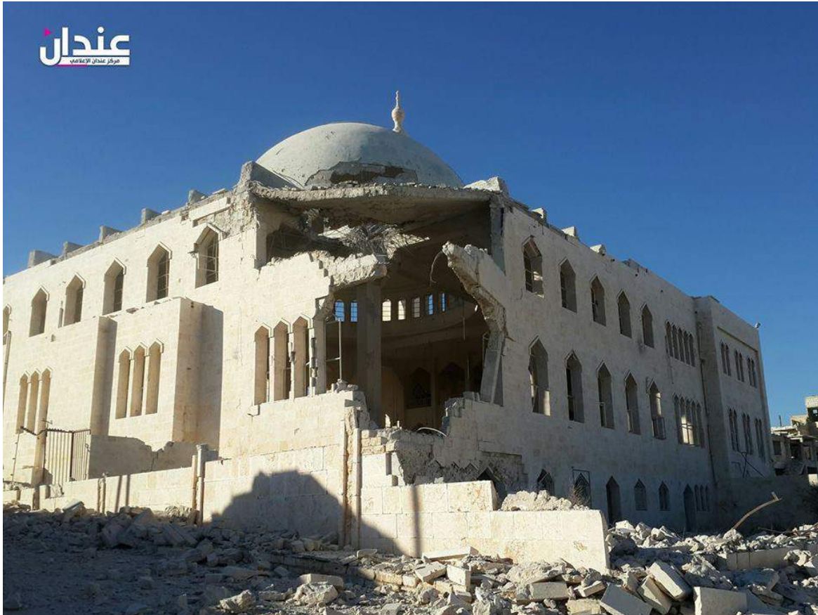
Collapse of the southeast corner of al-Hamza Bin Abd al-Muttaleb Mosque (SNHR; November 18, 2016)
