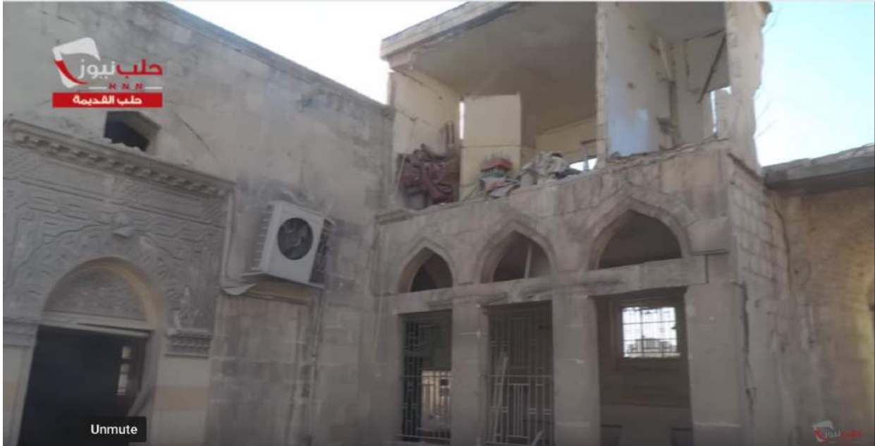
Video still of damage to the interior of Barsin Mosque (SNHR/Youtube; November 17, 2016)
