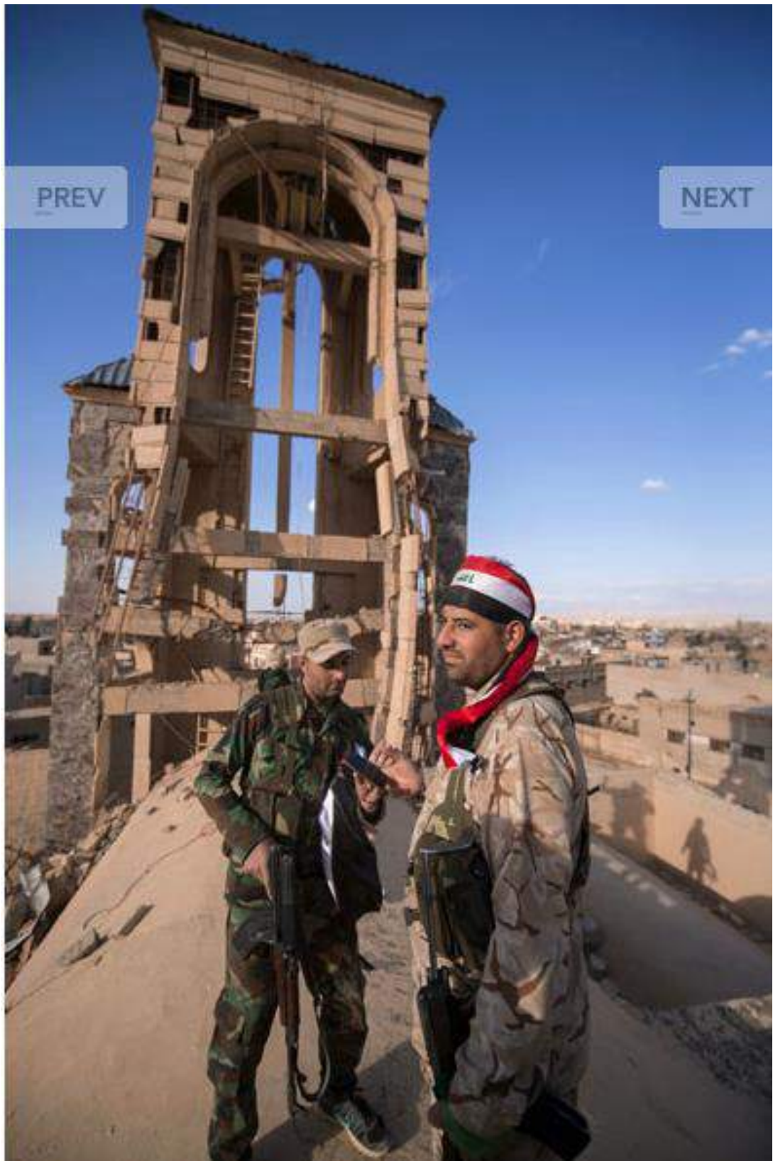
Damage to the bell tower at Mar Yohanna Church (Thomas Goisque; November 20, 2016)
