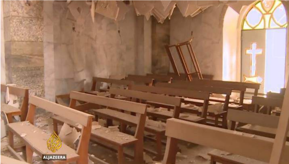
Video still of damage to the interior of Mart Shmone Church in Bashiqa (Al Jazeera, November 21, 2016)
