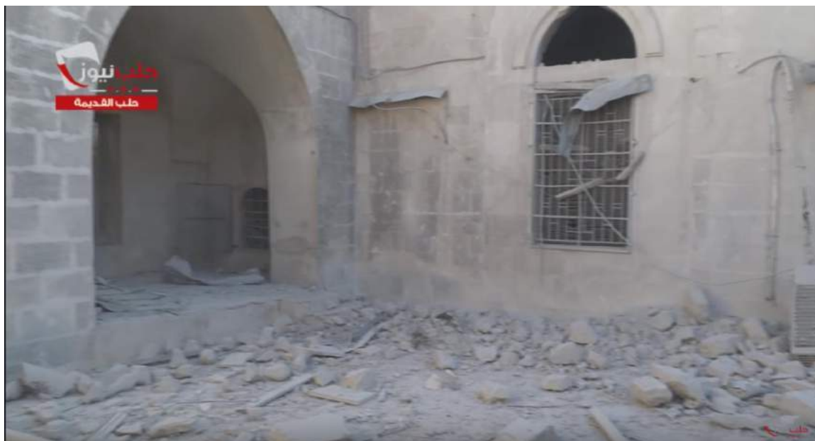
Video still of damage to interior of Barsin Mosque (SNHR/Youtube; November 17, 2016)
