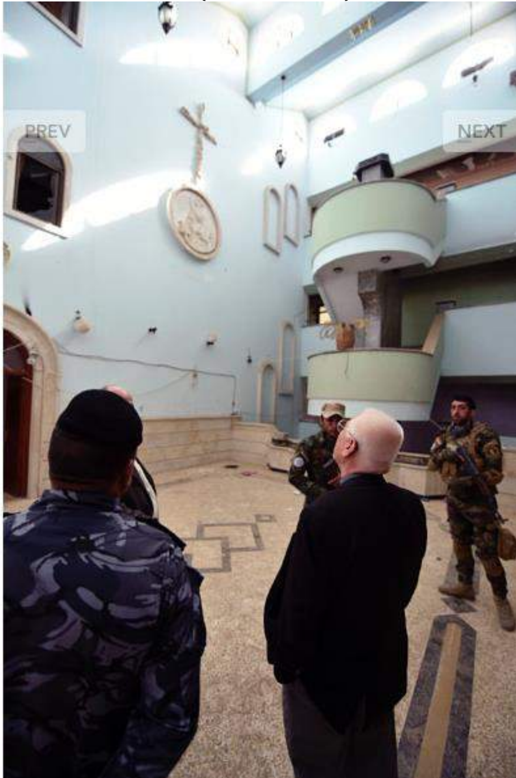
Iraqi soldiers and a priest inspect the damage to Dar Mar Polis Church Services (Thomas Goisque; November 20, 2016)
