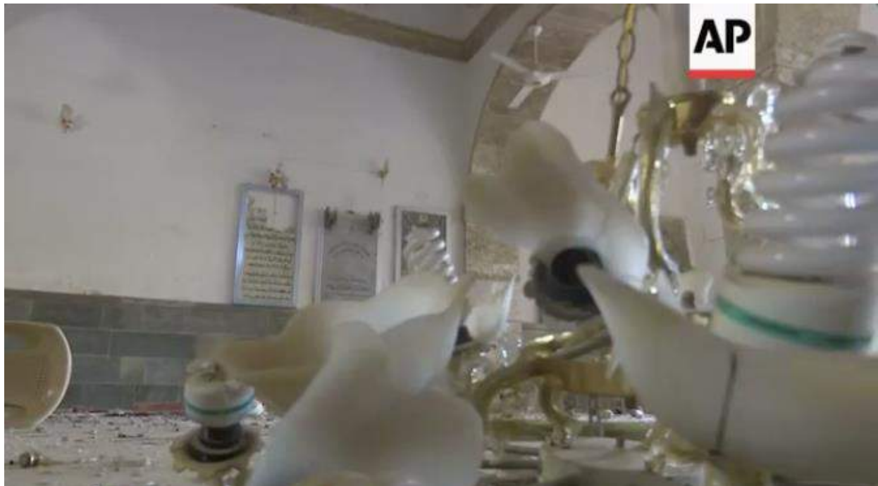
Video still of damage to the interior of Mart Shmone Church in Bashiqa (AP; November 18, 2016)
