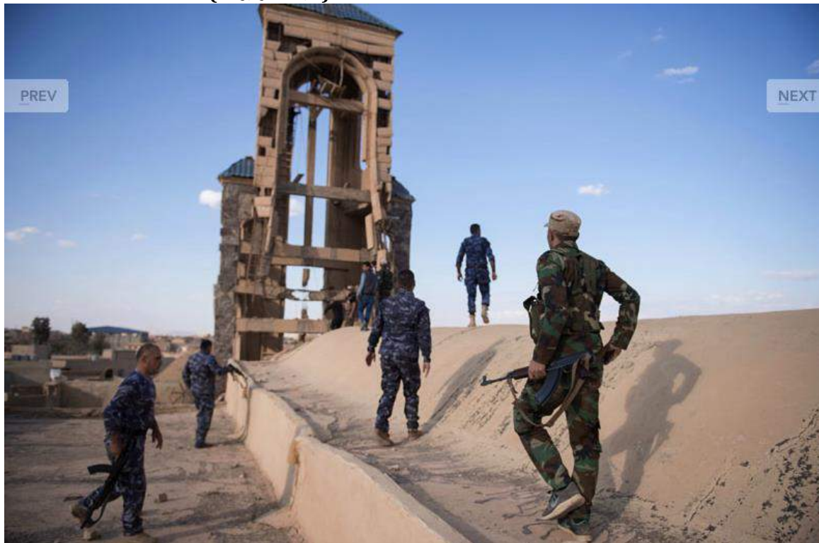
Damage to the bell tower at Mar Yohanna Church (Thomas Goisque; November 20, 2016)
