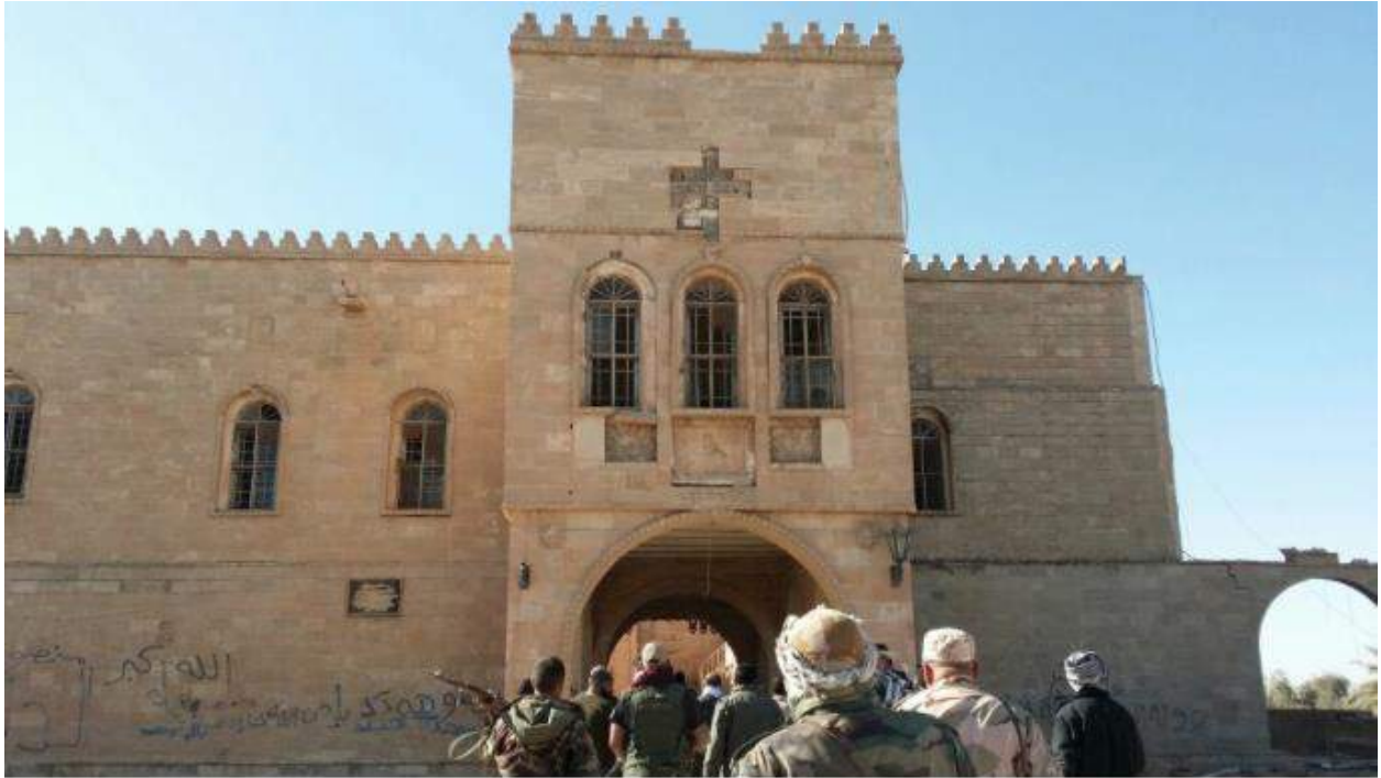
Graffiti and damage to the outer face of Mar Behnam Monastery (November 21, 2016)
