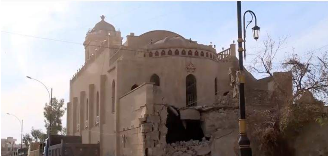
Video still of exterior damage to Mart Mariam Church in Bashiqa (Al Jazeera; November 28, 2016)
