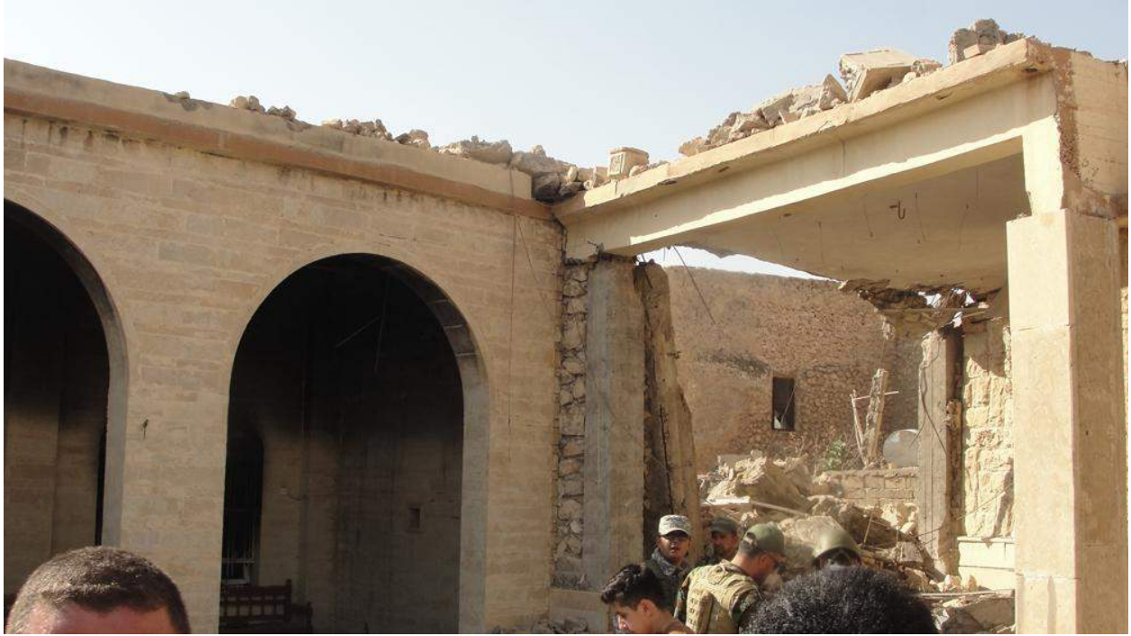
Damage to the Shrine of Pir Bub (Lalish Duhok; November 12, 2016)
