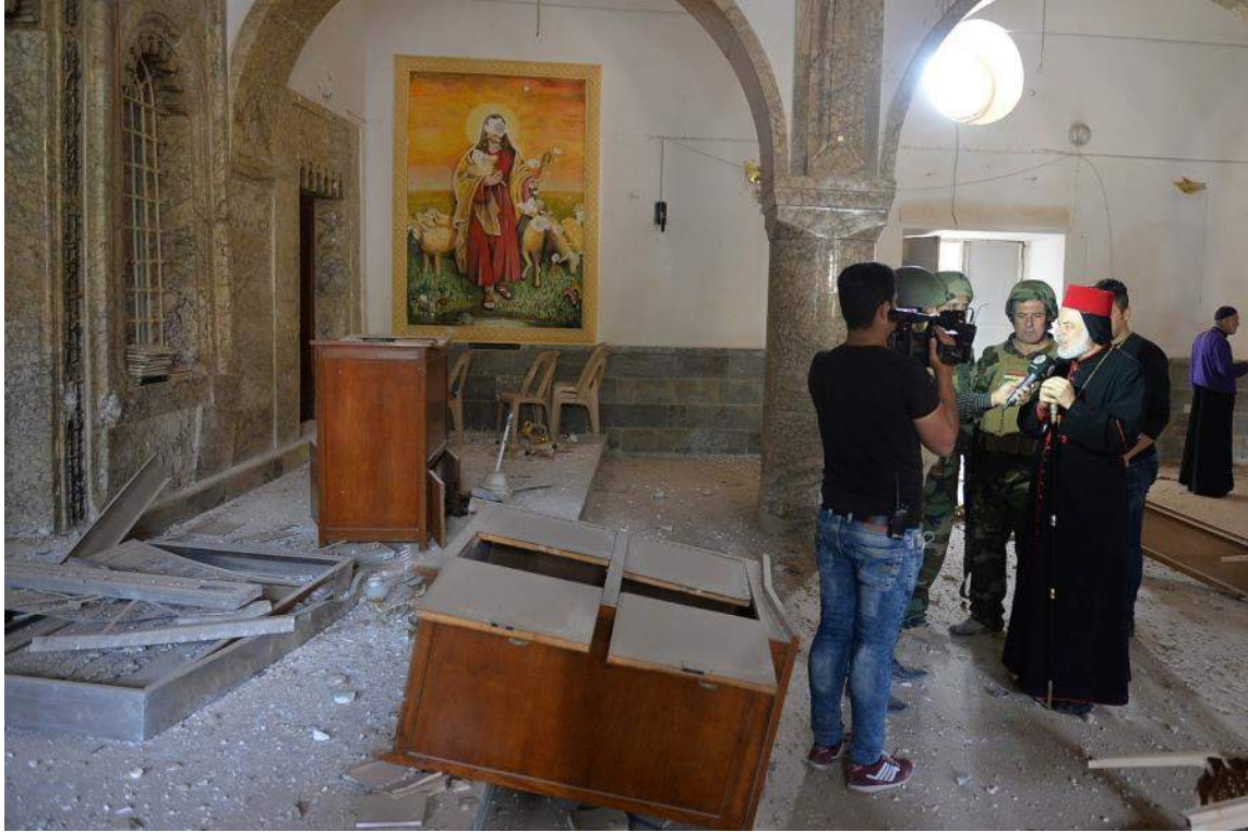
Damage to the interior of Mart Shmone Church in Bashiq (Stripes; November 9, 2016)
