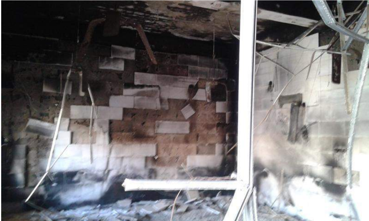
Damage to the Shrine of Pir Bub (Lalish Duhok; November 12, 2016)
