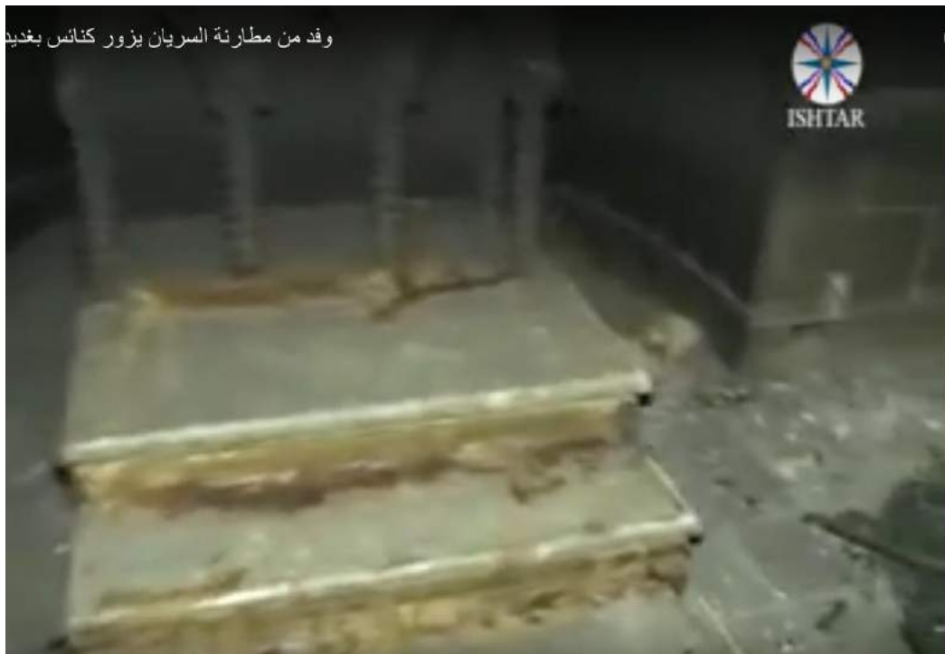
Video still of damage to the altar inside Mart Shmone Church in Bakhdida (IshtarTV; November 23, 2016)
