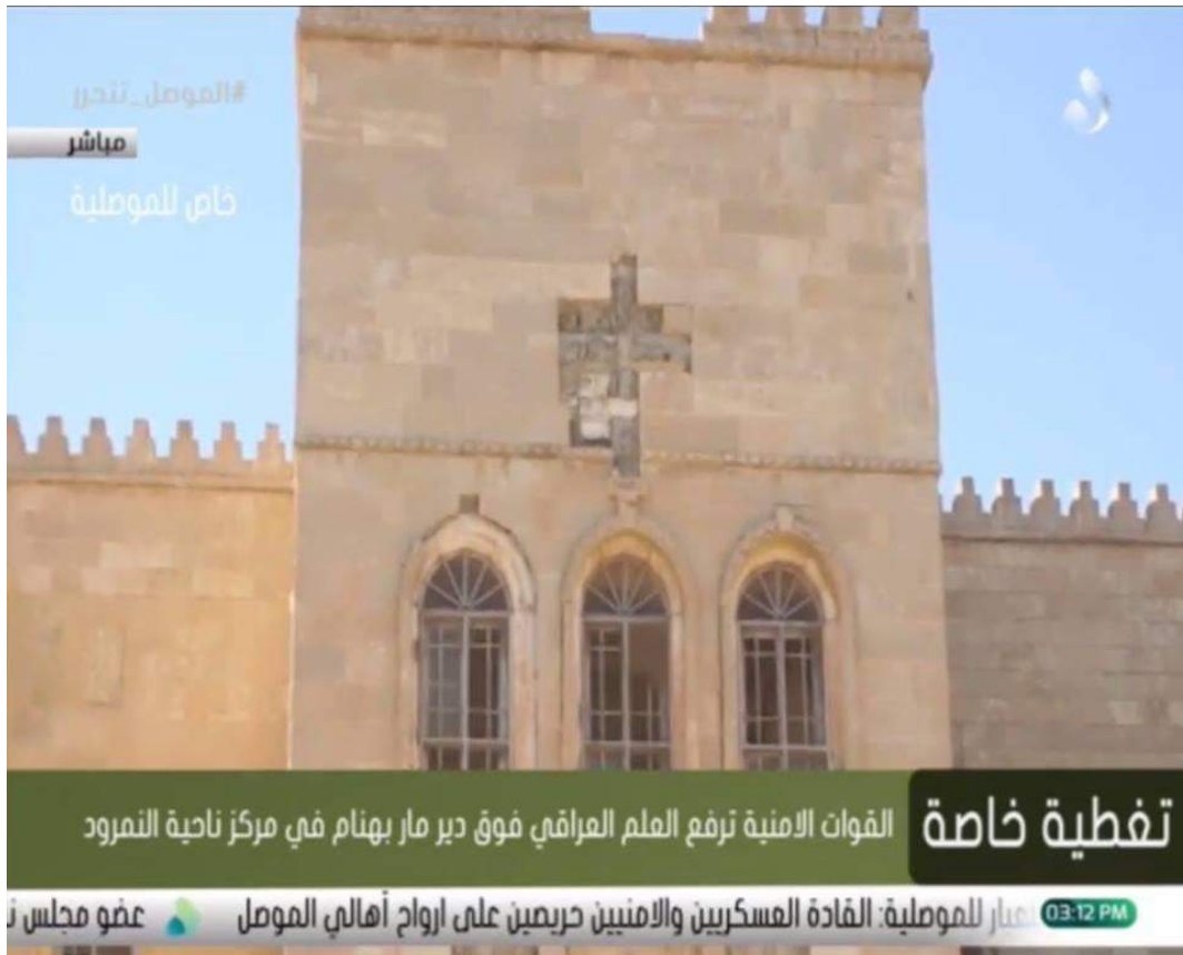
Damage to outer face of Mar Behnam Monastery (Shlama Foundation; November 20, 2016)
