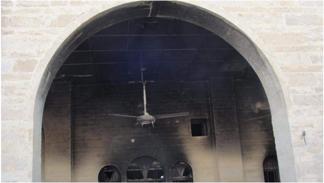
Damage to the Shrine of Pir Bub (Lalish Duhok; November 12, 2016)
