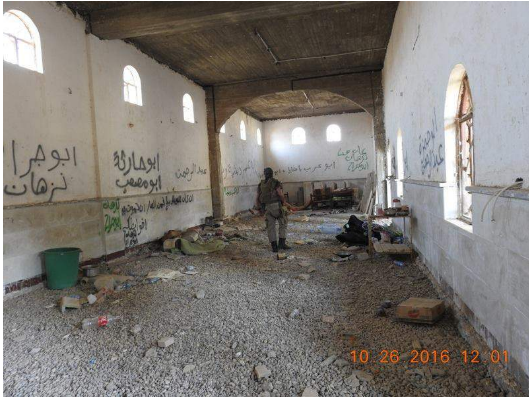
Damage to Mar Oraha Monastery (Twitter; October 26, 2016)
