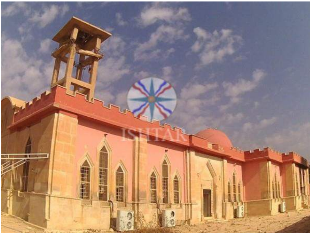
Damage to Mar Ada al-Rasool Church (Ishtar TV; October 31, 2016)
