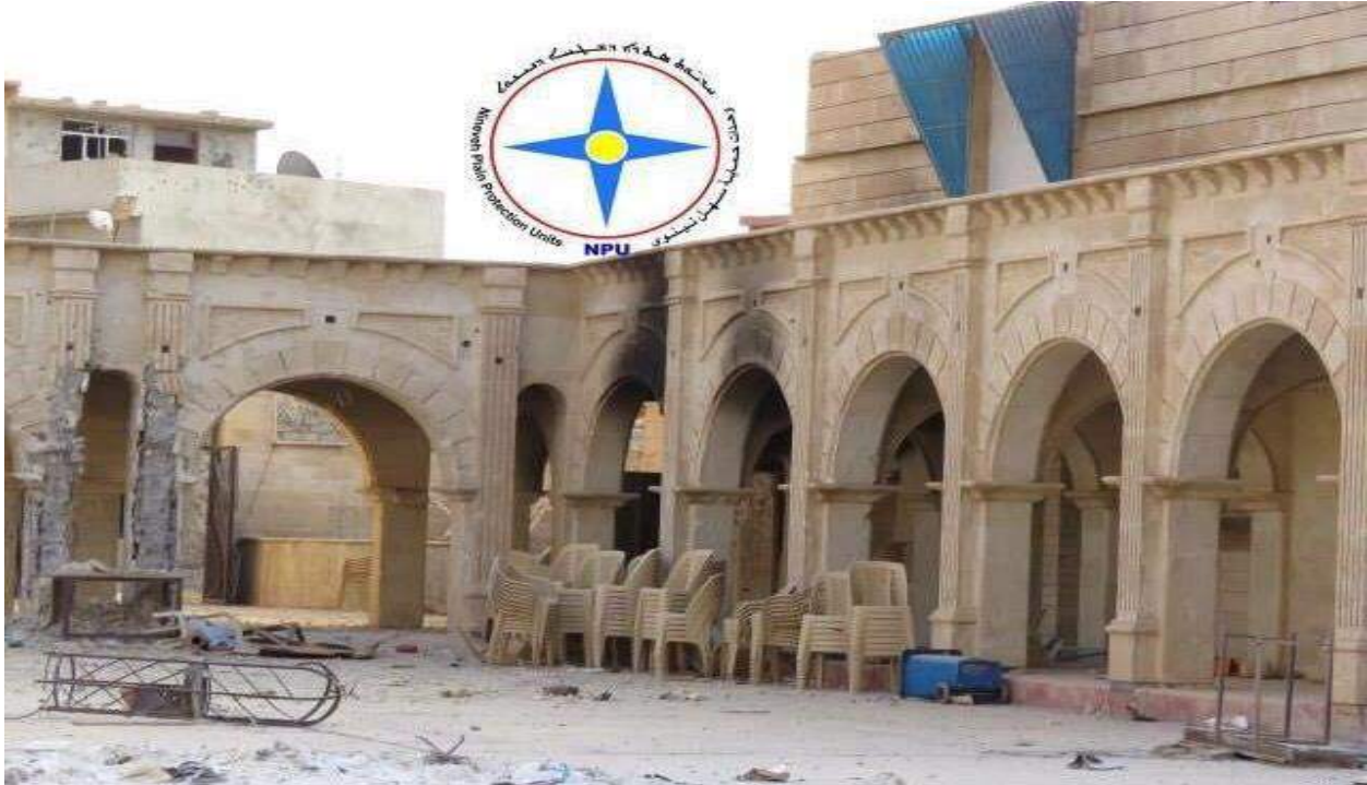
Damage to the courtyard at the al-Tahira Church (NPU; October 23, 2016)
