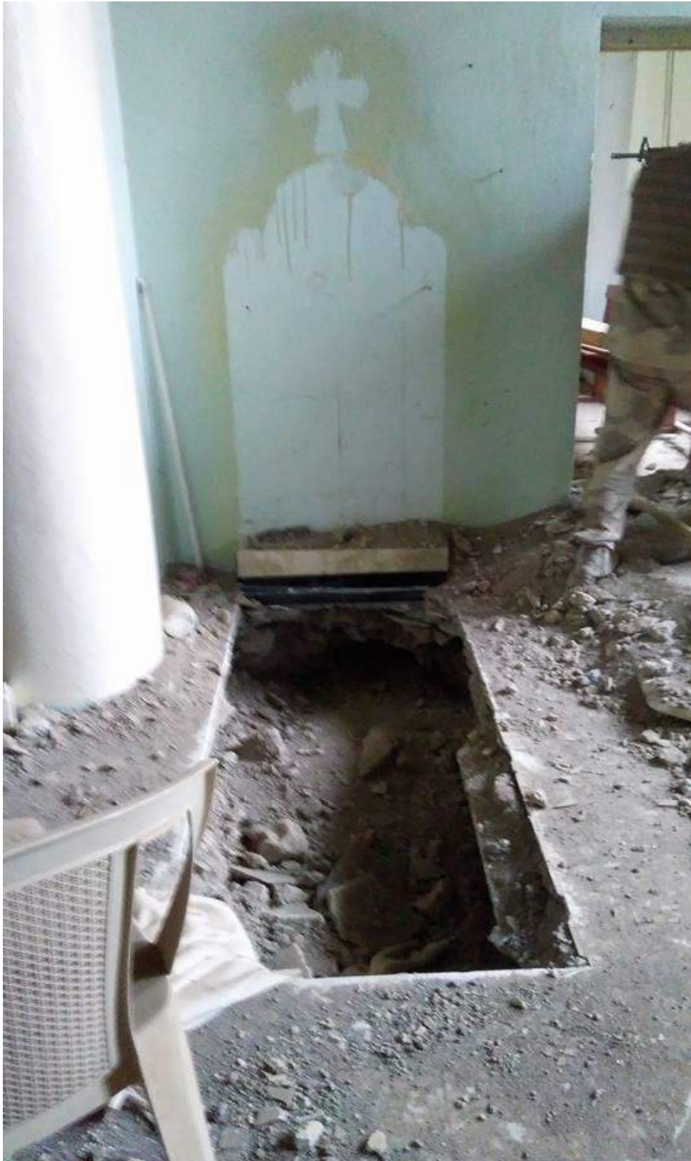
Damage to the interior of Mar Ada al-Rasool Church (Karamlesh; October 28, 2016)
