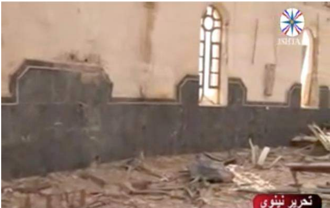
Video still of damage to the interior of the Church of the Resurrection (Ishtar TV; November 8, 2016)
