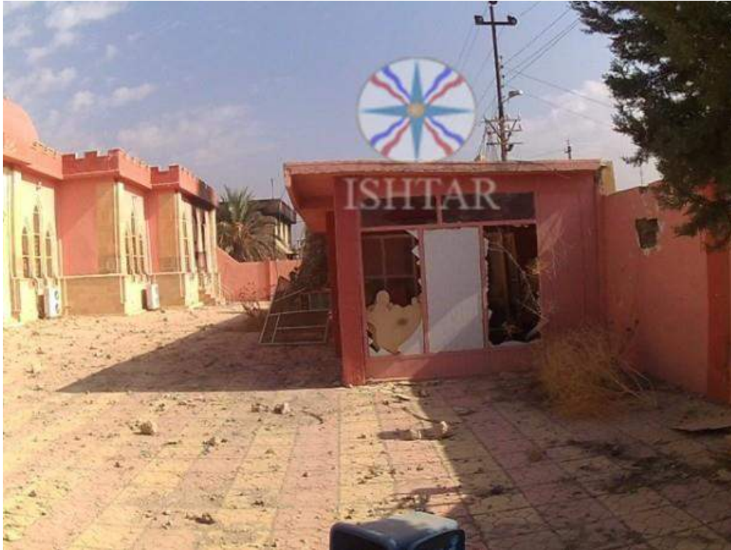
Damage to the exterior of Mar Ada al-Rasool Church (Ishtar TV; October 31, 2016)
