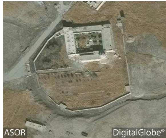
Mar Orah Monastery with damage to the southern and western walls (DigitalGlobe; November 12, 2016)
