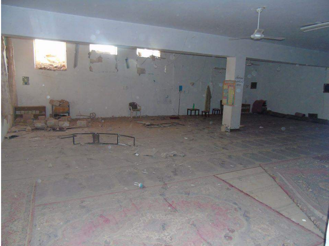
Damage to the interior of Abu Obeida ibn al-Jarrah Mosque (SNHR; November 11, 2016)
