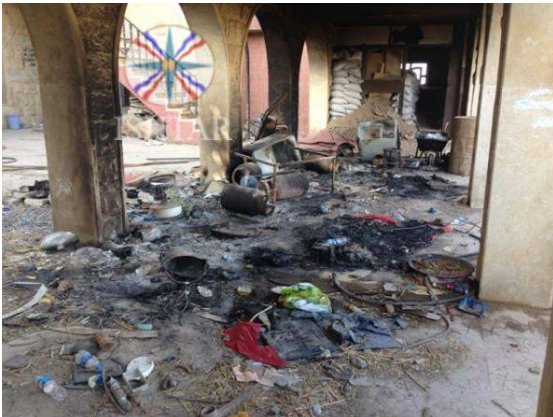
Damage in the courtyard of Mar Barbara Church (Ishtar TV; October 31, 2016)
