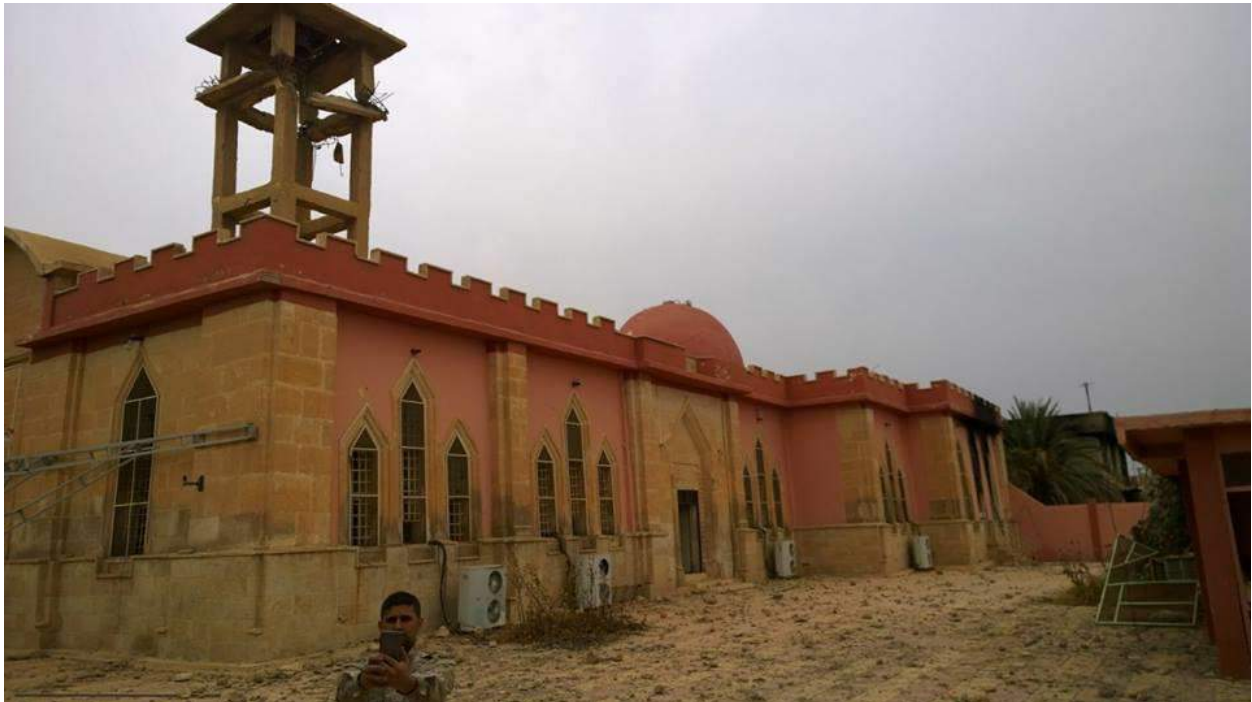
Damage to Mar Ada al-Rasool Church (Karamlesh; October 28, 2016)
