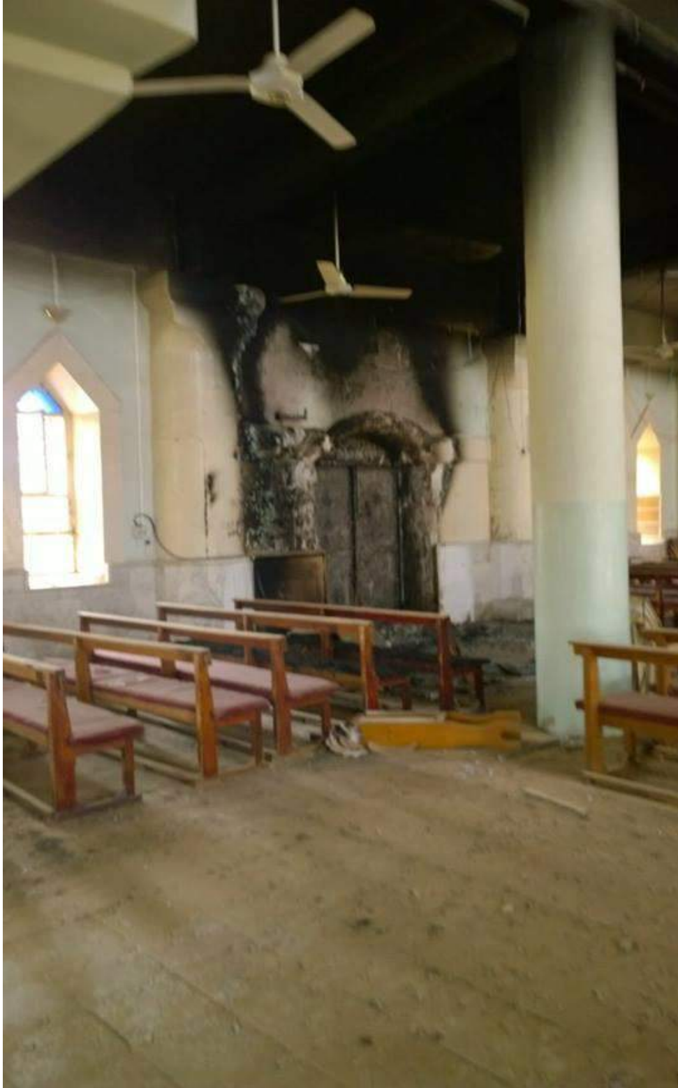
Damage to Mar Ada al-Rasool Church (Karamlesh; October 28, 2016)
