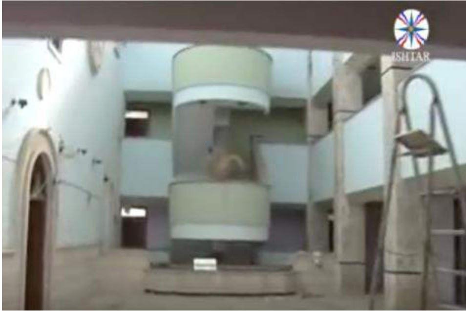
Video still of damage to the interior of Dar Mar Polis Church Services (Ishtar TV; October 31, 2016)
