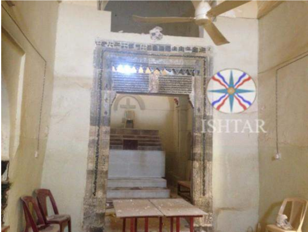
Damage to the interior of Mar George Church (Ishtar TV; October 31, 2016)
