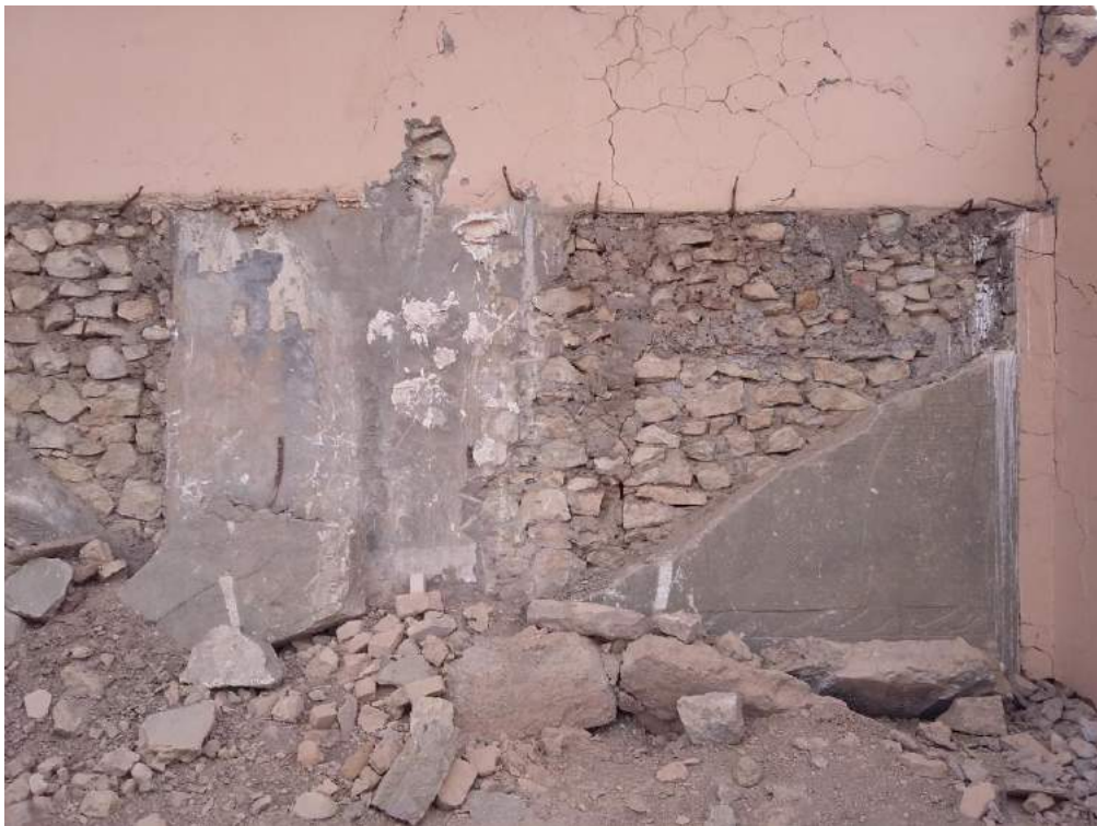
Damage to the outside facade of Gate D at the Northwest Palace at Nimrud (Courtesy of Max Delaney, AFP; November 15, 2016)
