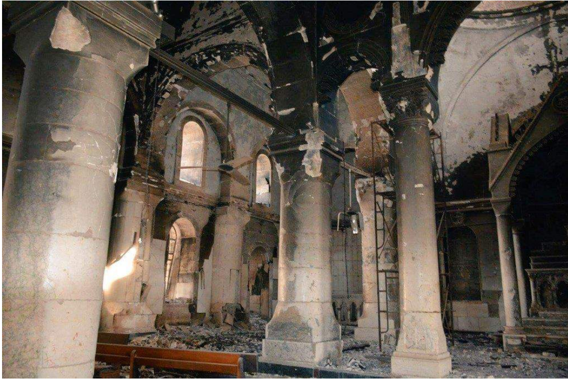
Extensive damage to al-Tahira Syriac Church (Iraqi Christian Relief Council; October 26, 2016)
