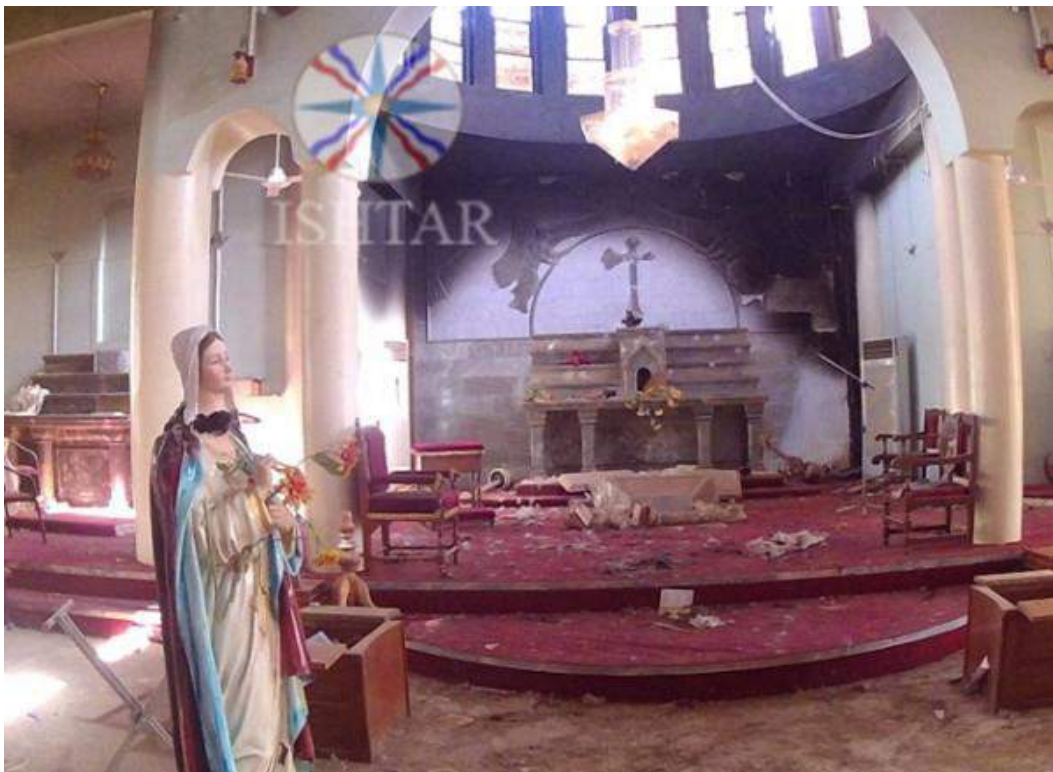
Damage to the interior of Mar Ada al-Rasool Church where a statue has been crudely reconstructed (Ishtar TV; October 31, 2016)
