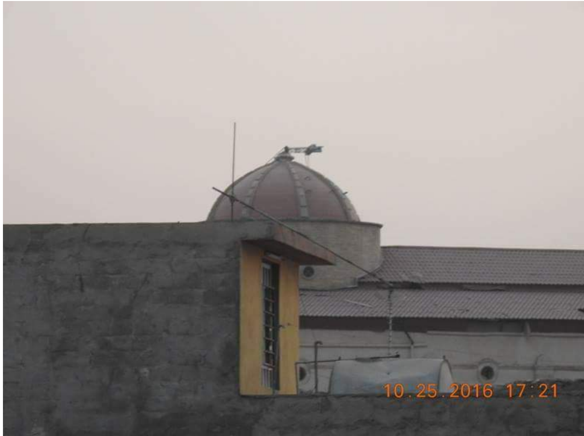
Damage to the dome of Mar Qoryaqos Church (This is Christian Iraq; October 25, 2016)
