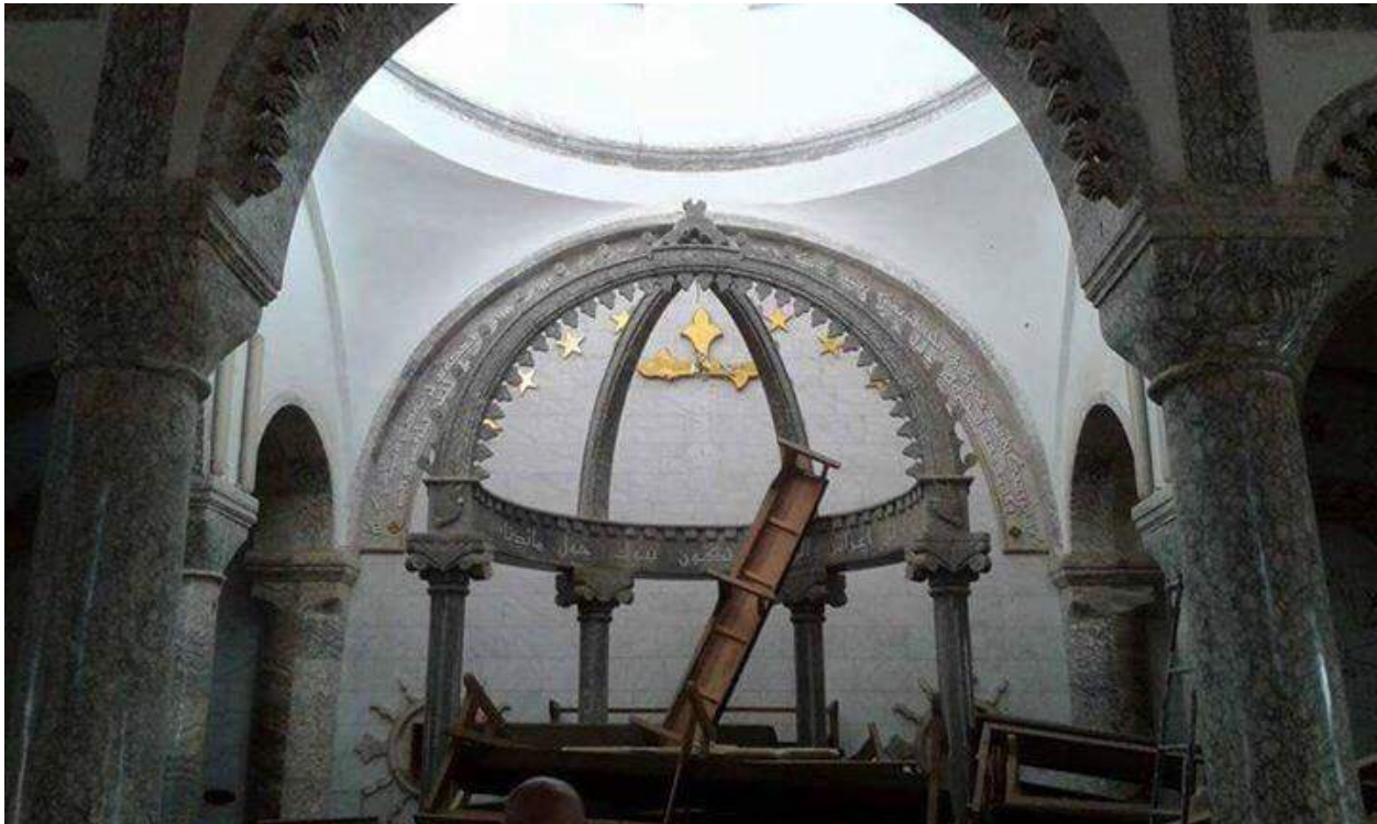
Damage to Mar Yohanna Church (Fraternité en Irak; October 23, 2016)
