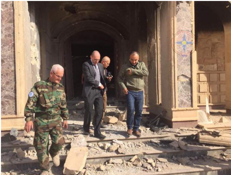
Members of the French Consulate in Erbil tour the damage to the Church of Saints Behnam and Sarah (NPU; November 14, 2016)
