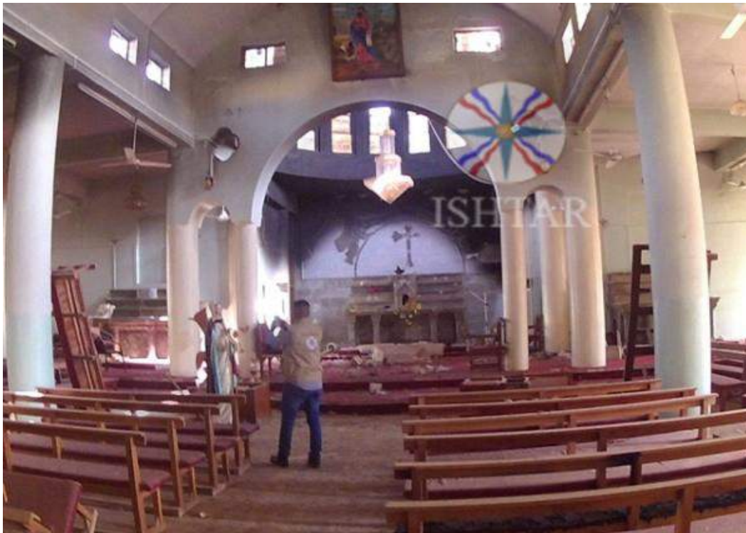
Damage to the interior of Mar Ada al-Rasool Church (Ishtar TV; October 31, 2016)
