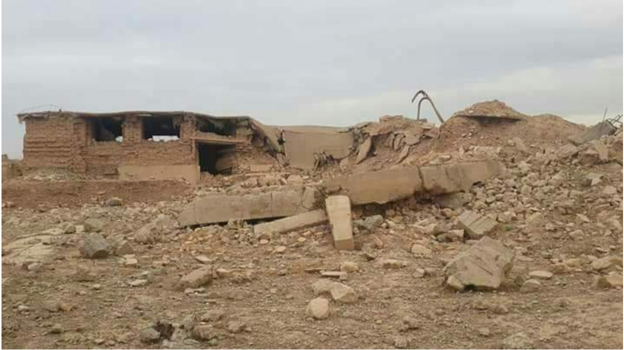
The Northwest Palace, rooms EB/EA after destruction in April (Al Harith Al Shwely; November 15, 2016)
