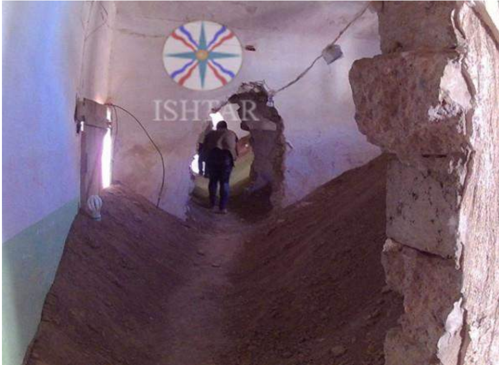
A large hole in the wall allowing militants to move between rooms at Mar Joseph Cultural Center (Ishtar TV; October 31, 2016)
