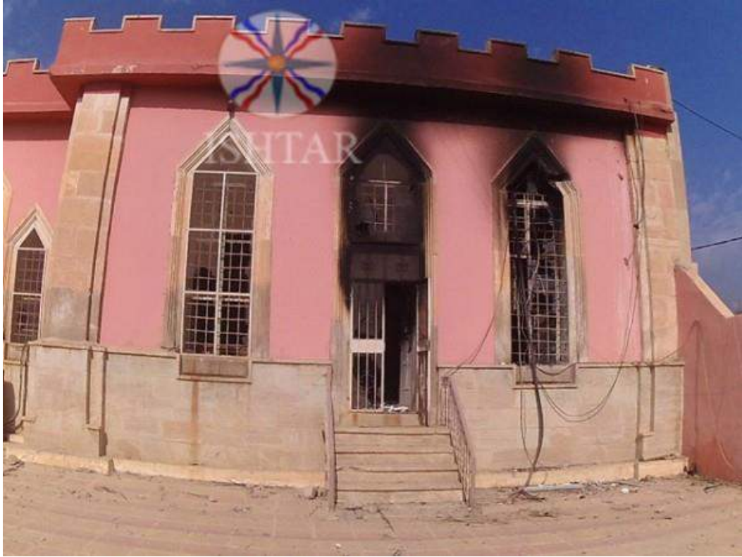
Fire damage seen on the outside of Mar Ada al-Rasool Church (Ishtar TV; October 31, 2016)
