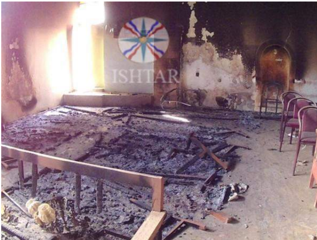
Fire damage to the interior of the Virgin Mary Church (Ishtar TV; October 31, 2016)
