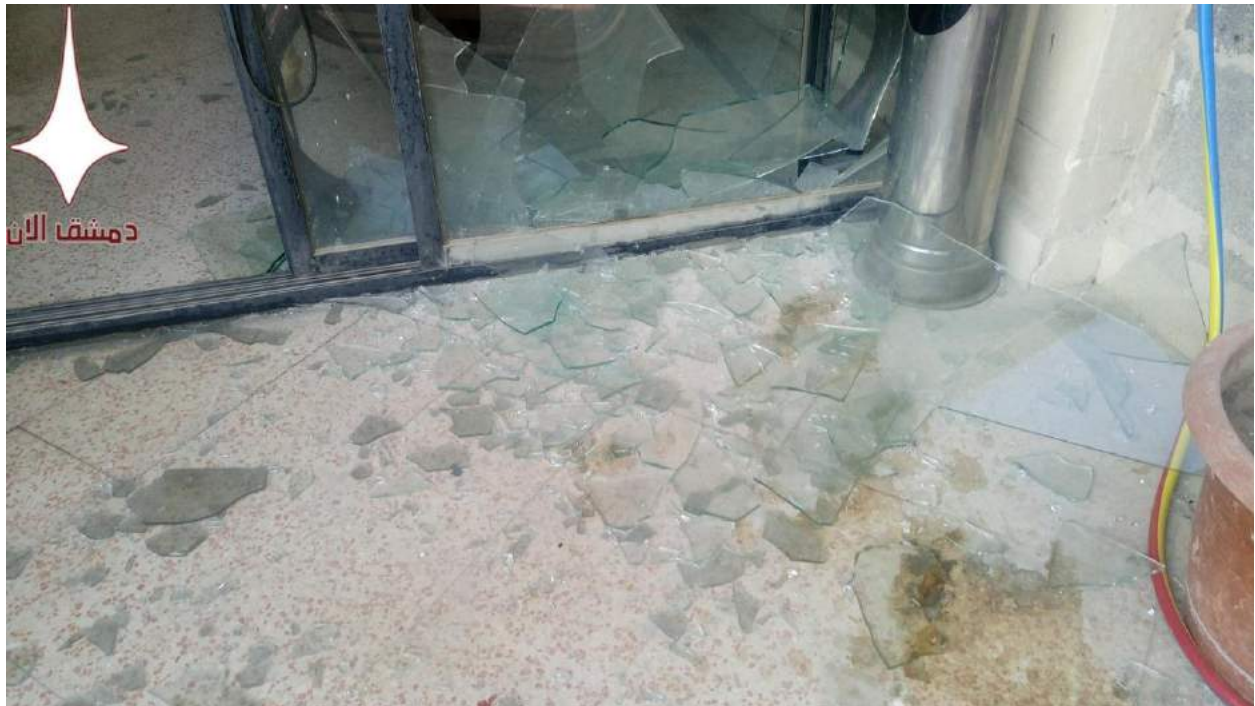
Broken windows at the Maronite Diocese building (Damascus Now; November 8, 2016)
