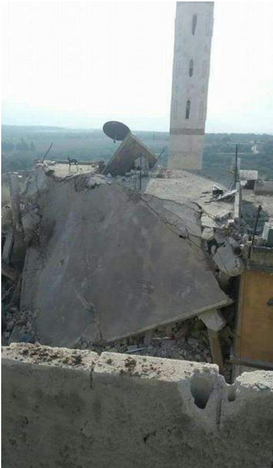
Severe damage to Mashmashan Mosque (SNHR; November 14, 2016)
