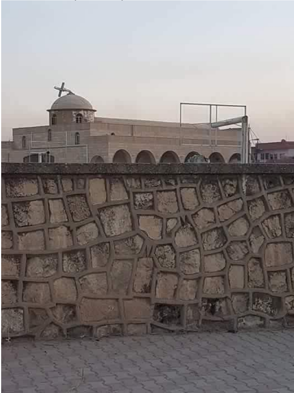
Damage to the belfry at Mar Yacob Church (Shlama Foundation; October 23, 2016)
