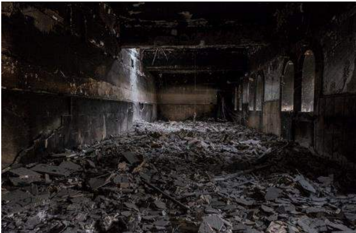
Extensive fire damage inside the al-Tahira Church (Getty Images; October 30, 2016)
