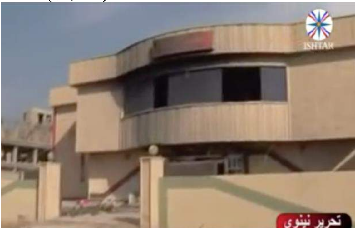
Video still of fire damage to the exterior of Ishtar Hall (Ishtar TV; November 8, 2016)
