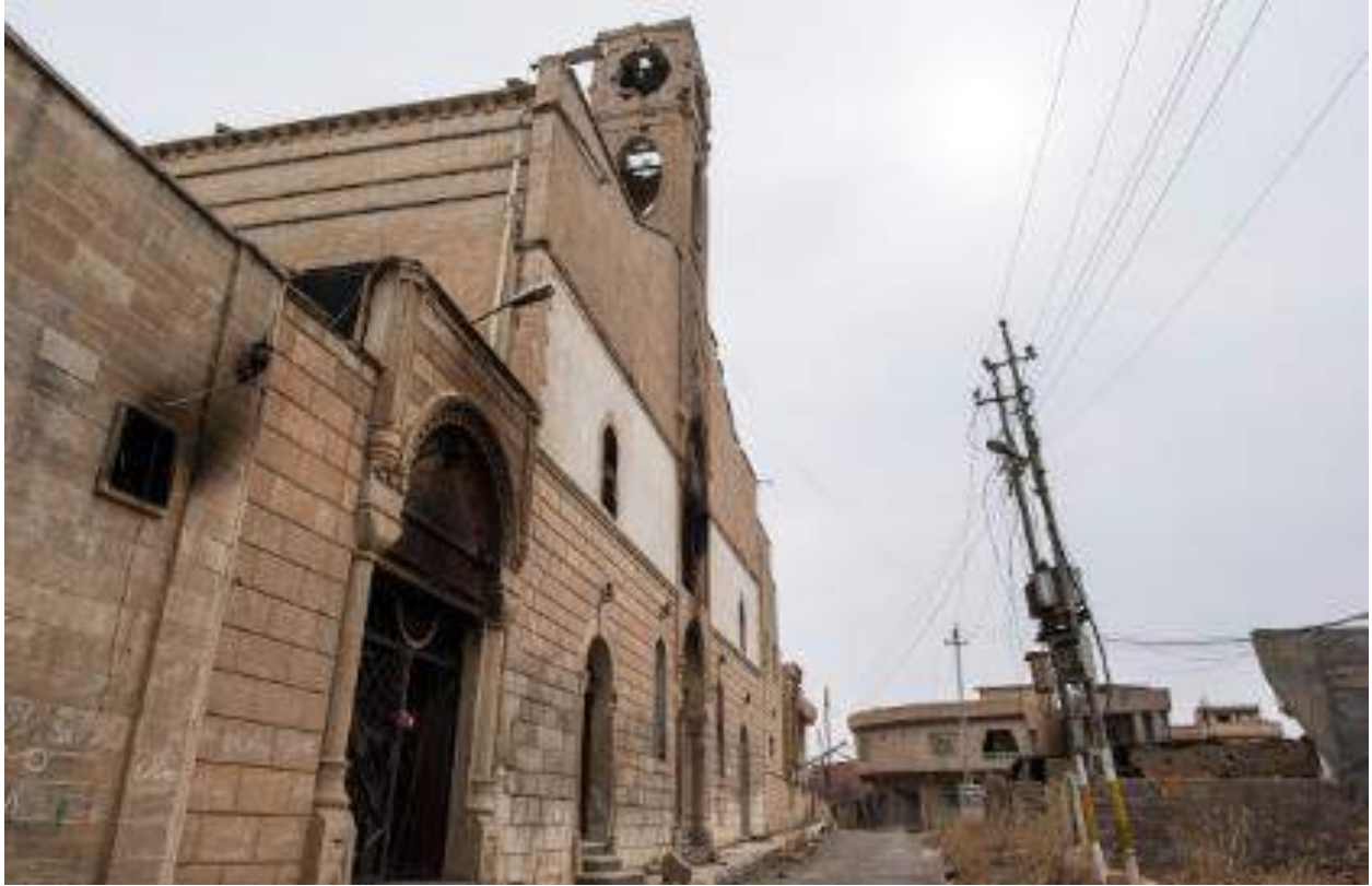
Fire and explosives damage to the exterior of the al-Tahira Church (Getty Images; October 30, 2016)
