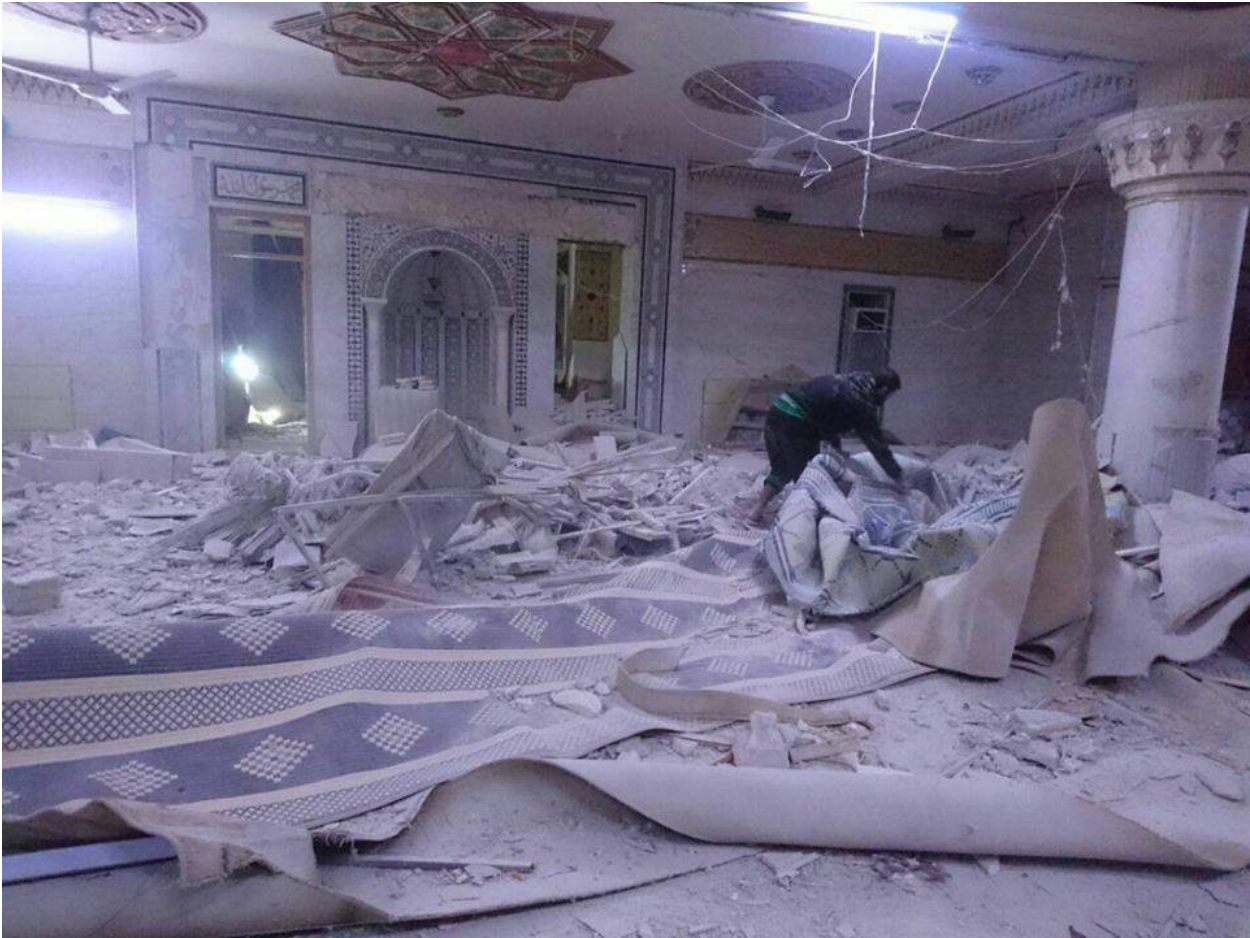
Rubble and damage in the interior of al-Huda Mosque (SNHR; November 13, 2016)
