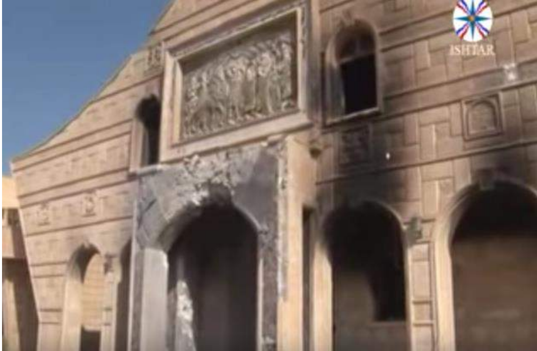
Video still of detail of damage to the Church of Saints Behnam and Sarah (Ishtar TV; October 31, 2016)
