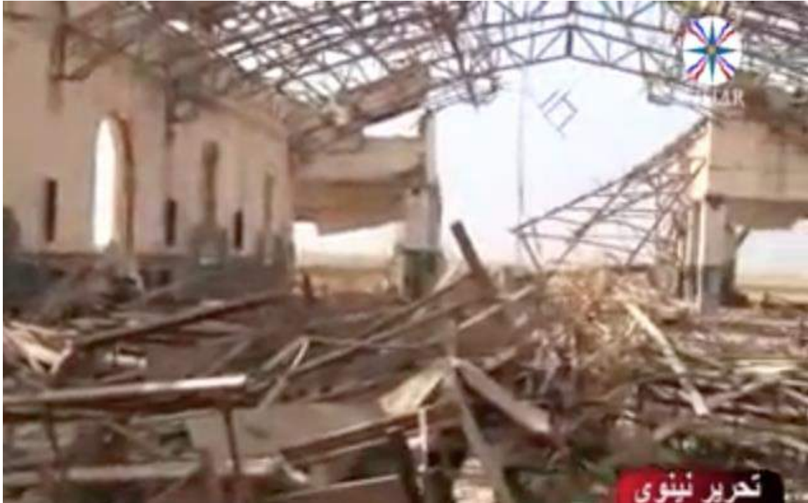
Video still of damage to interior of the Church of the Resurrection (Ishtar TV; November 8, 2016)
