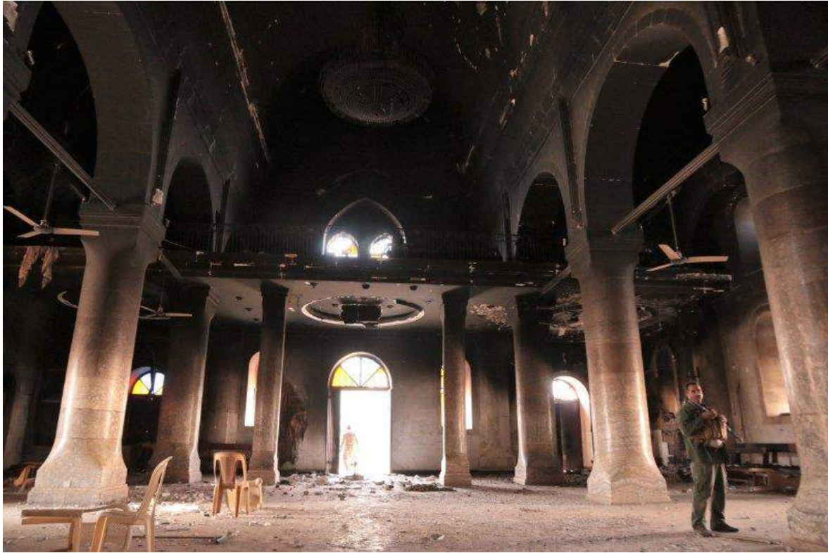
Damage to the interior of the al-Tahira Church (The Daily Beast; October 26, 2016)
