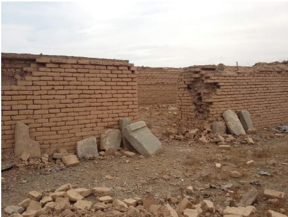
Damage to Northwest Palace at Nimrud (Courtesy of Max Delaney, AFP; November 15, 2016)
