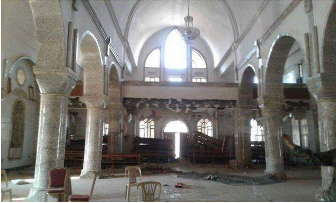
Damage to the interior of Mar Yohanna Church (Fraternité en Irak; October 23, 2016)
