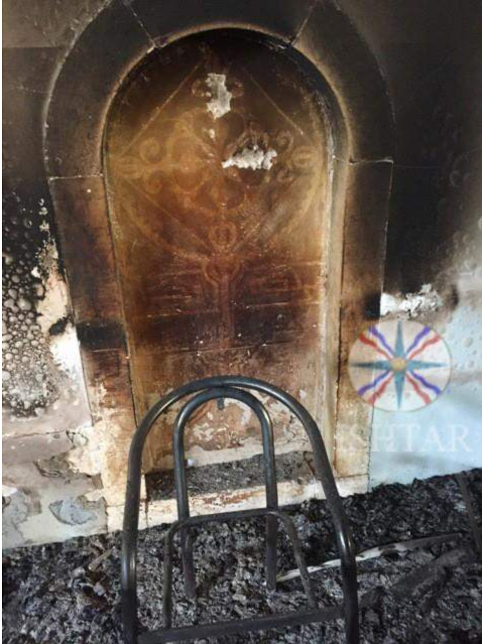
Fire damage to the interior of the Virgin Mary Church (Ishtar TV; October 31, 2016)
