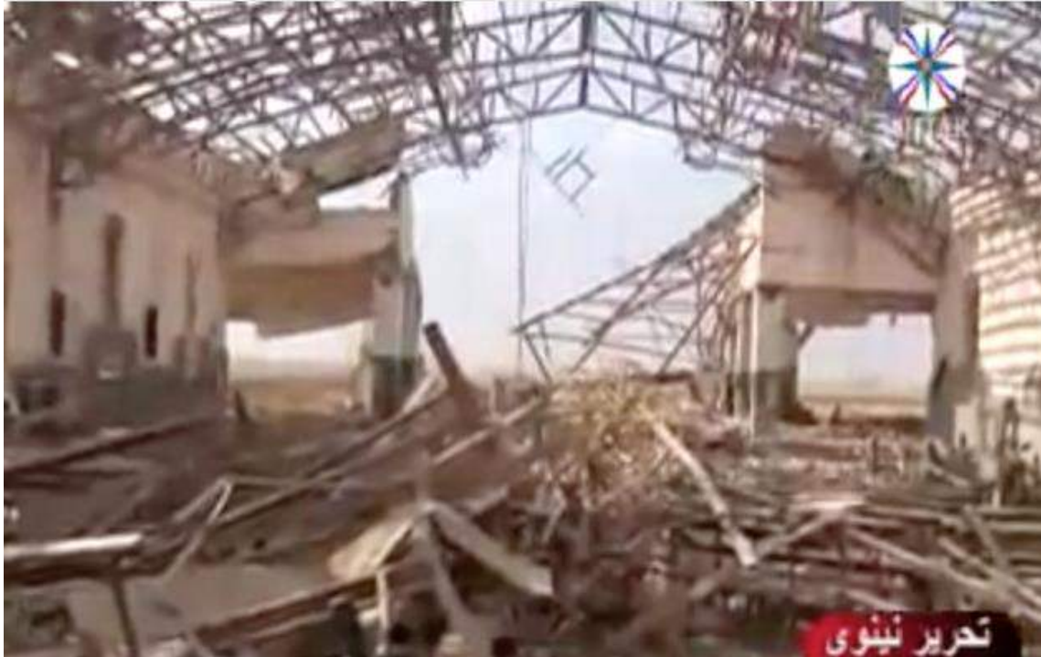
Video still of damage to the interior of the Church of the Resurrection (Ishtar TV; November 8, 2016)
