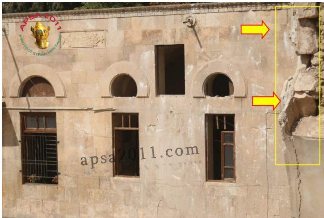
Damage to courtyard of al-Tawba Mosque, facing north (APSA; October 6, 2016)
