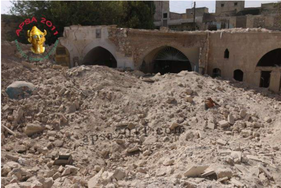
Severe damage to courtyard of al-Tawba Mosque, facing west (APSA; October 6, 2016)
