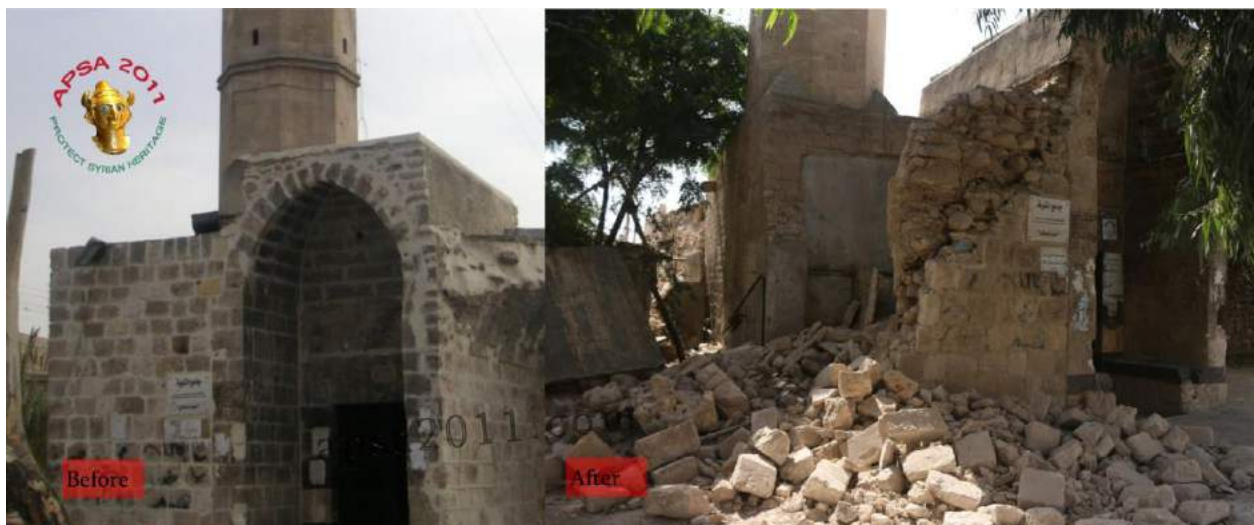
Severe damage to north wall and entrance of al-Tawba Mosque (APSA; October 6, 2016)
