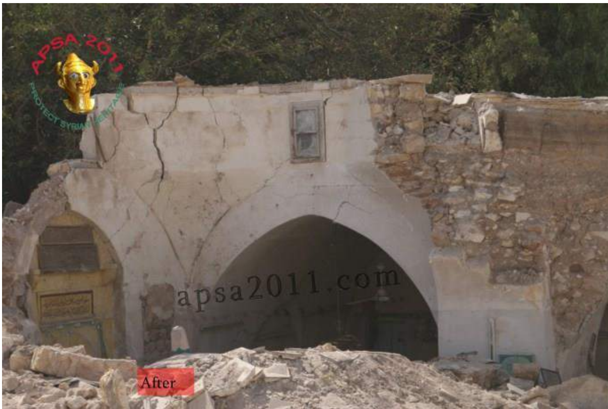
Damage to courtyard of al-Tawba Mosque, facing south (APSA; October 6, 2016)
