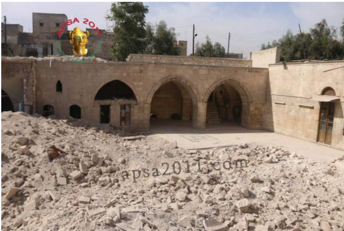
Damage to courtyard of al-Tawba Mosque, facing northwest (APSA; October 6, 2016)
