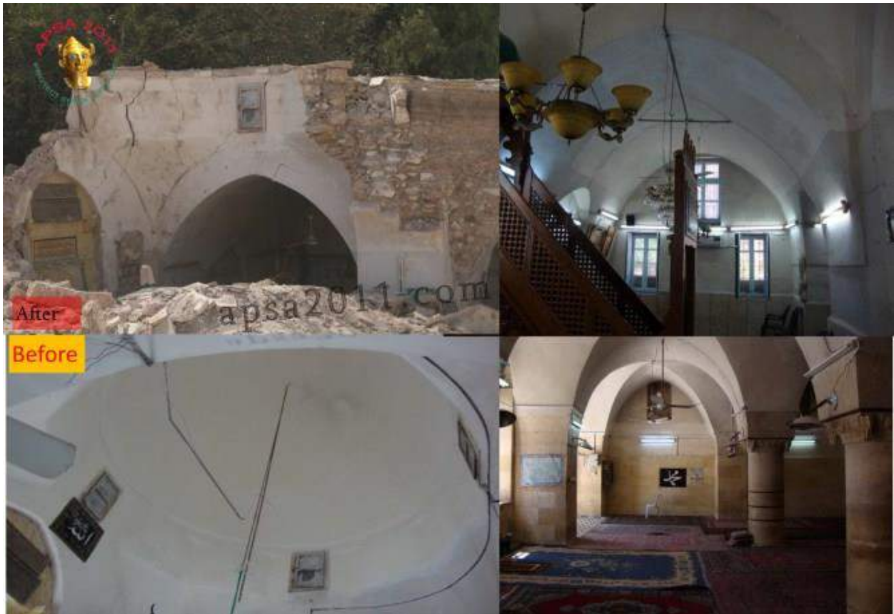
Damage to southern section of mosque and 'before' photographs (APSA; October 6, 2016)
