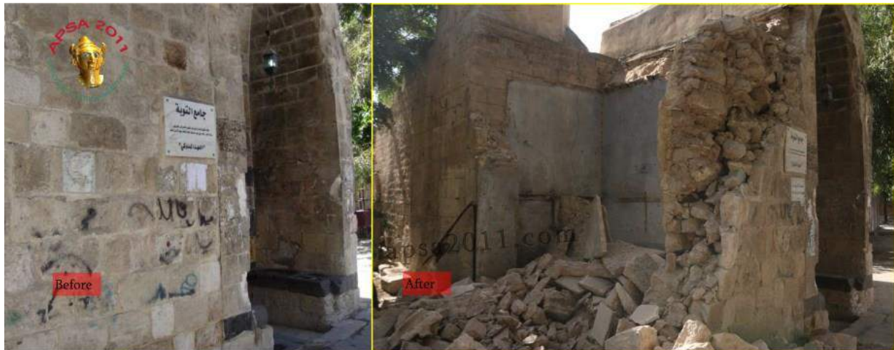
Severe damage to north wall and entrance of al-Tawba Mosque (APSA; October 6, 2016)
