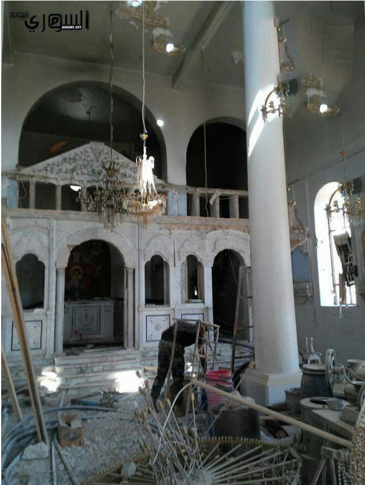
Damage to the interior of Saint Paul the Apostle Church (ASoury; September 5, 2016)
