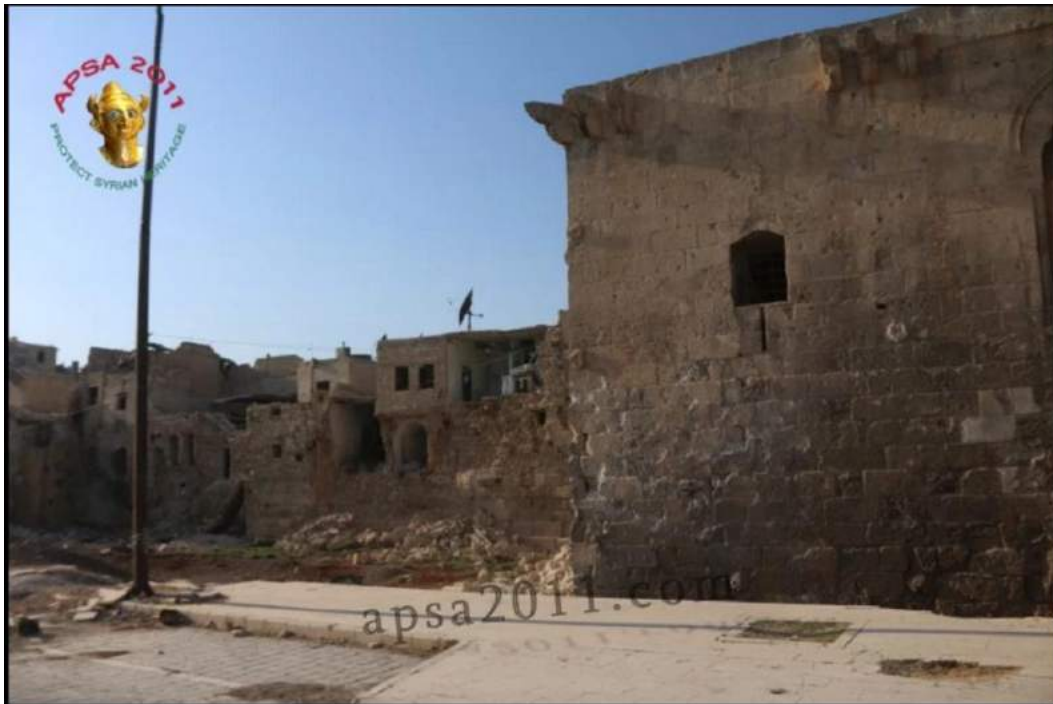
Damage to southern facade of the rampart tower and fortification wall (APSA; August 28, 2016)
