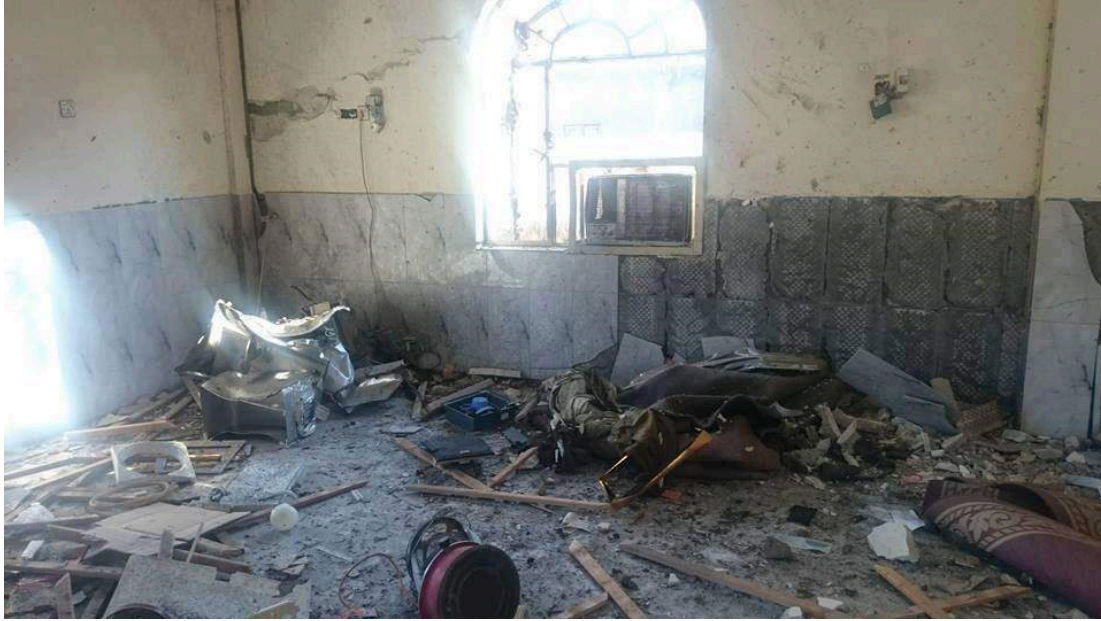
Damage to the interior of Ammar Bin Yasser Mosque (Iraq News Facebook Page; January 6, 2015)
