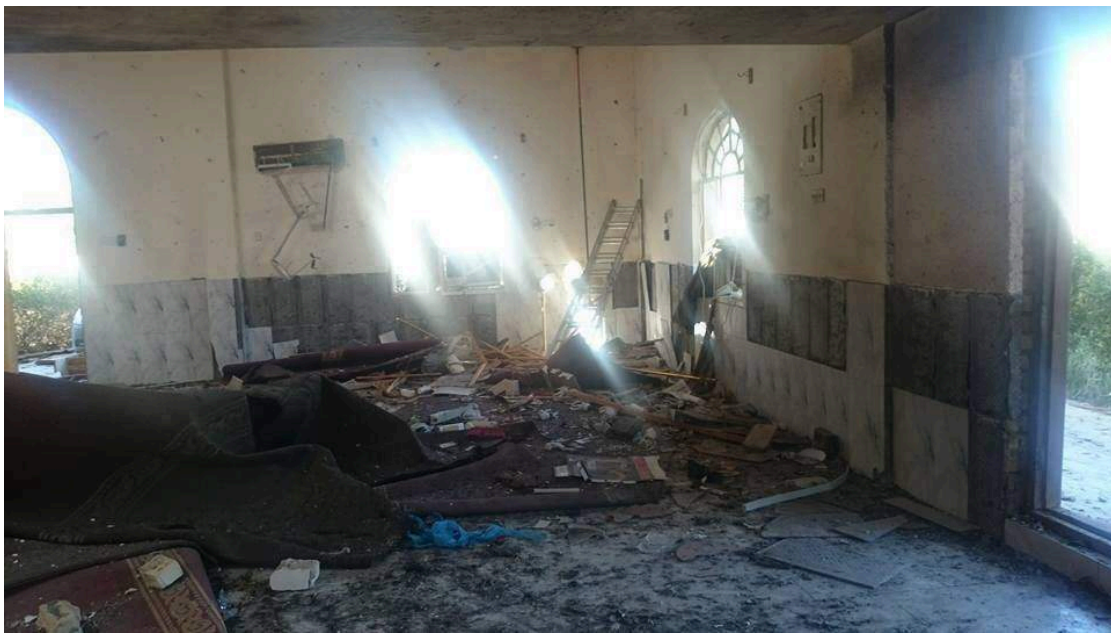
Damage to the interior of Ammar Bin Yasser Mosque (Iraq News Facebook Page; January 6, 2015)
