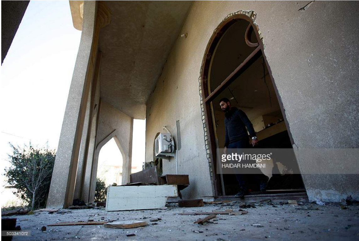
Damage to the exterior of Ammar Bin Yasser Mosque (Getty Images/AFP; January 4, 2016)
