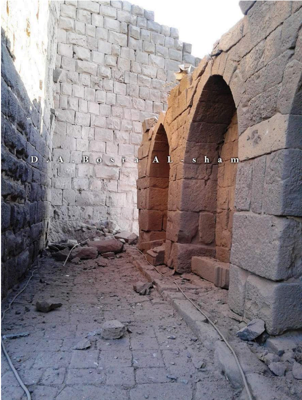
Damage to Ayyubid Citadel (Bosra al-Sham Department of Antiquities; December 22, 2015)
