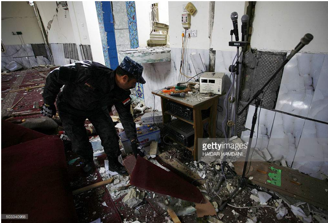
Damage to the interior of Ammar Bin Yasser Mosque (Getty Images/AFP; January 4, 2016)
