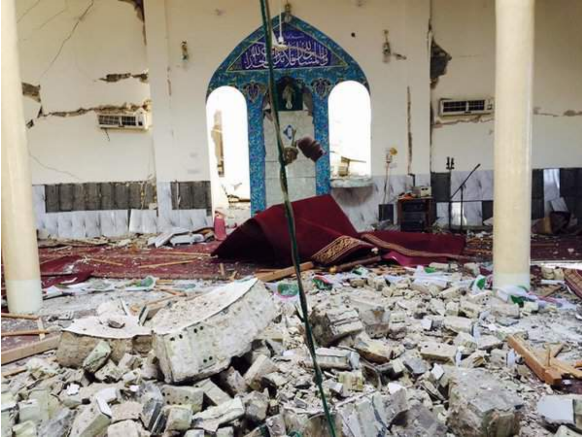
Damage to the interior of Ammar Bin Yasser Mosque (Al Mada Press; January 4, 2016)
