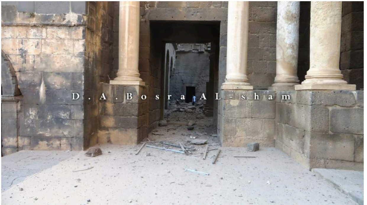
Damage to corridors in Ayyubid Citadel (Bosra al-Sham Department of Antiquities; December 22, 2015)
