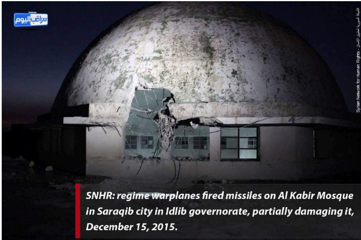
Damage to Al Kabir Mosque (SNHR; December 15, 2015)
