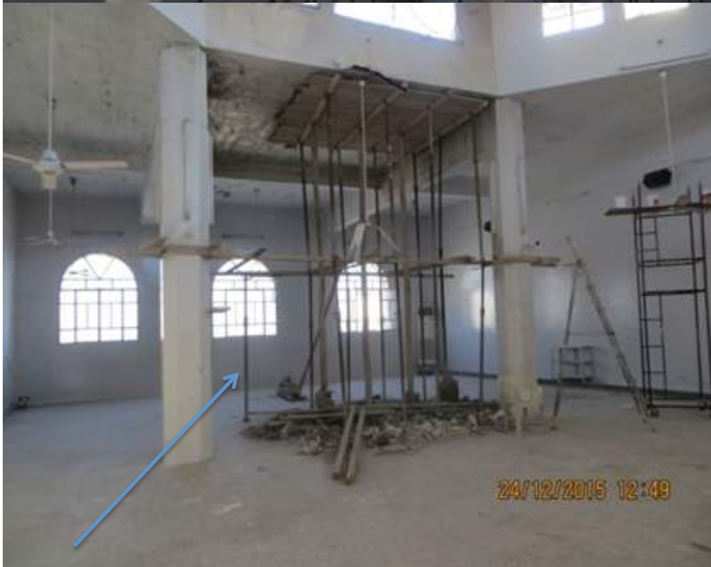
Scaffolding in place to hold shore up damaged section of the building
