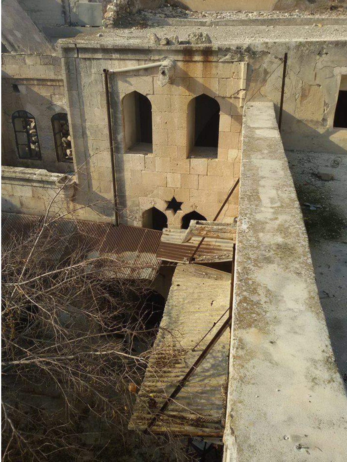
Damage to Old Arab House in Aleppo (Private Facebook Account; December 19, 2016)
