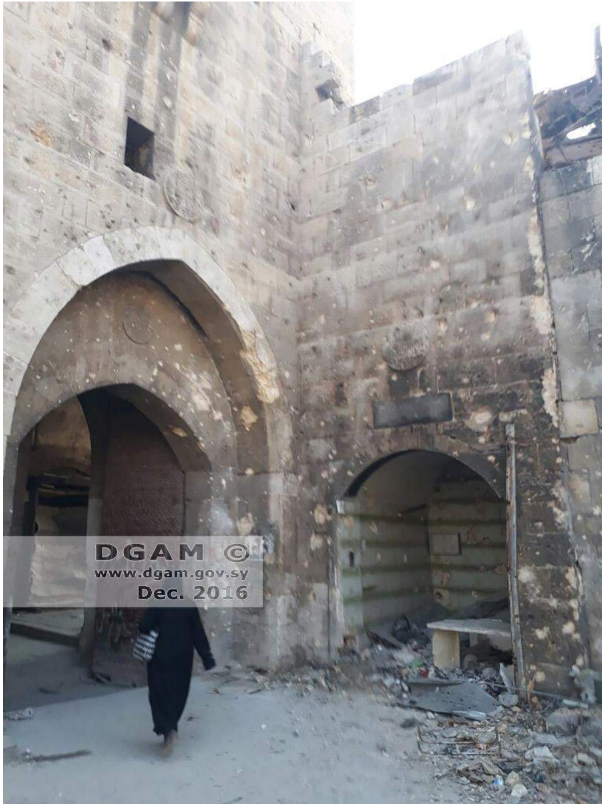
Smoke and impact damage to Bab al-Hadid (DGAM; December 20, 2016)
