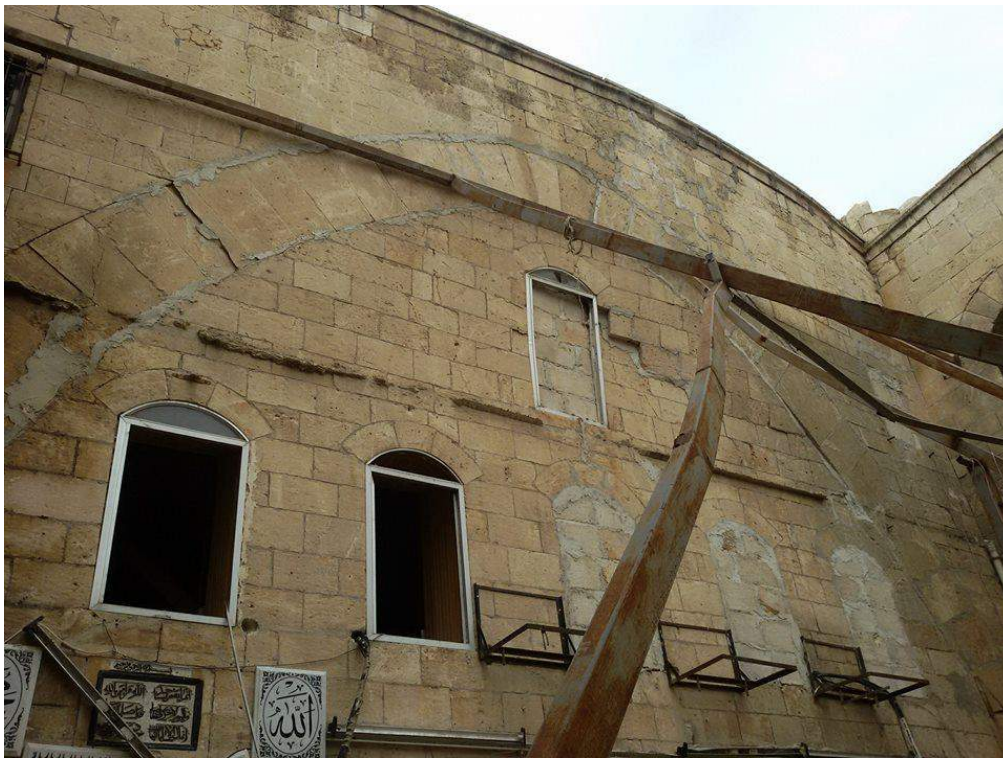
Light damage, with possible support beams, in the courtyard of Mosque and Madrasa Turuntaiya (Private Facebook Account; December 22, 2016)
