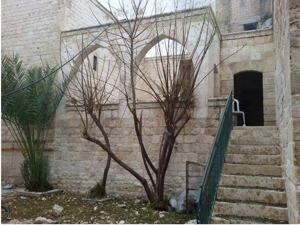
Minimal damage to one side of al-Tarsusi Mosque (Private Facebook Account; December 24, 2016)
