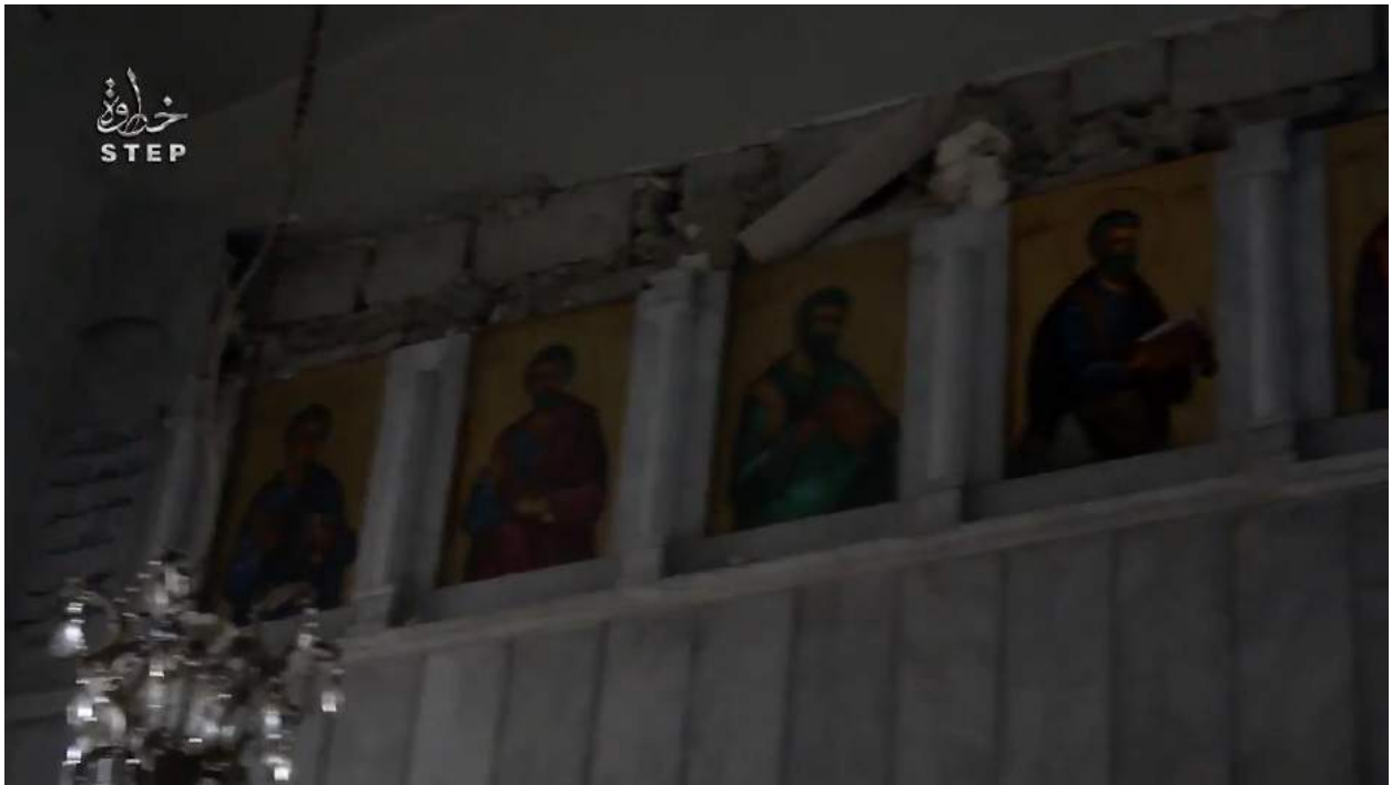
Video still of damage to the Church of Mary (Step News Agency; December 26, 2016)
