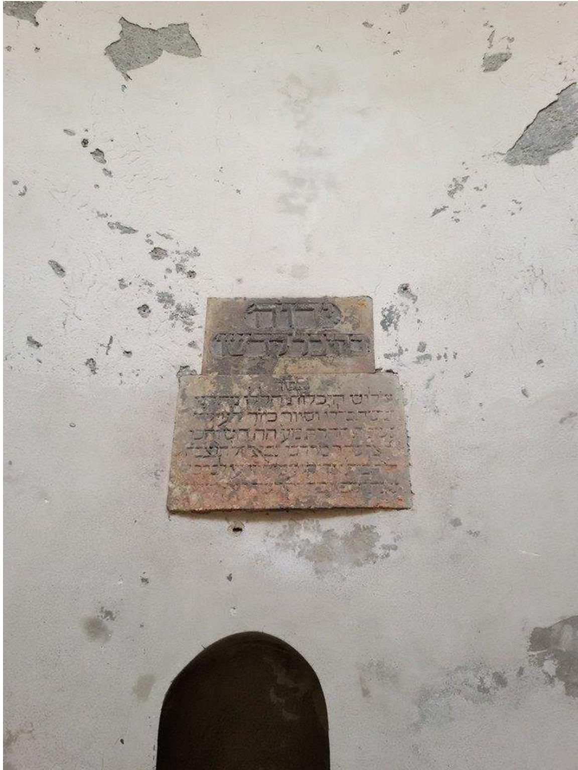
Damage to Bandara Synagogue (Private Facebook Account; December 17, 2016)
