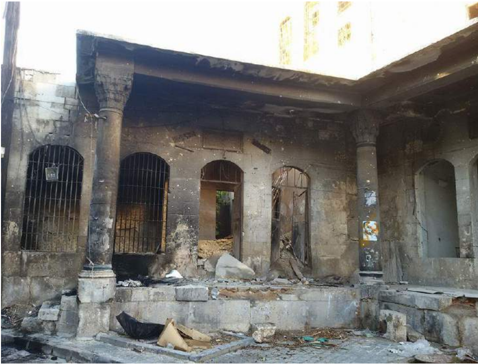
Fire and explosives damage to the Bab al-Nasr area (Private Facebook Account; December 15, 2016)
