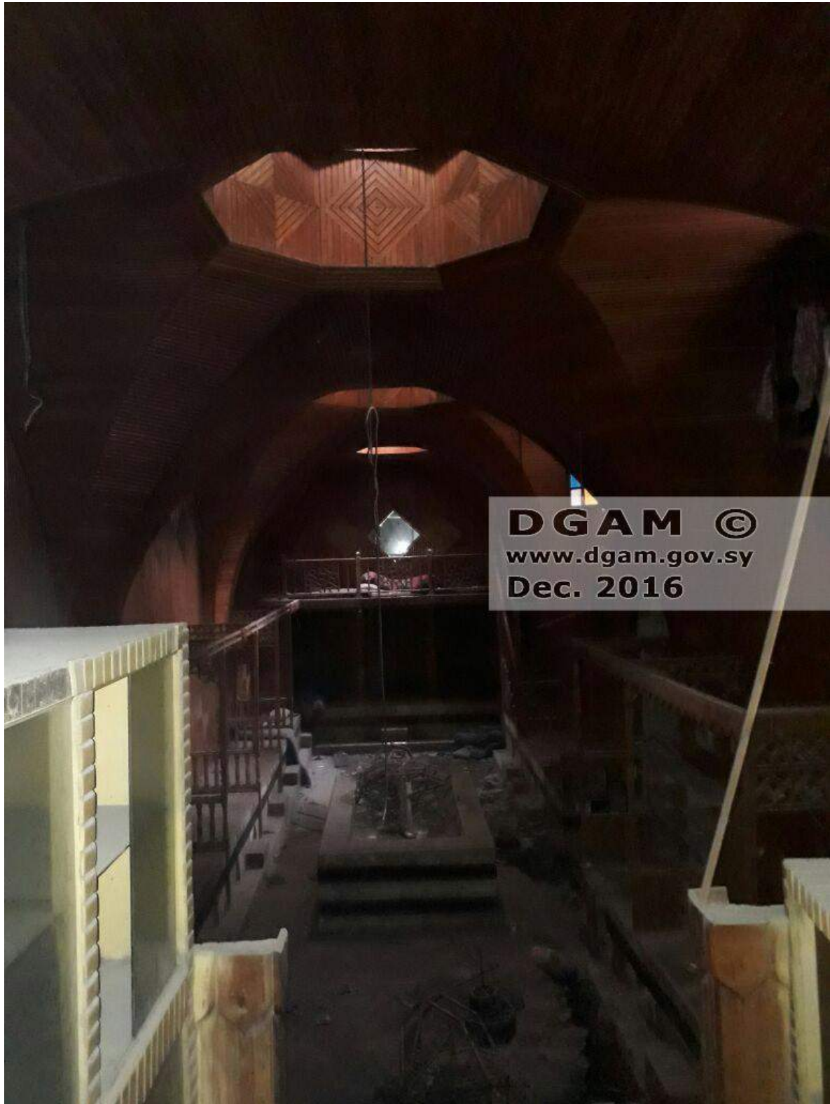
Damage to the interior of Hammam al-Nahasin (DGAM; December 16, 2016)
