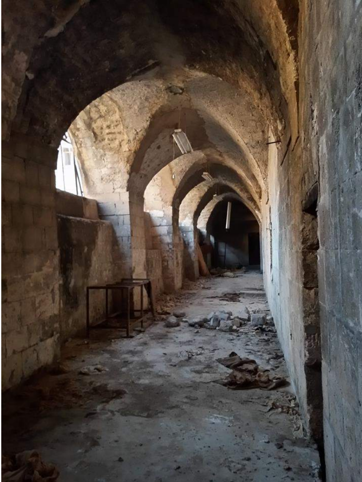
Damage to the interior hall of Musabnat al-Jabili (Private Facebook Account; December 19, 2016)
