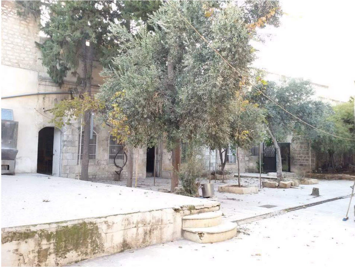
Minimal damage to the exterior of al-Mustadamiya Mosque (Private Facebook Account; December 20, 2016)
