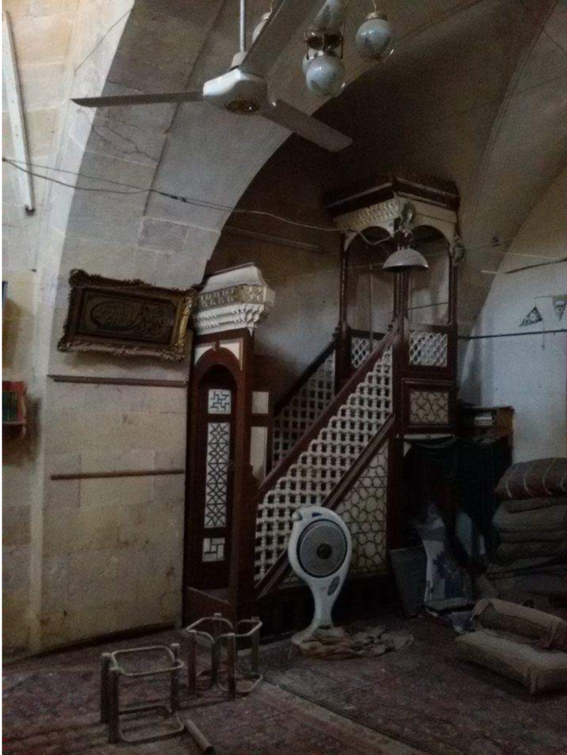
Minimal damage to the interior and minbar of al-Mustadamiya Mosque (Private Facebook Account; December 20, 2016)
