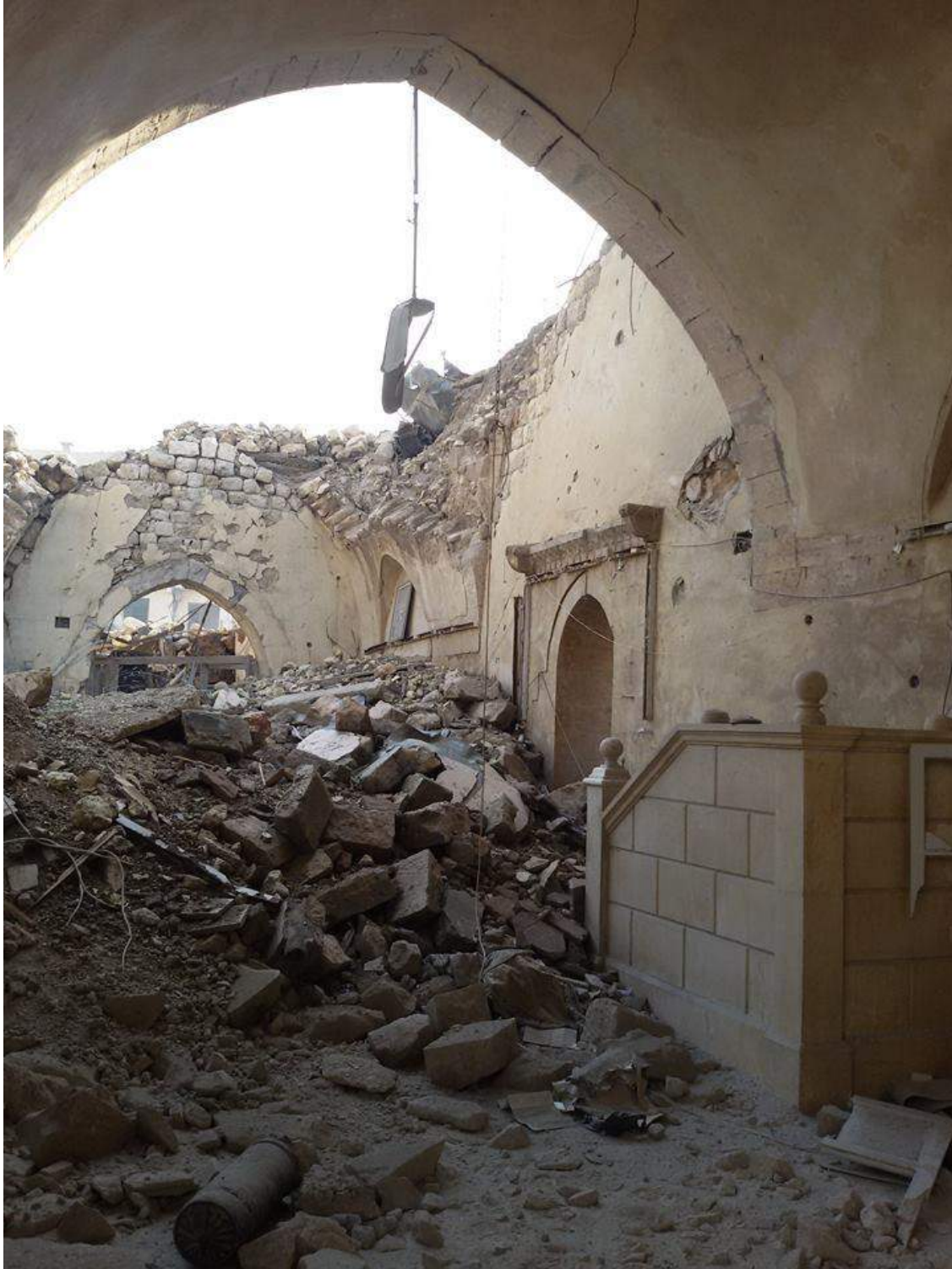
Extensive damage, including a collapsed roof, at al-Maidani Mosque (Private Facebook Account; December 19, 2017)
