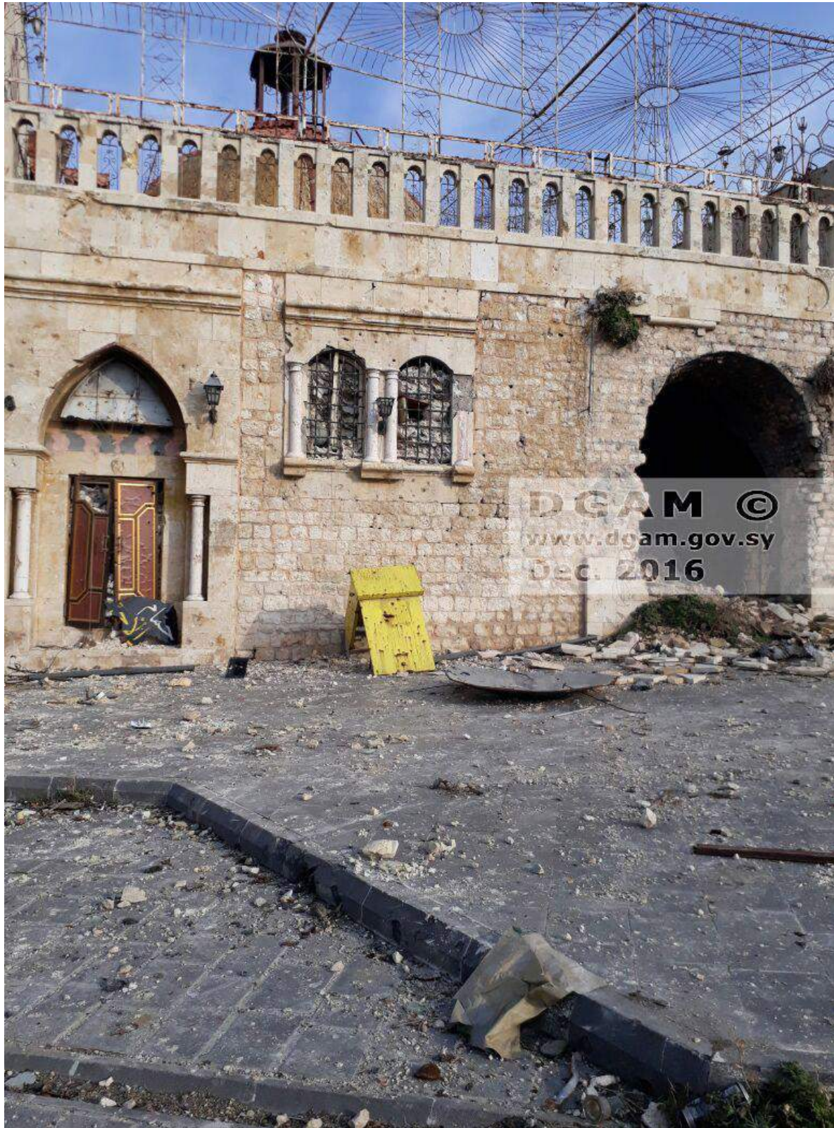
Damage to the exterior of Hammam Bab al-Ahmar (DGAM; December 24, 2016)
