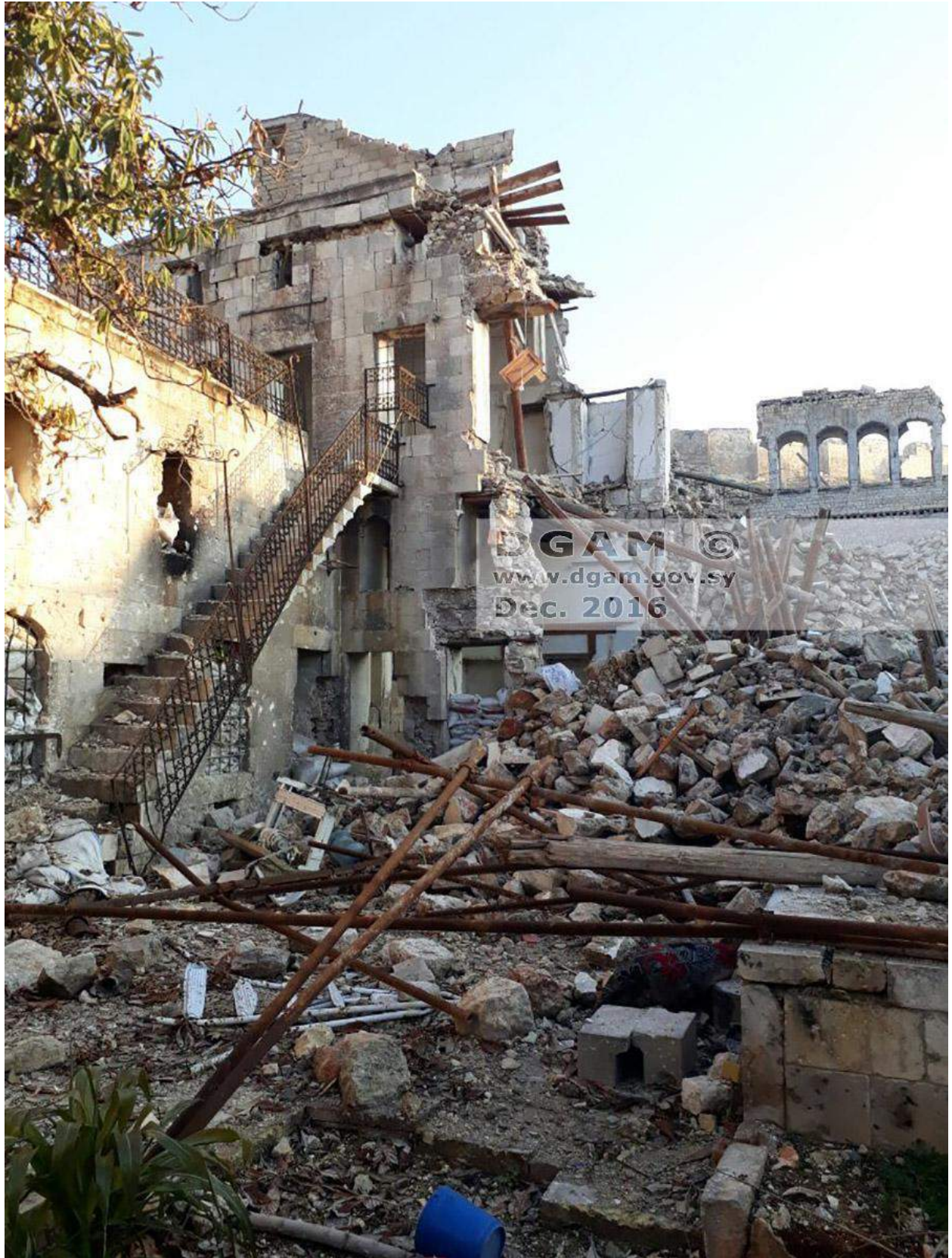
Damage to the exterior of Dar Qatar Agassi (DGAM; December 20, 2016)
