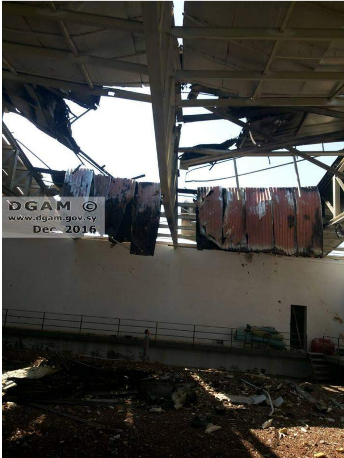
Extensive damage to Tayyibet al-Imam (DGAM; December 20, 2016)
