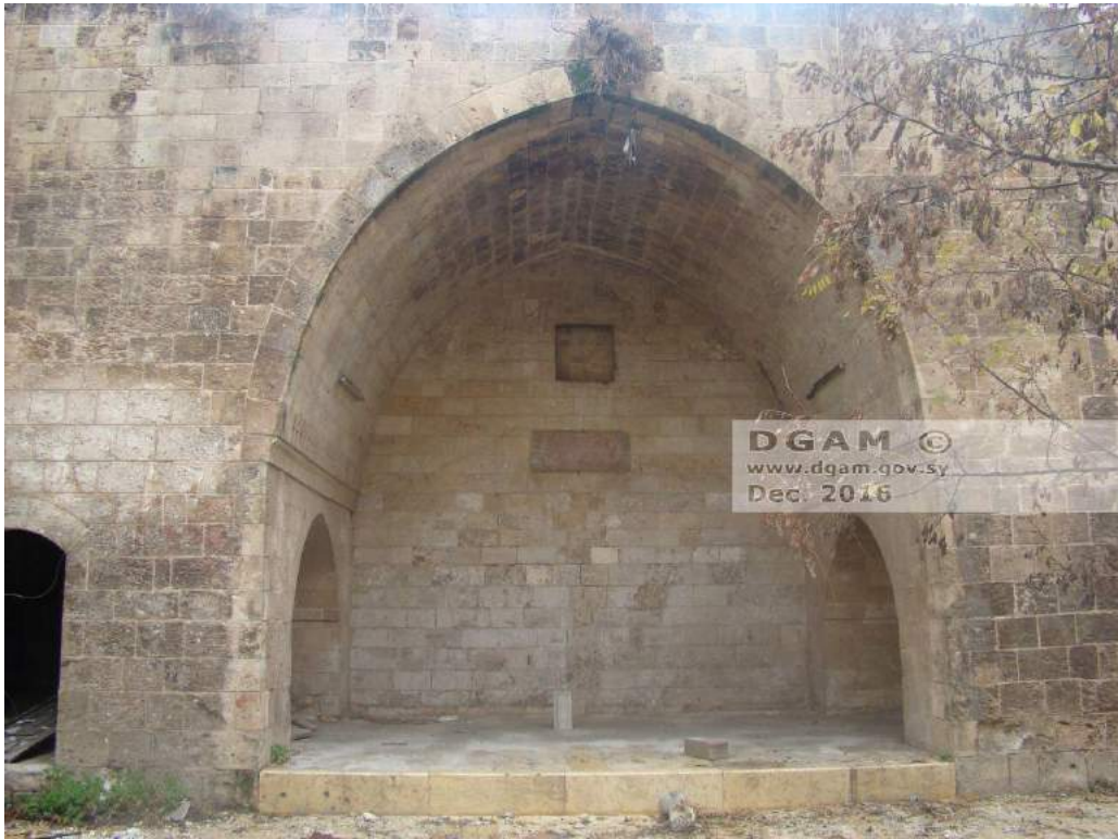
Minor damage to Bimaristan Nur al-Din (DGAM; December 31, 2016)
