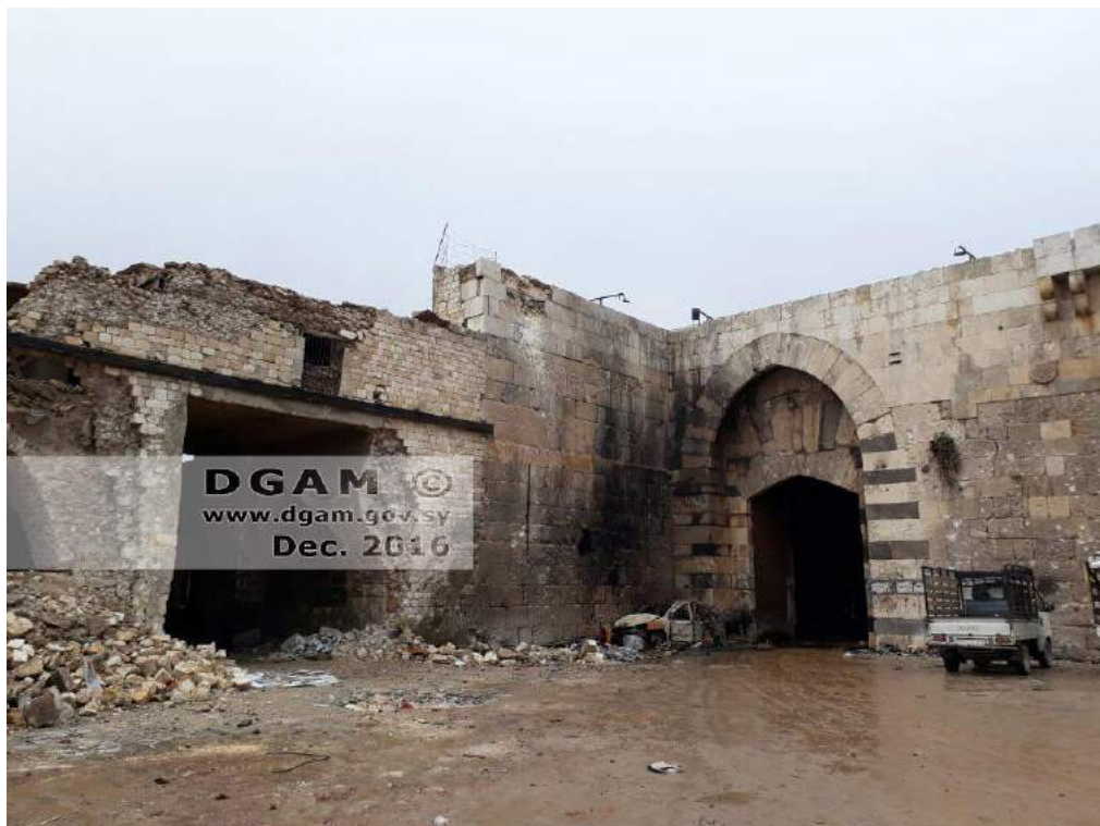
Collapsed wall and smoke damage to the exterior of Bab Qinnasrin (DGAM; December 24, 2016)
