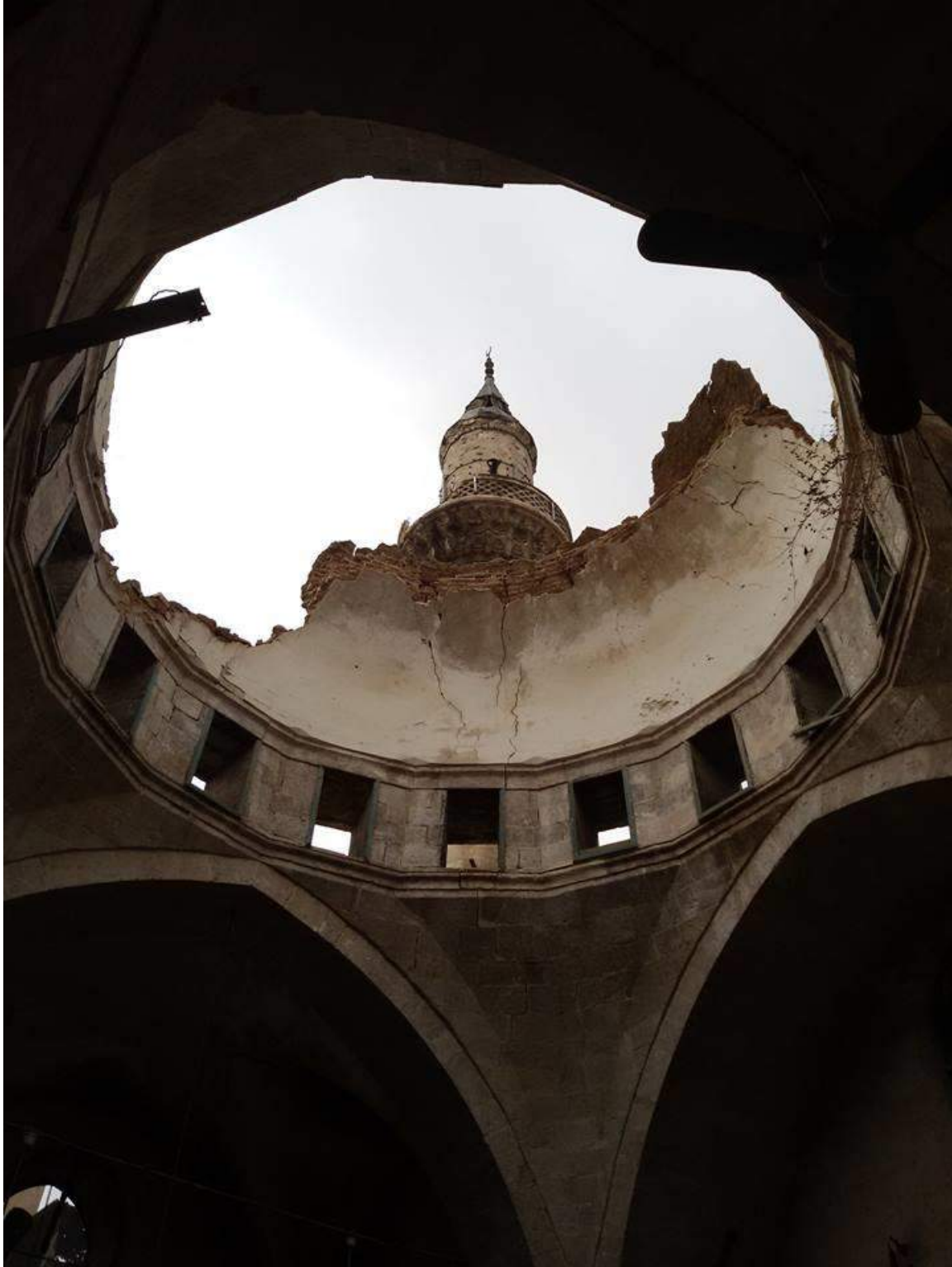
The collapse of the dome at Hajj Musa al-Amiri Mosque (Private Facebook Account; December 17, 2016)
