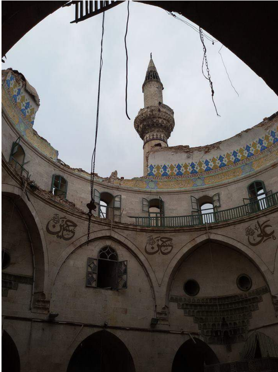
Damage to the dome of the Adliyah Mosque (Private Facebook Account; December 17, 2016)
