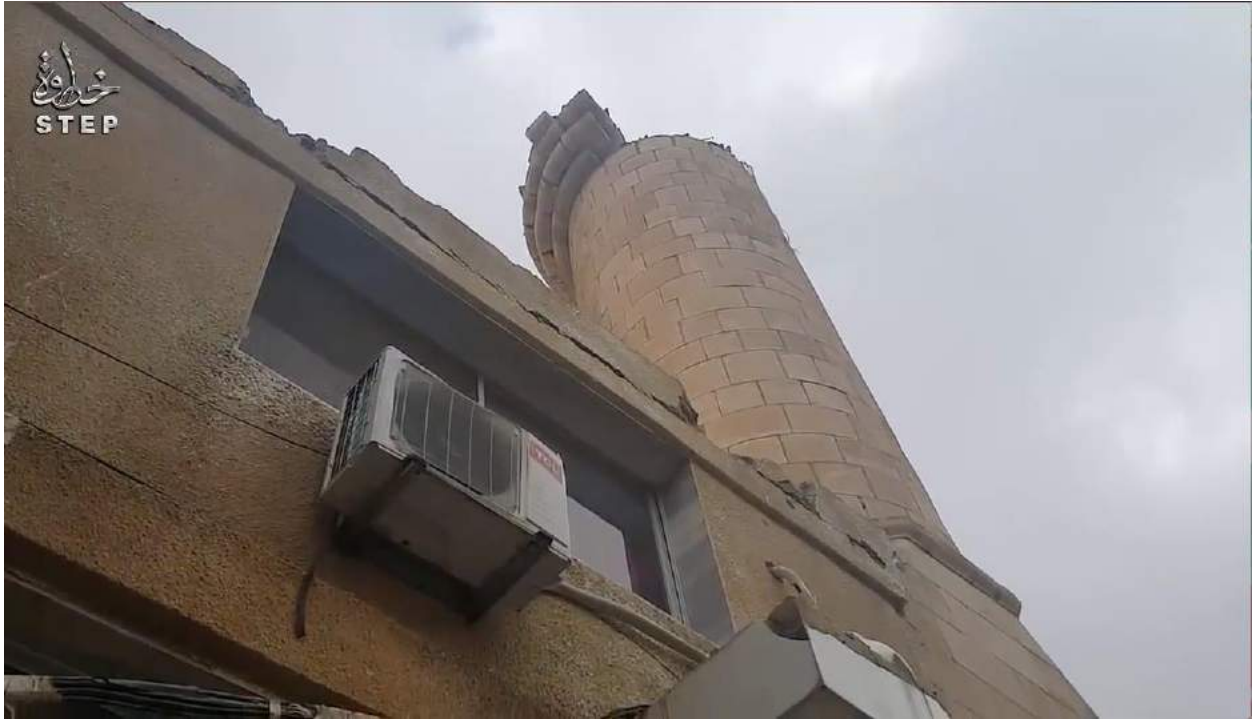
Video still of damage to the minaret at al-Husseiniya Village Mosque (Step News Agency: December 26, 2016)
