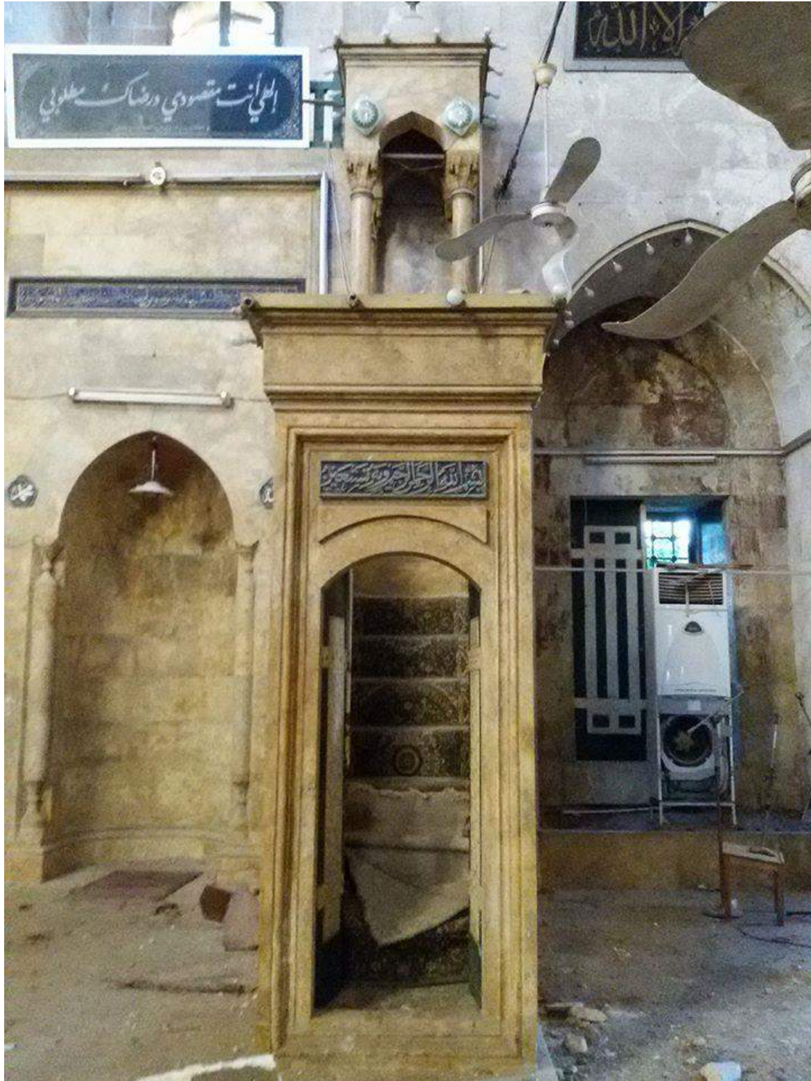
The largely undamaged mihrab and minbar of al-Uthmaniya Mosque (Private Facebook Account; December 15, 2016)
