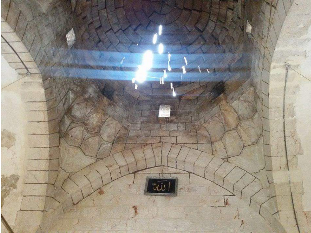
Possible light damage to the dome of Mosque and Madrasa Turuntaiya (Private Facebook Account; December 22, 2016)
