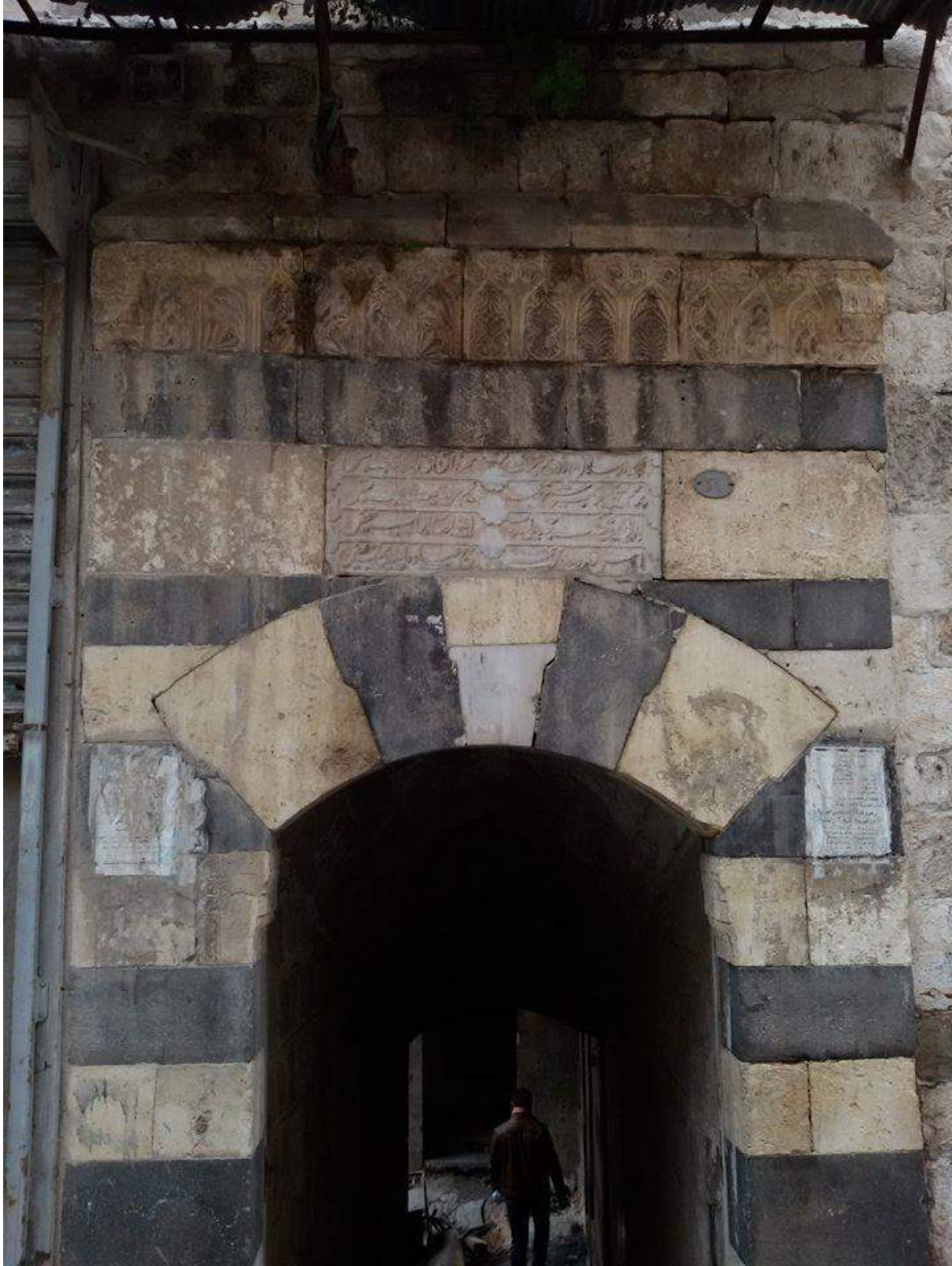
Damage to the facade of Khan al-Wazir (Private Facebook Account; December 17, 2016)
