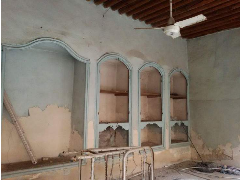
Damage to Old Arab House in Aleppo (Private Facebook Account; December 19, 2016)
