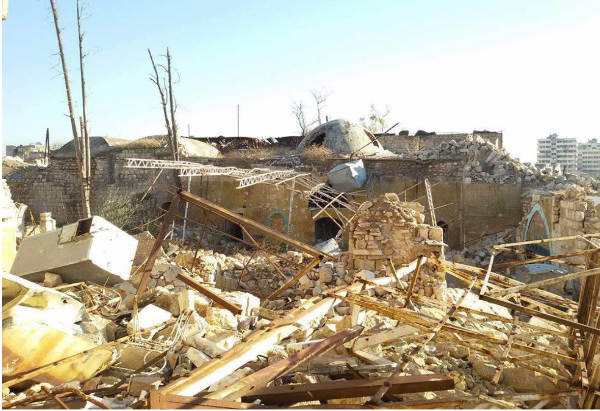
Extensive damage to Sharaf Mosque (Private Facebook Account; December 15, 2016)
