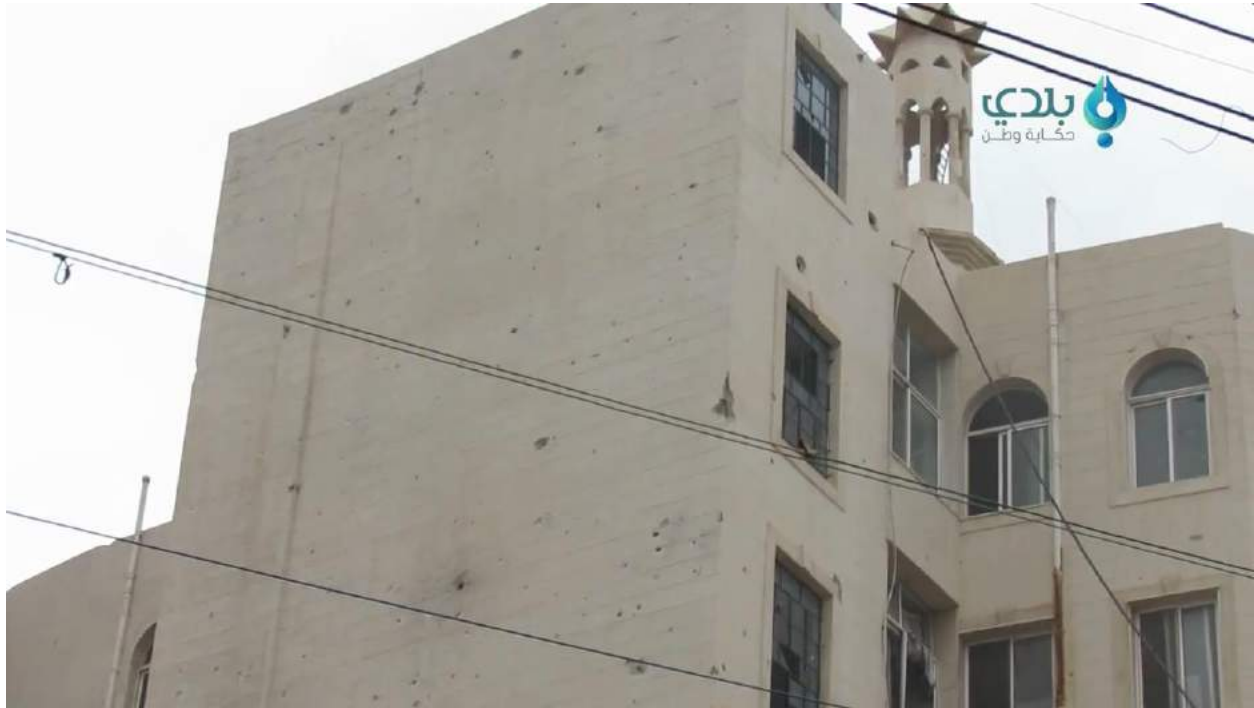
Video still of damage to al-Kabir Mosque (Baladi News; December 27, 2016)
