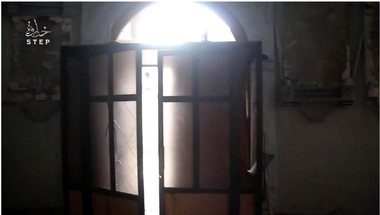
Video still of damage to the Church of Mary (Step News Agency; December 26, 2016)
