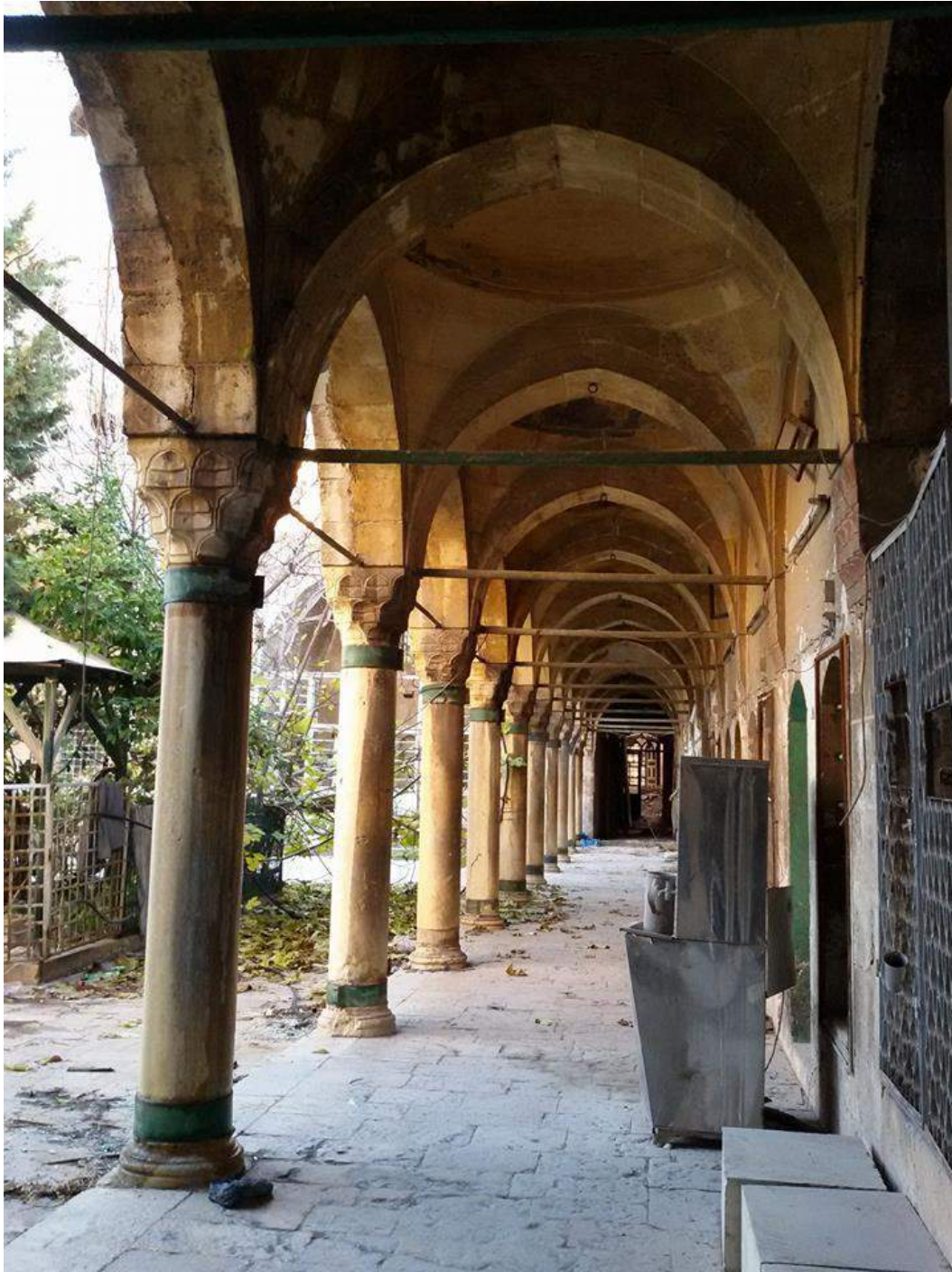
Damage to the courtyard of al-Uthmaniya Mosque (Private Facebook Account; December 15, 2016)
