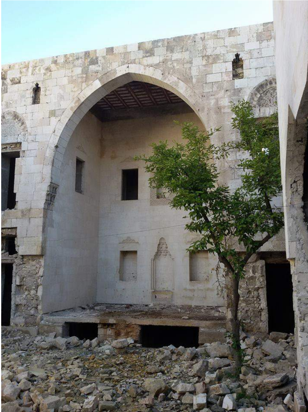
Extensive damage to Hotel Zamaria (Private Facebook Account; December 17, 2016)
