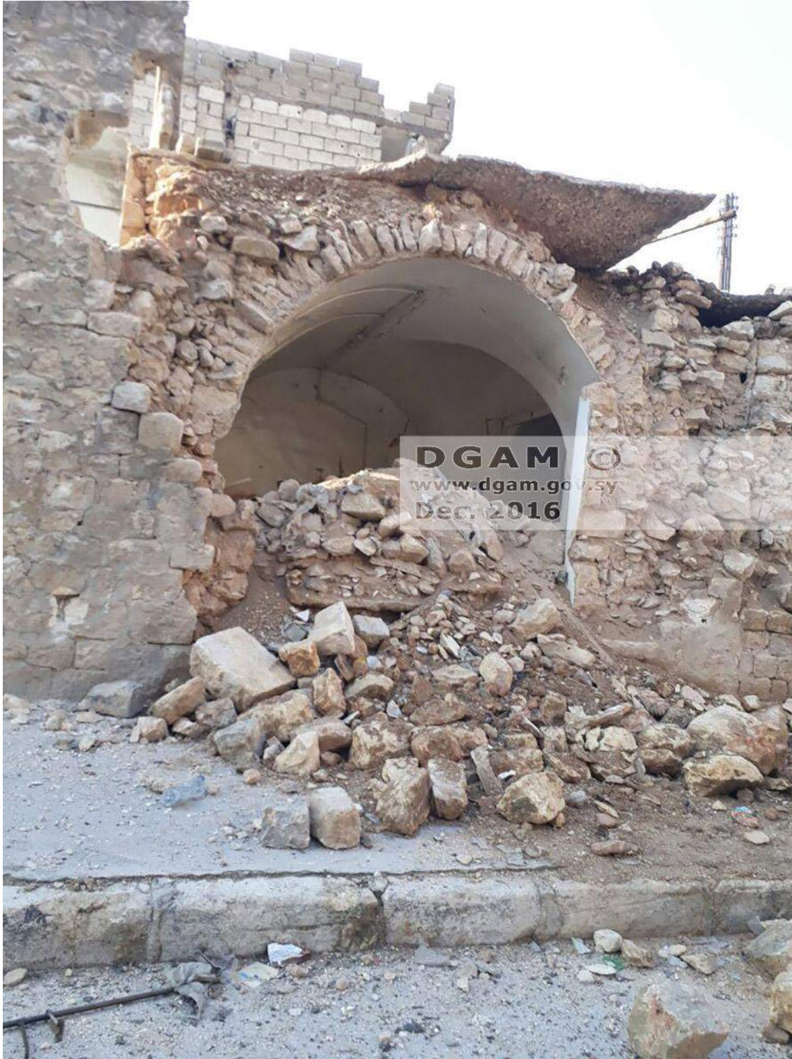
Structural damage to Jabri School (DGAM; December 20, 2016)
