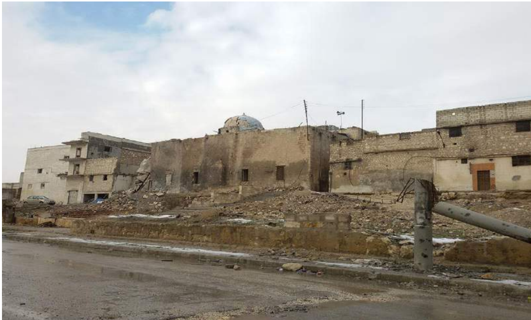
Damage to the exterior of Mosque and Madrasa Turuntaiya (Private Facebook Account; December 22, 2016)
