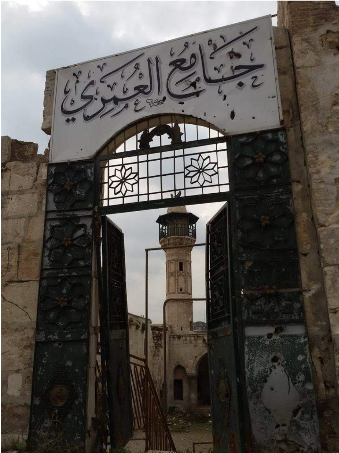
The entrance to al-Omari Mosque, showing overgrowth and damage in the courtyard as well as evidence of bullet holes in the facade (Private Facebook Account; December 17, 2016)
