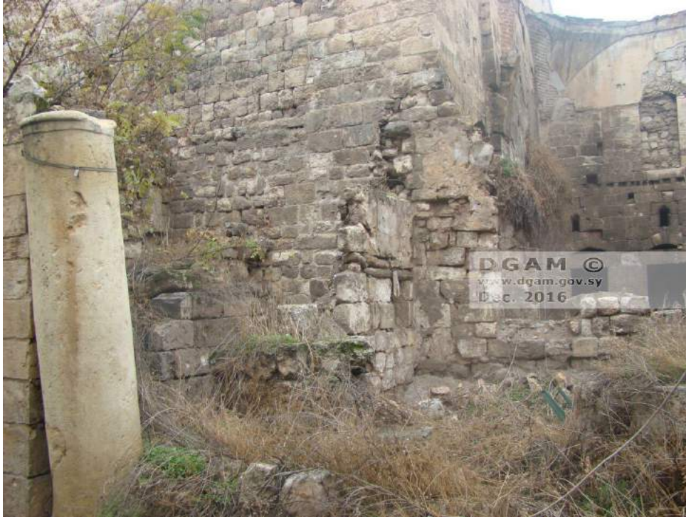
Moderate damage and overgrowth of vegetation at Bimaristan Arghun al-Kamili (DGAM; December 31, 2016)
