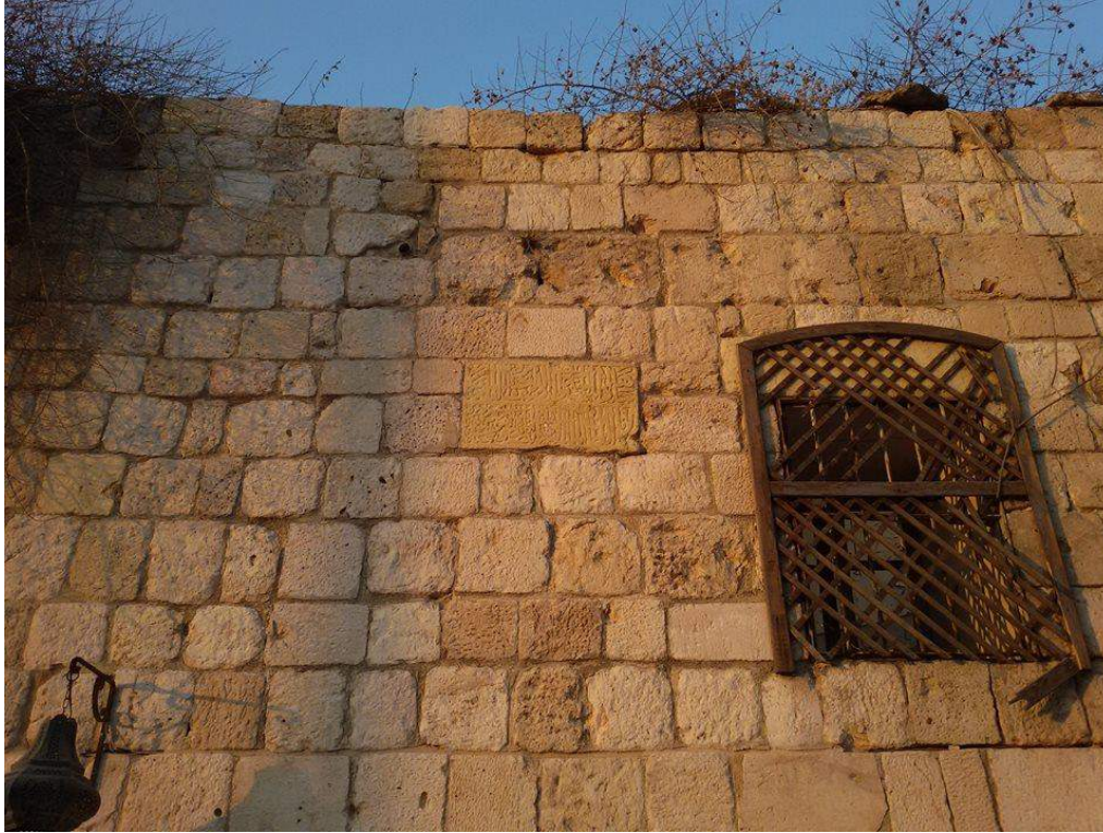
Vegetation overgrowth at Takkiya Nasimi (Private Facebook Account; December 19, 2016)
