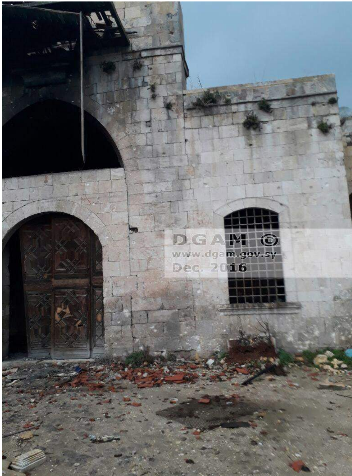
Damage to the exterior of the Khan al-Shouneh (DGAM; December 28, 2016)
