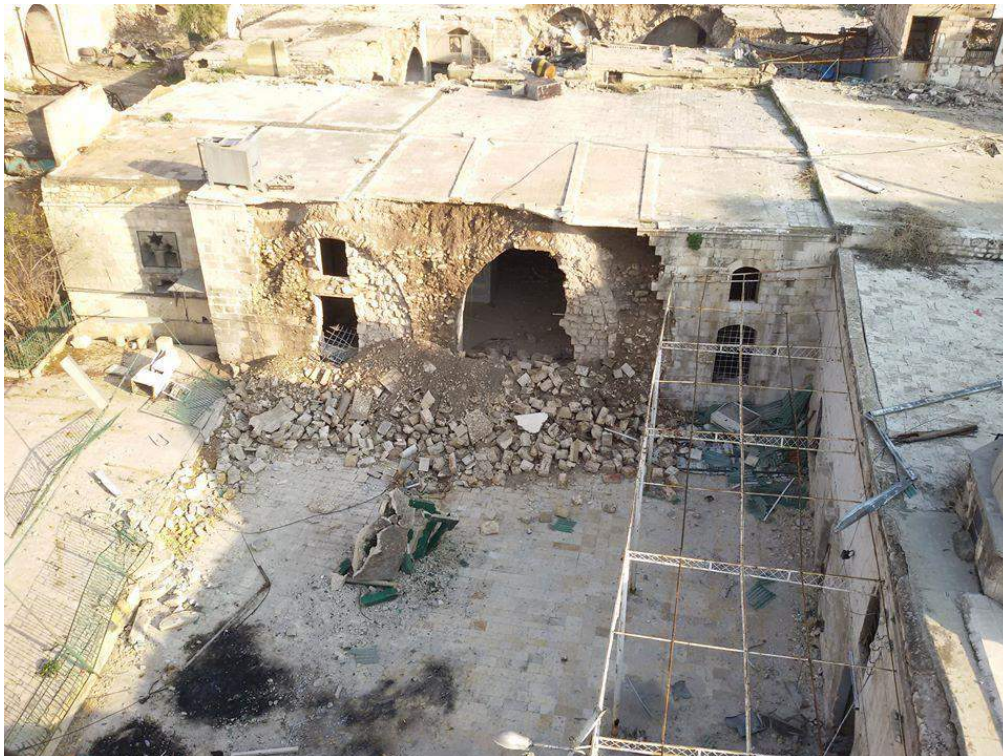
The collapsed facade of outer wall at al-Zaki Mosque (Private Facebook Account; December 19, 2016)
