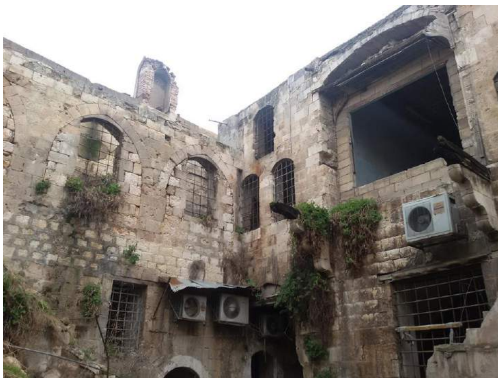
Vegetation on the walls of Khan al-Qassabiya (Private Facebook Account; December 24, 2016)
