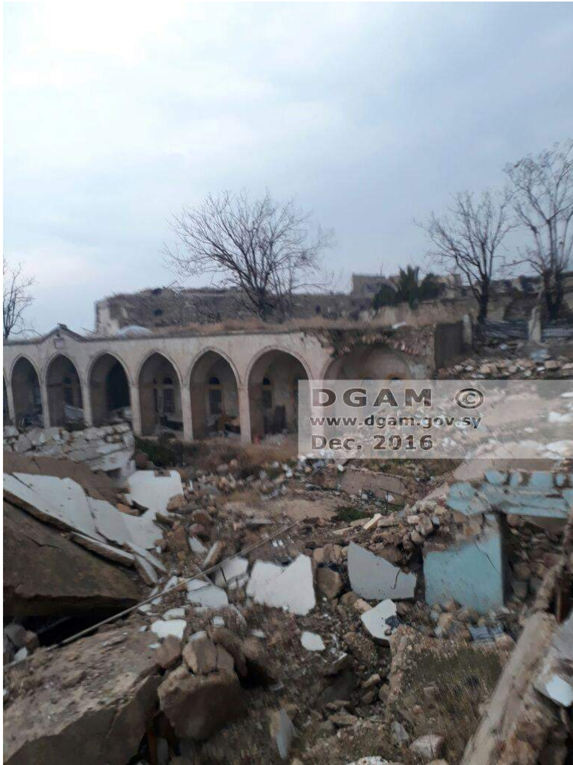
Extensive damage to Madrasa Khusruwiye (DGAM; December 28, 2016)
