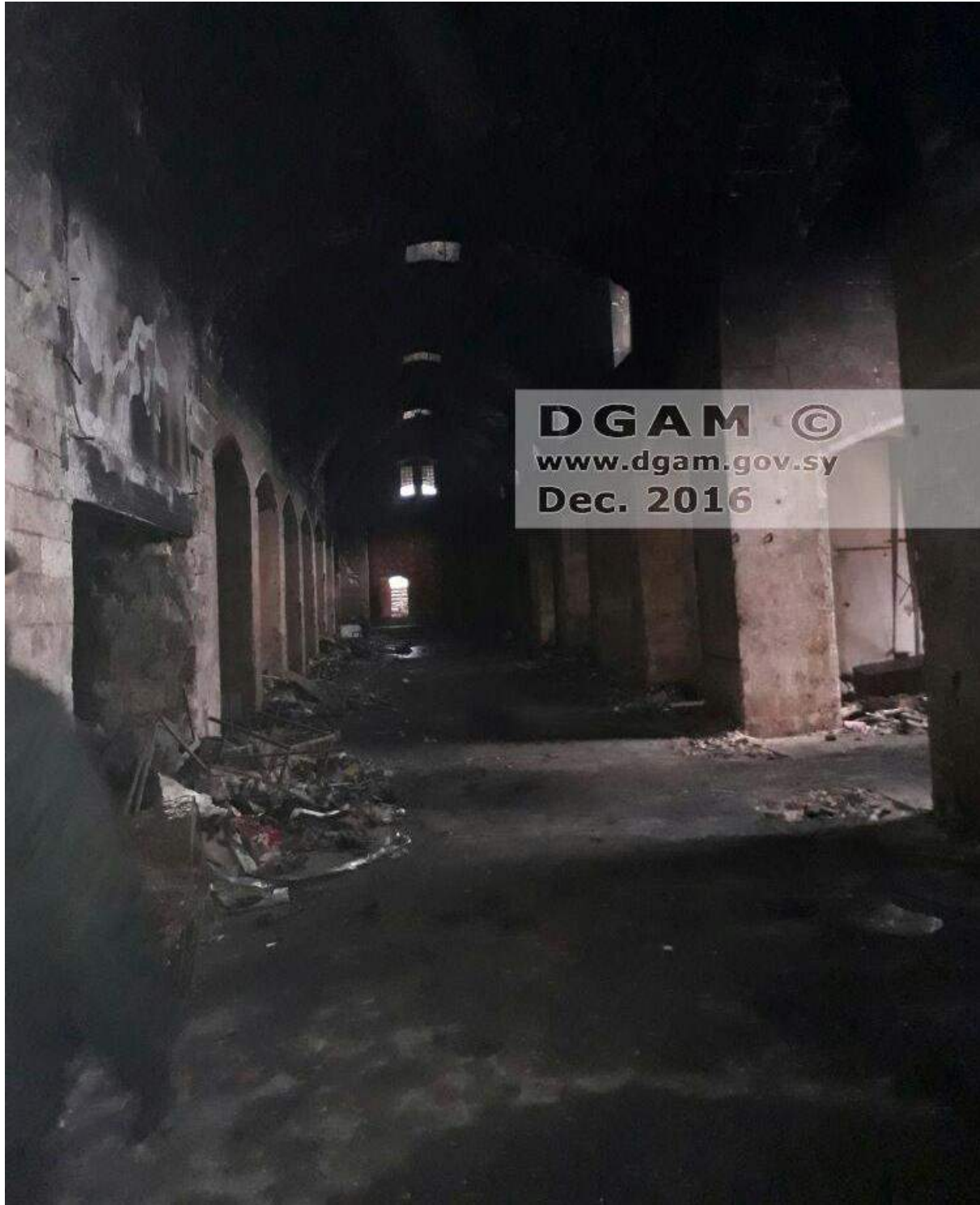
Damage to the interior of the Khan al-Shouneh (DGAM; December 28, 2016)
