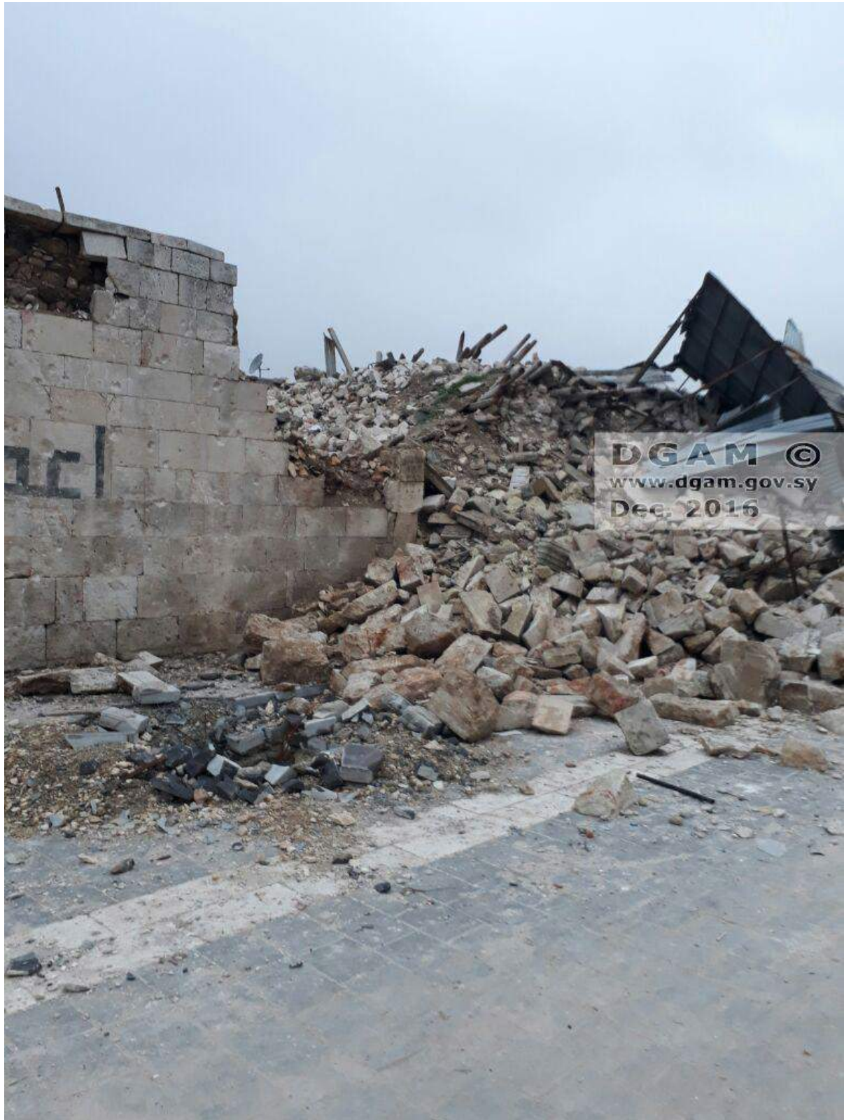
Collapse of the exterior wall of al-Zahrawi School (DGAM; December 25, 2016)
