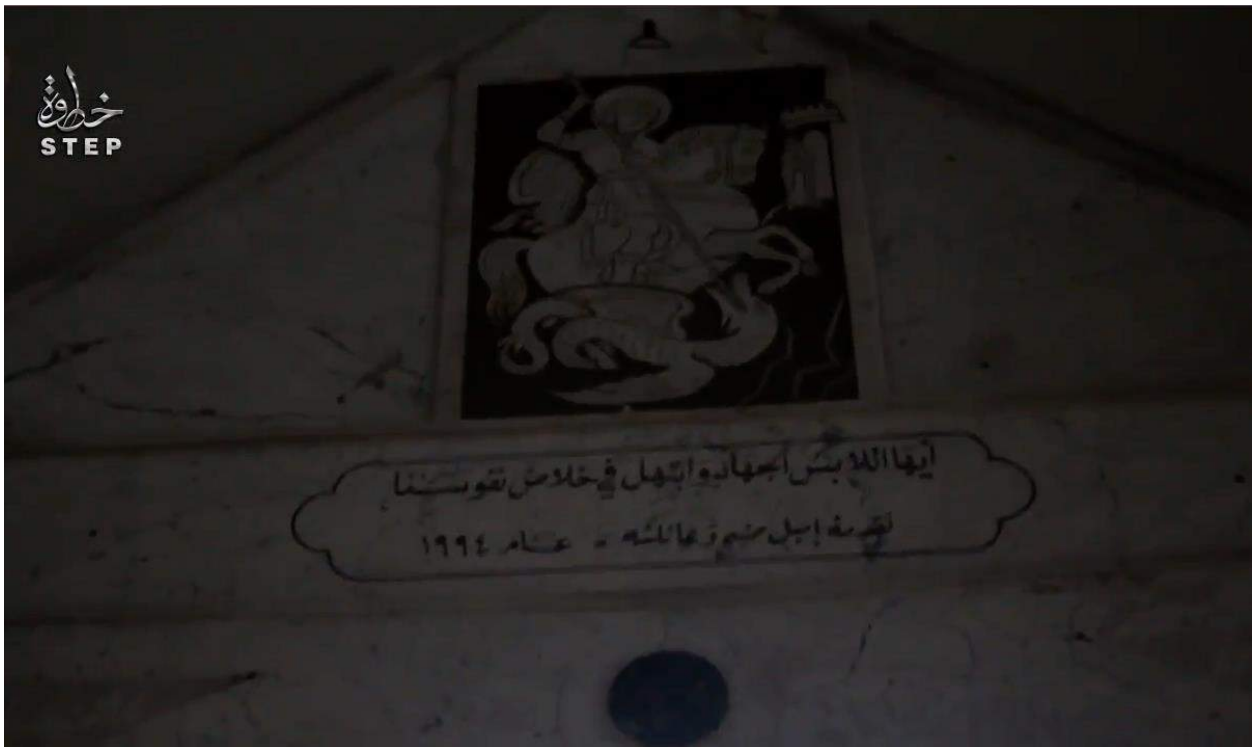
Video still of damage to the Church of Mary (Step News Agency; December 26, 2016)
