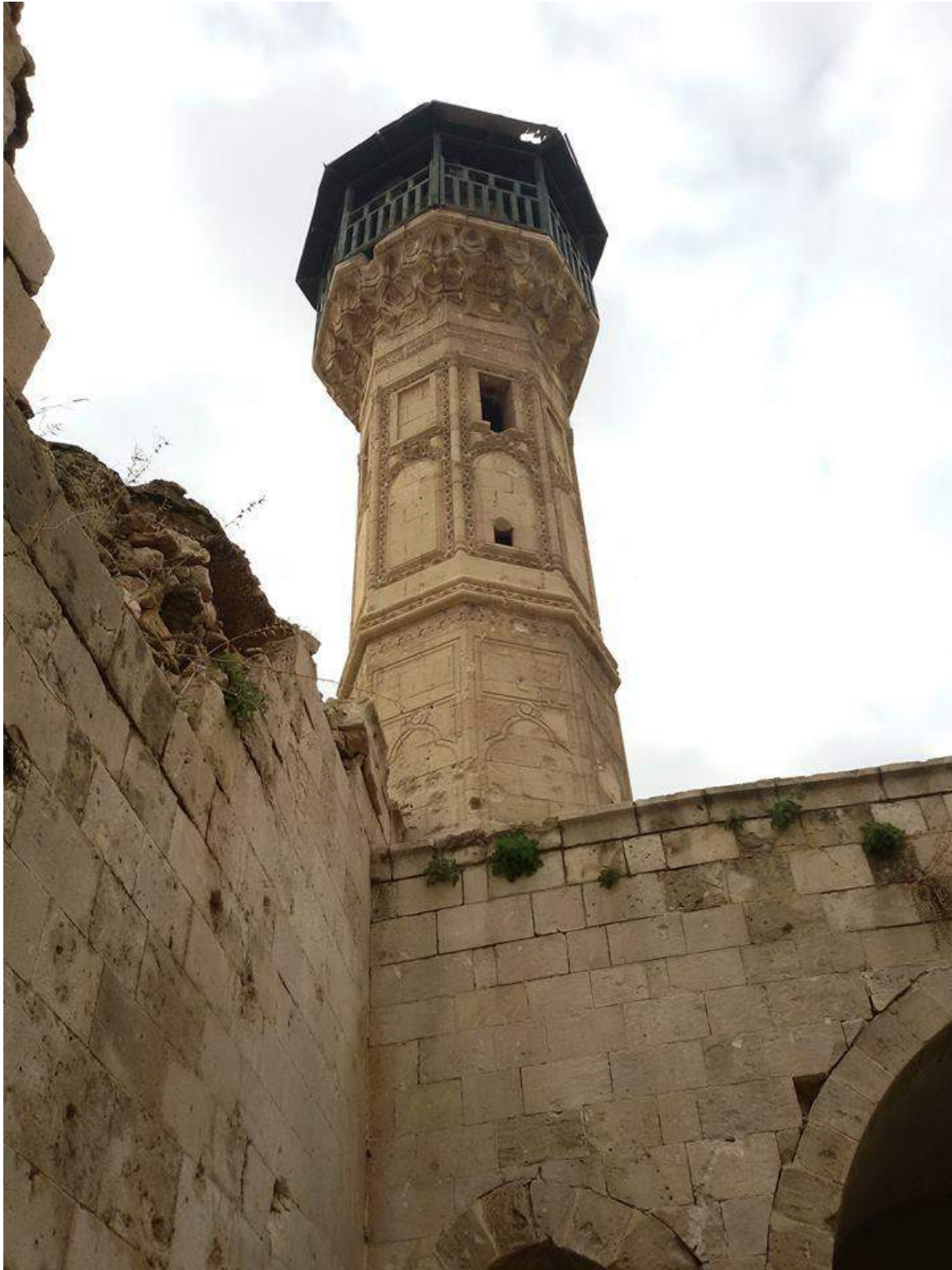
Light damage to al-Omari Mosque, including overgrowth (Private Facebook Account; December 17, 2016)
