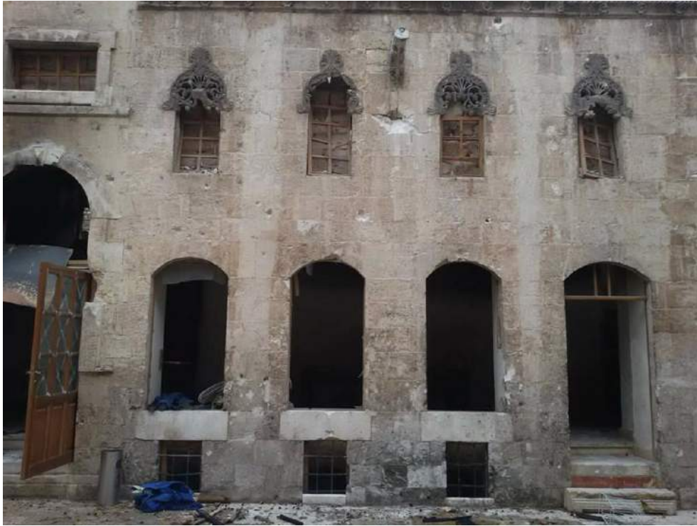
Explosives damage to al-Shibani Church and School (Private Facebook Account; December 24, 2016)
