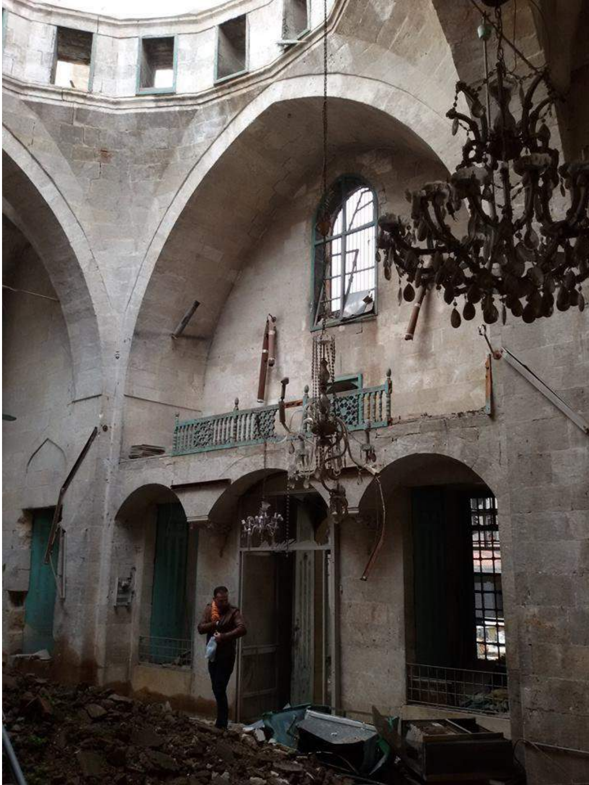
Damage seen to the interior of Hajj Musa al-Amiri Mosque (Private Facebook Account; December 17, 2016)
