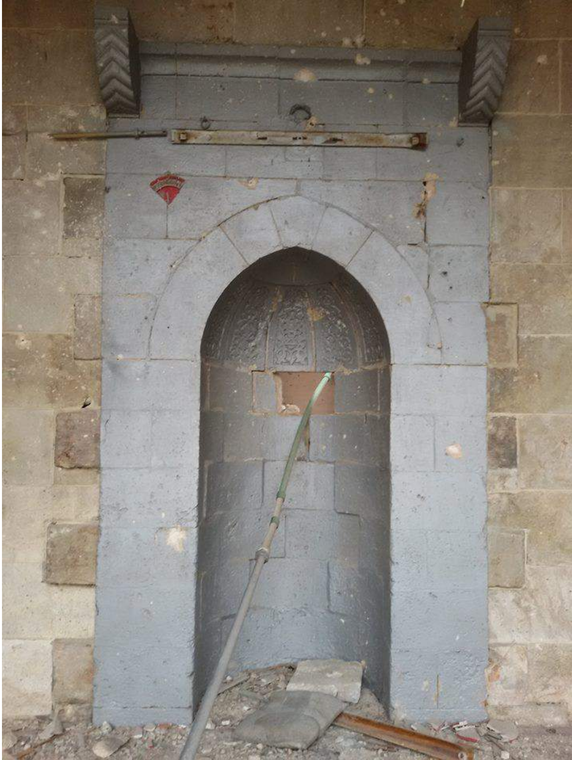
Damage to the mihrab at Dabbagha al-'Atiqa Mosque (Private Facebook Account; December 17, 2016)
