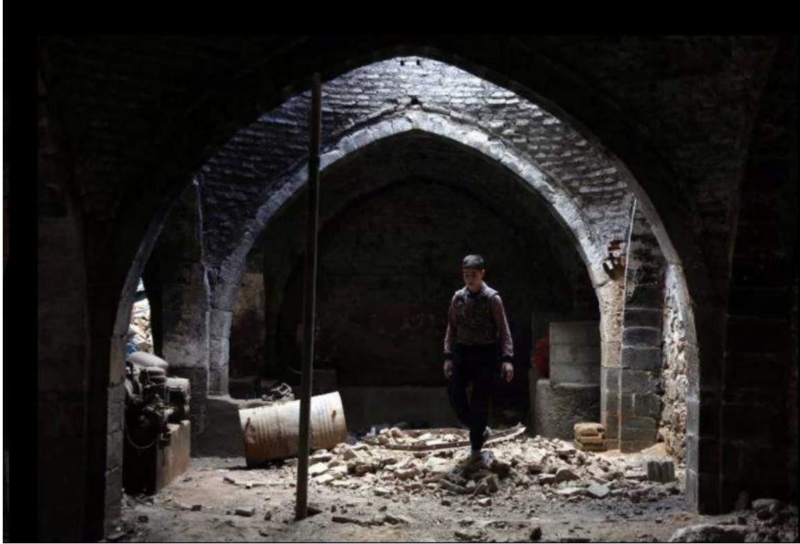
Extensive damage seen at Harasta Olive Oil Mill (Bisan Ilan Kurumu; November 22; 2016)
