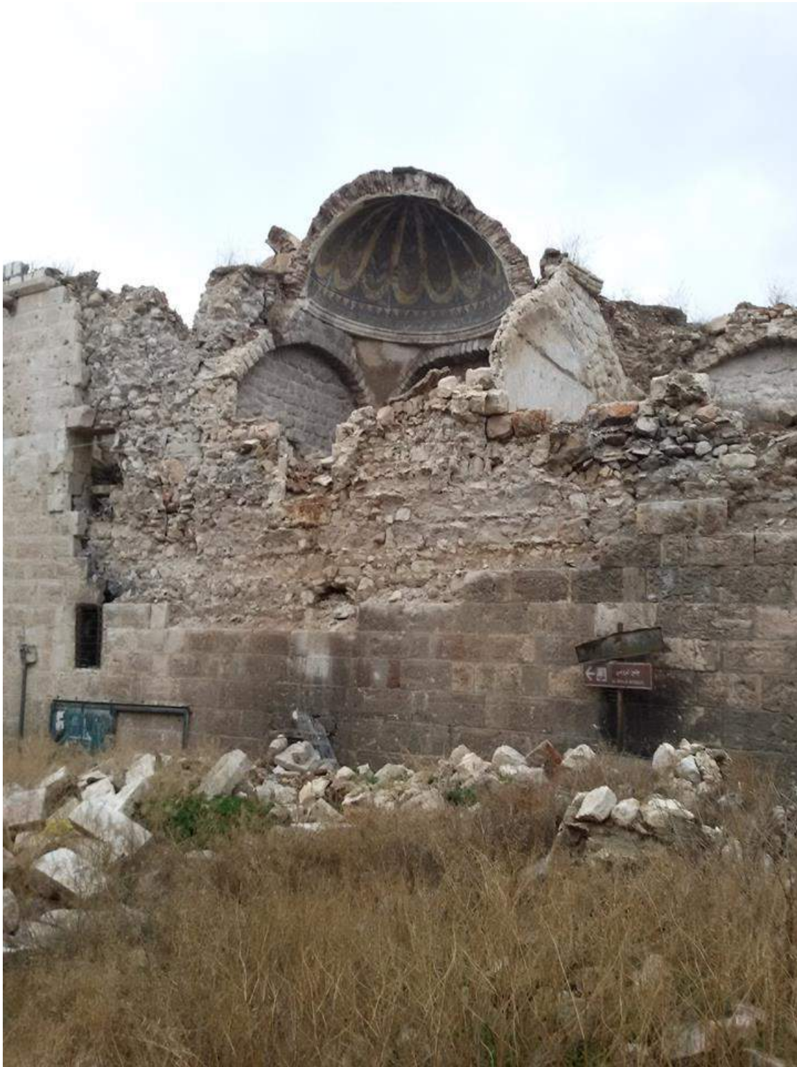
Extensive structural damage to Rumi Mosque (Private Facebook Account; December 17, 2016)
