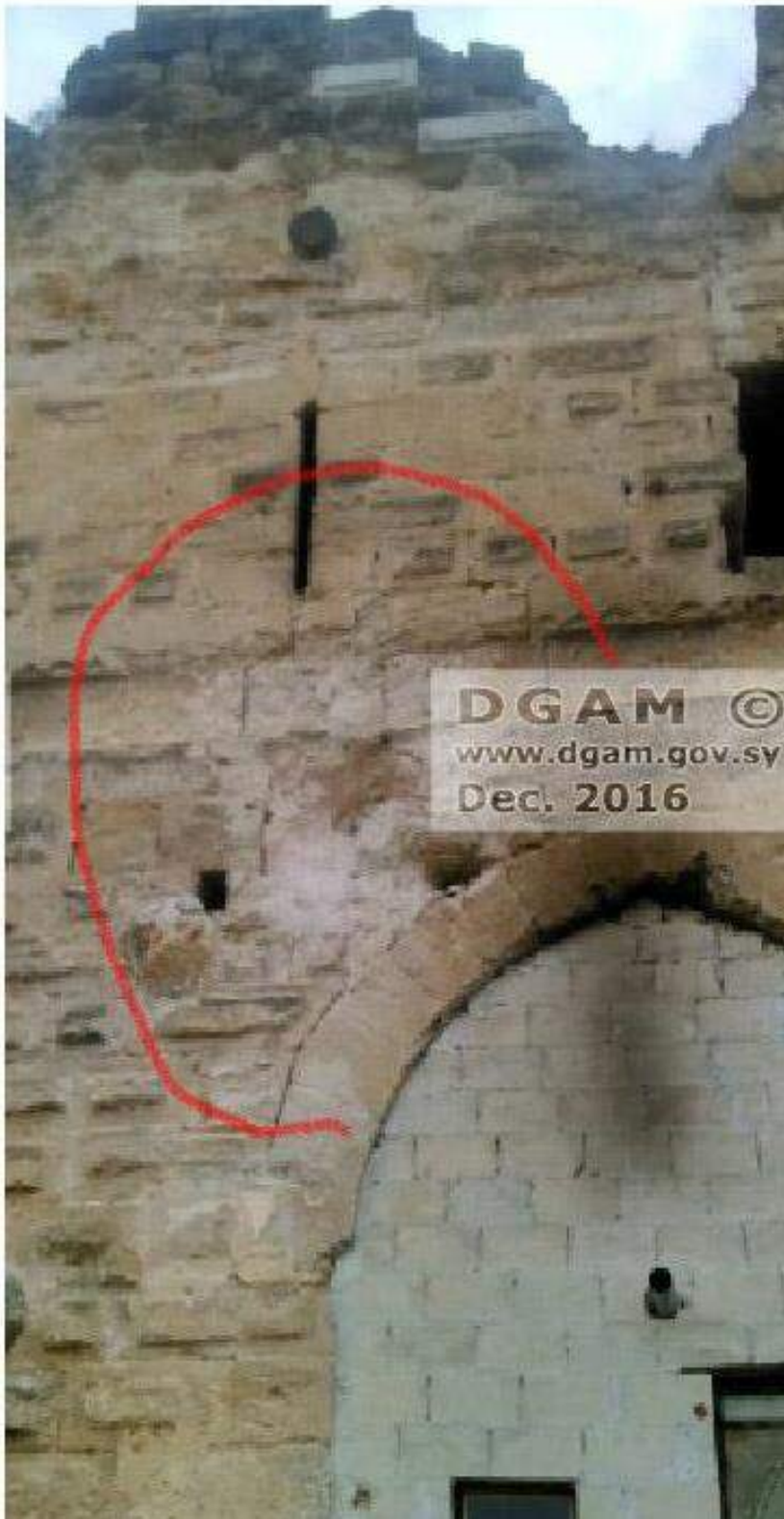
Mortar damage to the Shaizar Citadel (DGAM; December 20, 2016)
