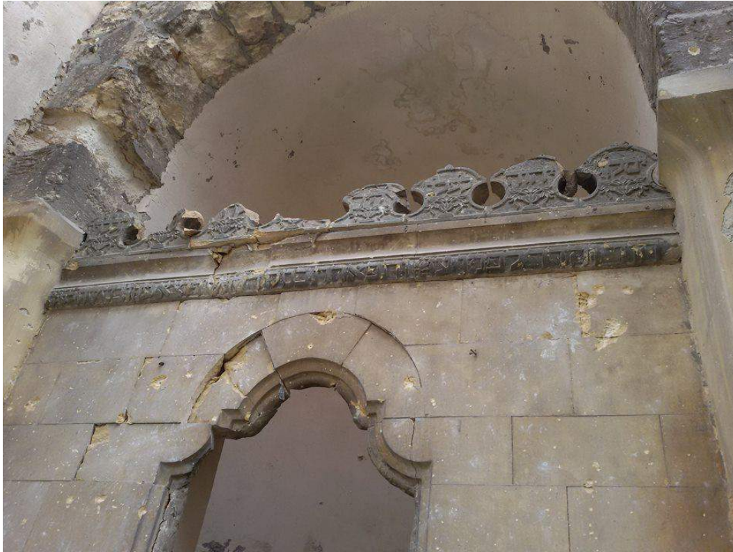
Damage to Bandara Synagogue (Private Facebook Account; December 17, 2016)
