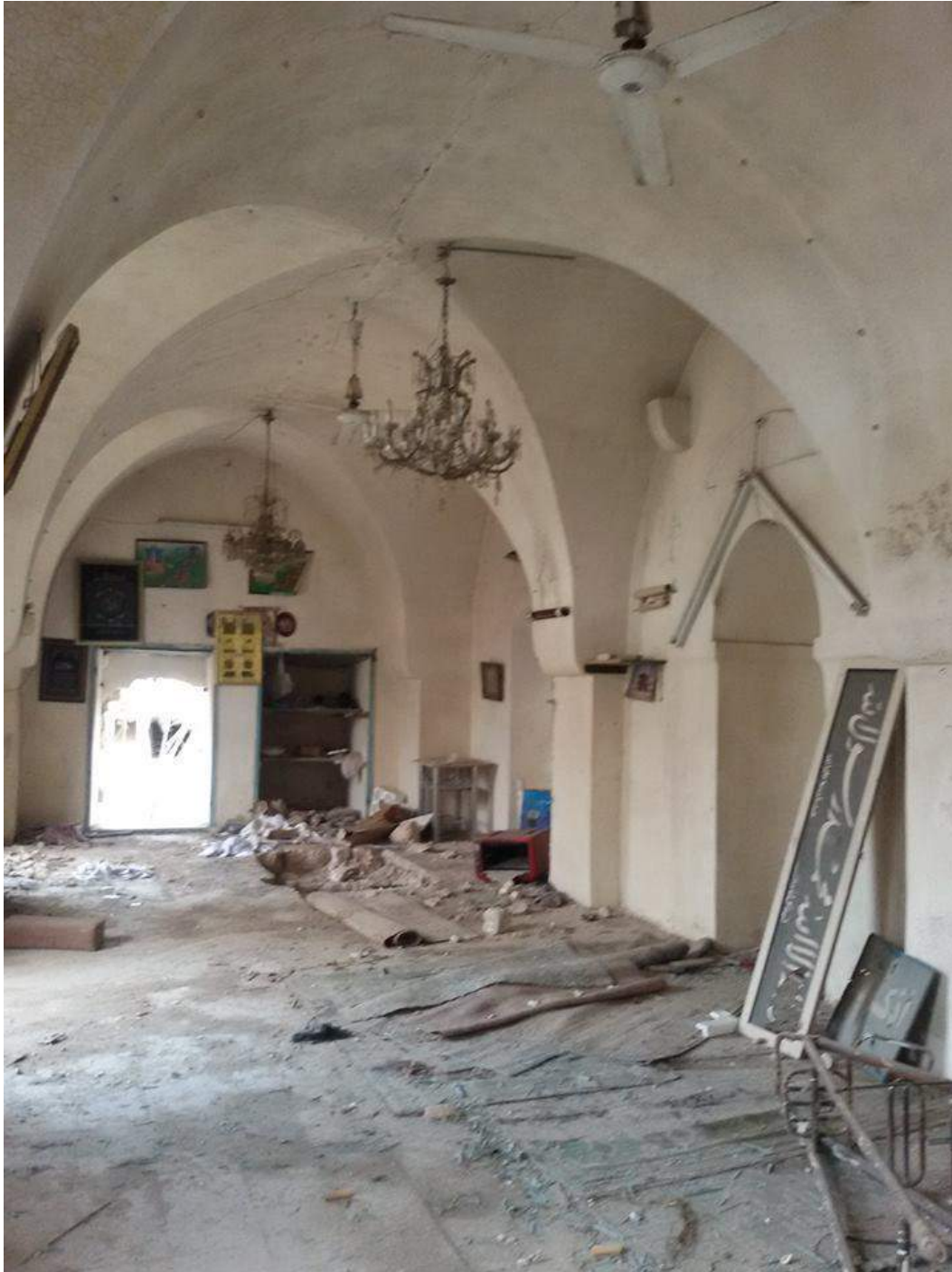
Damage to the interior of al-Arbaeen Mosque (Private Facebook Account; December 24, 2016)
