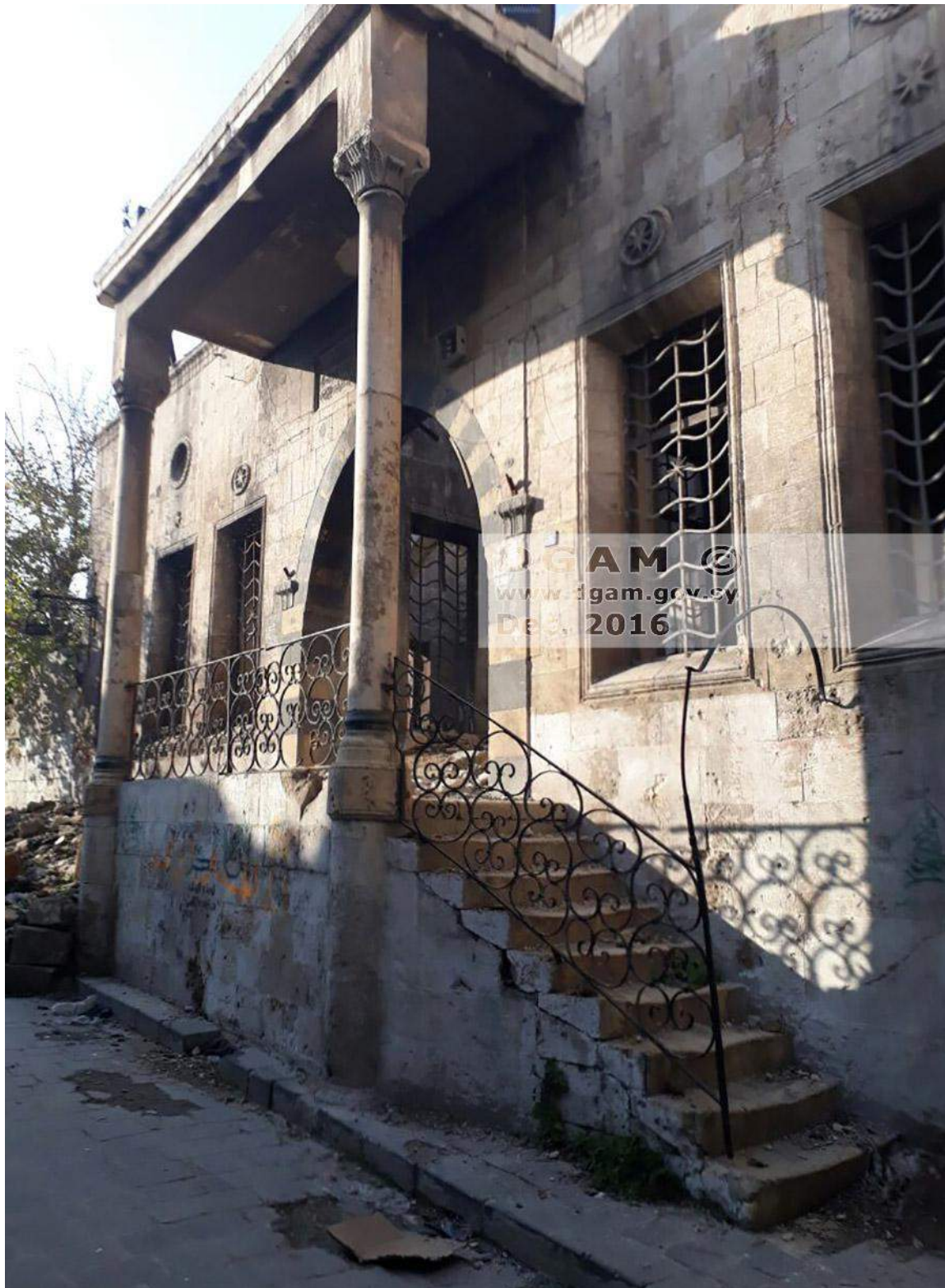
Exterior damage to the Police Station in Bab al-Hadid (DGAM; December 20, 2016)
