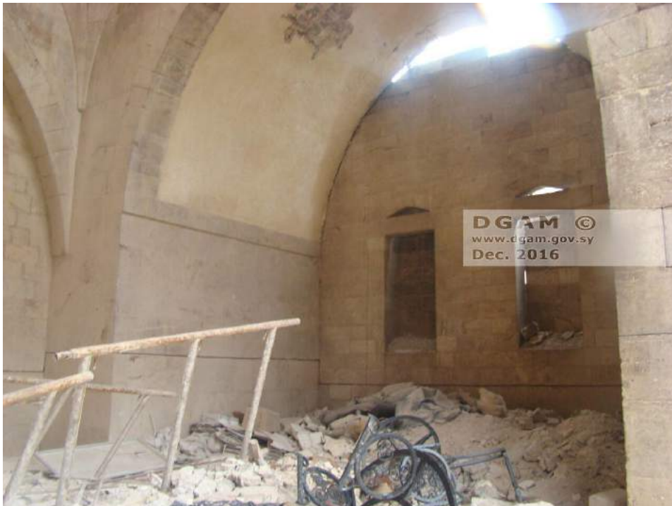
Damage and debris present at Bimaristan Arghun al-Kamili (DGAM; December 31, 2016)
