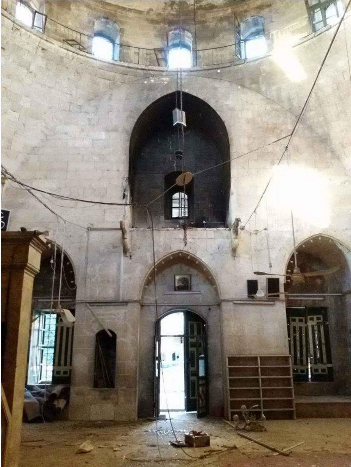
Damage to the interior of al-Uthmaniya Mosque (Private Facebook Account; December 15, 2016)
