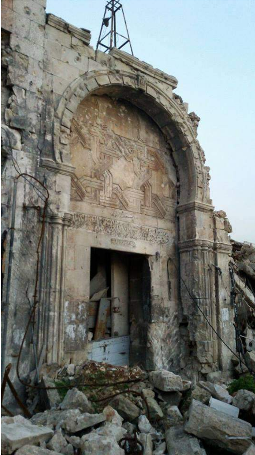
Extensive damage to Madrasa al-Sharafiya (Private Facebook Account; December 19, 2016)
