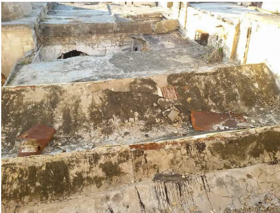
Damage to the roof of Musabinat al-Zanabli (Private Facebook Account; December 15, 2016)
