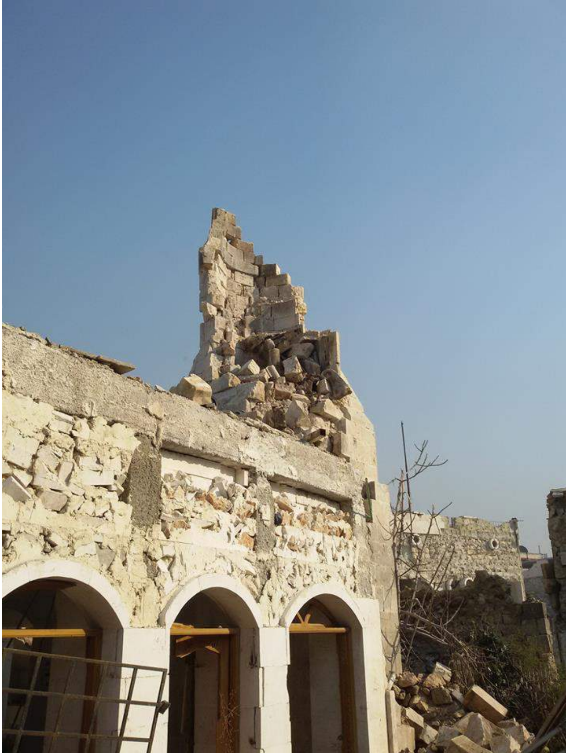
Extensive destruction of al-Maidani Mosque minaret (Private Facebook Account; December 19, 2017)
