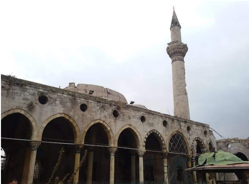
Damage, including a collapsed dome and damage to the courtyard of Adliyah Mosque (Private Facebook Account; December 17, 2016)
