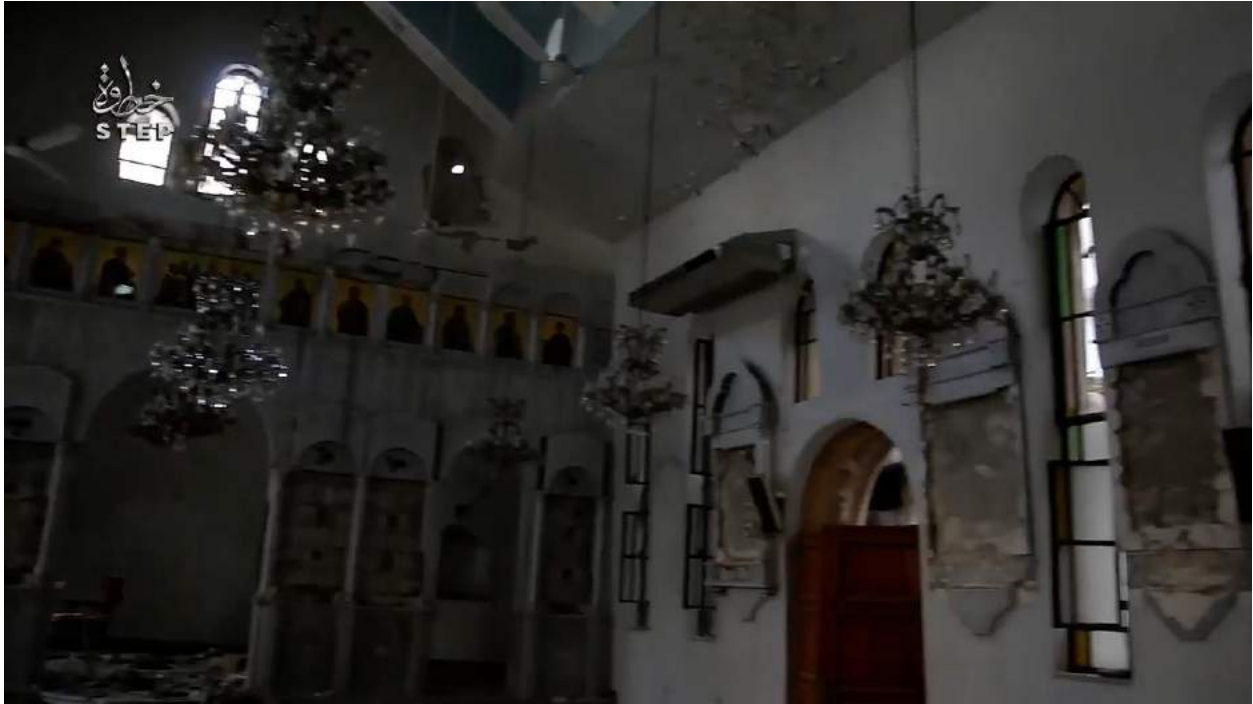
Video still of damage to Church of Mary (Step News Agency; December 26, 2016)
