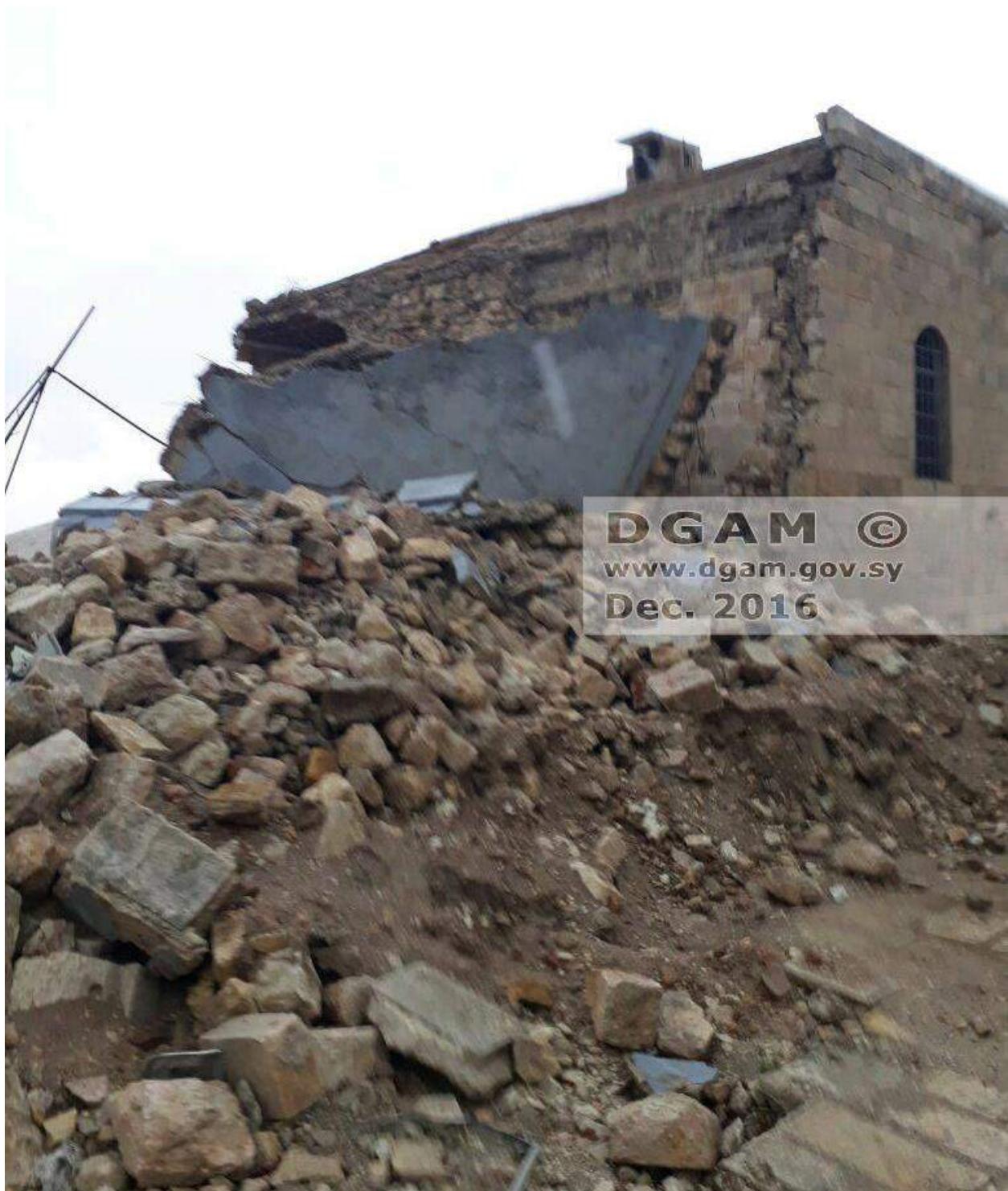
Collapse of the northwestern part of the museum of the citadel (DGAM; December 16, 2016)
