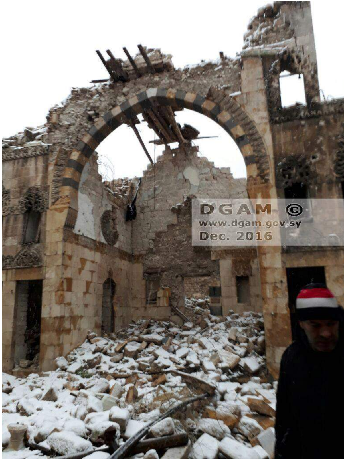
Severe damage to the Beit Ajaqbash and significant debris within the courtyard (DGAM; December 22, 2016)
