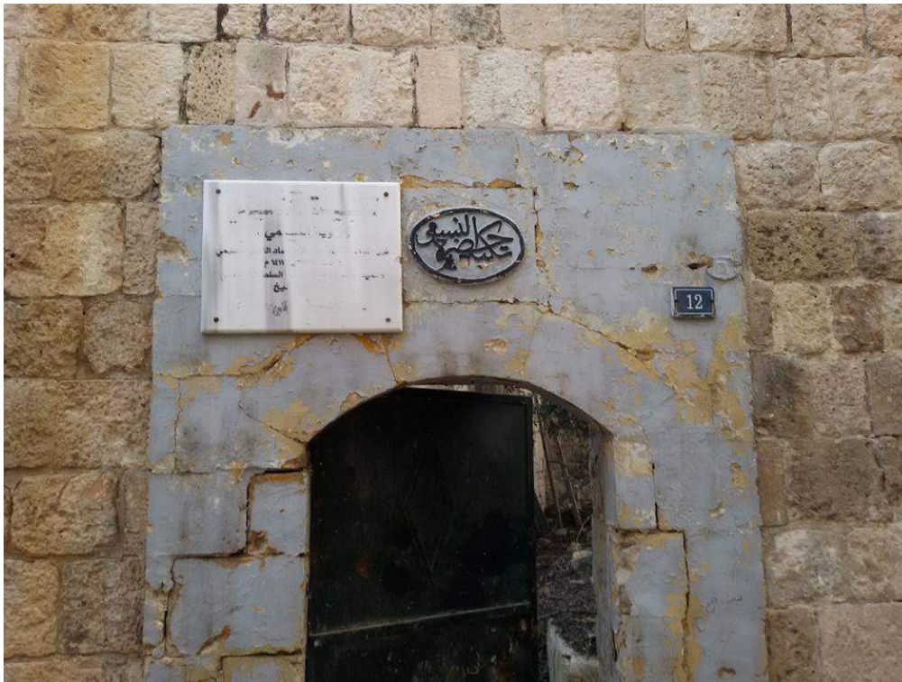
Damage to the placarde and door of Takkiya Nasimi (Private Facebook Account; December 19, 2016)
