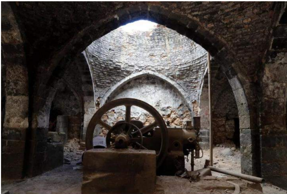
Extensive damage seen at Harasta Olive Oil Mill (Bisan Ilan Kurumu; November 22; 2016)
