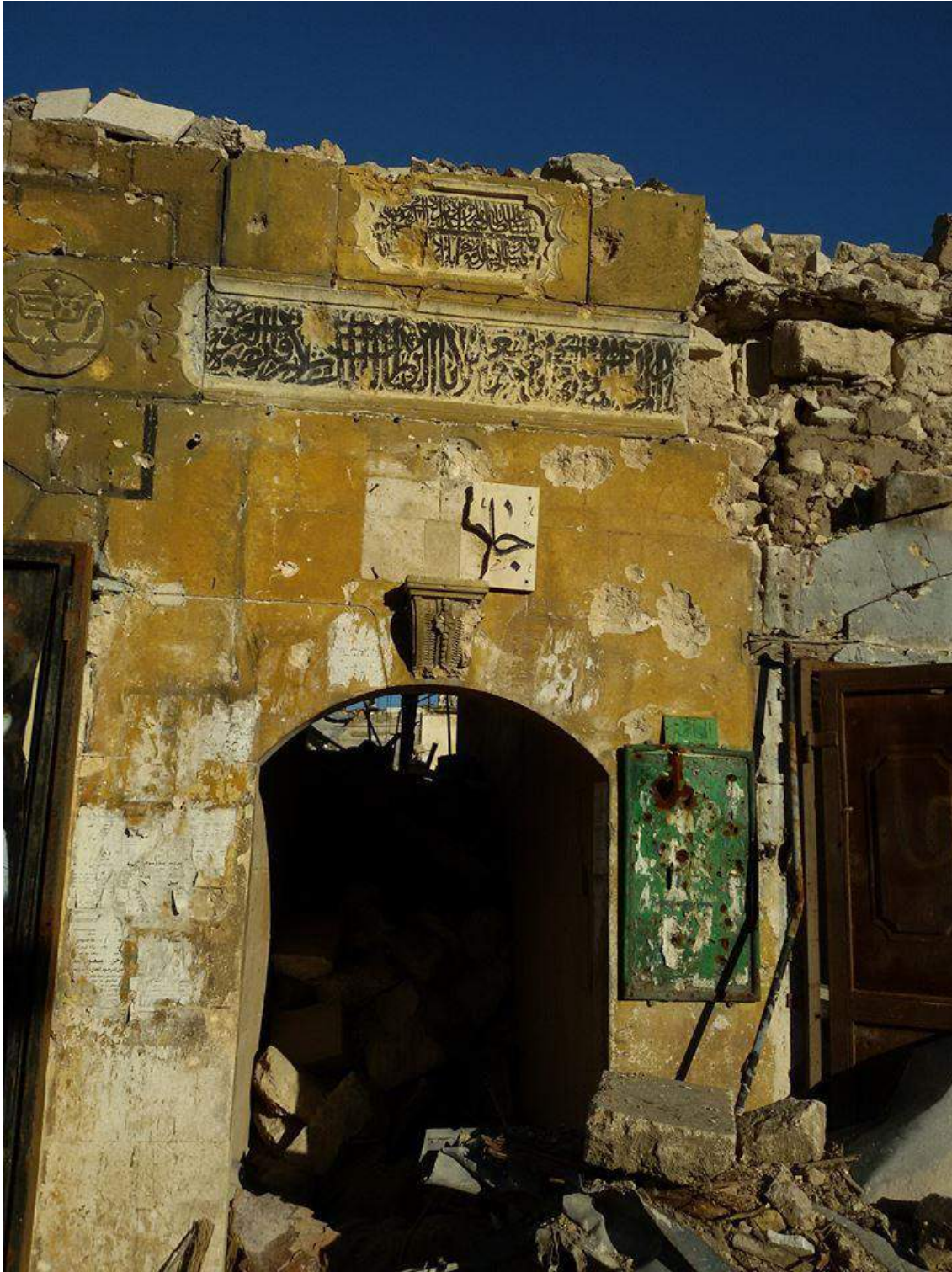
Extensive damage to Sharaf Mosque (Private Facebook Account; December 15, 2016)
