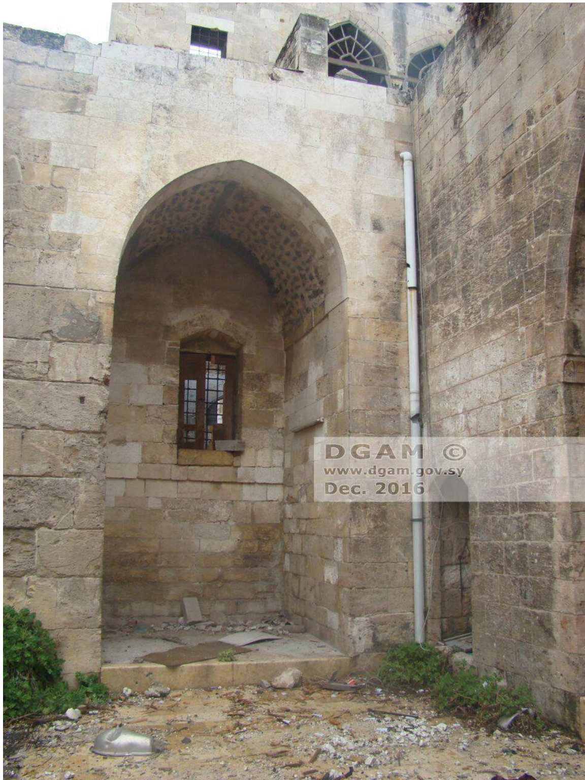
Damage to Bimaristan Nur al-Din (DGAM; December 31, 2016)
