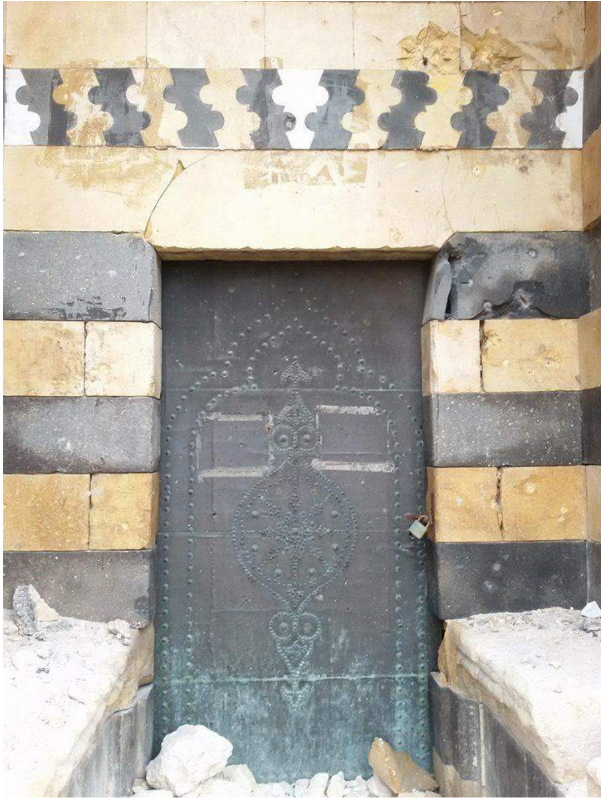
Light damage to Hammam Yalbugha al-Nasiri (Private Facebook Account; December 26, 2016)
