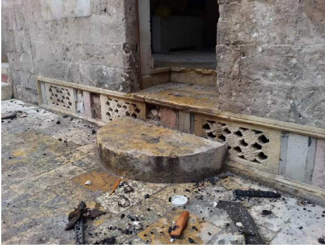
Minor damage, including presence of rubble, at al-Shibani Church and School (Private Facebook Account; December 24, 2016)
