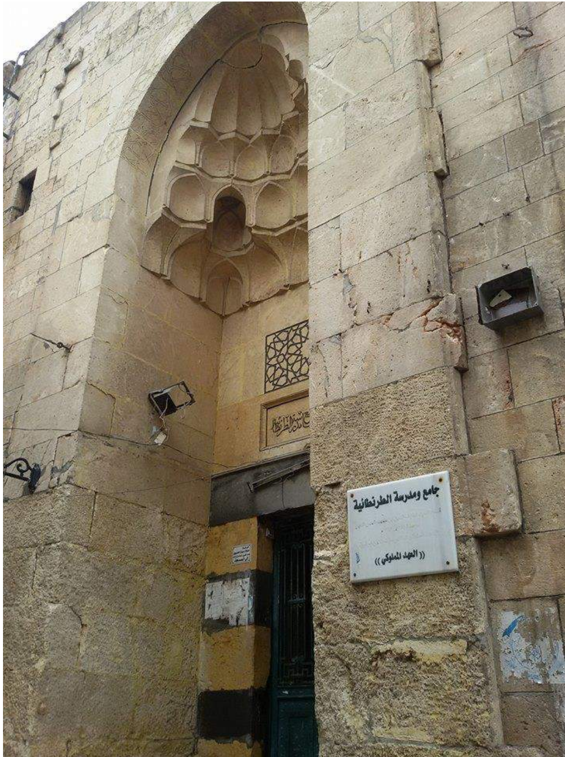
Light damage to the west portal of Mosque and Madrasa Turuntaiya (Private Facebook Account; December 22, 2016)
