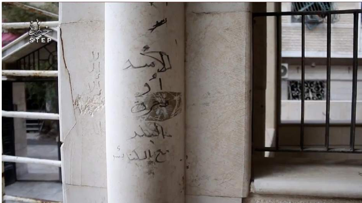
Video still showing vandalism at the Church of Mary (Step News Agency; December 26, 2016)
