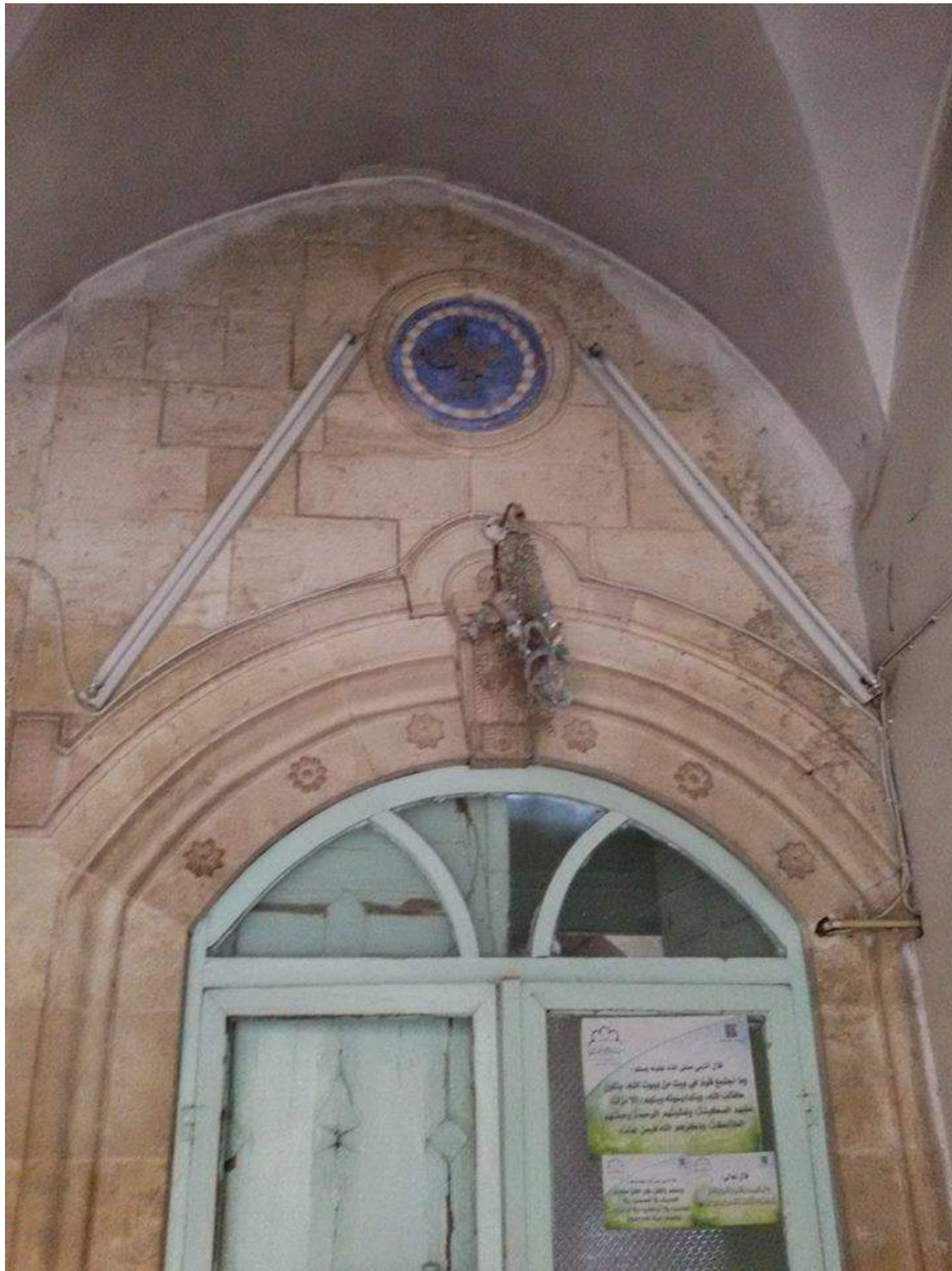
Minimal damage to the exterior of al-Mustadamiya Mosque (Private Facebook Account; December 20, 2016)
