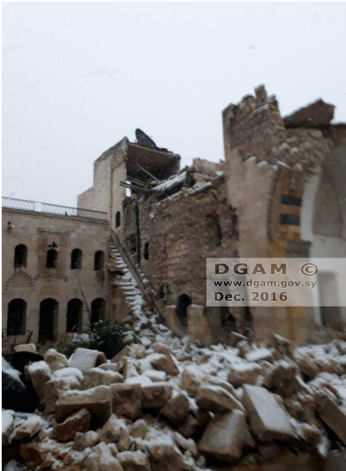
Severe damage to Beit Ghazaleh (DGAM; December 22, 2016)
