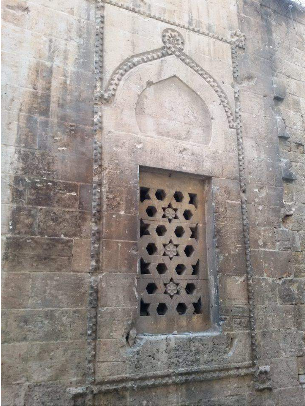
Light damage at Takkiya Nasimi (Private Facebook Account; December 19, 2016)
