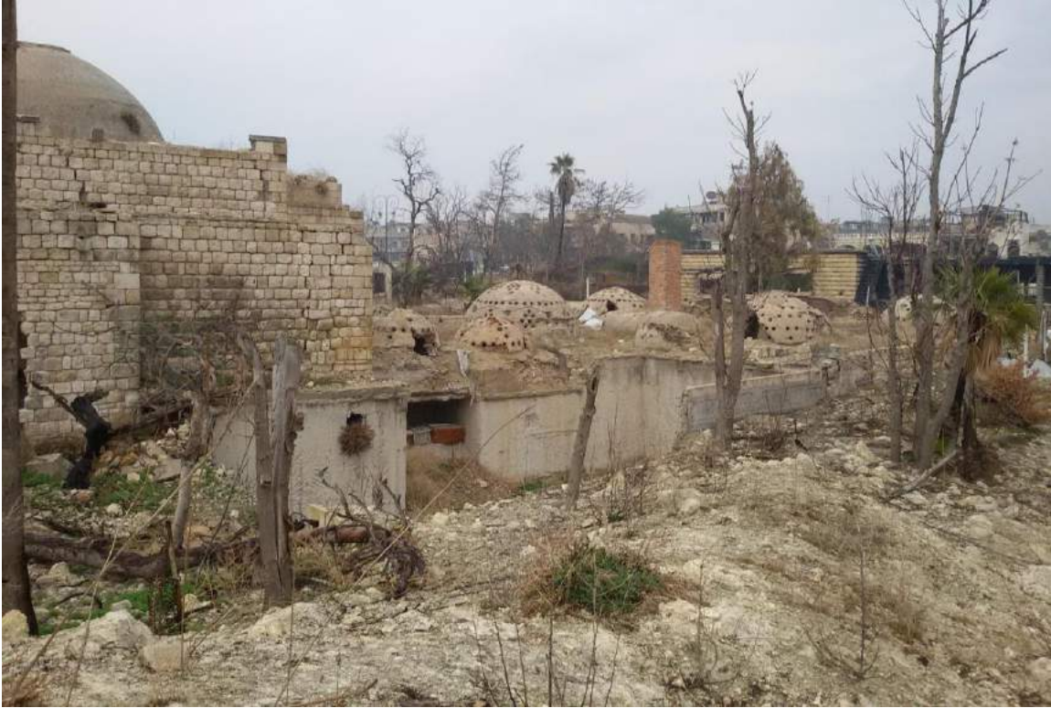
Damage to Hammam Yalbugha al-Nasiri (Private Facebook Account; December 26, 2016)
