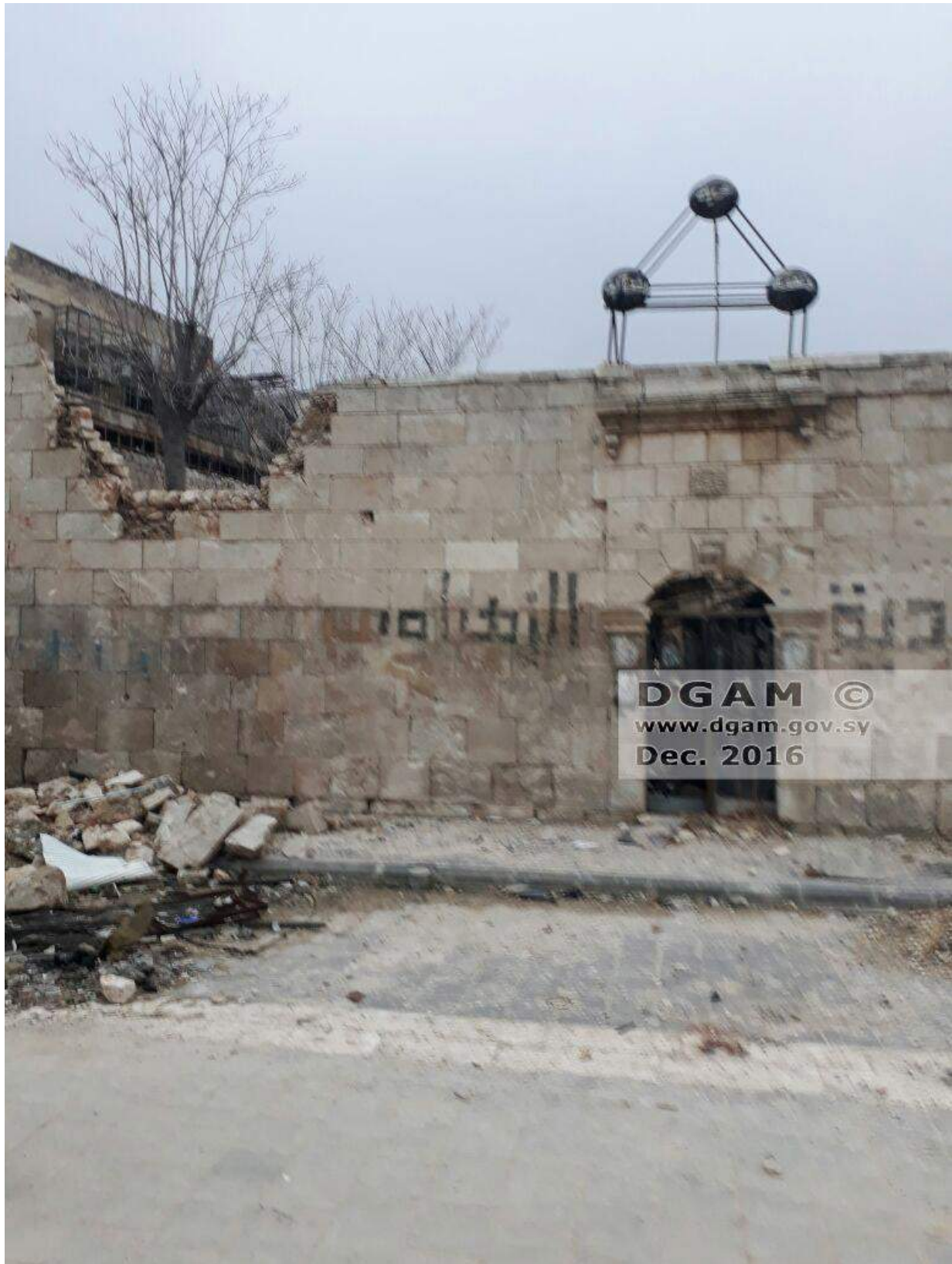
Damage to the exterior wall of al-Zahrawi School (DGAM; December 25, 2016)
