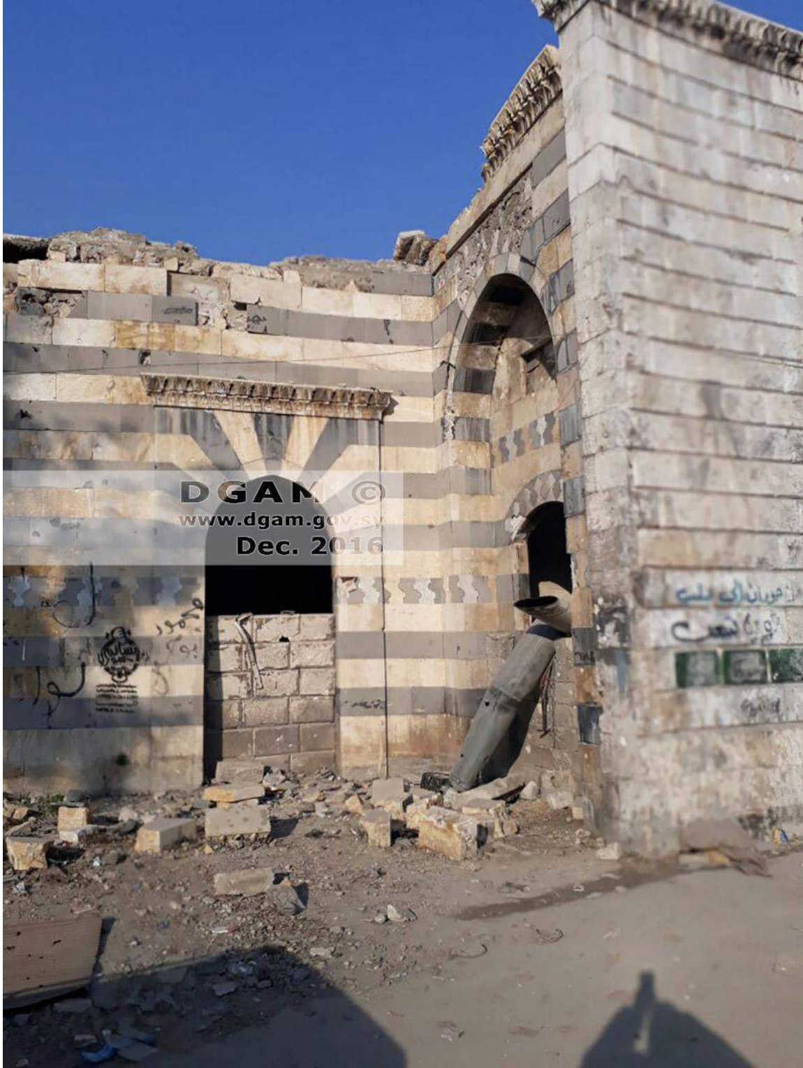
Structural damage to Jabri School (DGAM; December 20, 2016)
