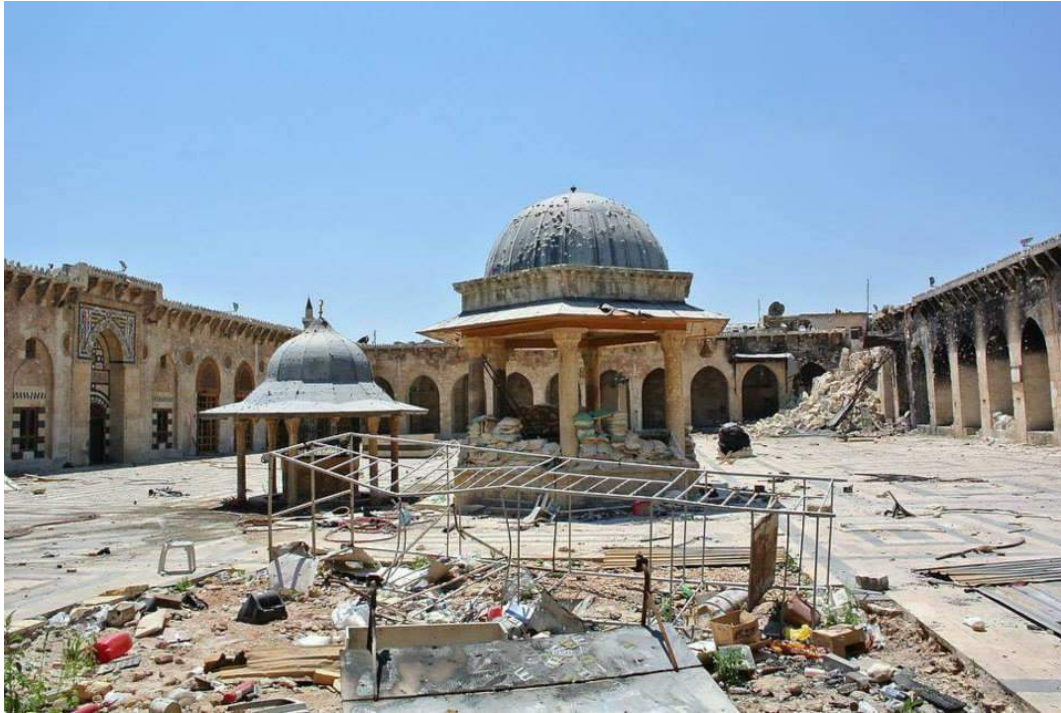
Damage seen inside the al-Umayyad Mosque (Aleppo Archaeology; December 18, 2016)
