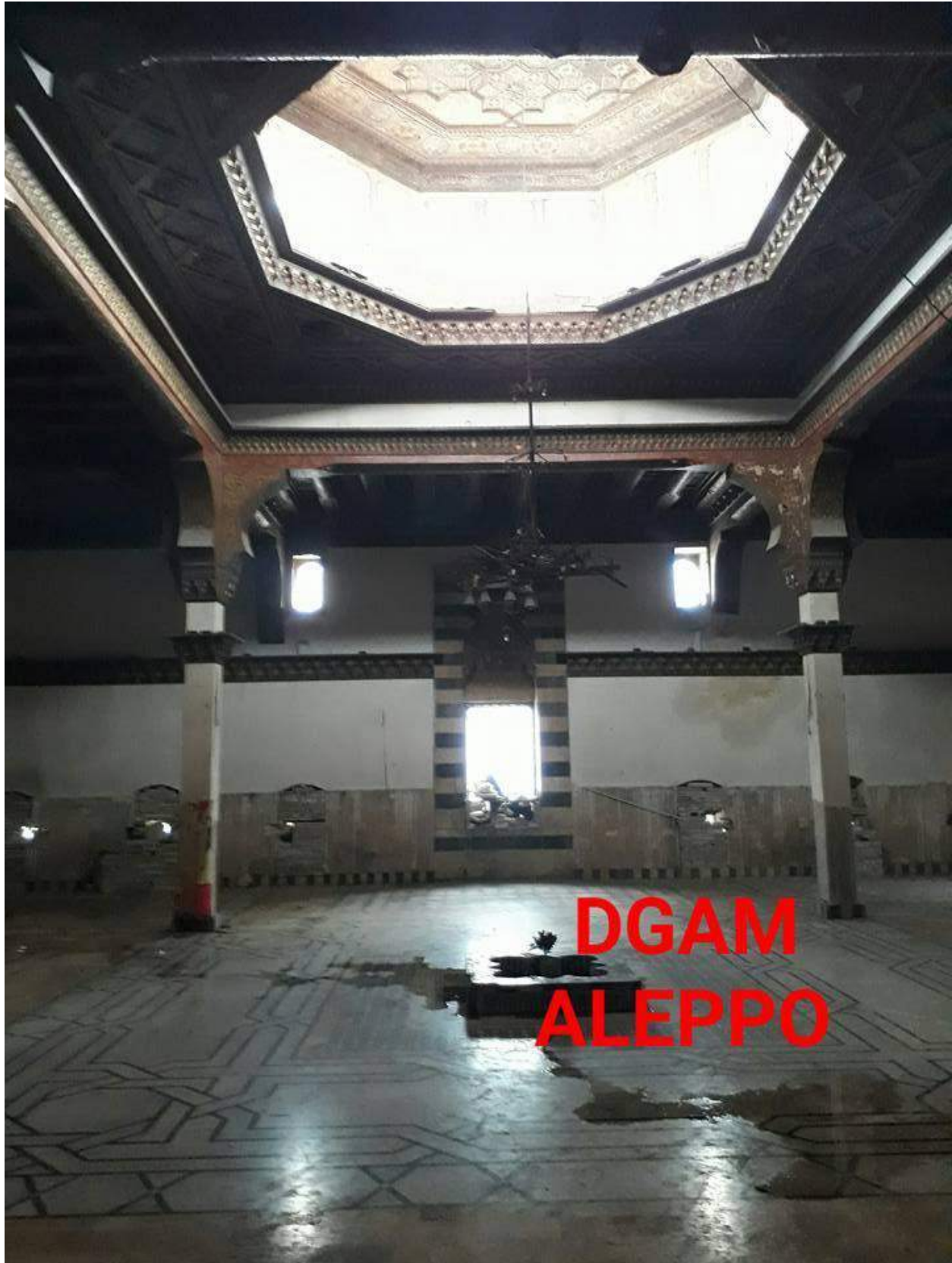
Damage to the interior of the Mamluk Throne Hall (DGAM; December 28, 2016)
