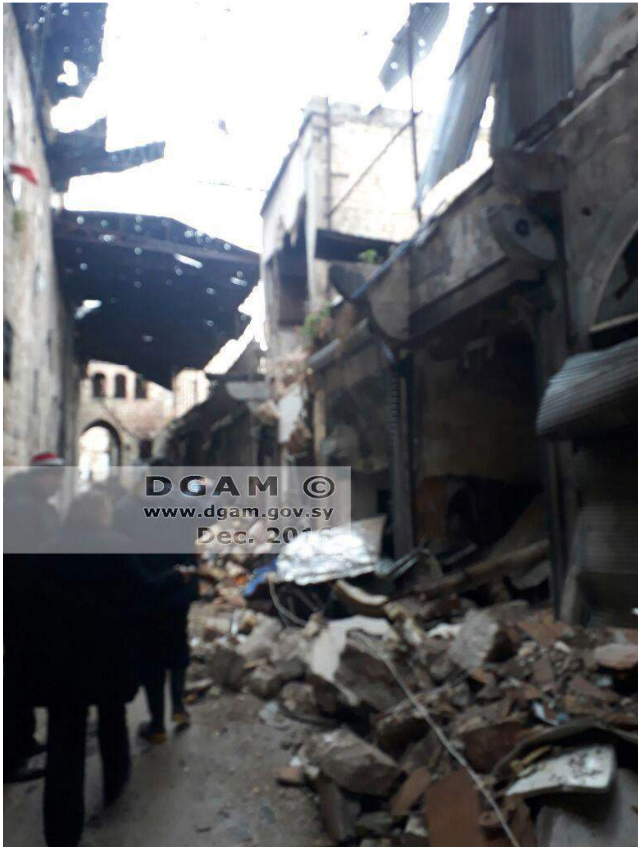
Collapsed roof and debris within the shops of the Suq al-Suweiqah (DGAM; December 16, 2016)
