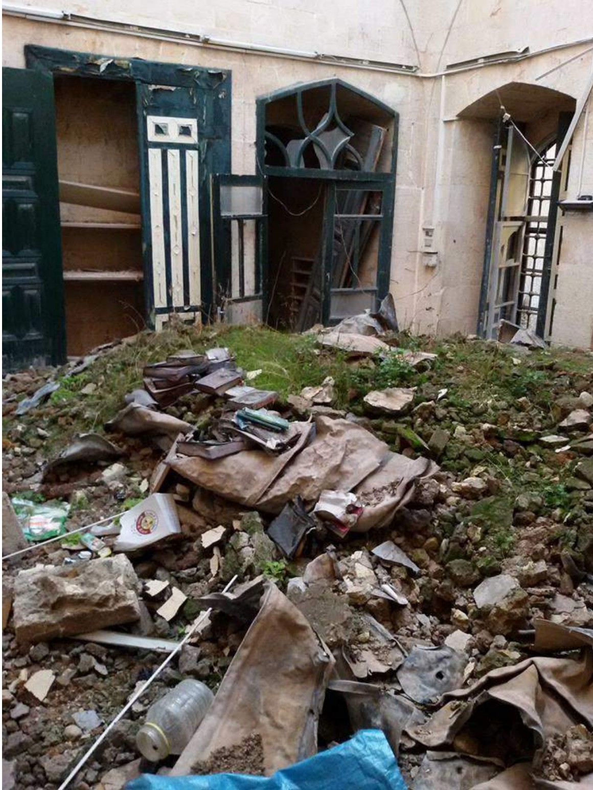
Damage and the presence of trash inside al-Uthmaniya Mosque (Private Facebook Account; December 15, 2016)
