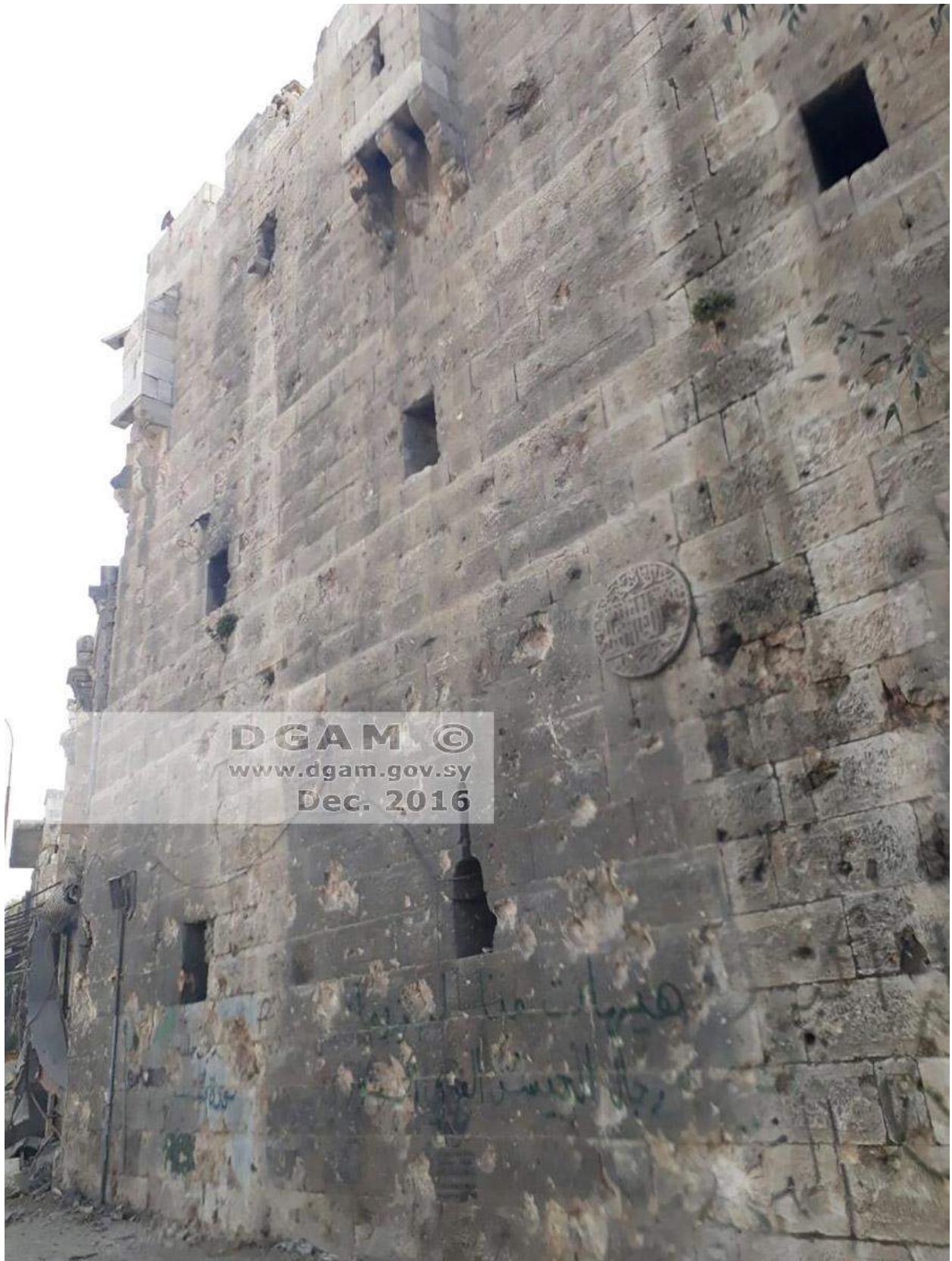
Impact damage and graffiti on the exterior of Bab al-Hadid (DGAM; December 20, 2016)
