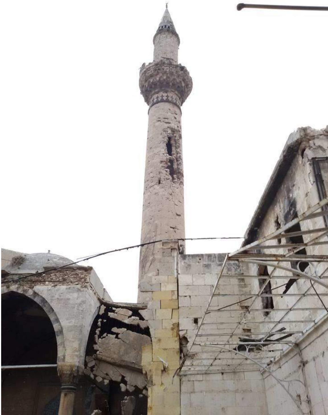
Structural damage to Adliyah Mosque (Private Facebook Account; December 17, 2016)
