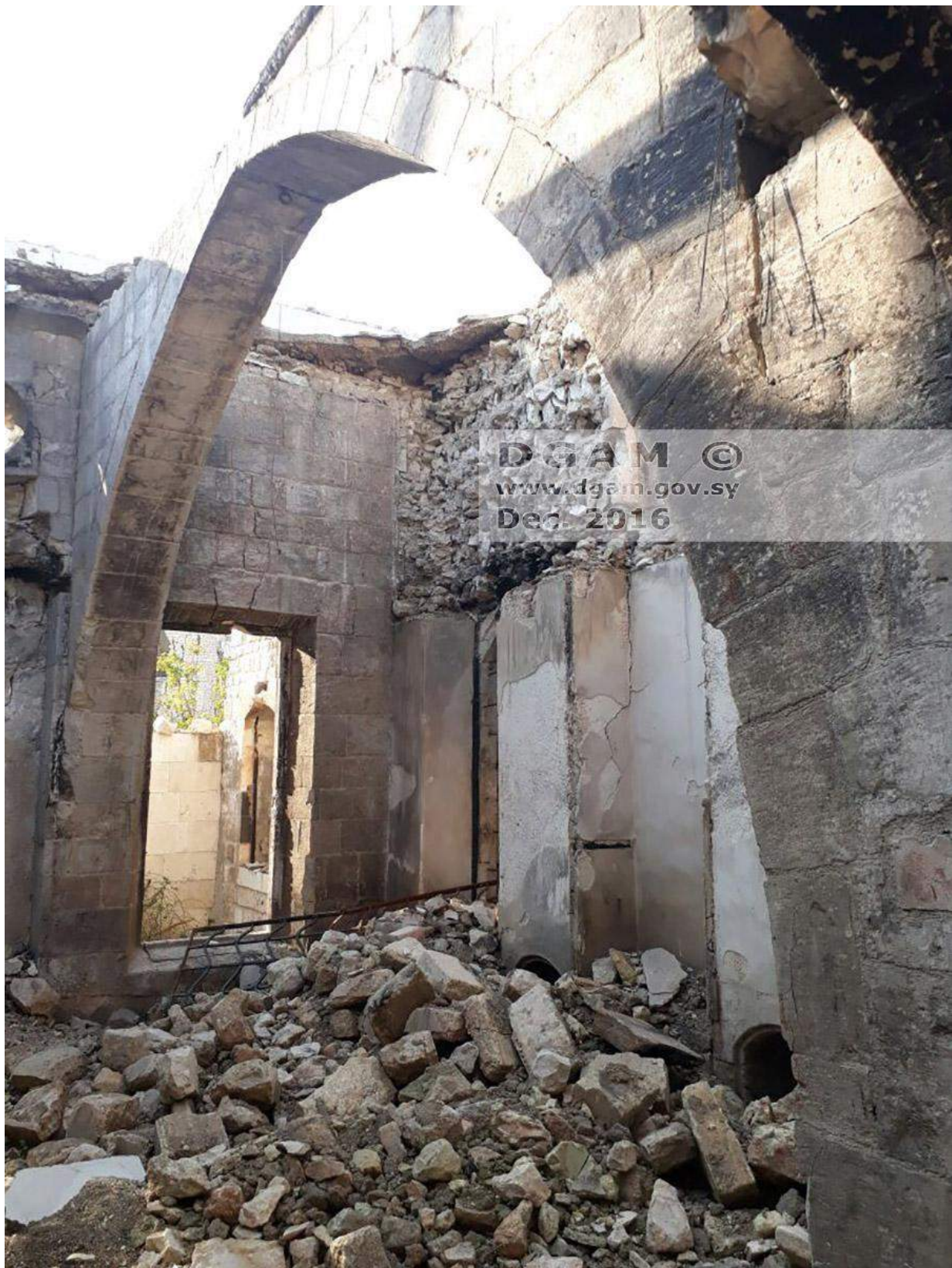
Interior damage to the Police Station in Bab al-Hadid (DGAM; December 20, 2016)
