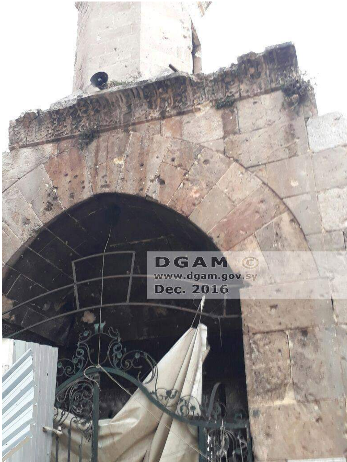
Moderate damage to al-Sultaniyah Mosque and Madrasa (DGAM; December 28, 2016)
