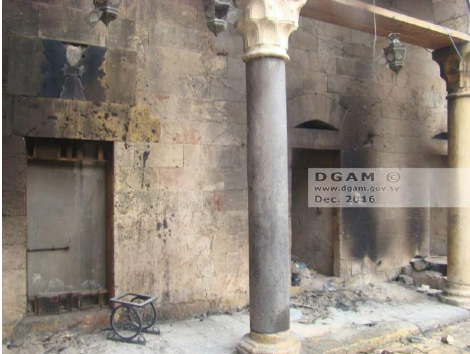
Damage, including possible fire damage, at Bimaristan Arghun al-Kamili (DGAM; December 31, 2016)
