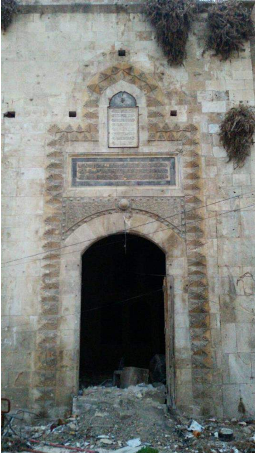
Damage to Madrasa Halawiya (Private Facebook Account; December 19, 2016)
