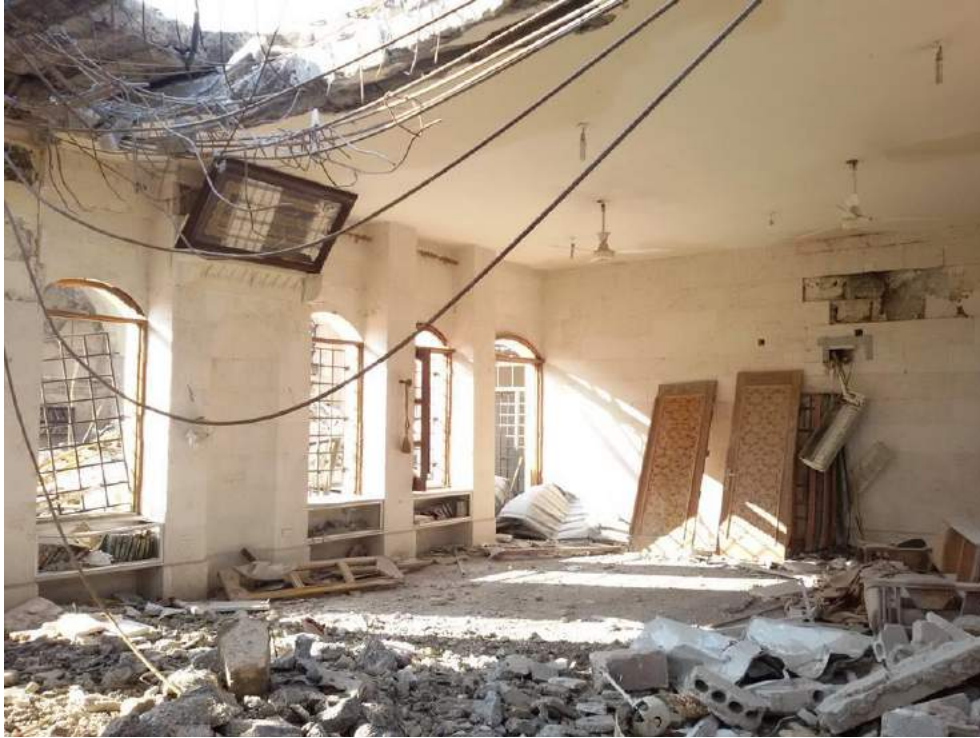
Extensive destruction inside al-Maidani Mosque (Private Facebook Account; December 19, 2017)
