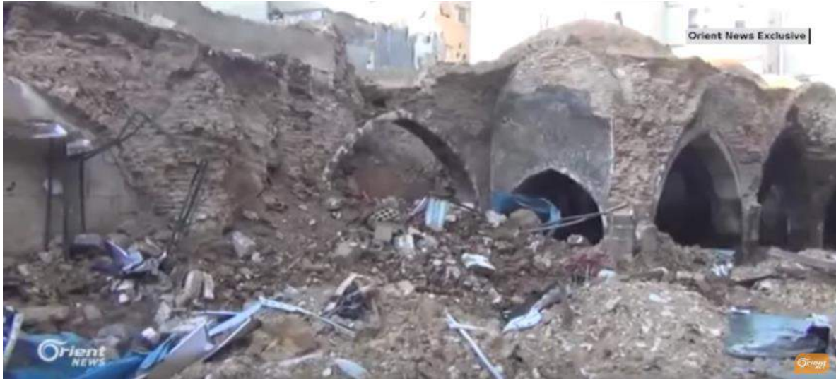
Video still shows damage to Harasta Olive Oil Mill (Orient News; December 24, 2016)
