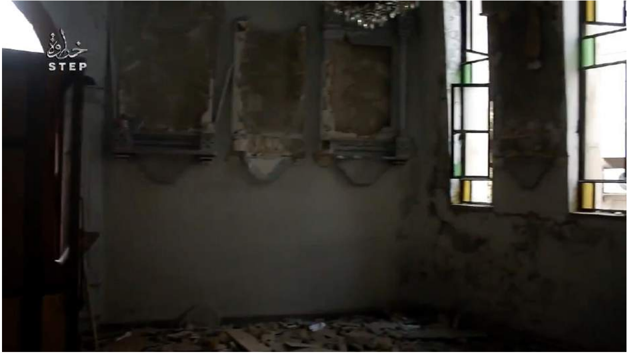
Video still of damage to the Church of Mary (Step News Agency; December 26, 2016)
