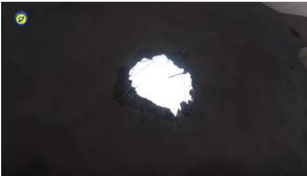
A video still shows a whole in the dome of the unnamed mosque in al-Jeenia (SCD; December 27, 2016)
