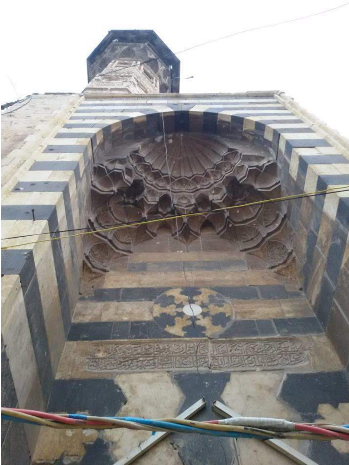
Saffahiya Mosque, makeshift electrical wiring is seen (Private Facebook Account; December 20, 2016)
