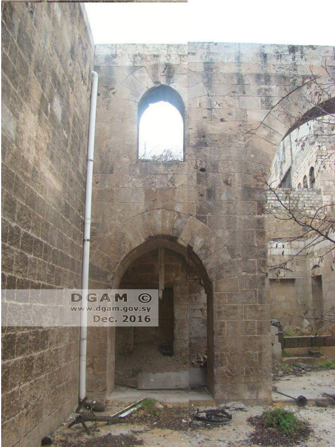
Damage and debris seen at Bimaristan Nur al-Din (DGAM; December 31, 2016)
