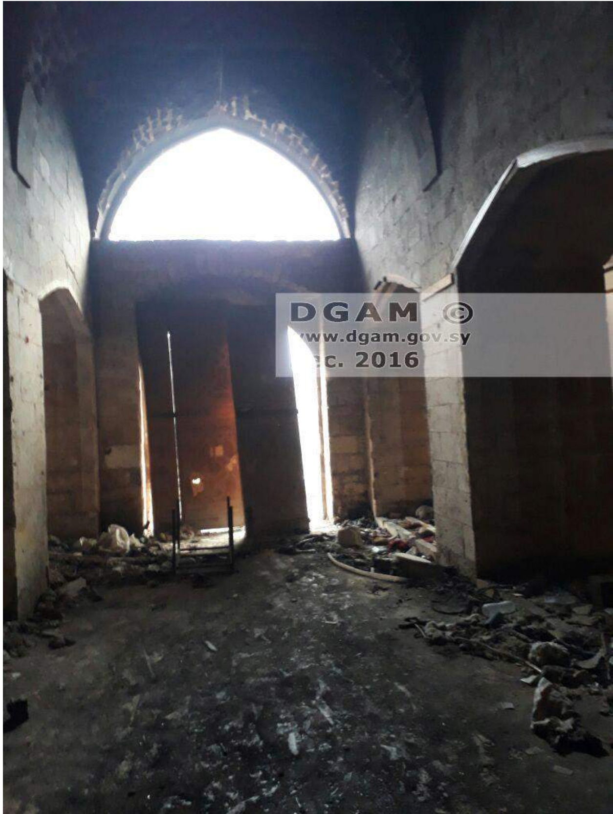
Damage to the interior of the Khan al-Shouneh (DGAM; December 28, 2016)
