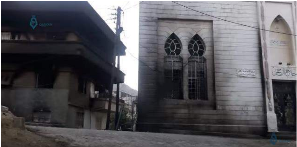
Video still shows what appears to be fire damage to al-Rahman Mosque (Qasioun News Agency; December 22, 2016)
