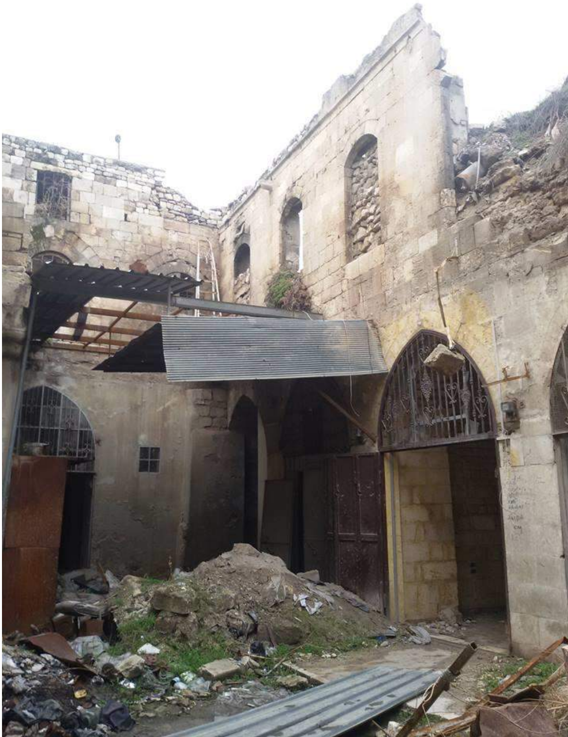
Damage to the metal roofs and upper walls in Khan al-Qassabiya (Private Facebook Account; December 24, 2016)
