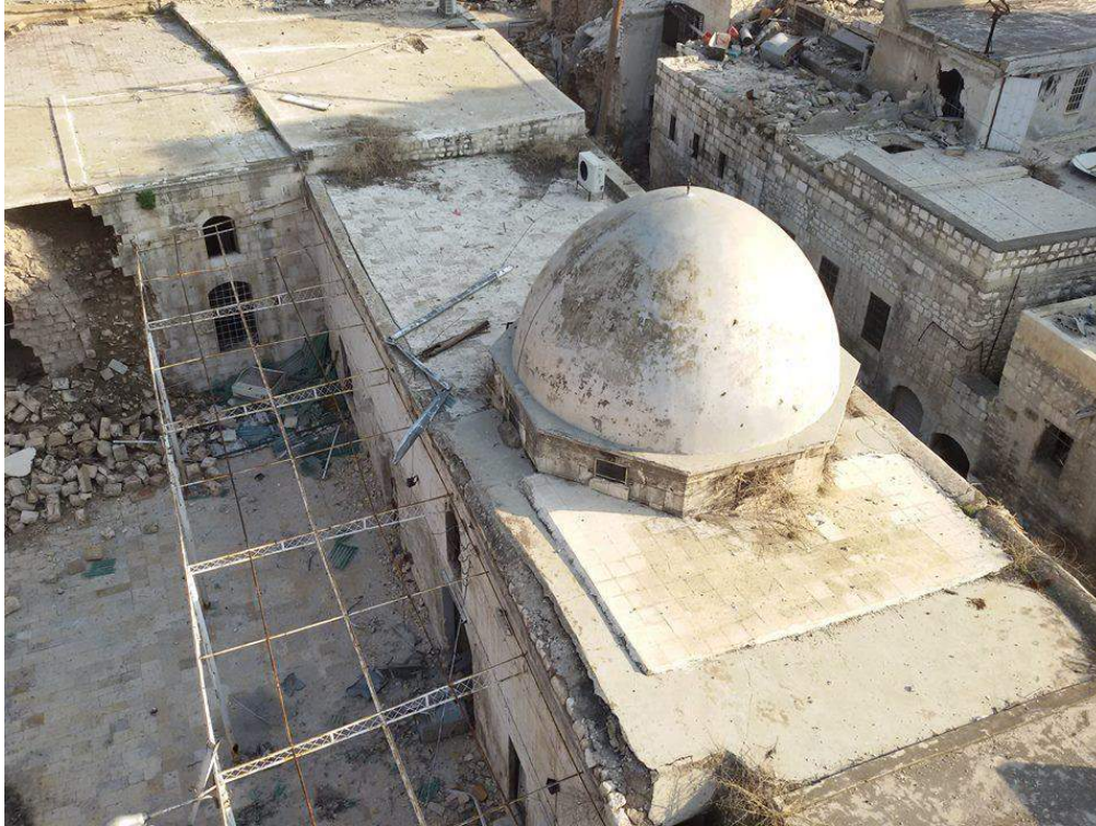
Light damage seen to the dome of al-Zaki Mosque and partial view of collapsed facade of outer wall (Private Facebook Account; December 19, 2016)
