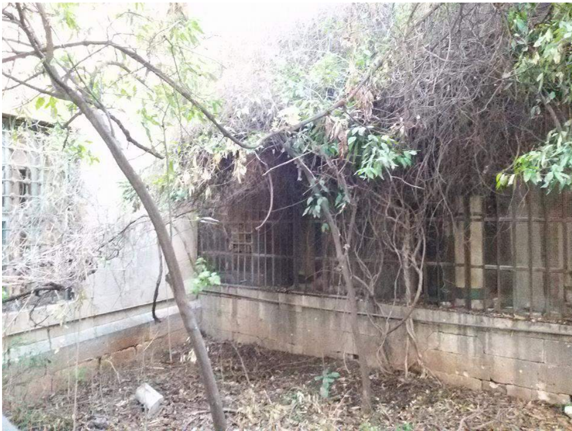
Overgrowth inside the Uthmaniya Mosque (Private Facebook Account; December 15, 2016)
