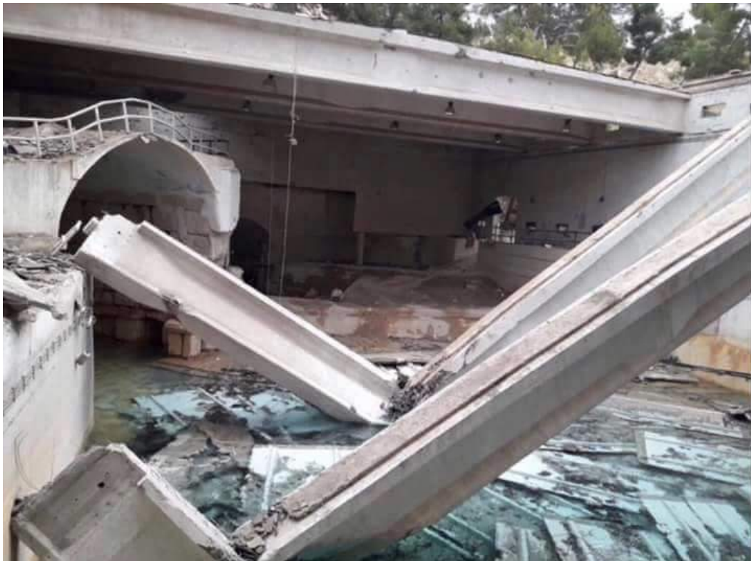
Damage to Ain al-Fijah Spring (Discover Syria; December 27, 2016)
