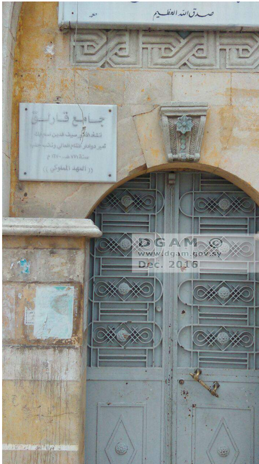
Light damage to Qarleq Mosque (DGAM; December 25, 2016)
