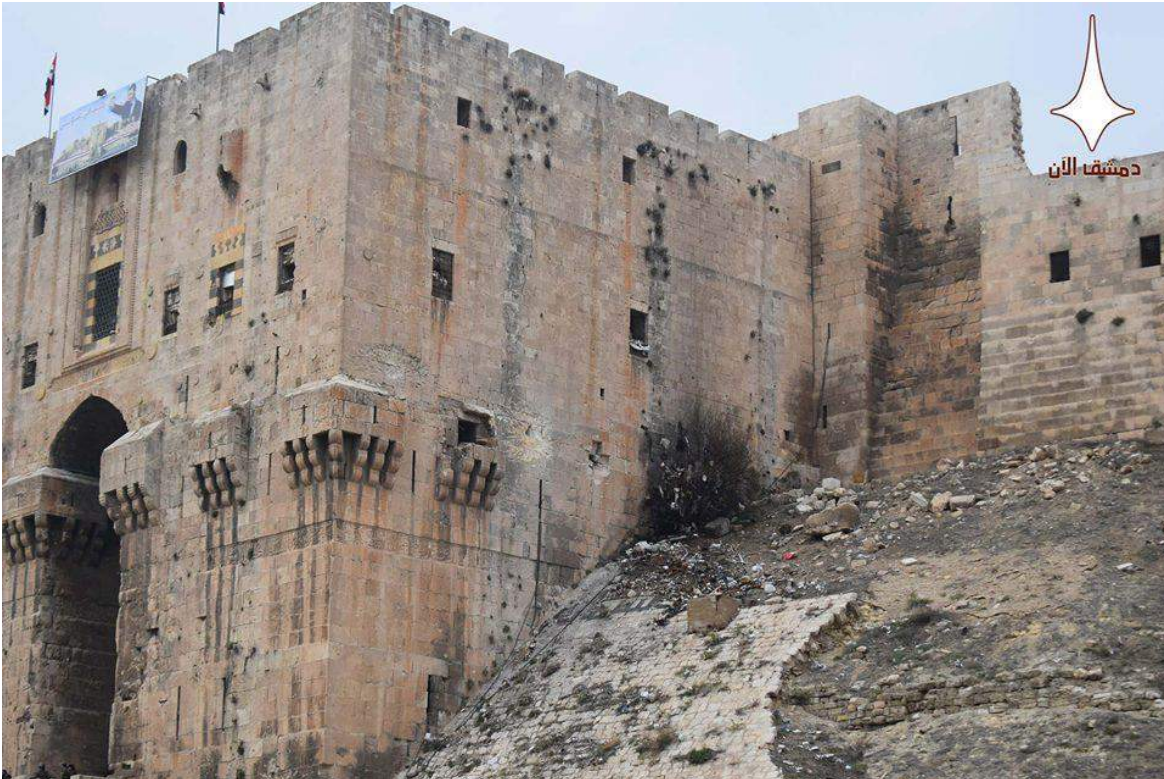
Damage to the Gate Tower (Dimashq al-Aan; December 19, 2016)
