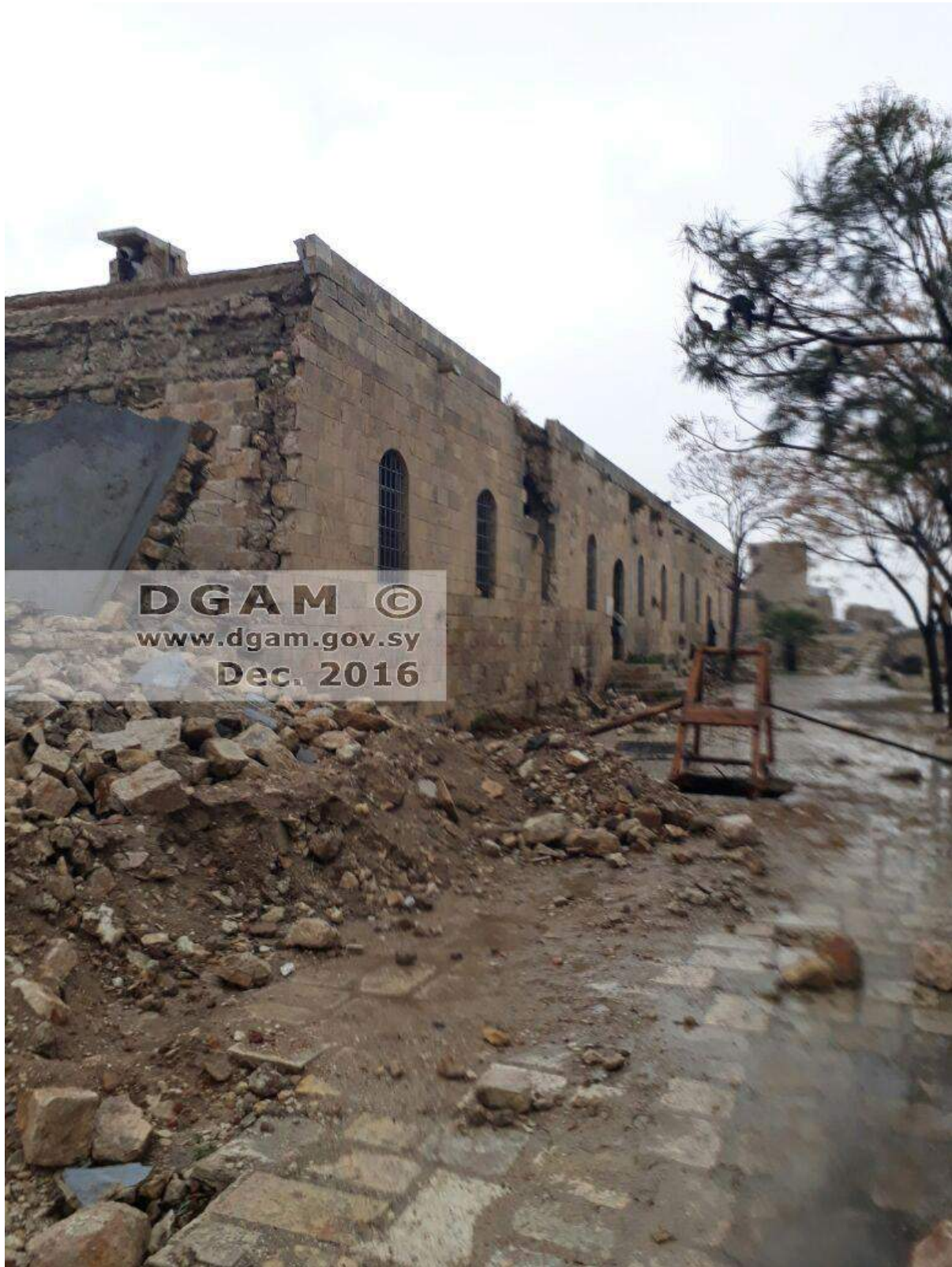
Collapse of the northwestern part of the museum of the citadel (DGAM; December 16, 2016)
