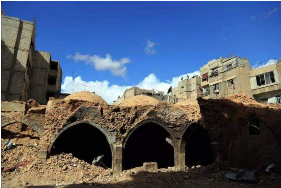
Extensive damage seen at Harasta Olive Oil Mill (Bisan Ilan Kurumu; November 22; 2016)
