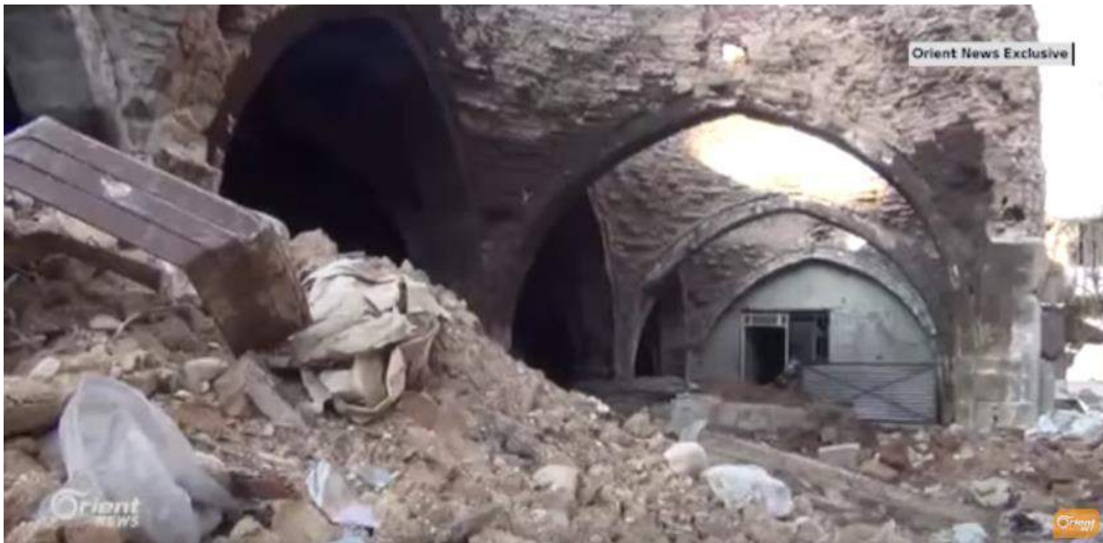
Video still shows damage to Harasta Olive Oil Mill (Orient News; December 24, 2016)
