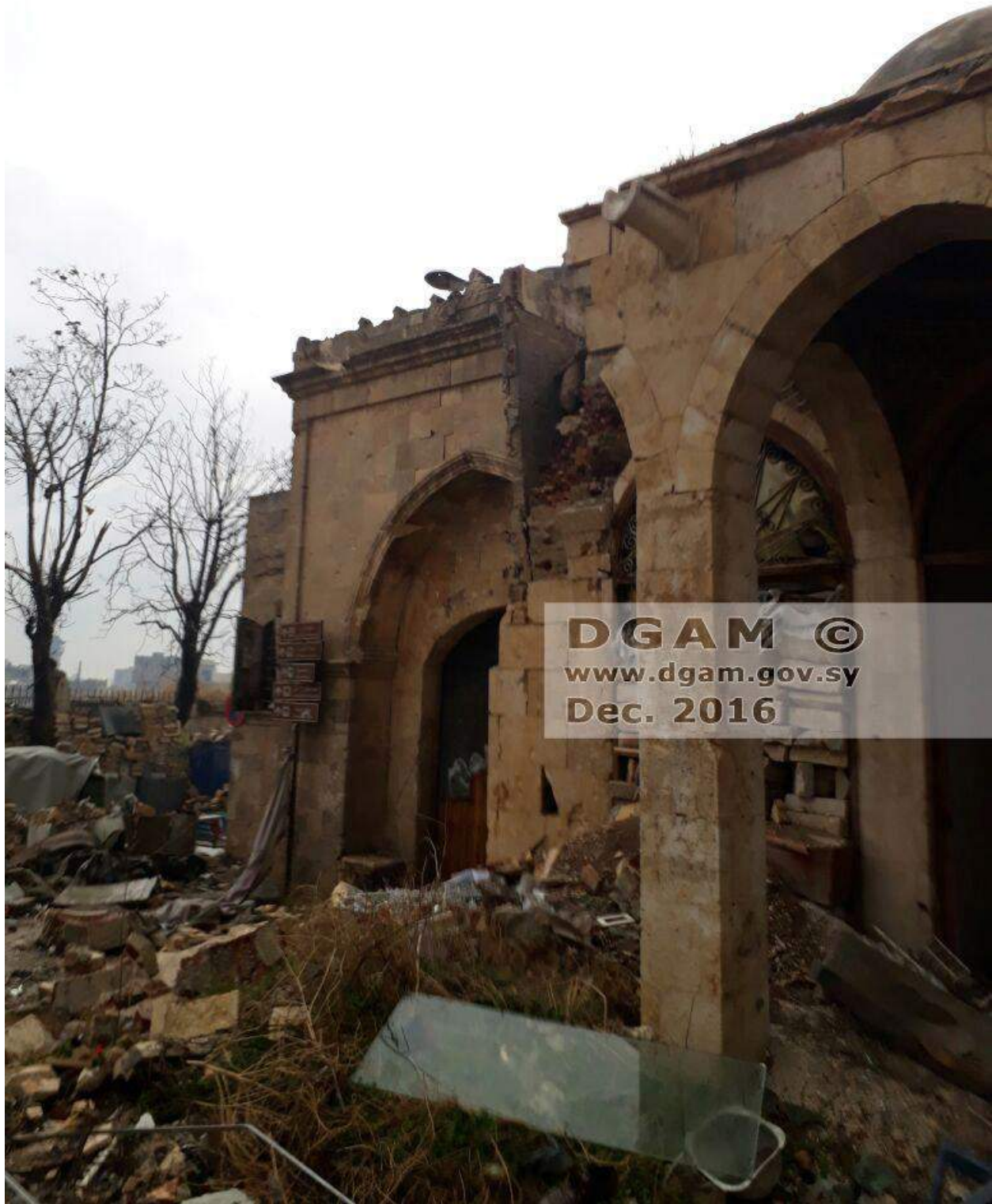
Damage to the exterior of the Khan al-Shouneh (DGAM; December 28, 2016)
