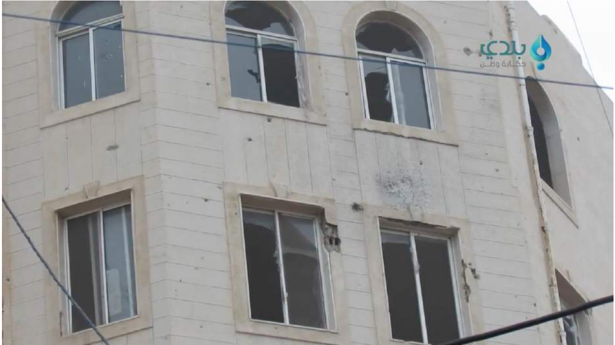
Video still of damage to al-Kabir Mosque (Baladi News; December 27, 2016)
