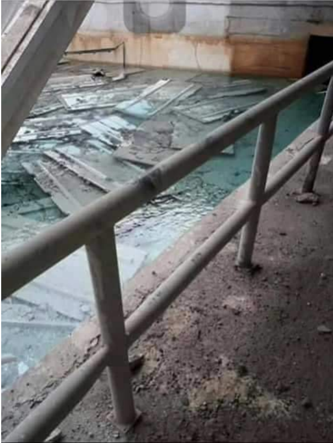
Damage to Ain al-Fijah Spring (Discover Syria; December 27, 2016)
