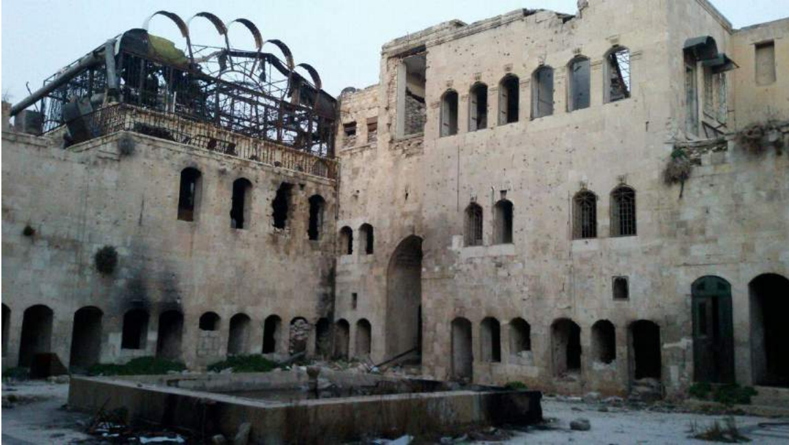
Damage to Madrasa Halawiya (Private Facebook Account; December 19, 2016)
