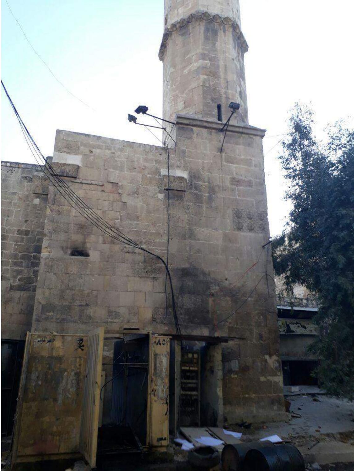
Light damage seen to Altunbugha Mosque (DGAM; December 20, 2016)
