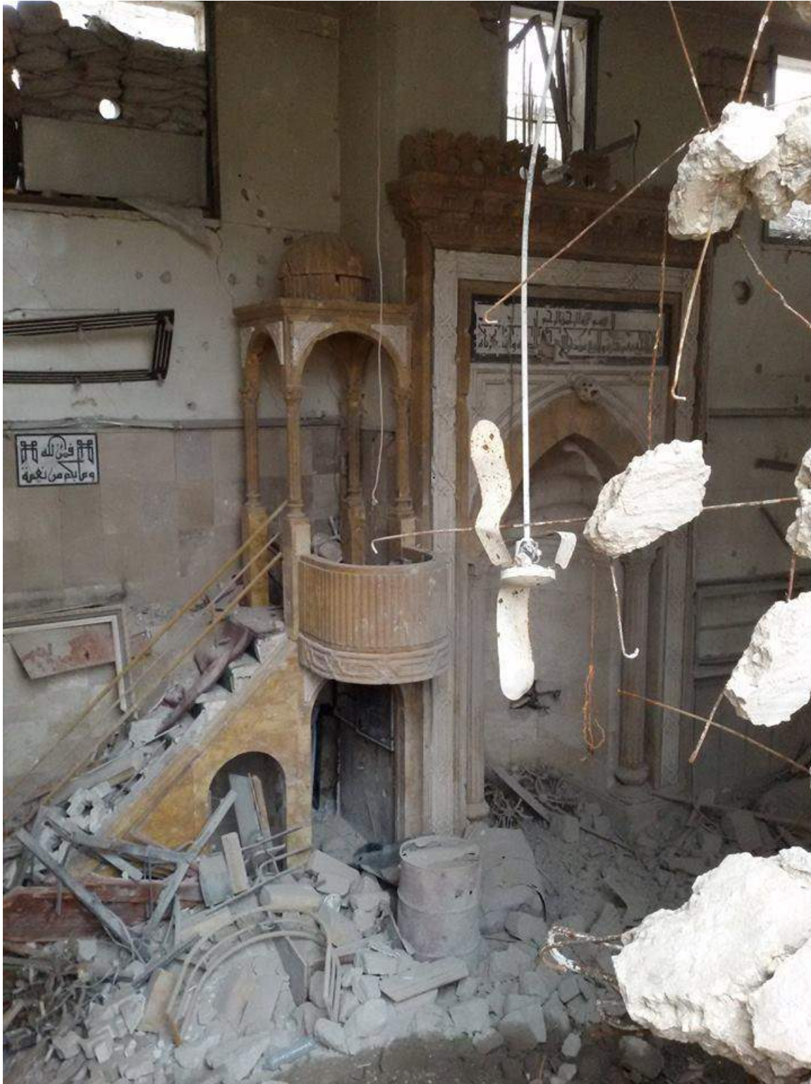
Damage to the interior of Mosque Suq Attarin (Private Facebook Account; December 17, 2016)
