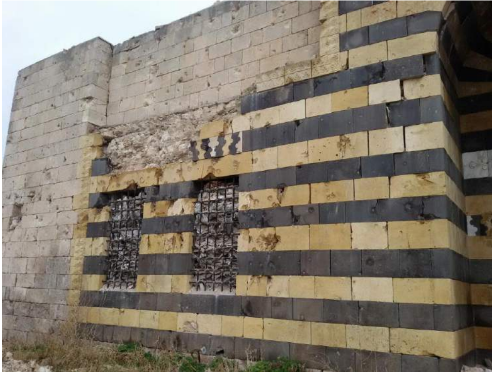
Medium damage to Hammam Yalbugha al-Nasiri (Private Facebook Account; December 26, 2016)
