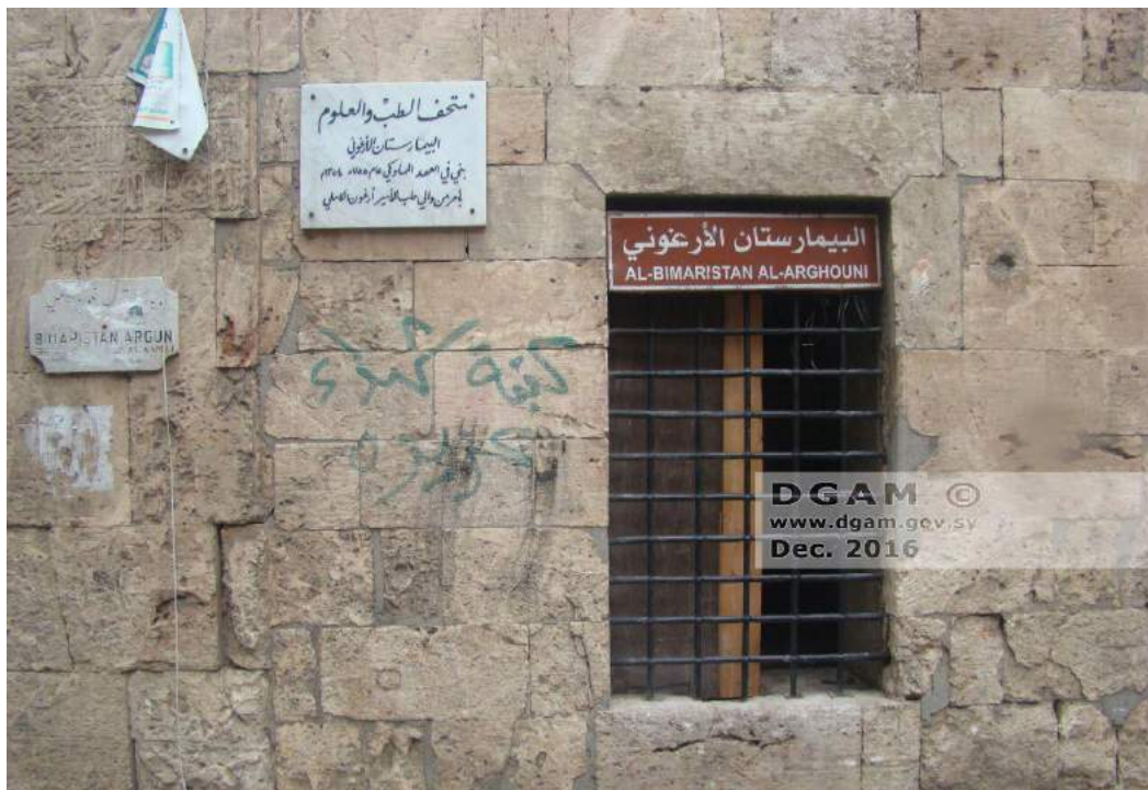
Moderate damage, including graffiti, to Bimaristan Arghun al-Kamili (DGAM; December 31, 2016)
