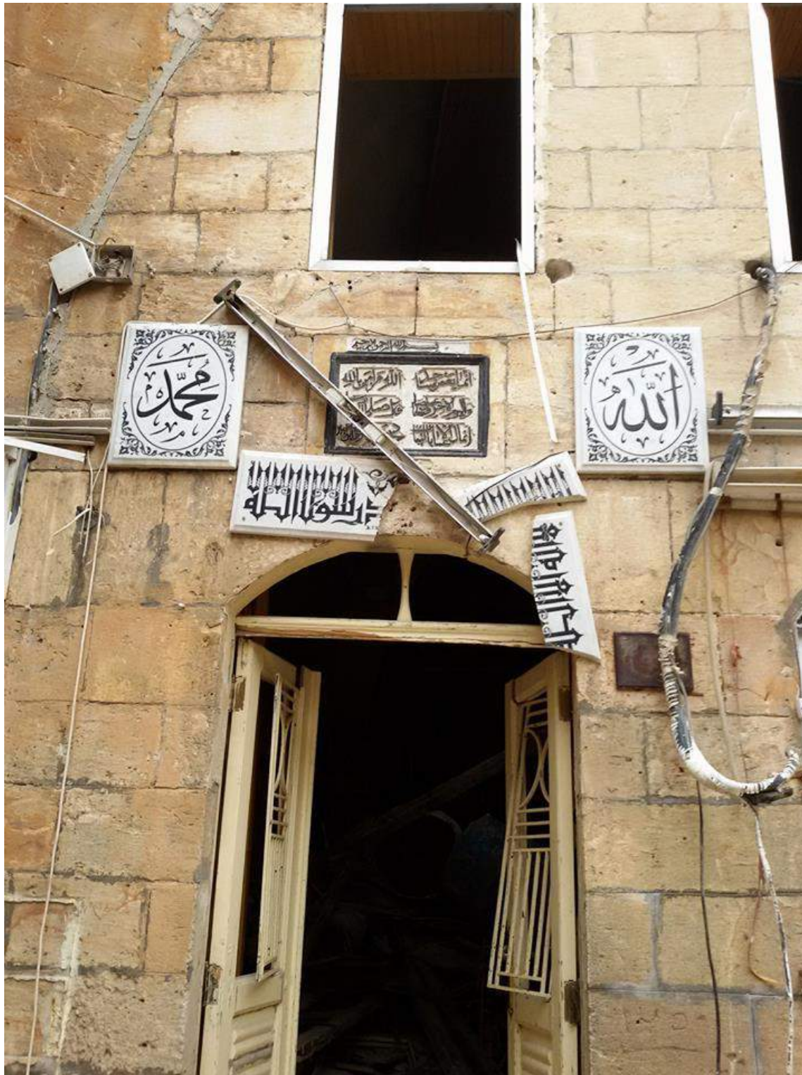
Damage to the exterior of Mosque and Madrasa Turuntaiya (Private Facebook Account; December 22, 2016)
