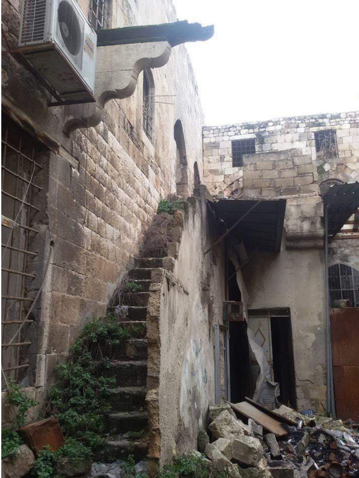
Damage to the stairwell and courtyard in Khan al-Qassabiya (Private Facebook Account; December 24, 2016)
