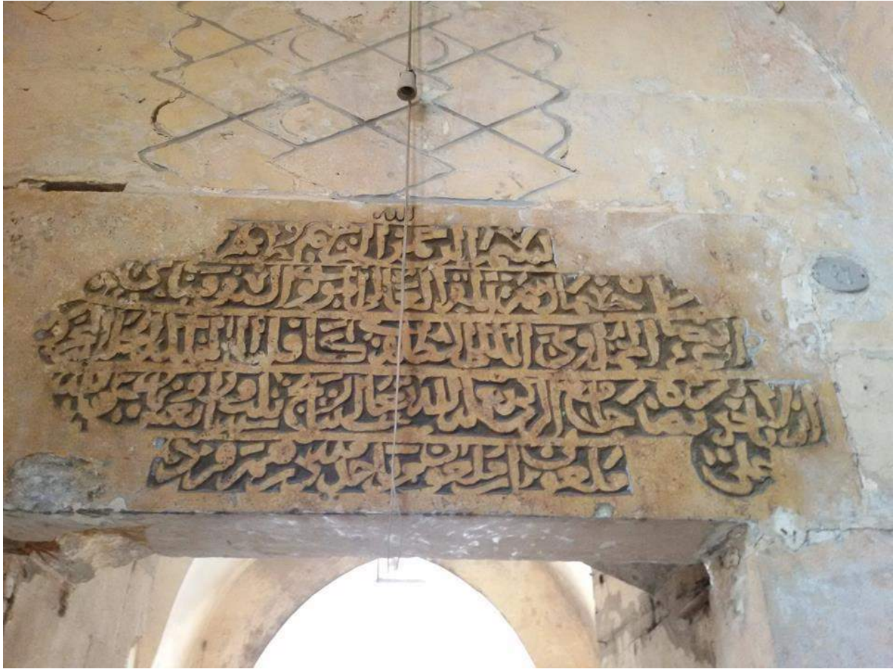
Light damage to inscription at al-Zaki Mosque (Private Facebook Account; December 19, 2016)
