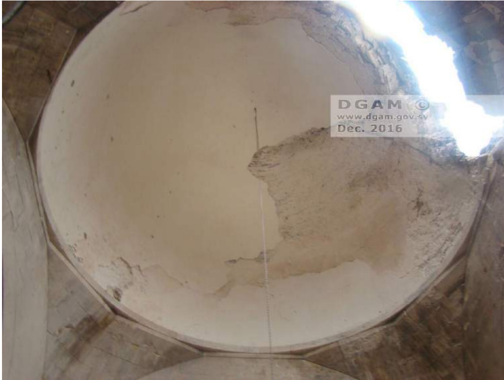
Structural damage to ceiling of Bimaristan Arghun al-Kamili (DGAM; December 31, 2016)
