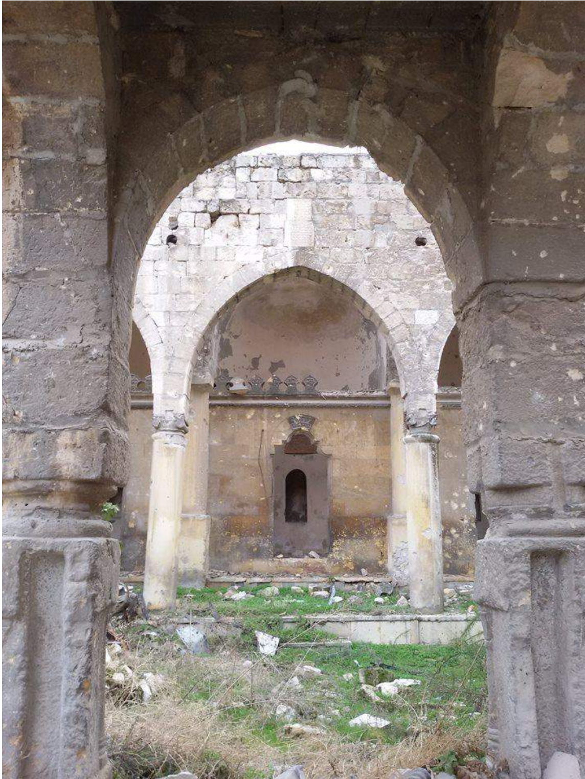
Damage, including broken religious pieces and overgrowth of vegetation, at Bandarā Synagogue (Private Facebook Account; December 17, 2016)
