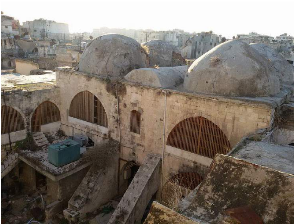
Damage to the courtyard and domes of Musabinat al-Zanabli (Private Facebook Account; December 15, 2016)
