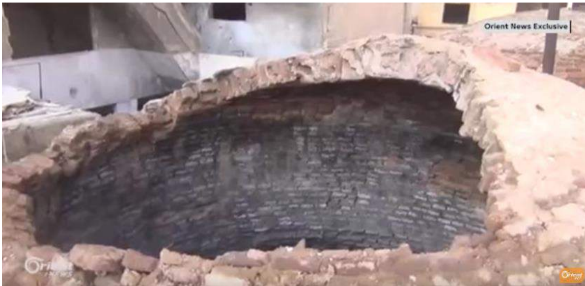
Video still shows damage to Harasta Olive Oil Mill (Orient News; December 24, 2016)
