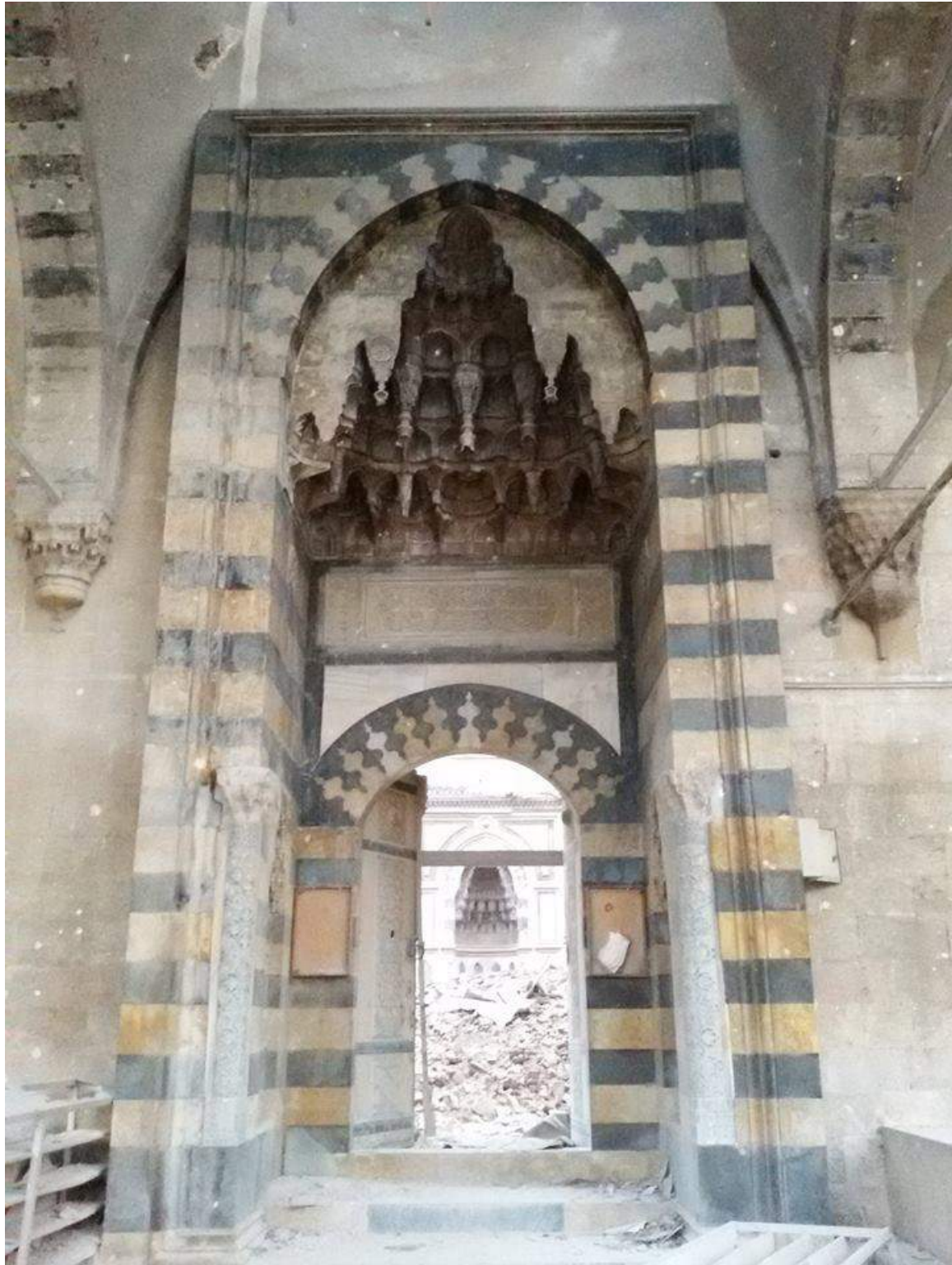
Damage seen at Adliyah Mosque (Private Facebook Account; December 17, 2016)
