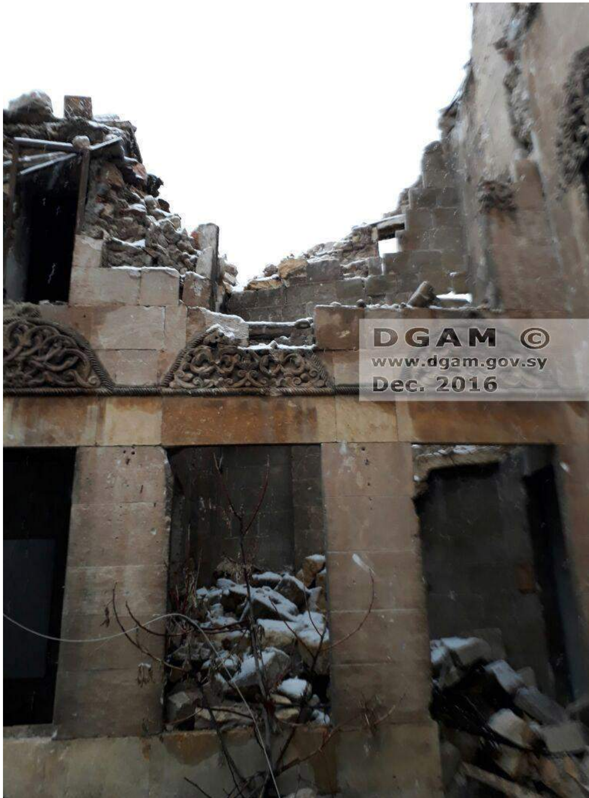
Damage to the Beit Ajaqbash (DGAM; December 22, 2016)
