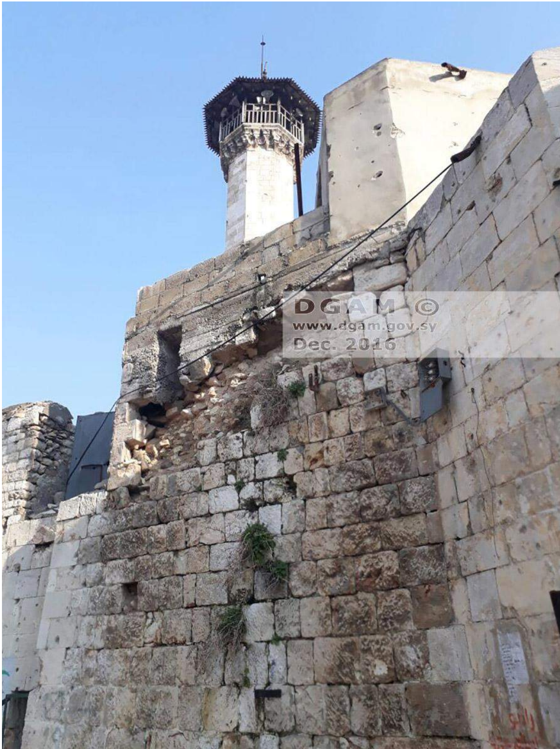
Damage to Banqusa Mosque (DGAM; December 20, 2016)
