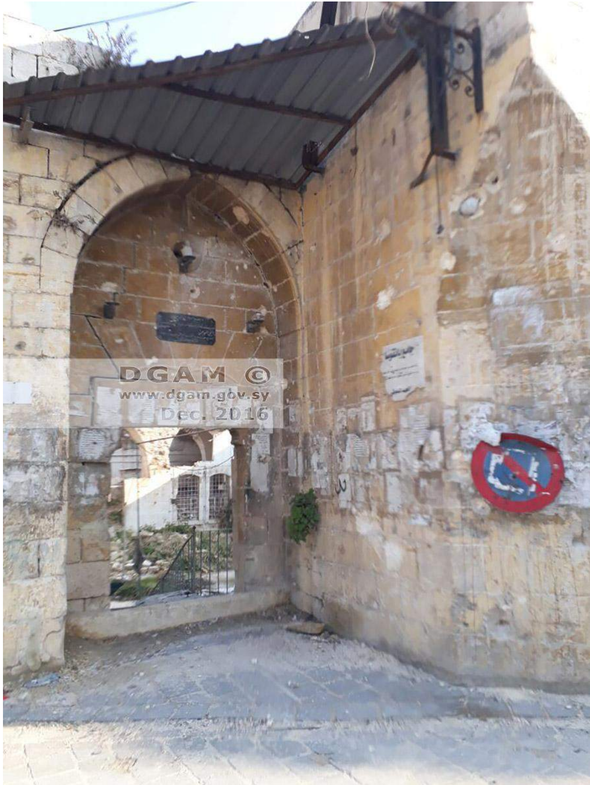
Damage to Banqusa Mosque (DGAM; December 20, 2016)
