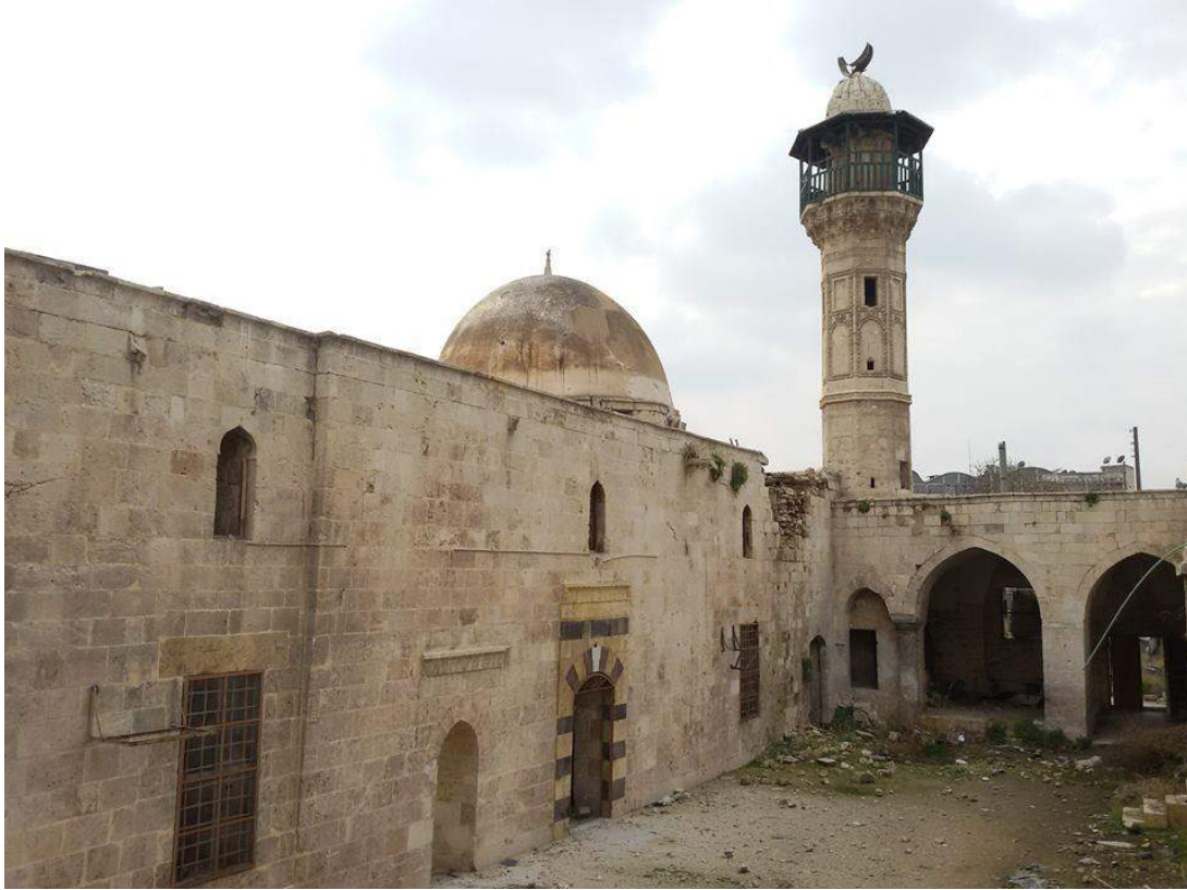
Light damage to al-Omari Mosque, including overgrowth (Private Facebook Account; December 17, 2016)
