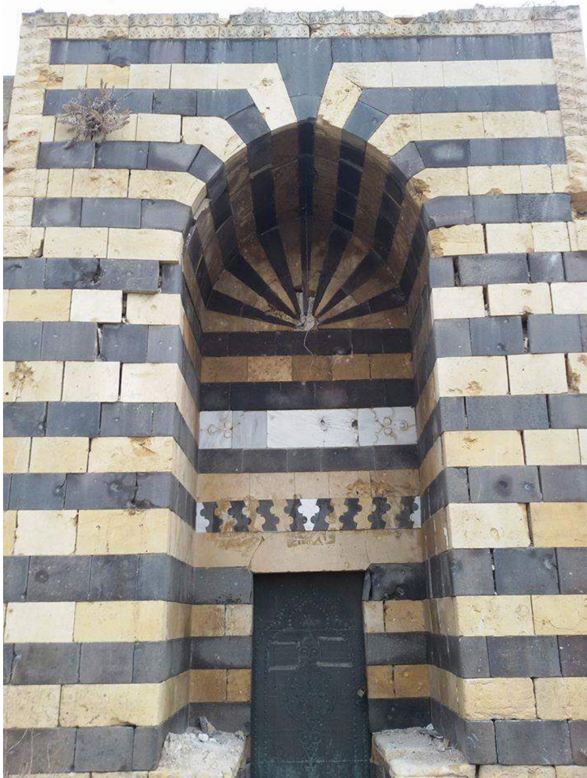
Light damage, including growth of vegetation, to Hammam Yalbugha al-Nasiri (Private Facebook Account; December 26, 2016)
