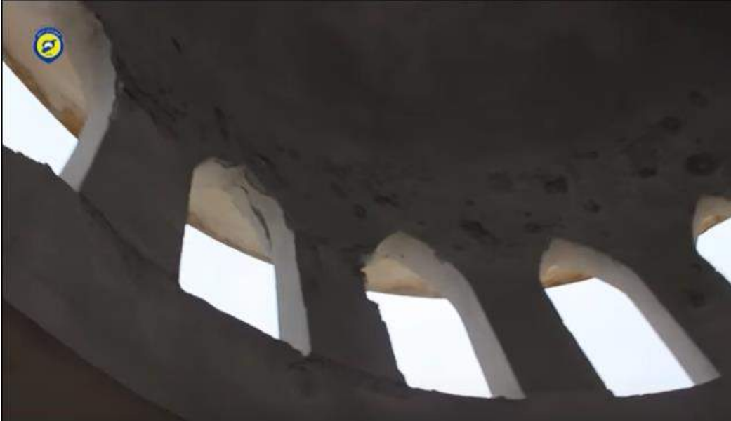
A video still shows damage to the dome of an unnamed mosque in al-Jeenia (SCD; December 27, 2016)
