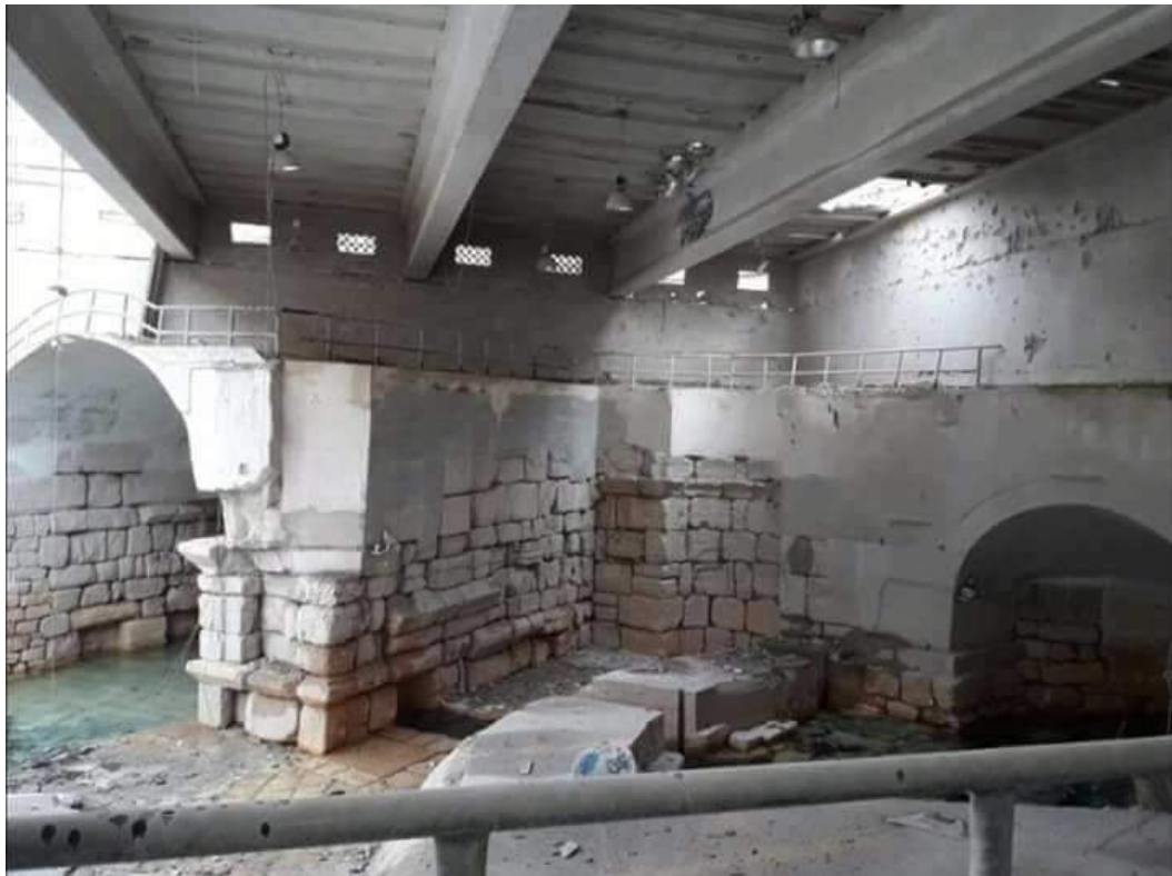
Damage to Ain al-Fijah Spring (Dimashq al-An; December 27, 2016)
