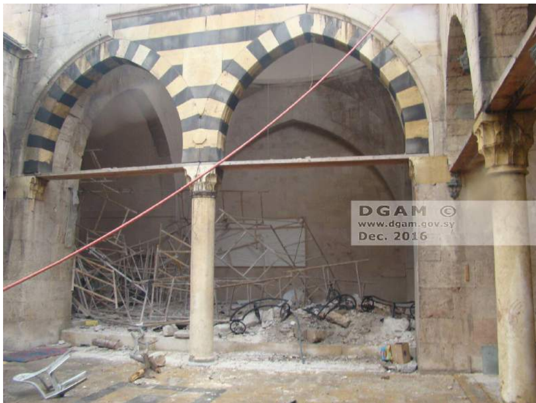
Damage and refuse present at Bimaristan Arghun al-Kamili (DGAM; December 31, 2016)
