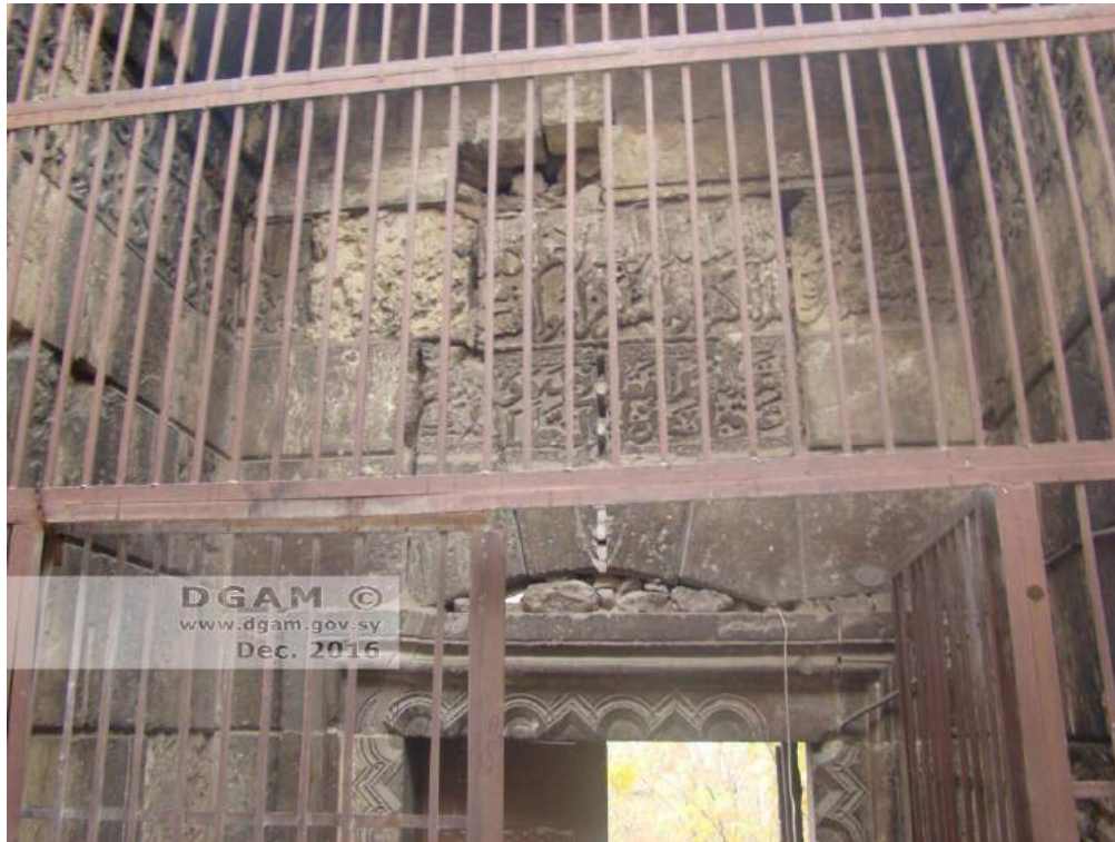
Possible explosives damage to Bimaristan Nur al-Din (DGAM; December 31, 2016)
