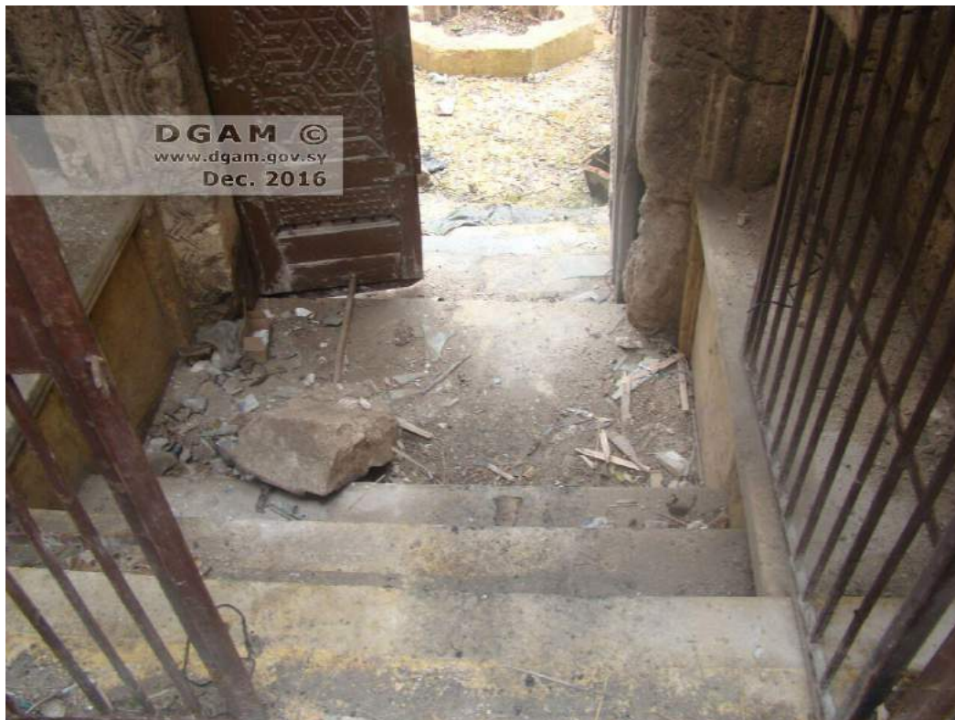
Some debris at Bimaristan Nur al-Din (DGAM; December 31, 2016)
