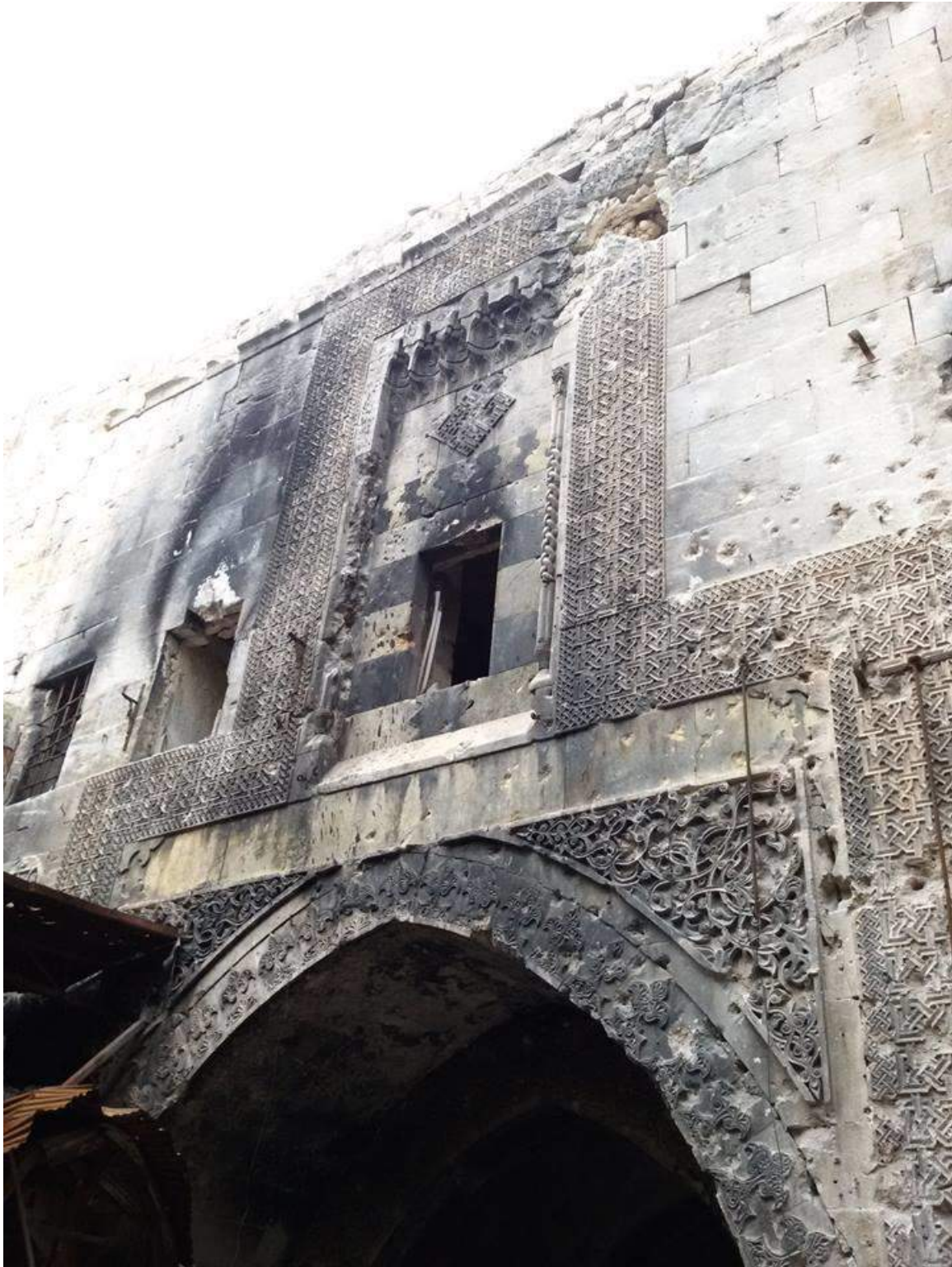
Smoke damage to Khan al-Wazir (Private Facebook Account; December 17, 2016)
