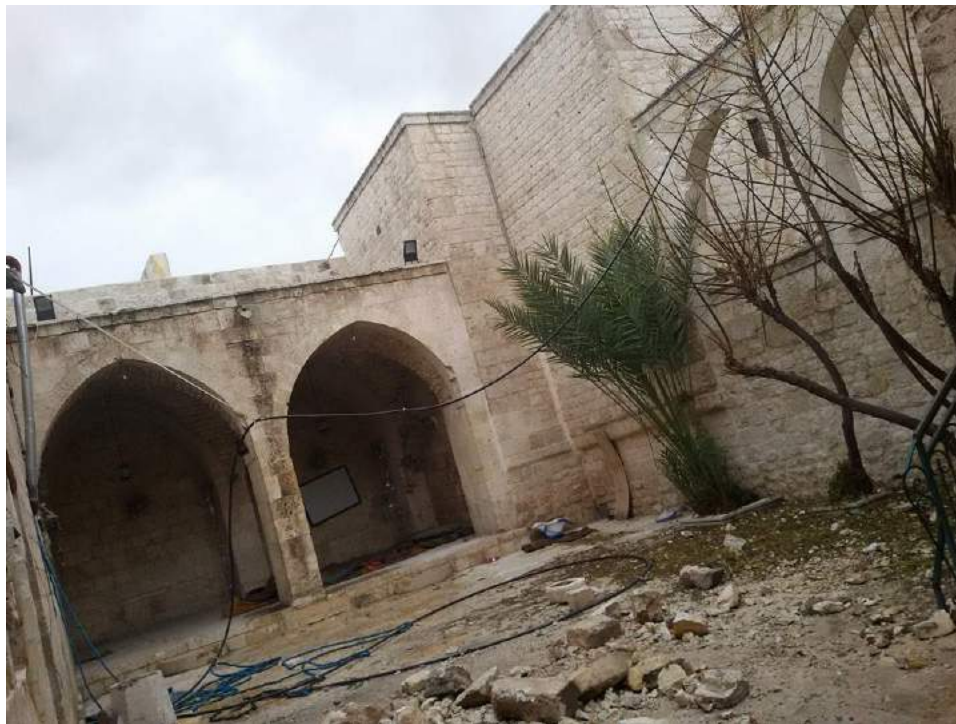
Damage in the courtyard of al-Tarsusi Mosque (Private Facebook Account; December 24, 2016)
