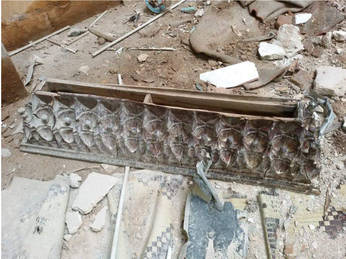
Damage to the interior of Hajj Musa al-Amiri Mosque (Private Facebook Account; December 17, 2016)
