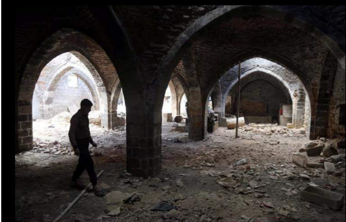
Extensive damage seen at Harasta Olive Oil Mill (Bisan Ilan Kurumu; November 22; 2016)
