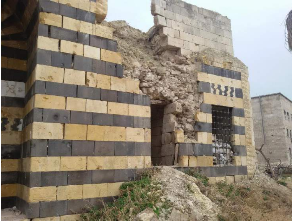
Explosives damage to Hammam Yalbugha al-Nasiri (Private Facebook Account; December 26, 2016)
