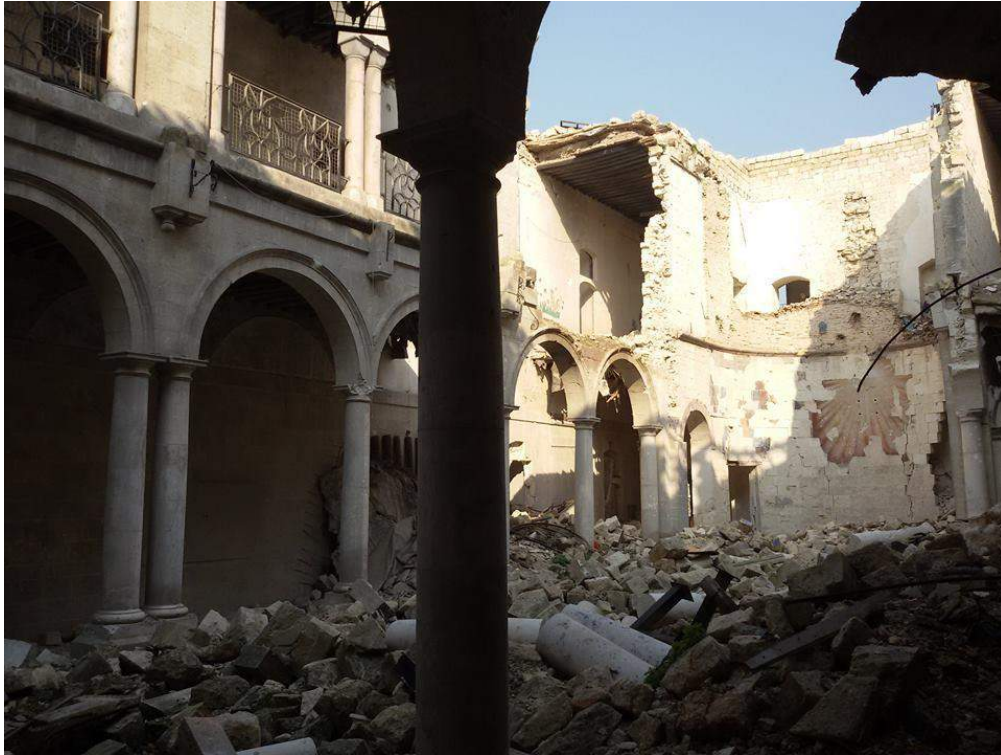
Severe damage to the Yassou'iya (Private Facebook Account; December 19, 2016)
