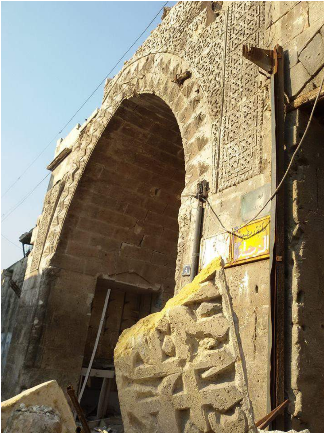
Damage to the Khan Uch Khan (Private Facebook Account; December 19, 2016)
