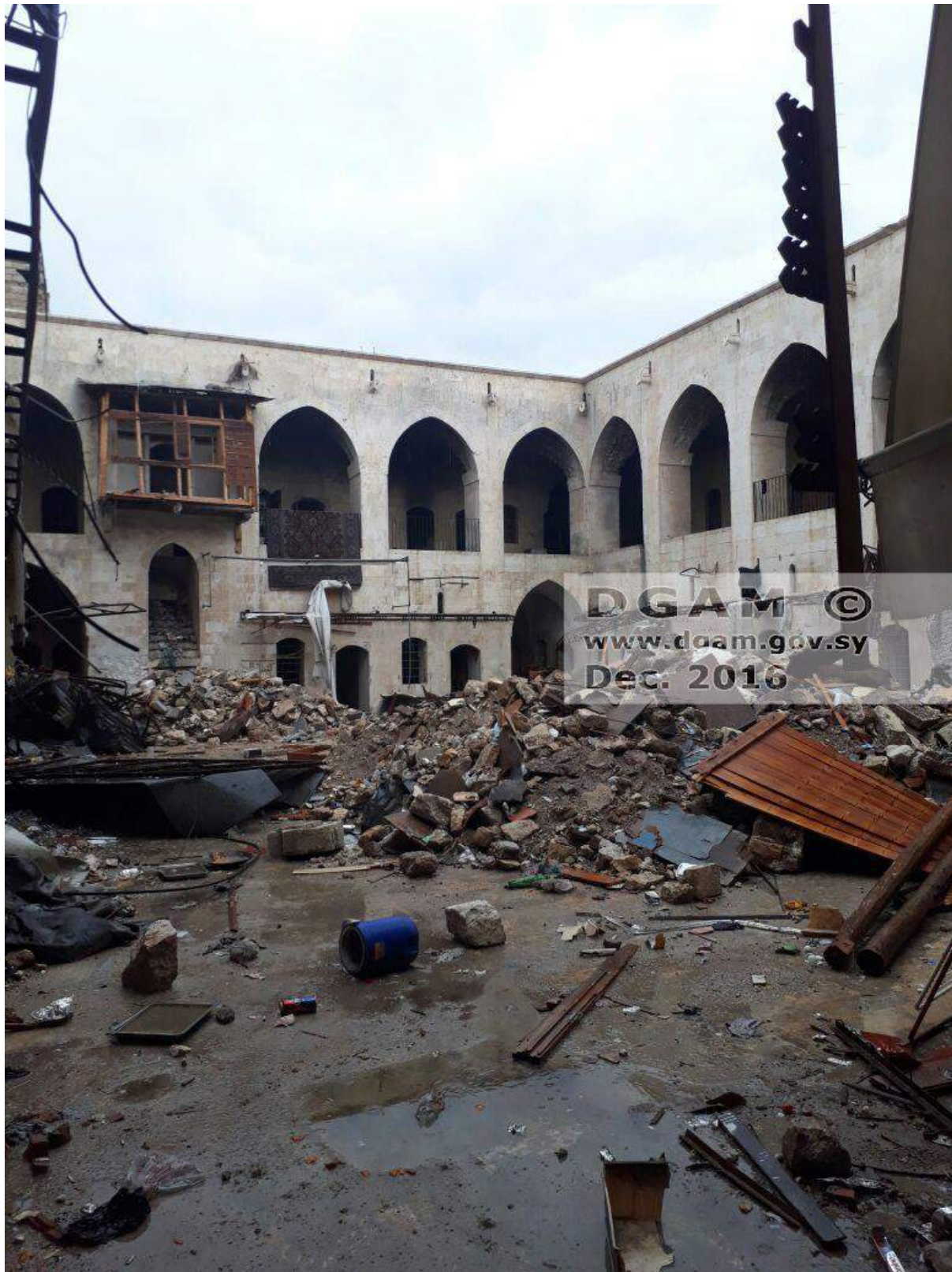
Damage to the Khan Hajj Musa and debris built up in the courtyard (DGAM; December 16, 2016)
