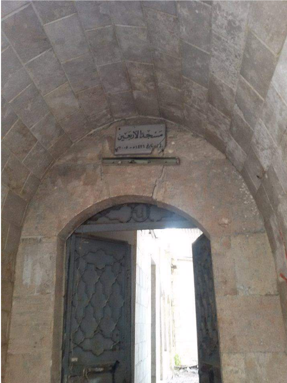
Light damage seen to an entrance to al-Arbaeen Mosque (Private Facebook Account; December 24, 2016)
