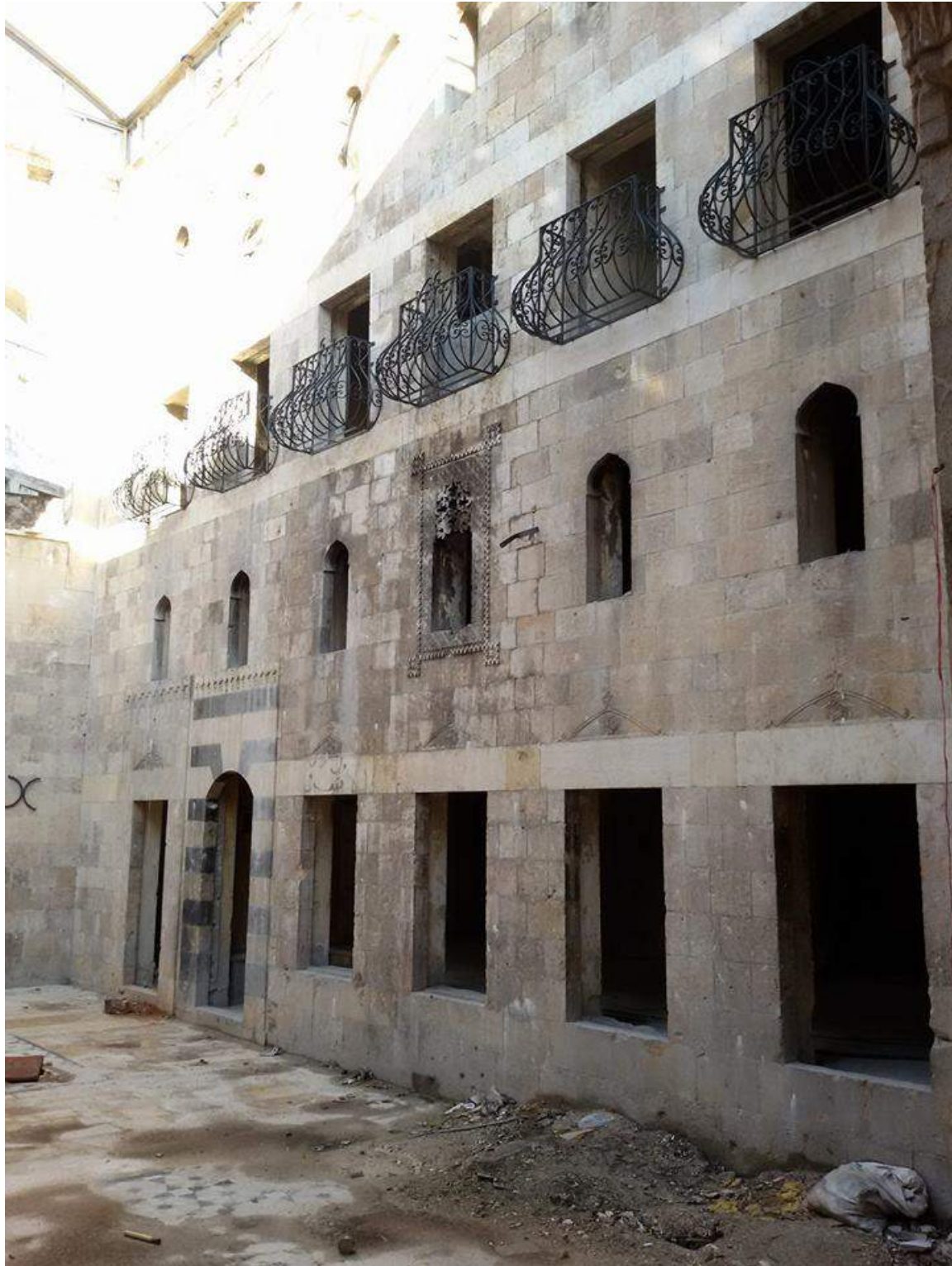
Minimal damage seen in this view of Hotel Zamaria (Private Facebook Account; December 17, 2016)
