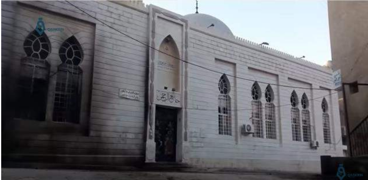
Video still shows what appears to be fire damage to al-Rahman Mosque (Qasioun News Agency; December 22, 2016)
