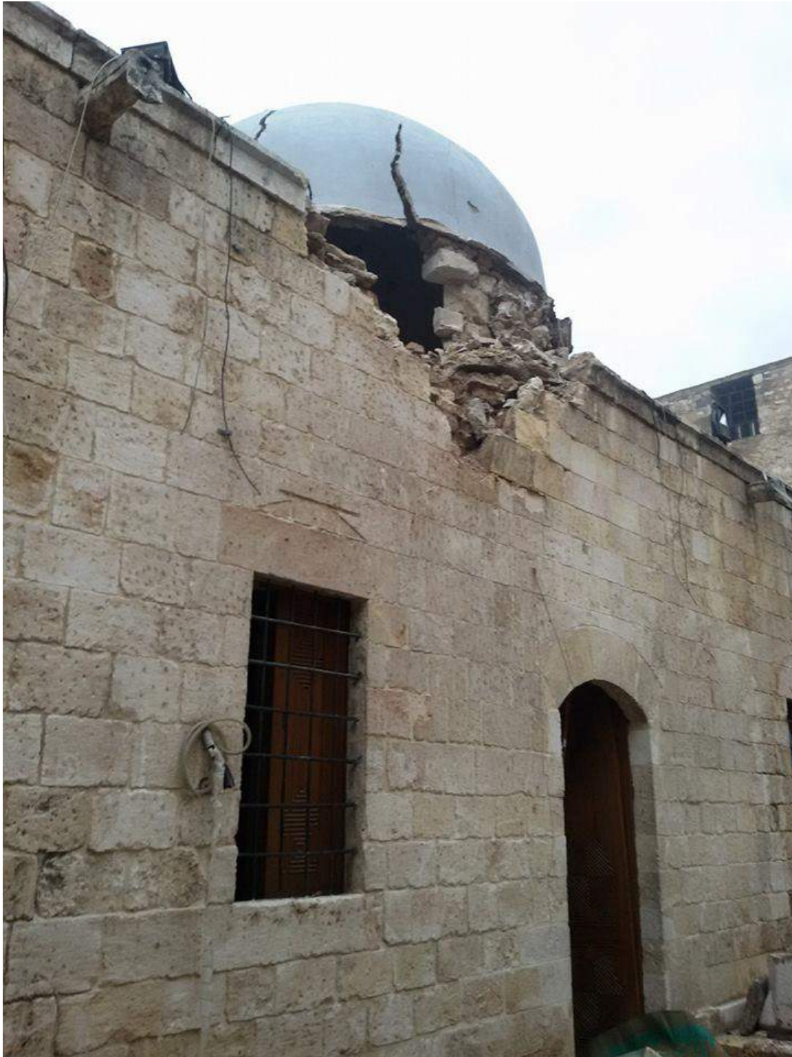
Possible explosives damage to the dome of al-Tarsusi Mosque (Private Facebook Account; December 24, 2016)
