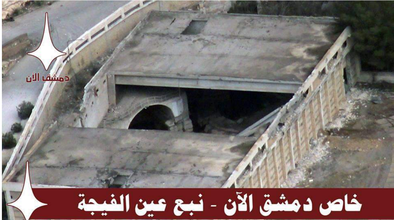
Damage to Ain al-Fijah Spring (Dimashq al-An; December 28, 2016)
