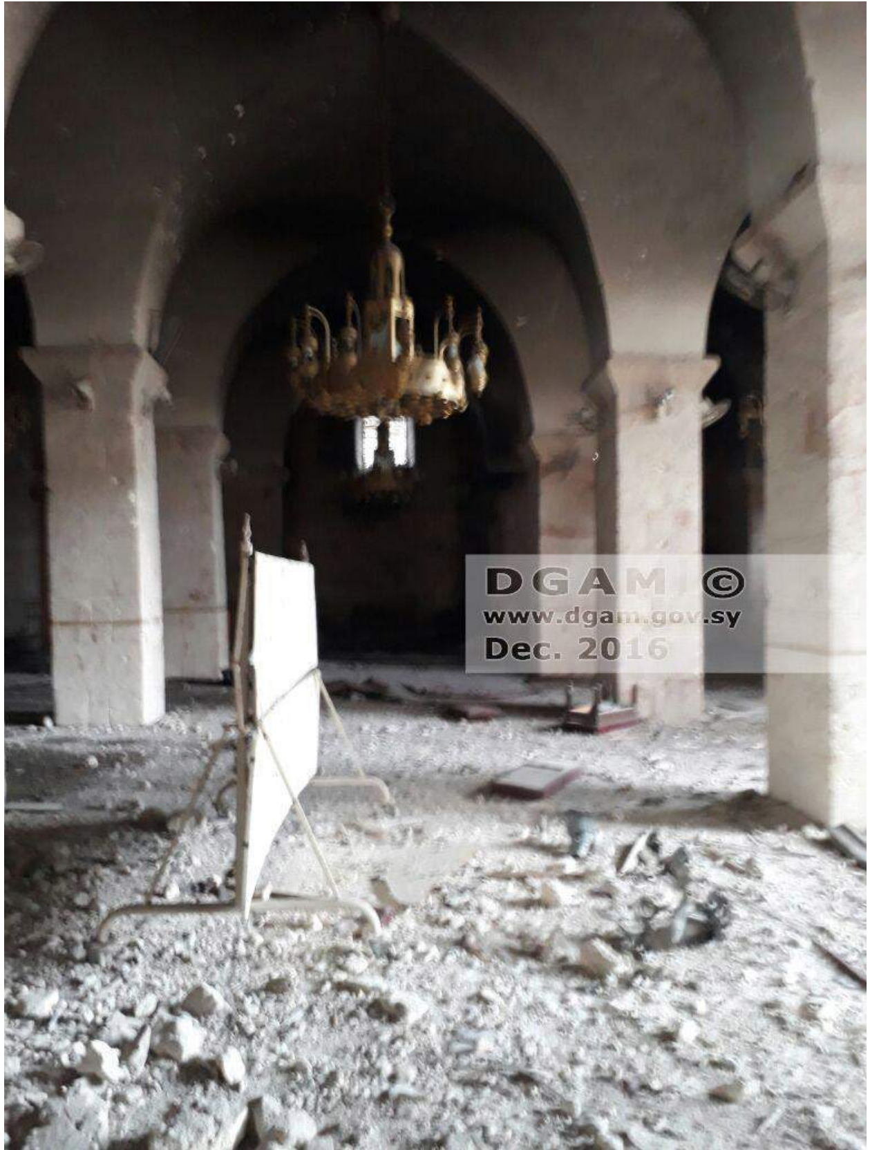
Damage to the interior of al-Kabir Mosque (DGAM; December 16, 2016)
