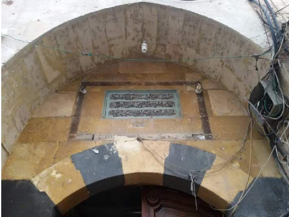
Light damage to al-Karamiya Mosque (Private Facebook Account; December 24, 2016)
