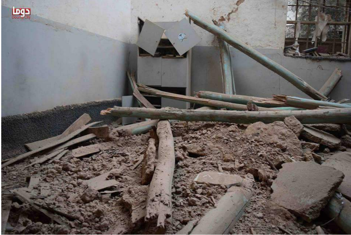
Damage to the interior of Om Habiba Mosque (SNHR; December 29, 2016)
