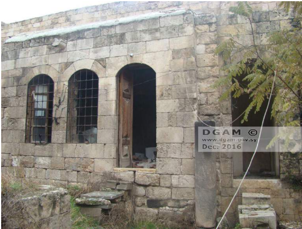
Moderate damage at Bimaristan Nur al-Din (DGAM; December 31, 2016)
