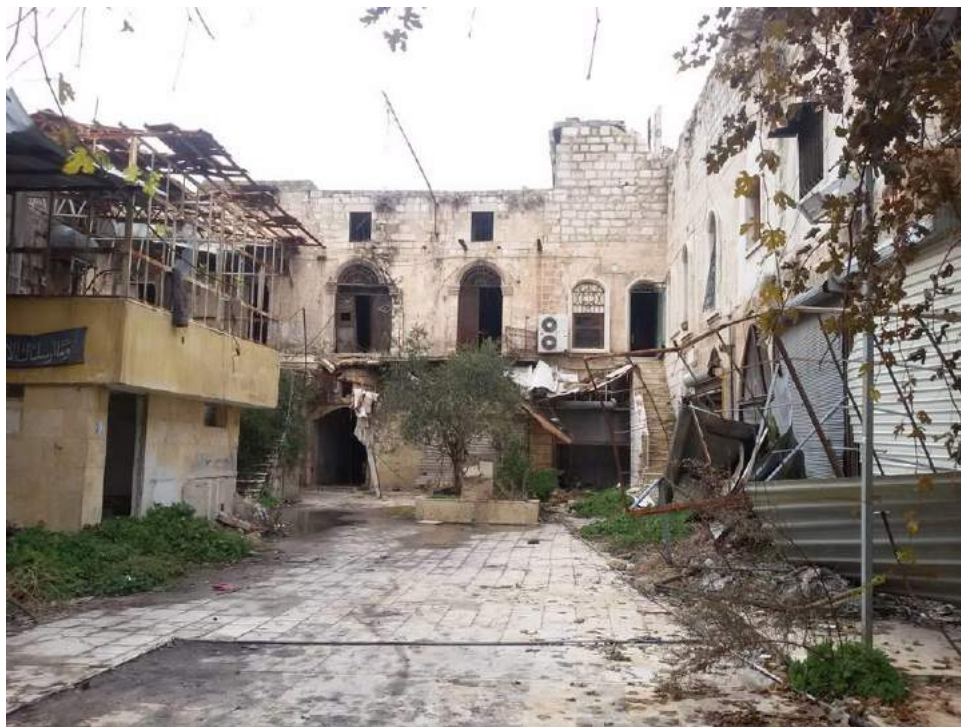
Damage to the shops in Khan al-Qassabiya (Private Facebook Account; December 24, 2016)
